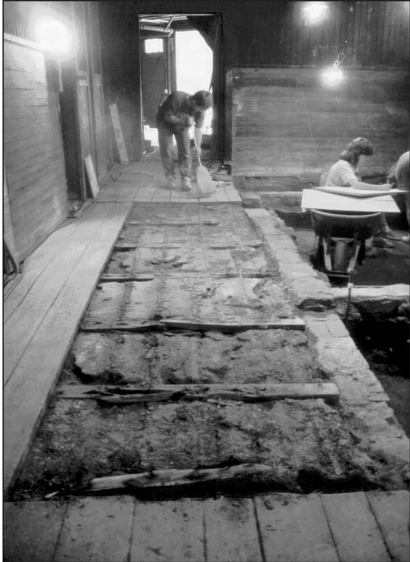
Figure 7. Excavated areas within the North (Stable) Room looking south across the floor openings. Enclosures A-C are to the right.
