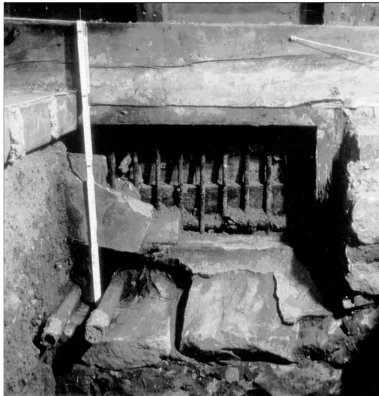
Figure 15. Window in Gas Holder basement's north wall with blockage in place (top) and after blockage was cleared (bottom).
