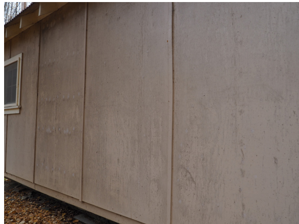
Image 89: Surface wear at exterior plywood.
