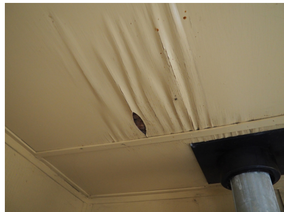
Image 162: Delamination and water damage at plywood ceiling surrounding chimney.
