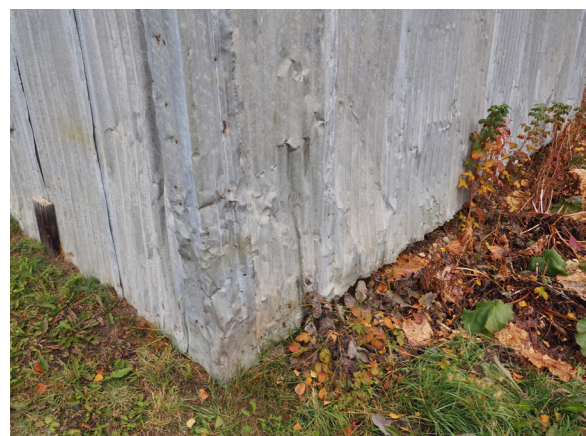
Image 244: Corrugated metal siding is dented throughout.
