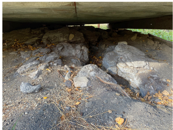
Image 18: Typical permafrost upheaval, located at Bunkhouse 2.
