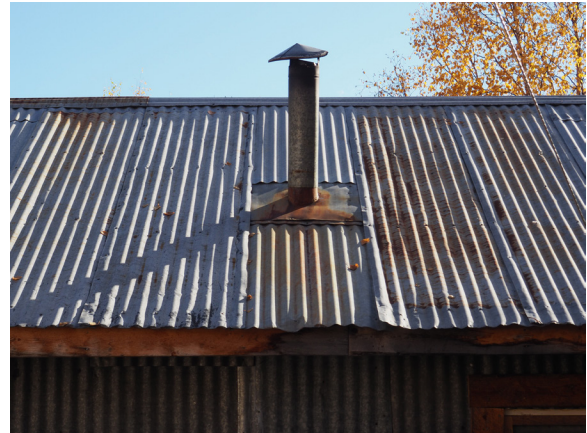
Image 196: Corrugated metal roof with mild corrosion and projecting chimney.
