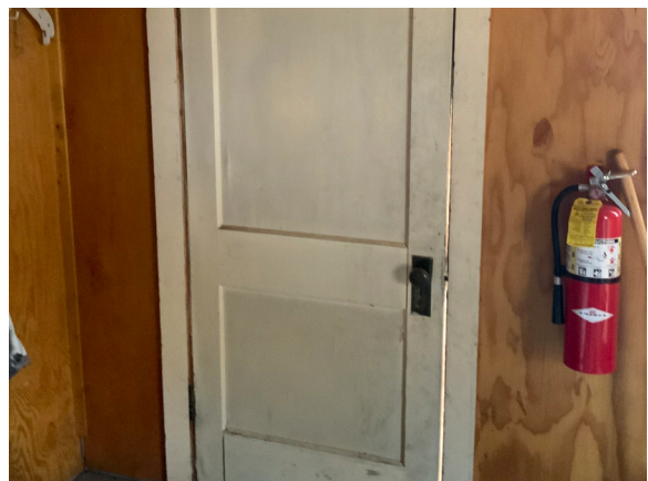
Image 143: Interior view of entry door and fire extinguisher.
