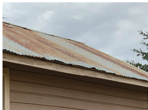
Image 213: Mild to moderate corrosion of corrugated metal roofing.
