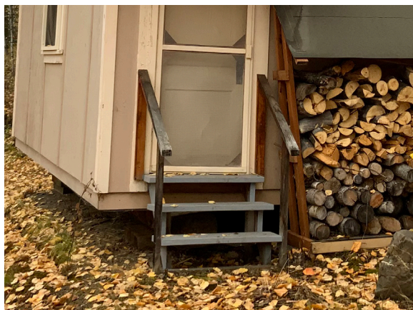
Image 157: Severe rot at west entry handrail.
