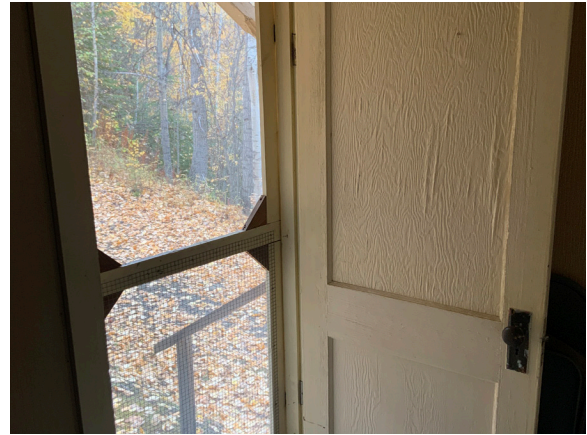
Image 158: East entrance door with exterior delamination at upper panel.
