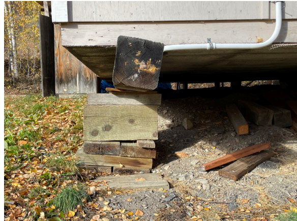
Image 263: Settled timber skid cribbing at Bunkhouse 1.
