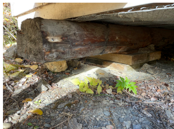
Image 153: Projecting log skids are weathered.
