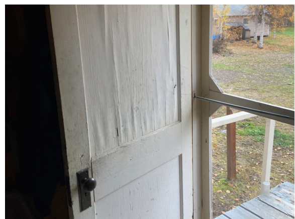
Image 136: Delamination of exterior door upper panel.
