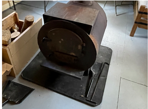
Image 82: Mild corrosion at barrel stove.
