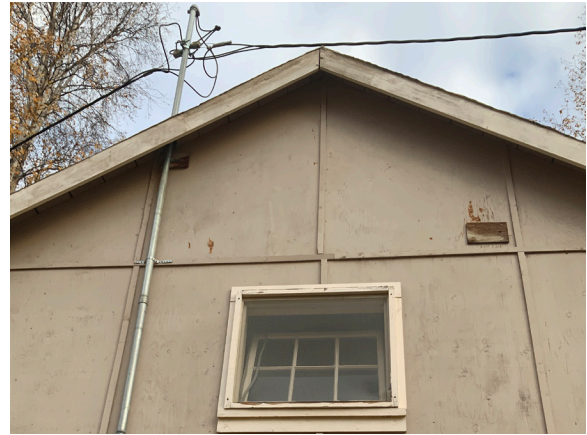
Image 30: South elevation plywood exterior sheathing with surface wear and patched penetrations.
