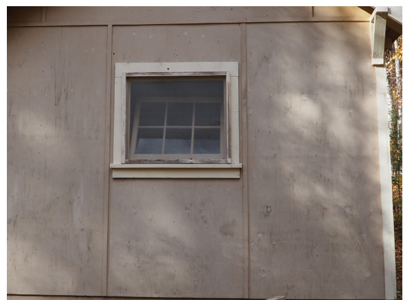
Image 109: Surface wear at exterior plywood sheathing, south elevation.
