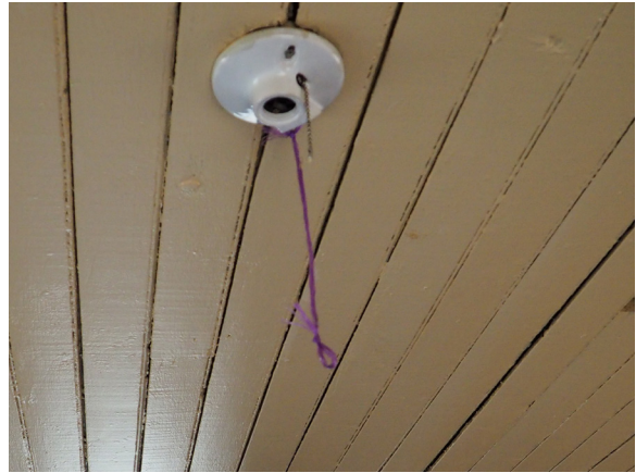
Image 63: Porcelain socket missing light bulb.
