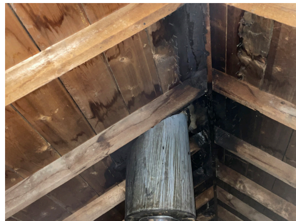
Image 105: Fire damage surrounding chimney in attic.
