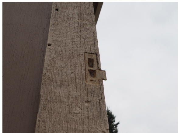
Image 234: Remnants of door hardware at exterior corner board trim, evidence that wood trim was salvaged from another building.
