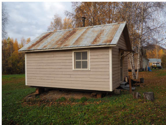
Image 48: Moderate corrosion of corrugated metal roofing at east elevation.
