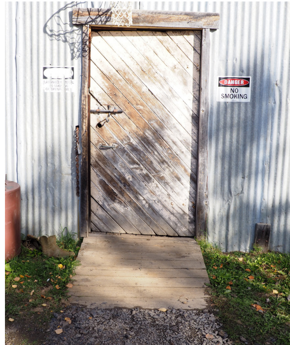
Image 248: West entry with surface deterioration at exterior.
