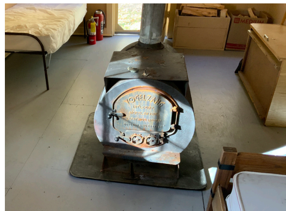
Image 100: Mild corrosion at barrel stove.
