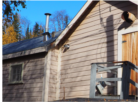
Image 170: Wood rot at intersecting roofs at the west elevation.
