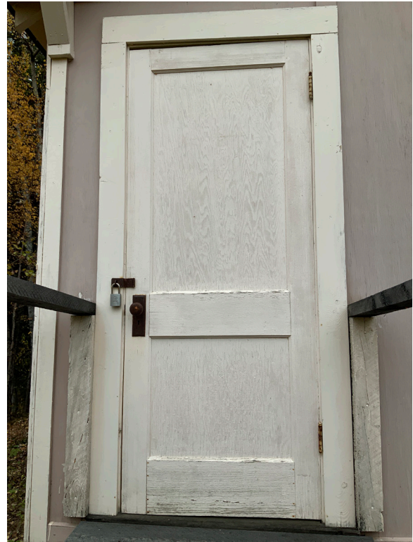
Image 239: Surface weathering at entry door.
