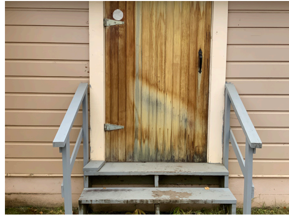
Image 179: Surface wear at door D1.
