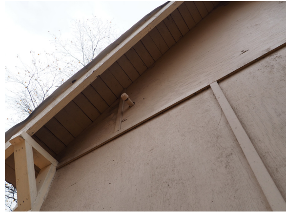
Image 91: Abandoned fuel line at south elevation.
