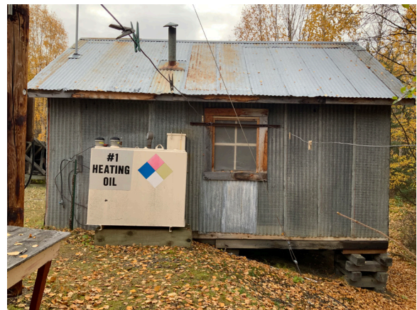
Image 21: Oil tank located at the north elevation of the Laundry Building.
