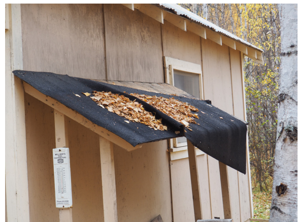
Image 118: Detail of failing rolled asphalt roof covering at wood shed.
