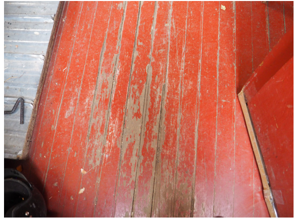
Image 187: Surface wear at wood floor near main entrance in mess hall.
