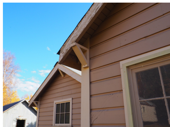
Image 169: Paint weathering at north elevation bargeboards.
