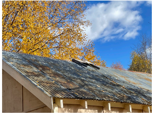
Image 27: Mild corrosion at corrugated metal roofing.
