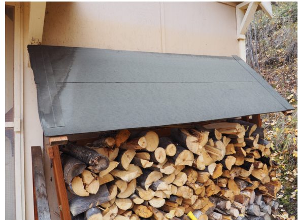
Image 159: Wood shed roof with biogrowth.
