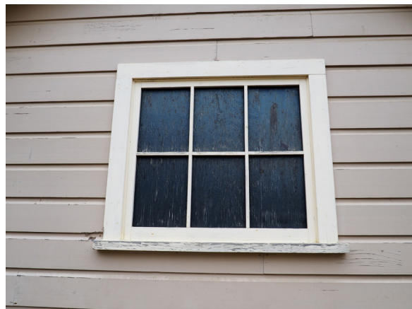
Image 177: Pantry window N1 infilled with plywood for security.
