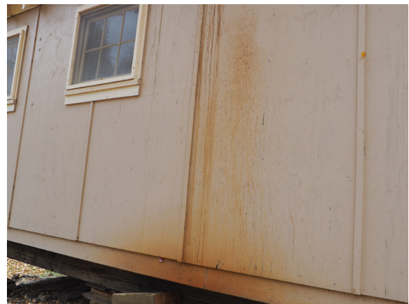
Image 31: Rust staining at the east elevation below chimney location.
