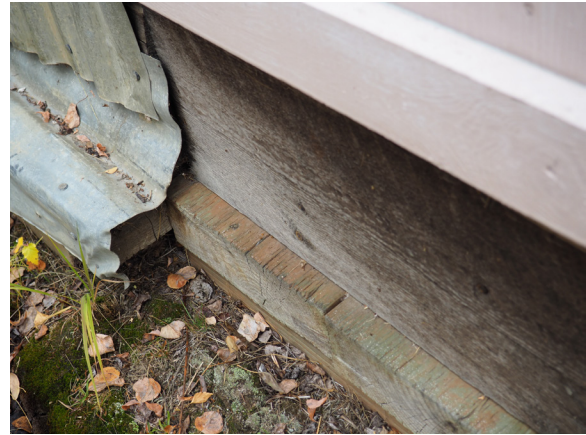
Image 236: Wood sills are flashed in corrugated metal at the north addition.
