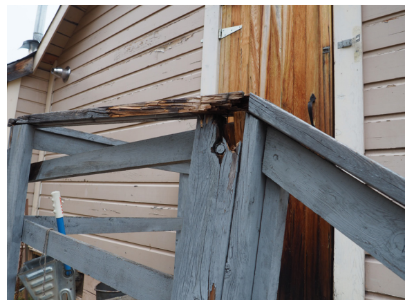
Image 181: Severe wood rot at west elevation handrail.
