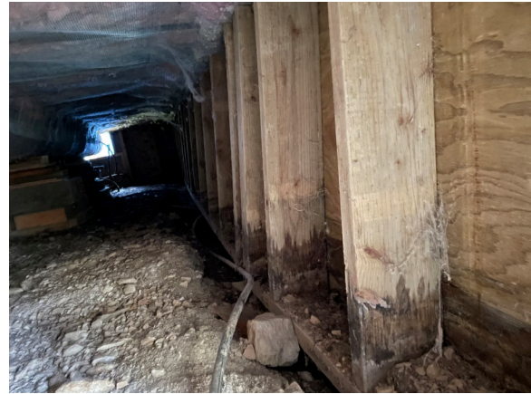
Image 260: Decayed perimeter skirting supported directly on soil.
