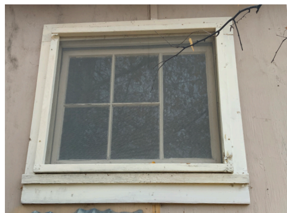
Image 35: Typical 6-lite hopper window. Window W1 is missing a muntin.
