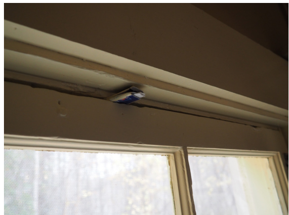
Image 114: Paper shim used to hold window closed.
