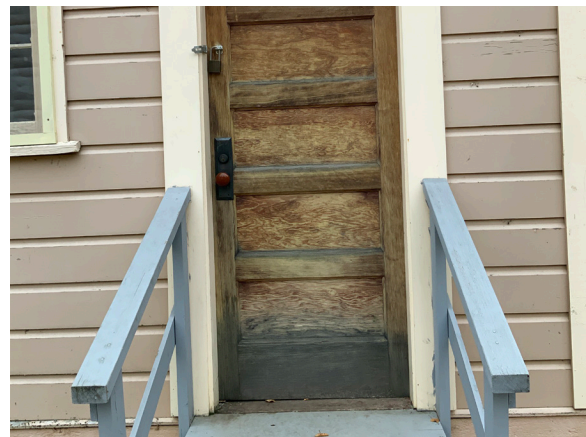
Image 180: Surface wear at door D4
