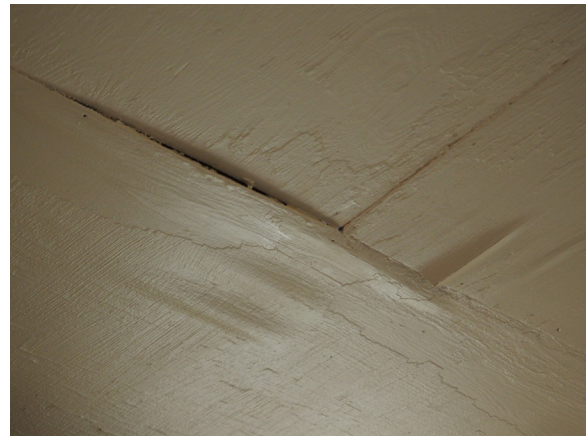
Image 42: Detail of water damage at plywood ceiling.
