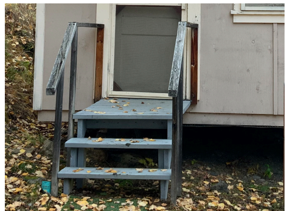
Image 160: Severe rot at east entry handrail.
