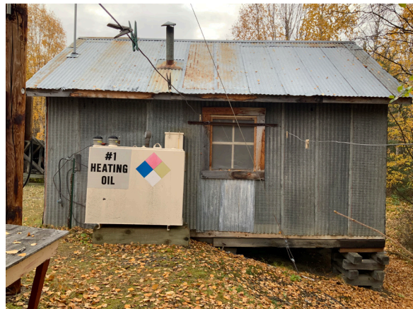
Image 267: Fuel oil tank at Laundry building.
