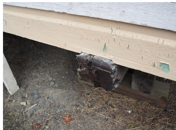
Image 216: Projecting log skids are weathered.
