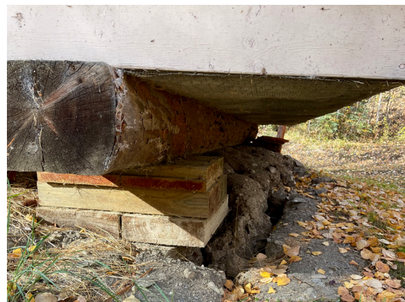
Image 74: Permafrost melting with upheaval.
