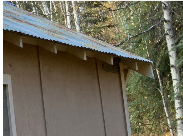
Image 110: Frieze board patched at east elevation.
