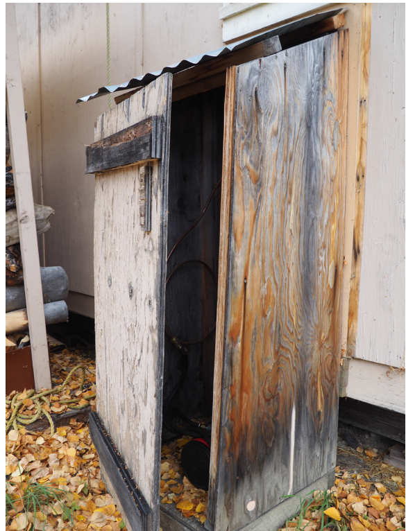
Image 40: Severe plywood deterioration at the propane shed, west elevation.
