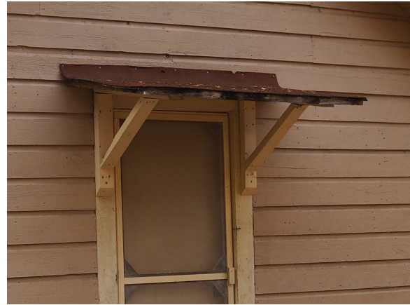
Image 51: North entrance awning with eave trim rot.
