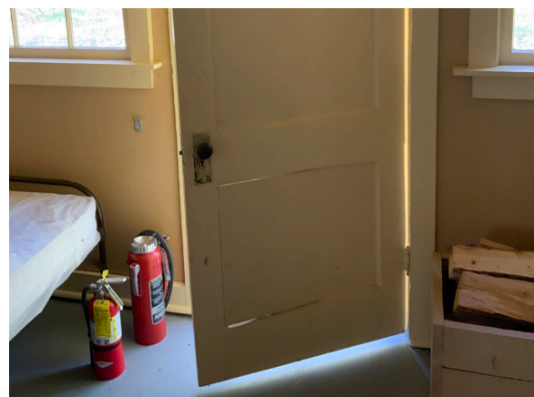
Image 96: Natural light is visible through lowermost panel of exterior door.
