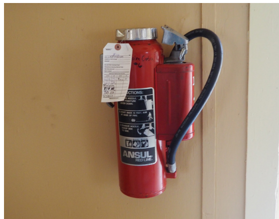
Image 83: Fire extinguisher mounted at north wall.
