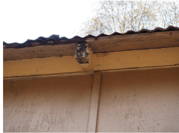
Image 69: Rotting rafter tail at east elevation.
