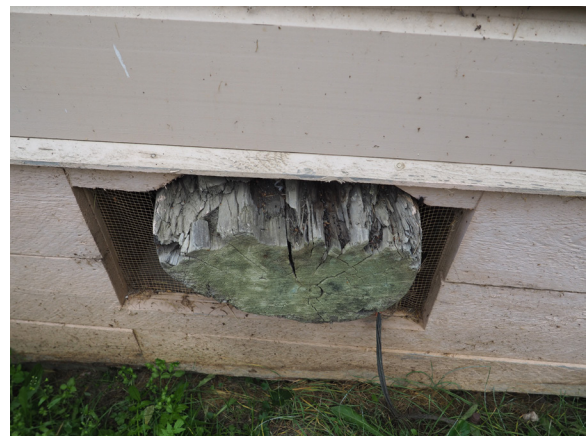
Image 175: Active wood rot at projecting log skid at east elevation.
