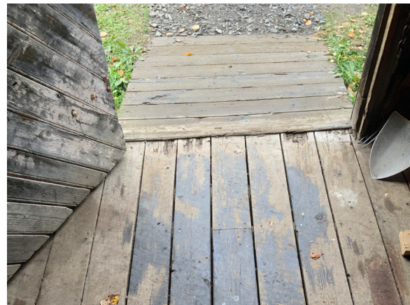
Image 251: Wood floor has surface wear and staining.
