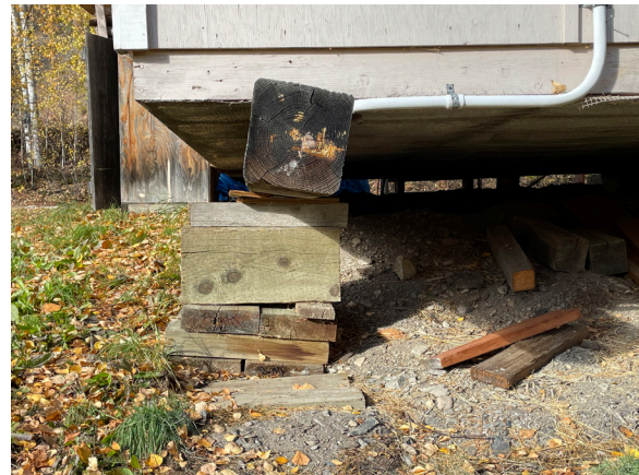
Image 33: Replacement skid is warped and unstable.
