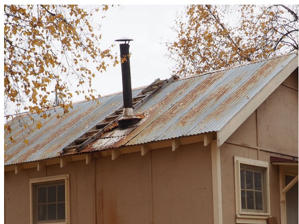
Image 29: Chimney is not braced and is leaning.
