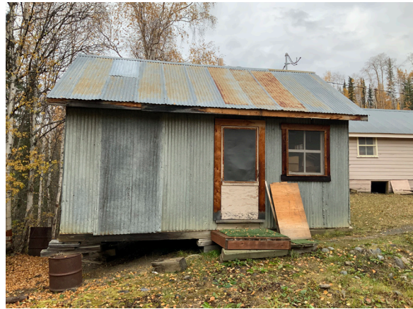
Image 266: Unstable cribbing at Laundry building.
