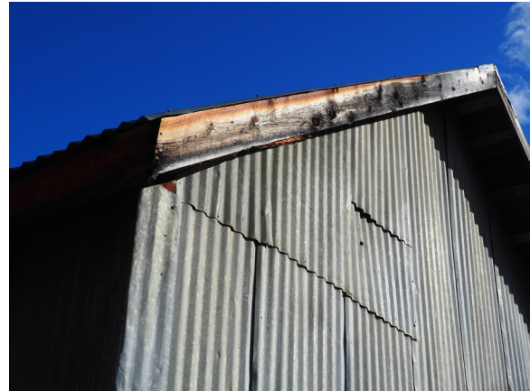
Image 242: Natural finish bargeboards with surface weathering.
