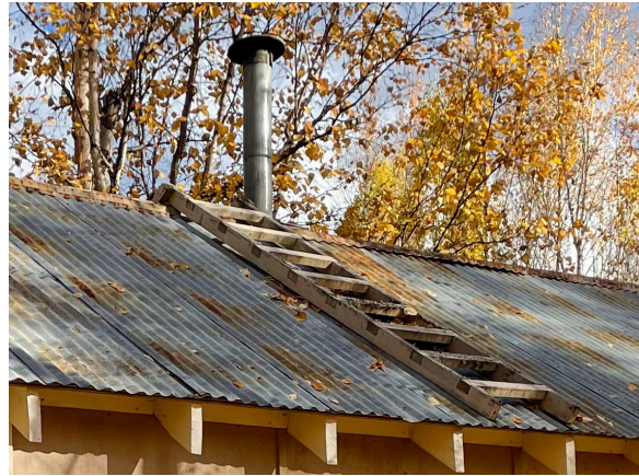
Image 88: Deteriorating roof access ladder.
