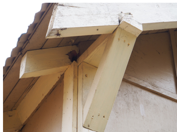
Image 106: Cracked bargeboard at north elevation.
