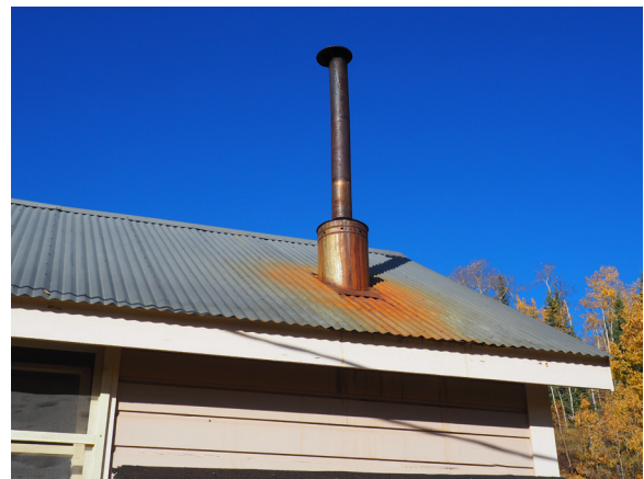
Image 171: Moderate corrosion surrounding Mess Hall chimney projection. Chimney is not braced.
