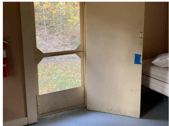
Image 58: Entry door with missing handleset.
