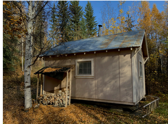
Image 104: Mild corrosion at east elevation corrugated metal roofing.
