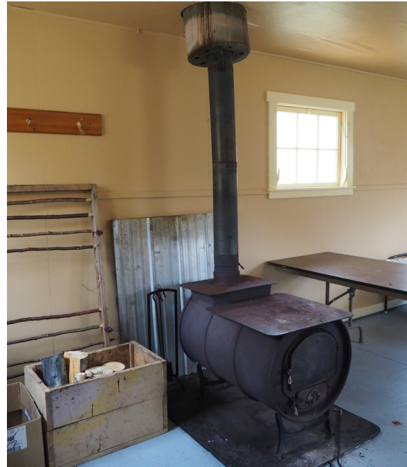
Image 44: Wood barrel stove with surface corrosion and inadequate heat shielding at adjacent wall.
