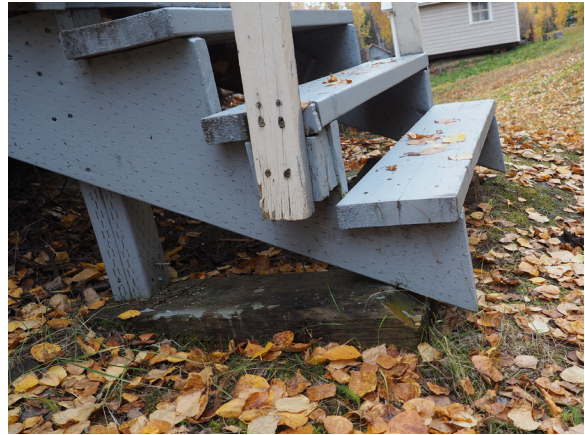
Image 78: Stringer rests on deteriorated wood sill.
