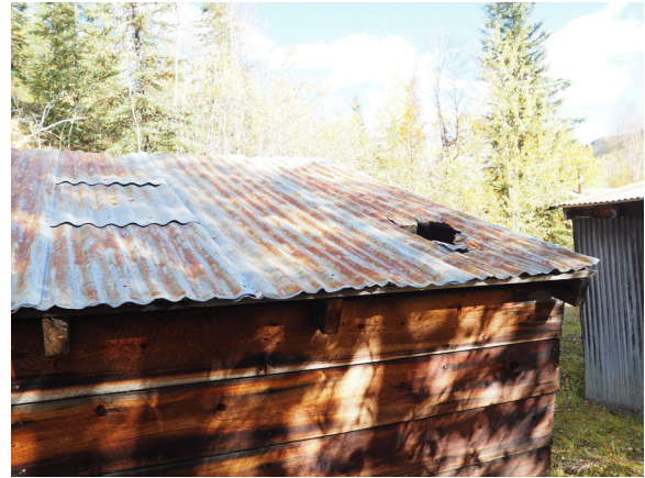
Image 254: Moderate corrosion and abandoned chimney hole at roof.
