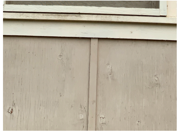
Image 131: Detail of typical paint weather at exterior plywood and trim.
