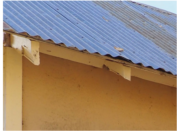
Image 128: Fractured rafter tail at east elevation.
