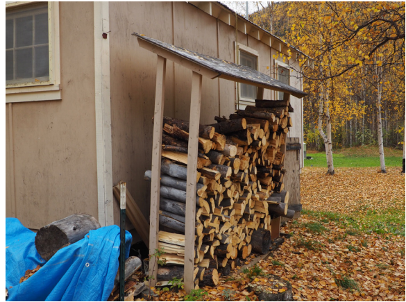
Image 39: Wood shed at west elevation is leaning away from building and unstable.
