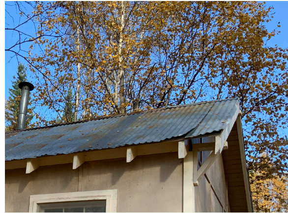
Image 85: Bent and uplifting corrugated metal roofing.
