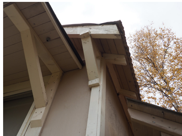
Image 126: Exposed tongue and groove sheathing at underside of primary roof and awning roof.
