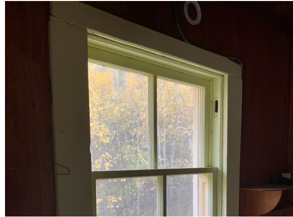
Image 220: Detail of missing double hung sash ropes.
