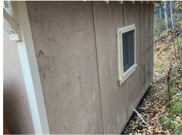
Image 151: Mildew discoloration at north elevation plywood sheathing.
