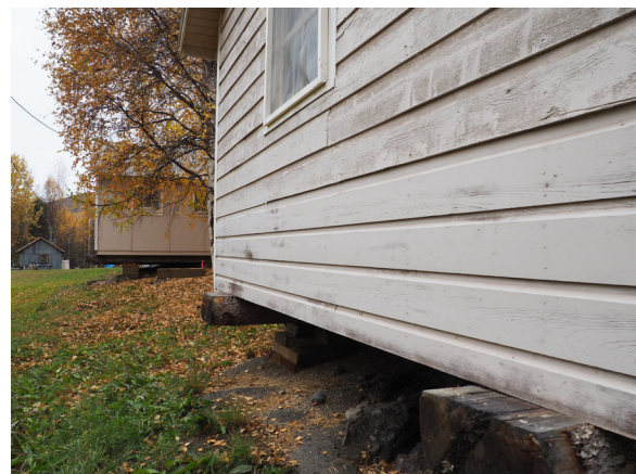
Image 53: Paint weathering at exterior drop siding. Lowermost boards have been replaced with new siding.
