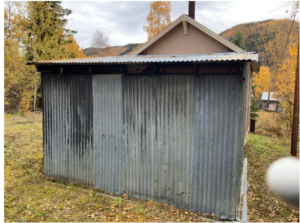
Image 233: Corrugated metal siding is dented throughout.
