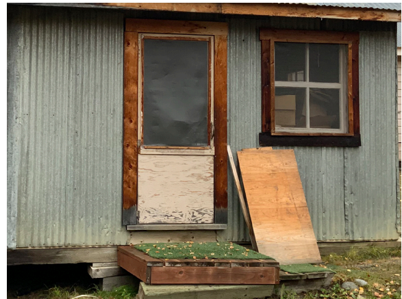
Image 203: South entry screen door, severely weathered.
