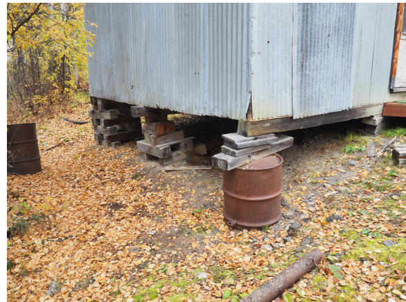
Image 199: Severe erosion at the west end of the building, with various cribbing and barrels used to support the building.
