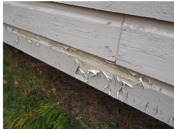
Image 215: Typical paint failure at exterior drop siding.
