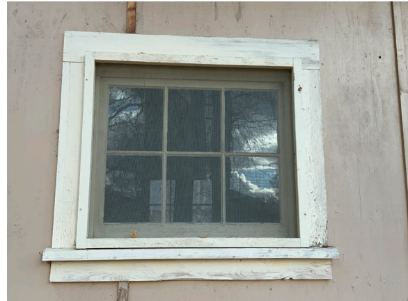
Image 75: Hopper window with paint deterioration at exterior.
