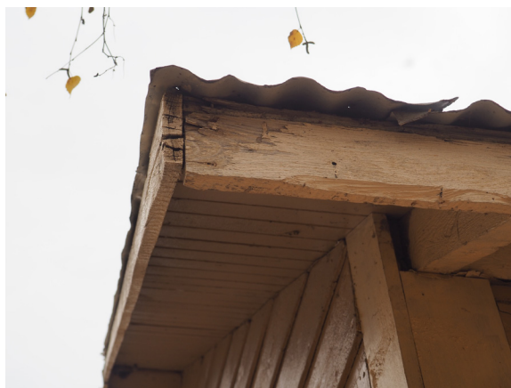
Image 49: Rot and cracking at east fascia board.
