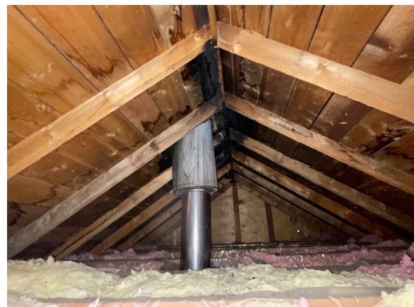
Image 121: Fire damage at roof framing surrounding chimney.
