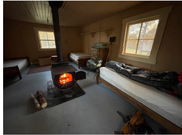
Image 226: Wood stove with corrugated metal heat shield.
