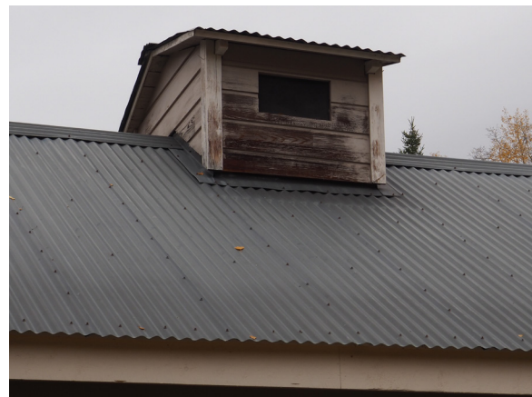
Image 168: Paint weathering at roof cupola.
