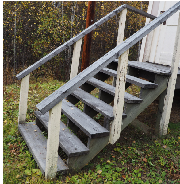
Image 240: Severe wood rot at entry stair.
