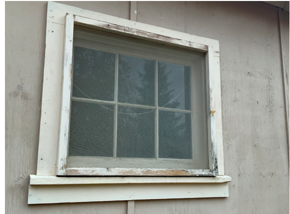
Image 134: Hopper window with exterior screen and paint weathering.
