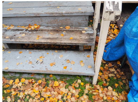
Image 37: North elevation entry stair with moderate rot at stair treads.
