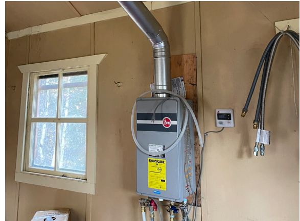
Image 208: Wall mounted on-demand hot water heater, not in use.
