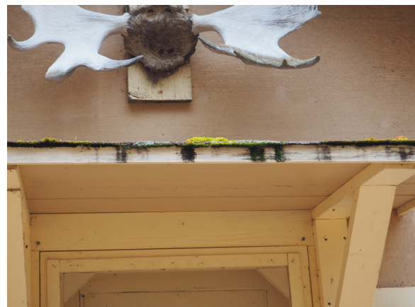
Image 87: Active biogrowth at north entry awning and associated trim rot.
