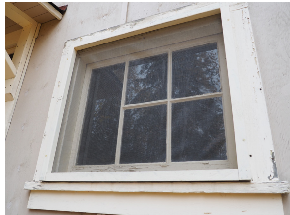
Image 154: Typical hopper window with exterior screen. Window W1 is missing a muntin.
