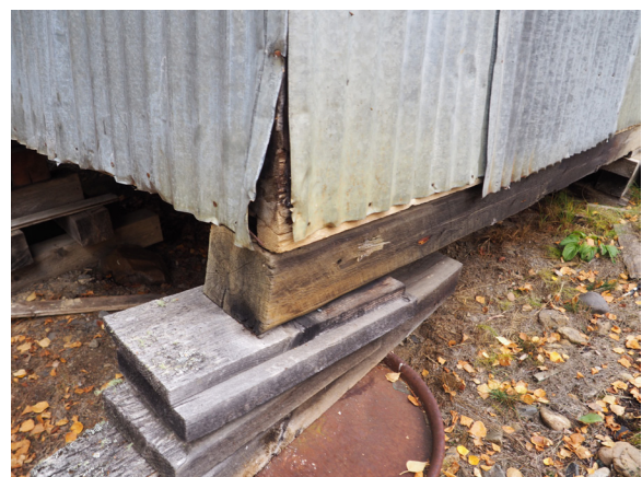
Image 198: Bent corrugated metal siding at southwest corner revealing wood framing.
