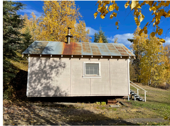
Image 125: Moderate corrosion at corrugated metal roofing surrounding chimney.
