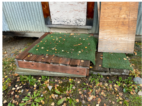
Image 204: South entry landing is unstable with wood rot.
