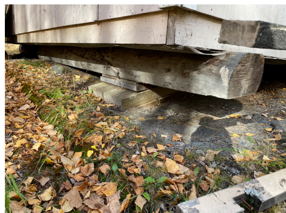
Image 112: Melting permafrost with cribbing supporting log skids.
