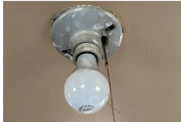
Image 45: Typical porcelain socket, one of two at ceiling.
