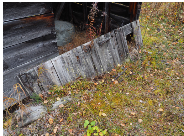
Image 256: One panel of the original double door is rotting on the ground.
