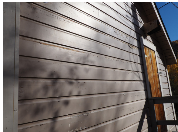
Image 172: Detail of exterior drop siding and paint weathering.
