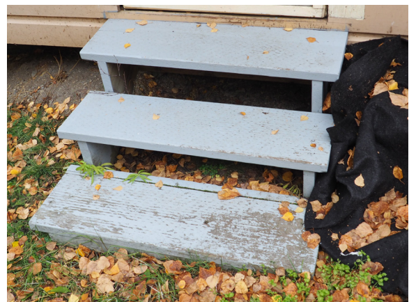
Image 59: Entry stair settling into grade.
