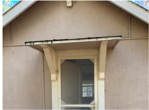
Image 107: North entry awning with active biogrowth and rot.
