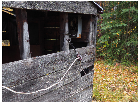
Image 255: Typical exterior siding with severe wood rot and active biogrowth. Siding is missing throughout.
