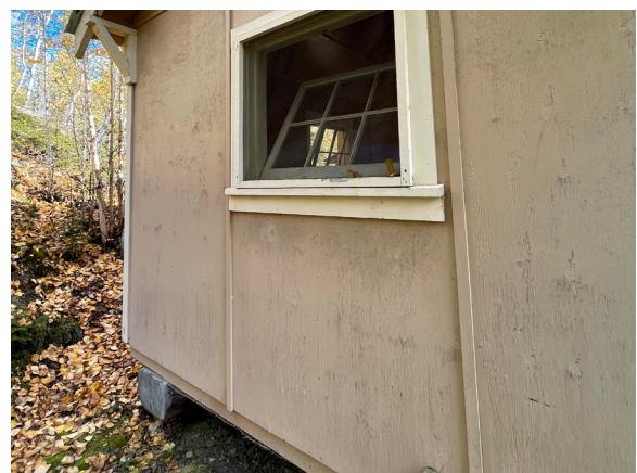
Image 130: Surface weathering at exterior plywood, north elevation.
