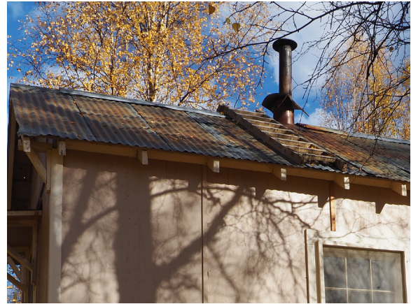
Image 66: Mild corrosion, access ladder, and chimney projecting through ridge.
