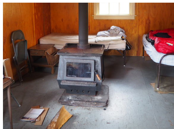
Image 140: Wood stove with inadequate heat shield at floor.
