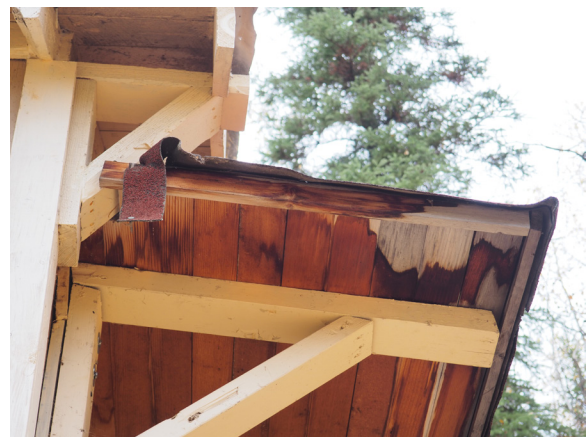
Image 147: Active rot at east elevation entry awning.
