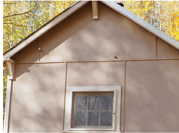
Image 72: Surface damage at the south elevation gable.
