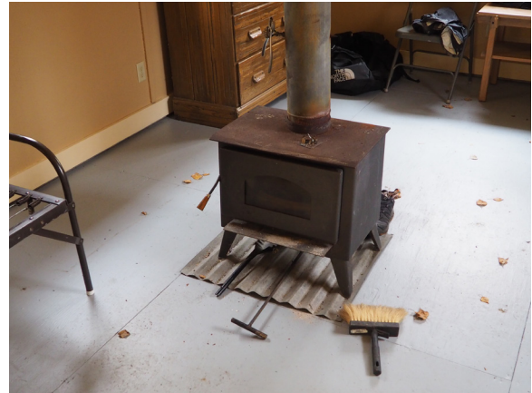
Image 122: Wood stove with inadequate heat shield at floor.
