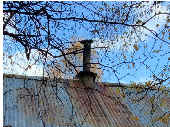
Image 52: Chimney projecting from the ridge with chimney cap, storm collar, and severe corrosion.
