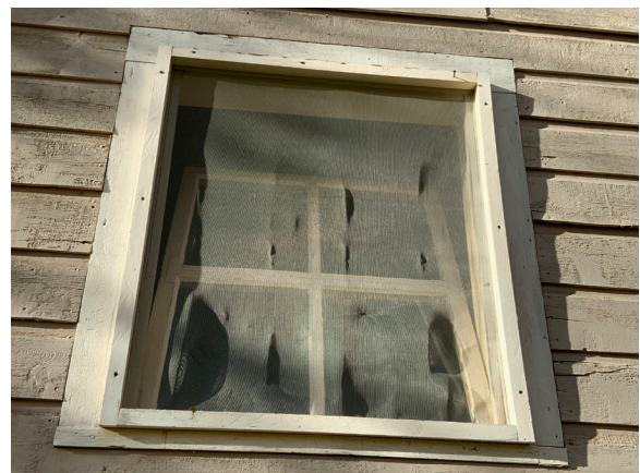
Image 56: Typical warped and torn window screen.
