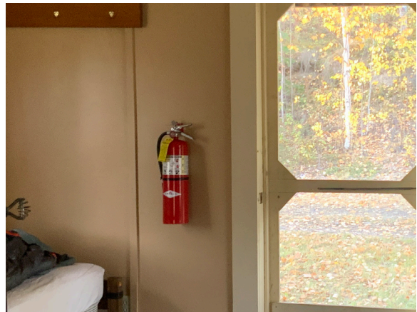
Image 64: Fire extinguisher mounted at north wall.
