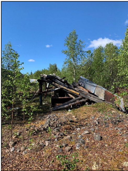
Historic cache collapsed (NPS 2020).
