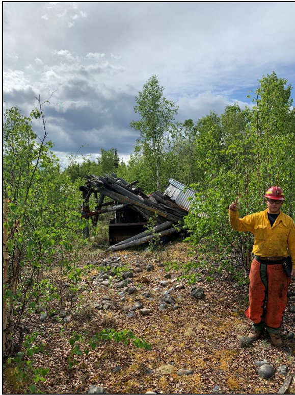
The cache has collapsed on the bulldozer (NPS 2020).
