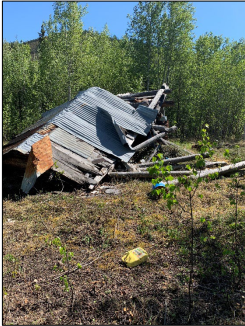
Collapsed cache (NPS 2020).
