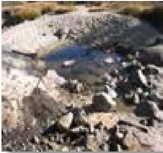
Fig. 1-18. Ponding at culvert below Budd Creek
