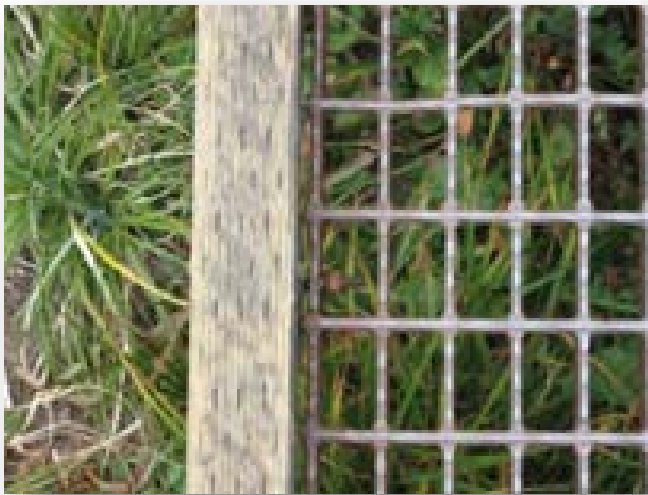
Figure 3- 5: plants growing beneath grate
