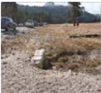
Fig. 1-17. Culvert set too low in meadow
