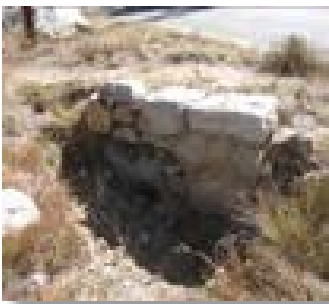
Fig. 1-16. Partially blocked culvert
