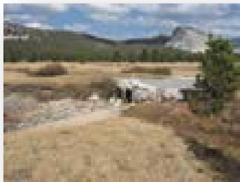
Fig. 1-26. Scour downstream of culvert on Unicorn Creek
