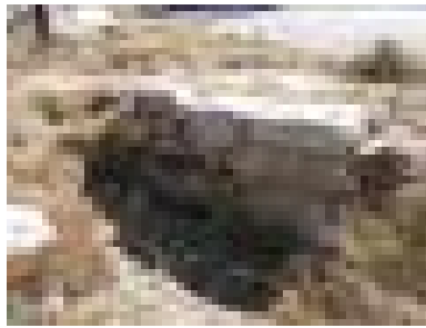
Partially blocked culvert.
