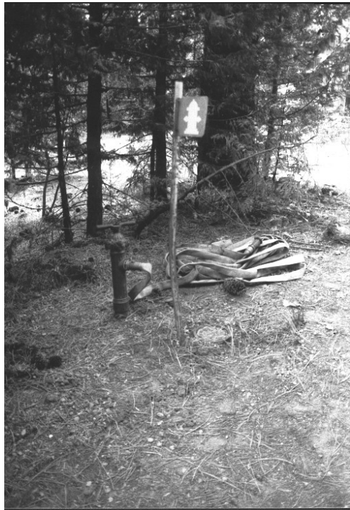
Fire hydrant and hose in the vicinity of the rangers' dormitory. HRA, 1999.
