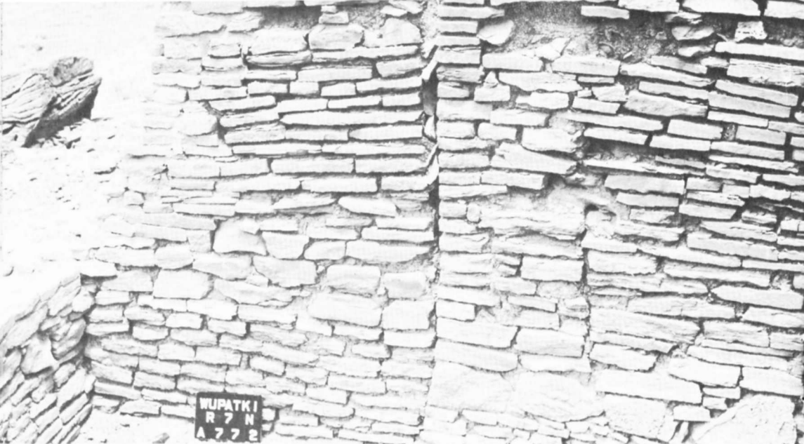
Break in wall due to lack of bonding
