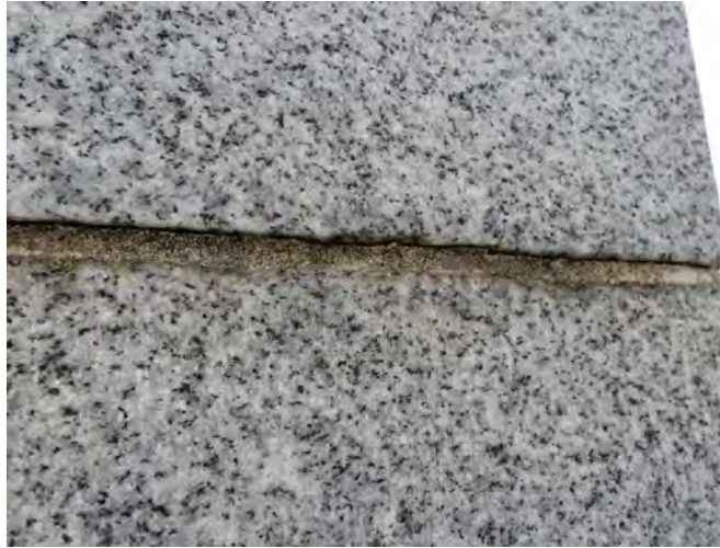
Figure 29. Example of delaminated mortar joint; delaminations permit moisture ingress during rainstorms.
