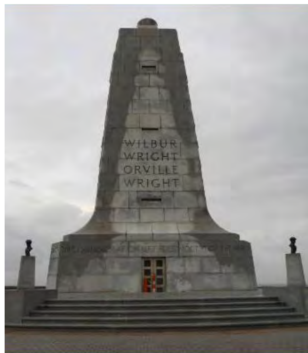
FIGURE 2–42. View of moisture at the exterior of the Monument during the moisture intrusion investigation, 2017. (Evaluation and Testing Report Wright Brothers National Memorial Monument prepared for Amidon, Inc.)
