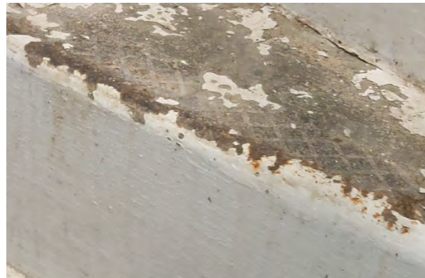
FIGURE 3-51. Surface wear and rust at risers, typical.
