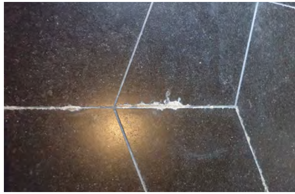
FIGURE 3-42. Typical joint conditions at Memorial Room floor.
