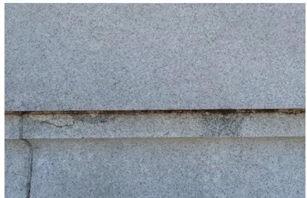
FIGURE 3–32. Typical condition of spalls at underneath of terrace cap.
