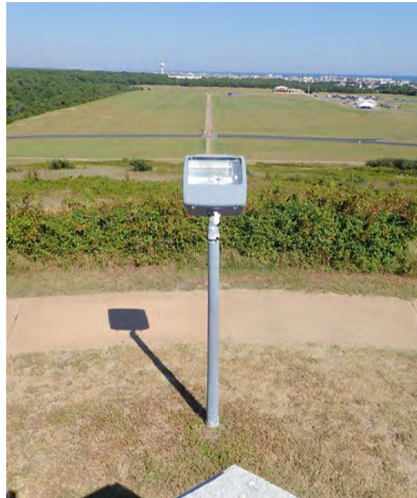
FIGURE 3-8. Site lighting fixture, facing north.
