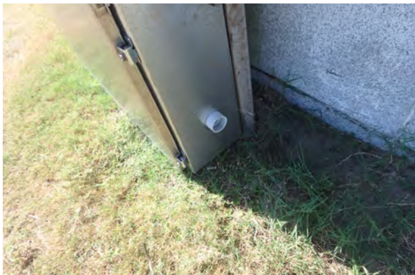
FIGURE 3–61. Opening in Main Service Enclosure.
