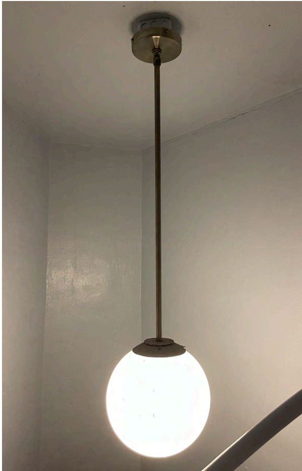
FIGURE 3-49. Typical Art Deco inspired light fixture in both Level B and Level C.
