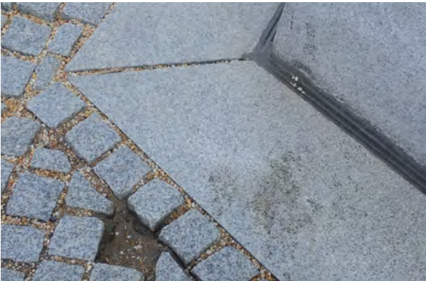
FIGURE 3–34. Missing terrace granite paver and broken sealant joint at base of the Monument.
