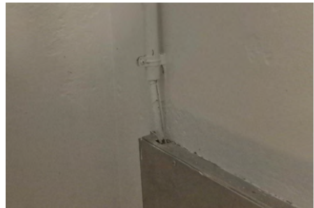
FIGURE 3-69. Lightning grounding conductor.
