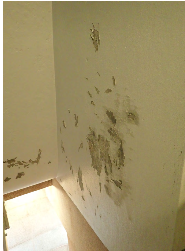
FIGURE 3-50. Paint peeling and popping off at stairwell, below access hatch.
