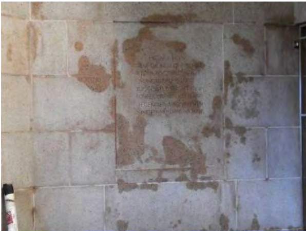
FIGURE 5-5. Moisture staining on the ground level walls (Atkinson-Noland & Associates, Inc. et al, 2017).
