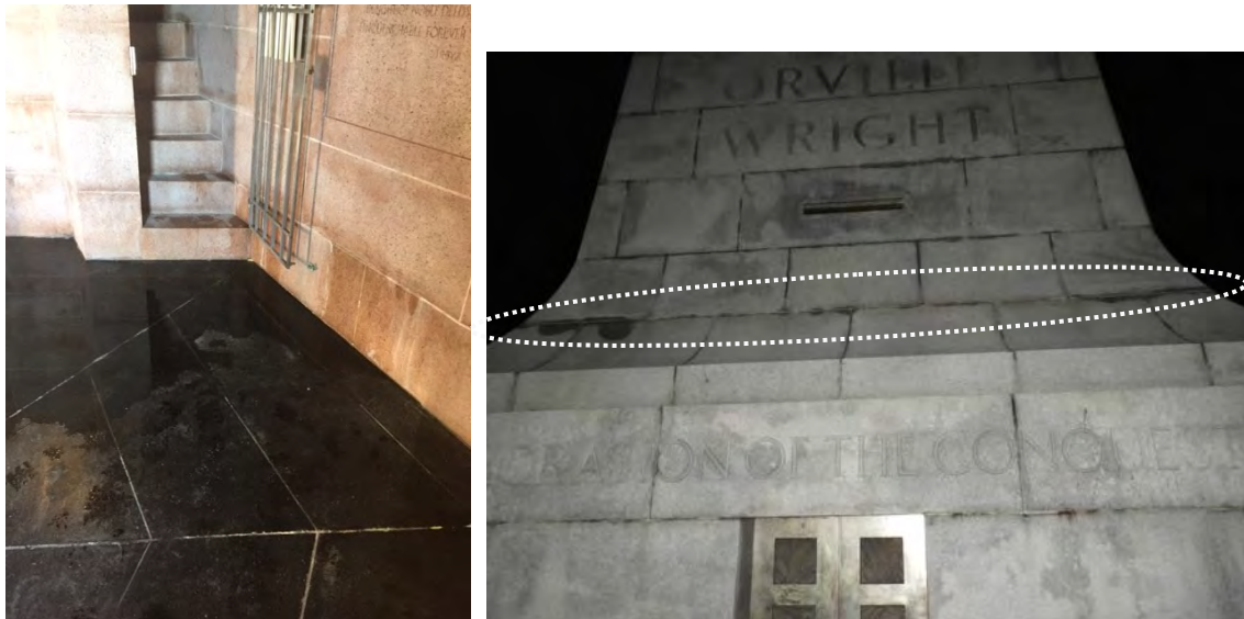
Figure 28. Water pooling in lobby (left) and exiting joint at flashing (right).
