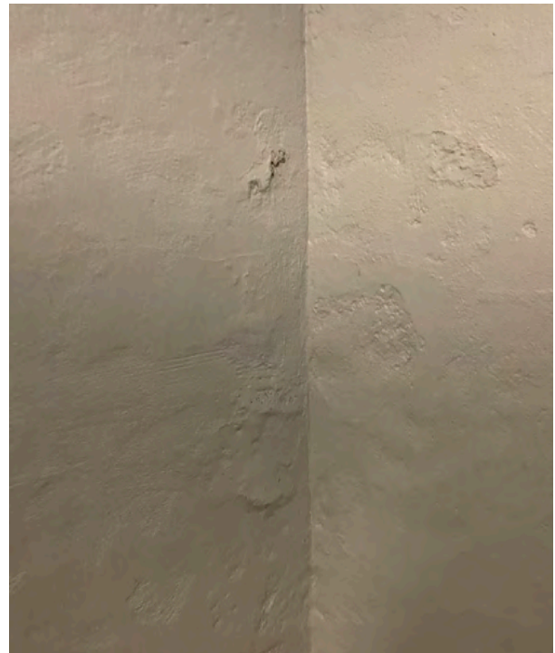
FIGURE 3–13. Interior of the pylon, showing bubbling paint and surface pockets.
