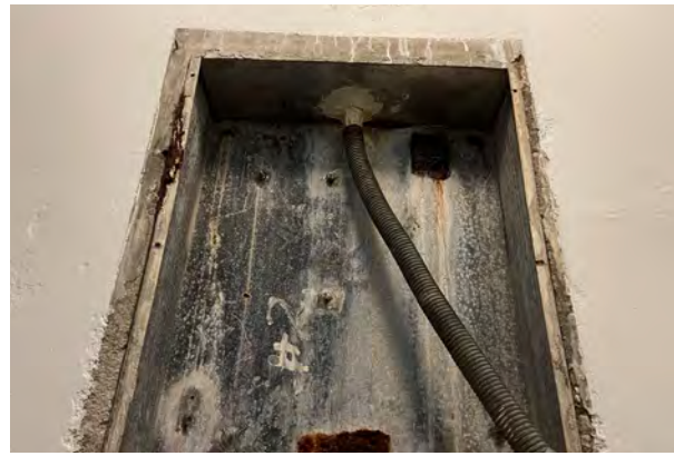
FIGURE 3–63. Electrical box and repairs at Level C.
