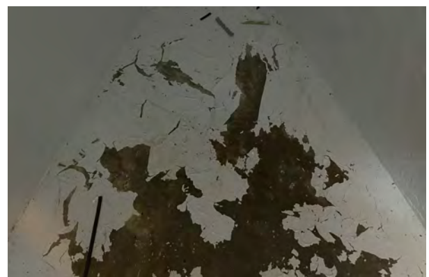
FIGURE 3-54. Peeling and worn paint at intermediate landing in the pylon.
