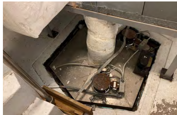
FIGURE 3-52. Metal light and mechanical diffuser at center of the floor in Level B.
