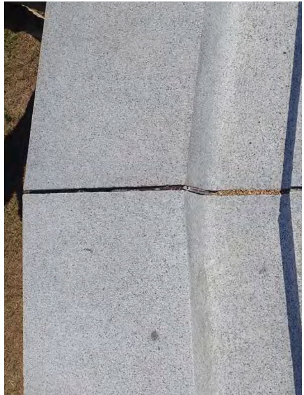
FIGURE 3–31. Typical condition of open top joints at terrace wall.
