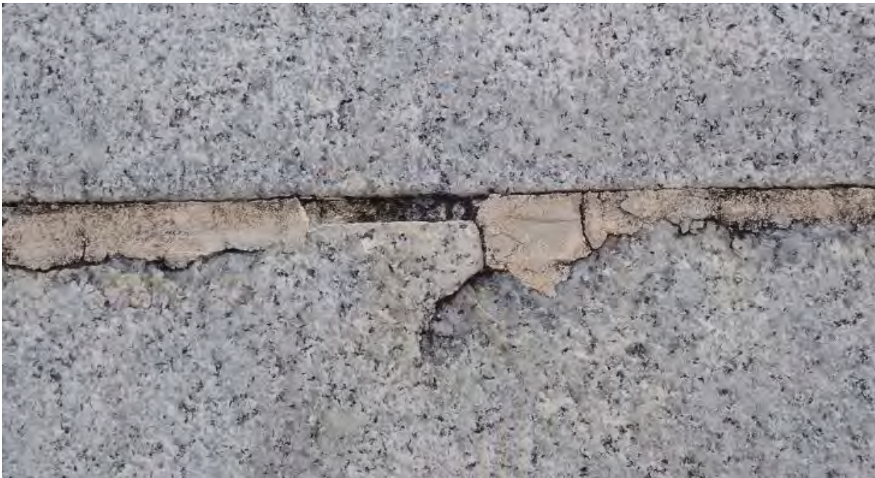
FIGURE 5-2. Typical condition of mortar joints at Monument, rake out and repoint (QE 2021).
