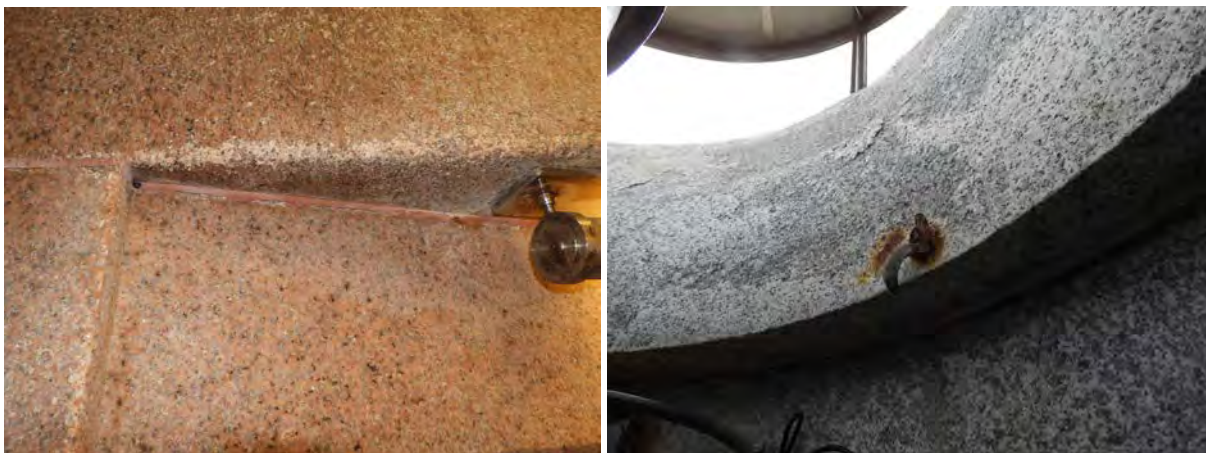
Figure 14. Scrapings removed from deteriorating stone surfaces. Left: stone at interior stairs, 2 nd level. Right: interior granite surface at top beneath beacon.
