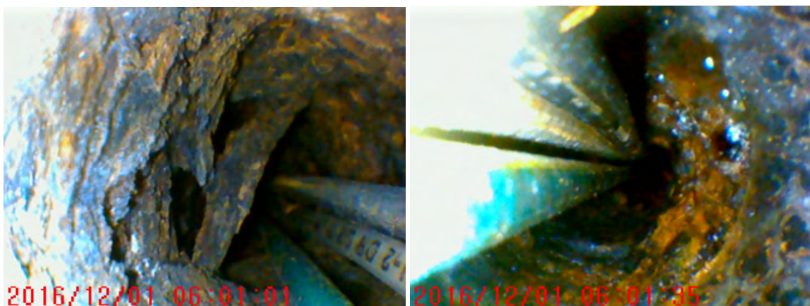
Figure 24. Videoscope evaluation at 1 st level conduit above removed light fixture. Severe corrosion and moisture noted.
