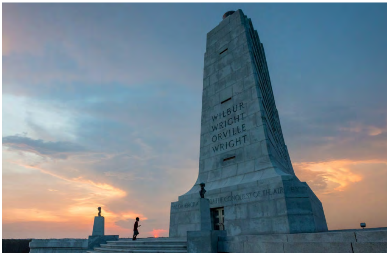
FIGURE 2–43. The Wright Brothers Monument showing signs of moisture penetration, three to four years after the 2014-15 masonry cleaning, 2018. ( https://ncseagrant.ncsu.edu/coastwatch/previous-issues/2018-2/winter-2018/bundle-up-and-explore-coastal-winter-adventures/ )
