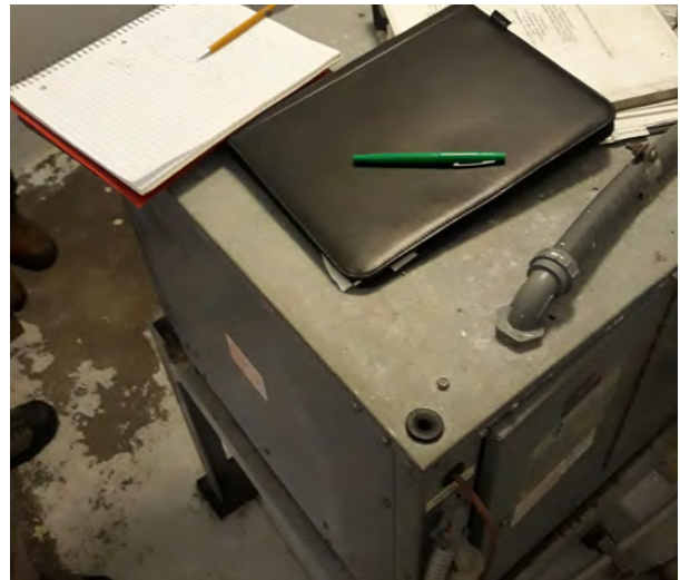
FIGURE 3-58. Existing dehumidification unit.
