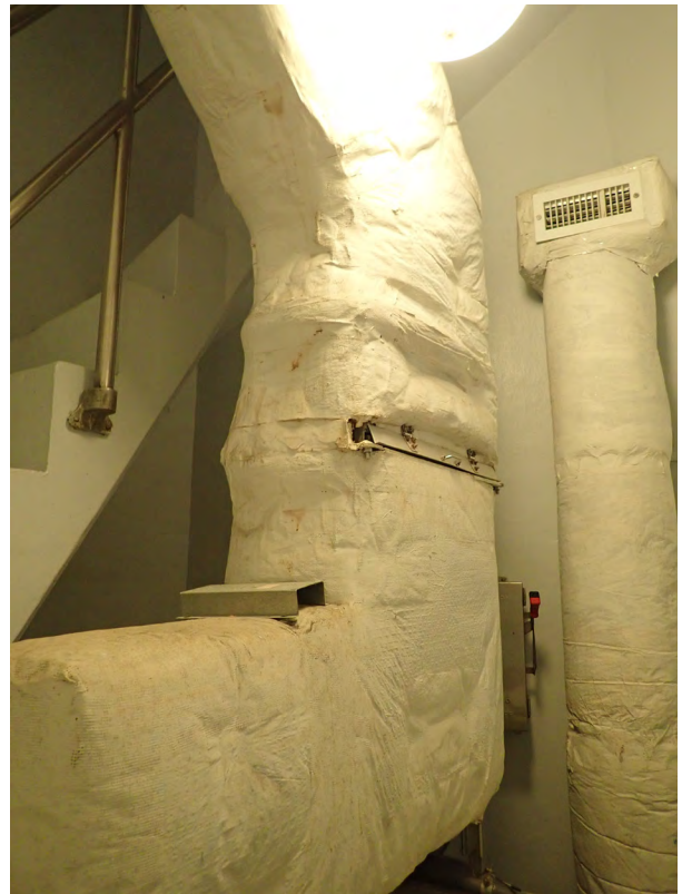
FIGURE 3-48. Center of Level B containing MEP equipment.
