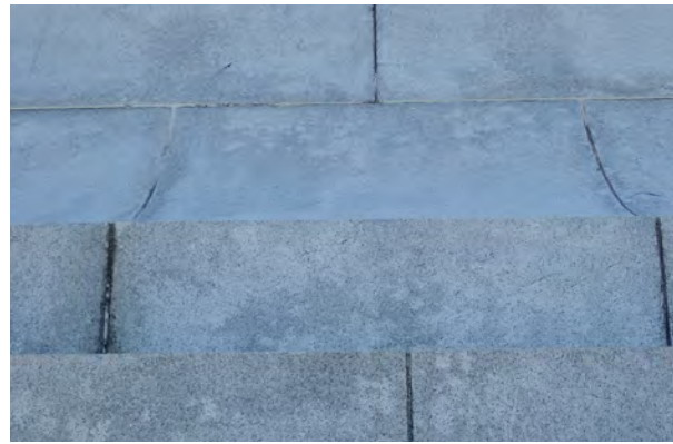
FIGURE 3-16. Close up view of the curved profile stone (Course D), with non matching sealant in joints.
