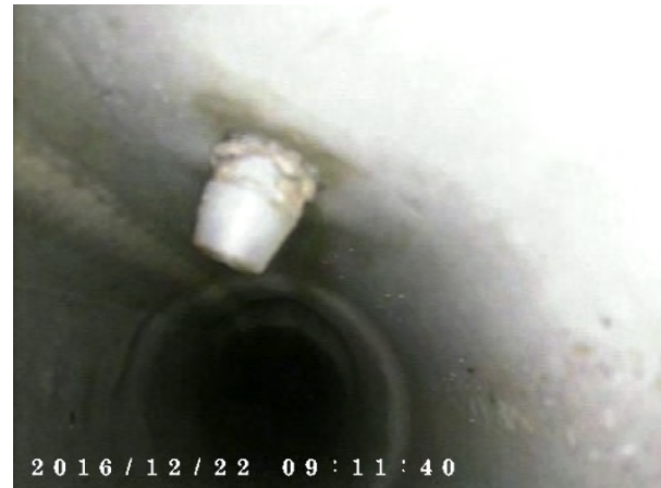
FIGURE 5-9. Bolt intrusion in roof drain pipe (Atkinson-Noland & Associates, Inc. et al, 2017).
