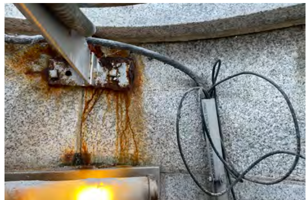
FIGURE 3-24. Beacon attachment and light below, surface staining and rust at metal.
