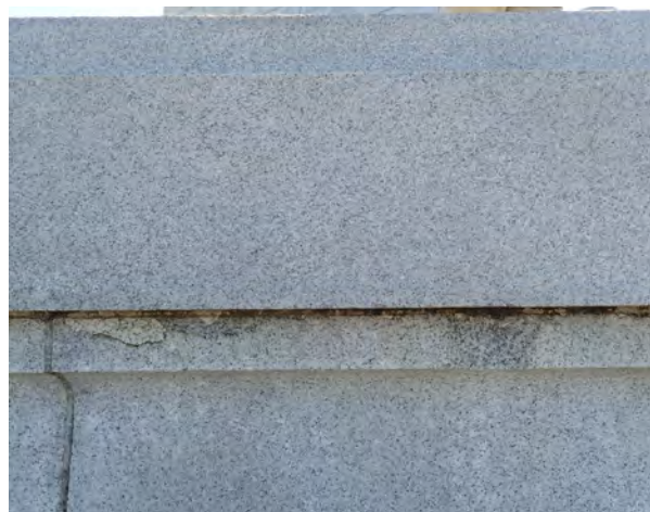
FIGURE 5-1. Typical spall condition at pedestal walls (QE 2021).
