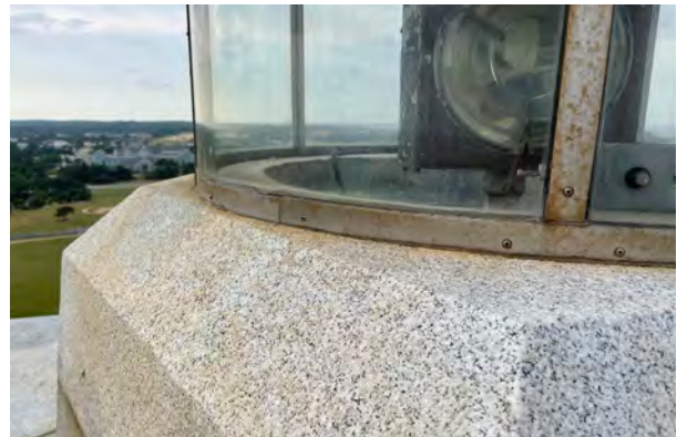
FIGURE 3-25. Exterior of beacon with failed sealant joints and surface rust.
