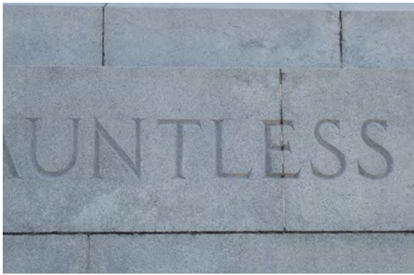
FIGURE 3-14. Close up view of the base courses, showing typical open joints and deterioration.
