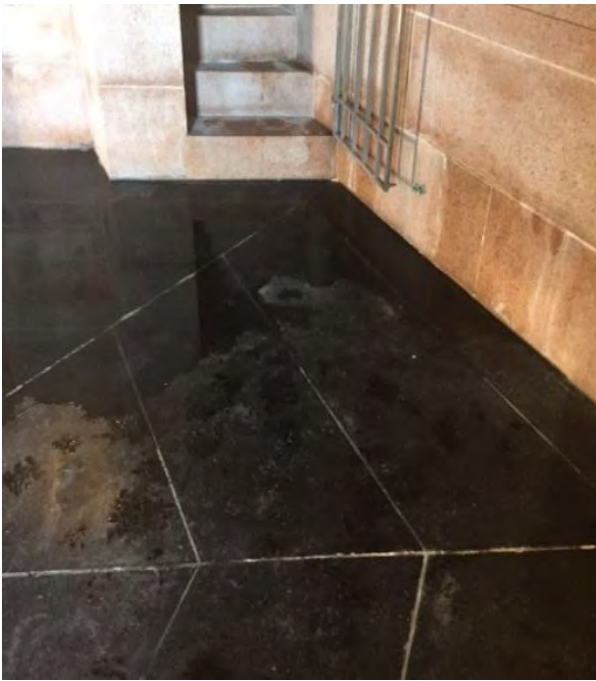
FIGURE 5-4. Moisture staining on the ground level floor (Atkinson-Noland & Associates, Inc. et al, 2017).
