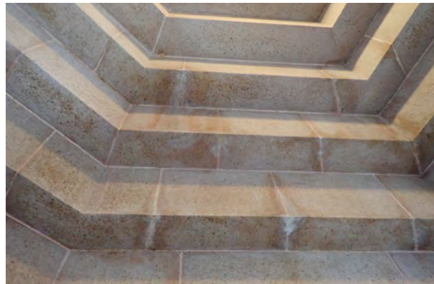
FIGURE 3-43. Water staining at joints in ceiling.
