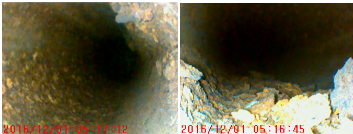
Figure 22. Videoscope images at conduit to left of 3 rd level electrical panel. Corrosion was moderate to severe with oxidation flakes collecting at the bottom of the conduit.
