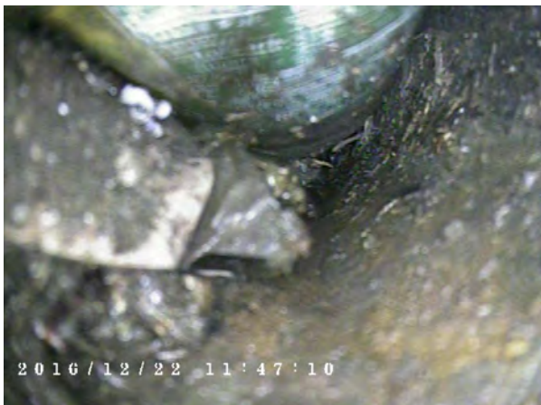
FIGURE 5-11. Drain line blockage (Atkinson-Noland & Associates, Inc. et al, 2017).
