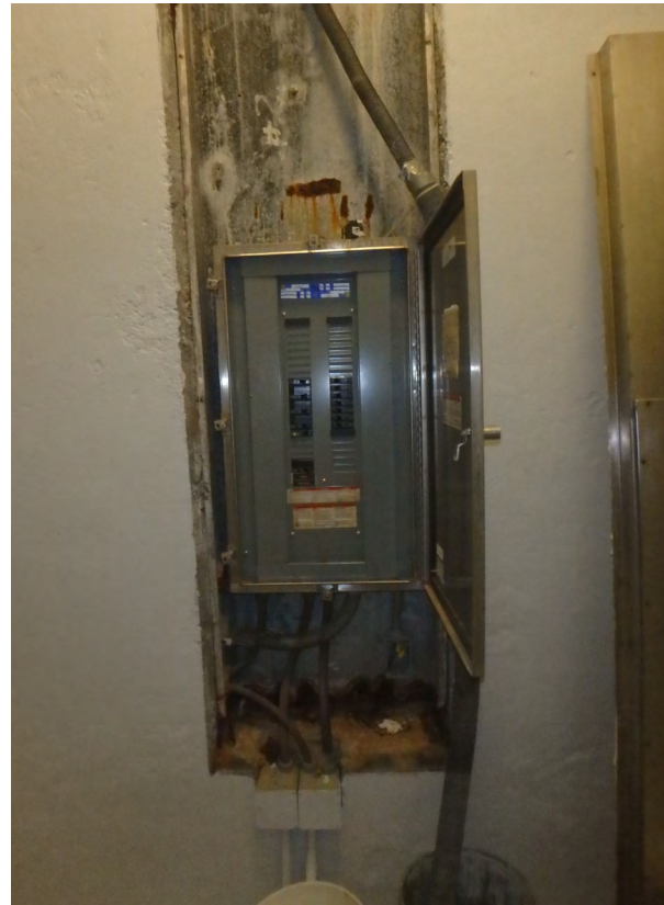
FIGURE 3–64. Old panel metal box, panel rust.
