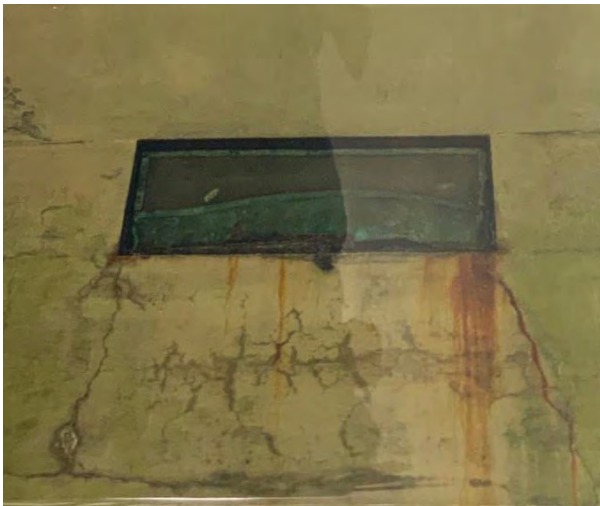
FIGURE 2-38. Condition of the Powerhouse interior vent opening prior to the stabilization, 2000. (WRBR Collection)
