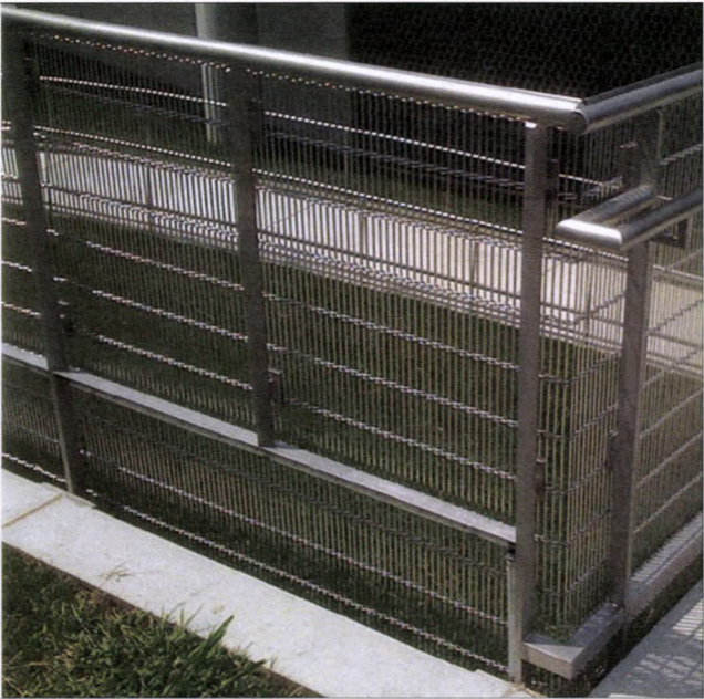
Stainless Steel Guardrail
