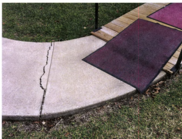
FIGURE 68. View southeast of the concrete walk as it approaches the wood ramp to the Cassidy House front porch. The walk is slightly raised and exhibits cracking. Photograph by Oculus, October 16, 2012.
