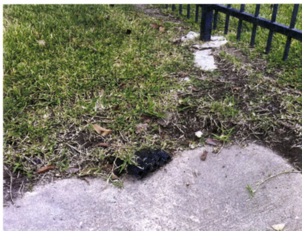
FIGURE 97. This exposed drainage piping is at the top of a concrete flume that drains to the sidewalk on South Hervey Street looking east. Photograph by Oculus, October 16, 2012.
