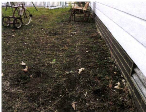
FIGURE 73. Looking west at the ground surface of the south play yard adjacent to the south wall of the Cassidy House. Note bare soil patches and moss indicating poor drainage. Photograph by Oculus, October 16, 2012.
