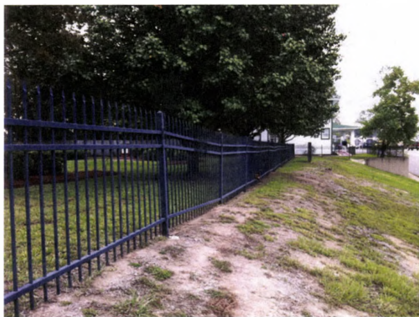
FIGURE 150. View south showing erosion on the bank just outside the metal perimeter fence. Photograph by Oculus, October 16, 2012.
