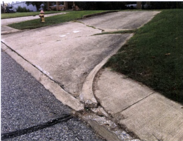
FIGURE 175. Looking northeast at a detail of the concrete apron connecting West Division Street and the visitor center driveway. Note the deterioration of concrete. Photograph by Oculus, October 16, 2012.
