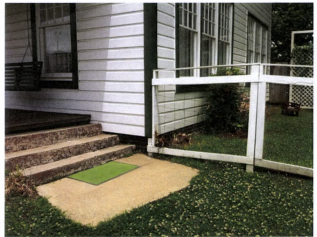
FIGURE 229. View toward the east. Note the surviving concrete steps; the major changes in the building siding; the missing porch screen walls and door; the missing curved concrete walk; and the play yard fence constructed to match the historic period fence. A lattice structure and fence screen the Vincent Foster property. Photograph by Oculus, May 29, 2013.
