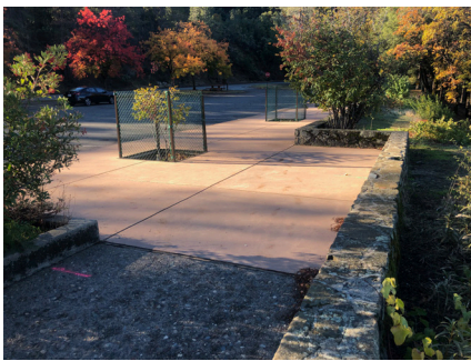
Figure 3 The portion of concrete replaced south of the courtyard has a different texture and pinkish color.
