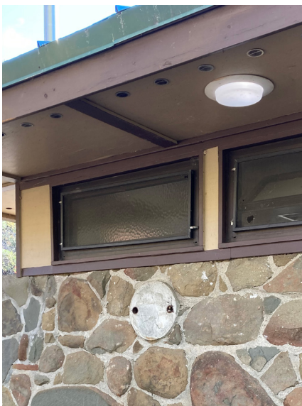
Figure 19 Large grouted cylinders of wall with metal wall anchors exist where a flagpole was previously mounted.
