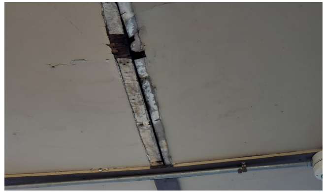
Figure 8 Redwood trim is missing from this canopy soffit likely due to a water leak in the roof above
