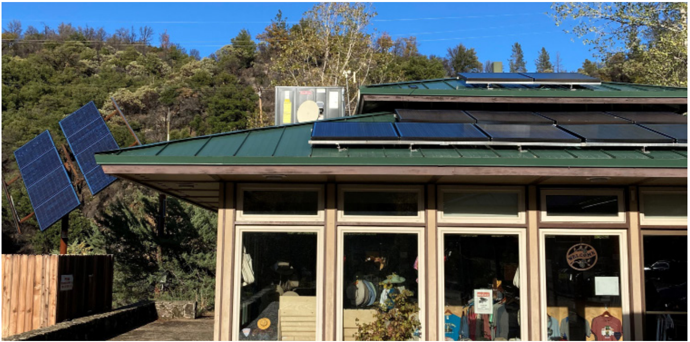
Figure 25 The packaged mechanical unit and solar panels are poorly placed on the roof of the primary building elevation.
