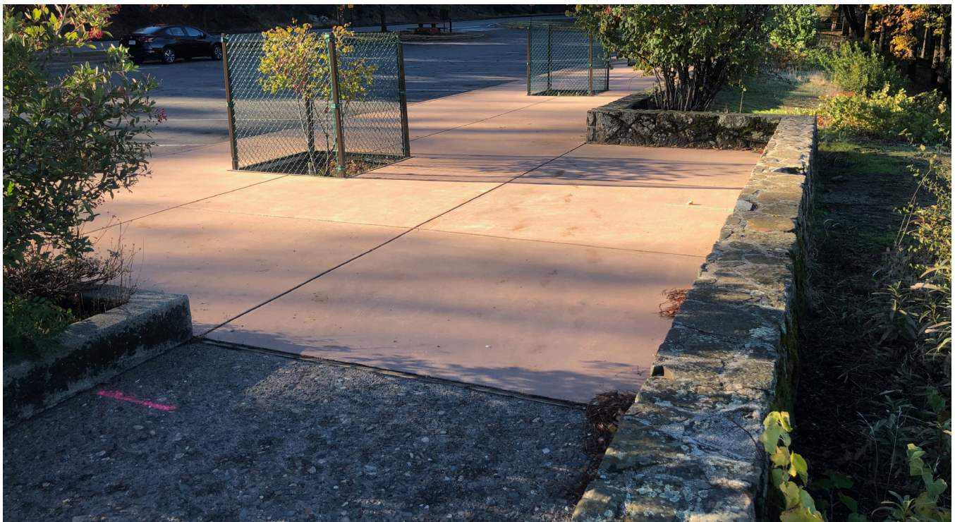
Figure 13 Detail showing replacement integrally-colored concrete at south end of the promenade.
