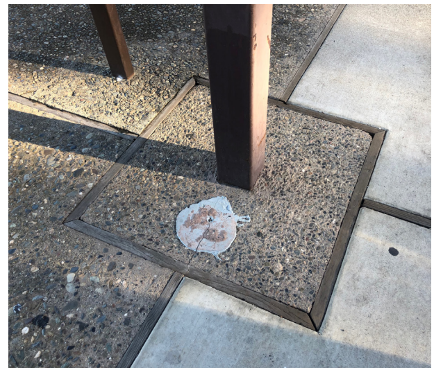
Figure 2 Incompatible material was used to fill a previous post location.
