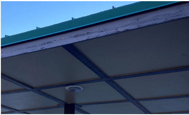
Figure 7 Peeling paint at a typical redwood canopy fascia. Note that the original 1x4 redwood fascia trim is covered by the metal roofing.
