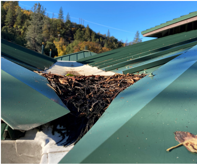
Figure 17 Organic debris has built up at the valley gutter.
