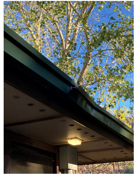
Figure 16 Portions of gutter are damaged and require replacement.
