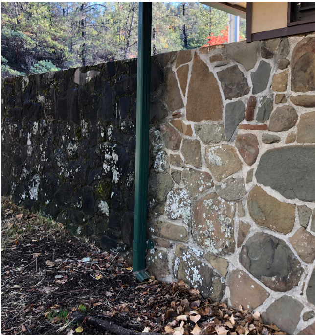
Figure 42 The masonry wall extension at the east end of the north façade, looking southeast. This image also illustrates the mortar repairs and the biological growth on the east end of the north wall.
