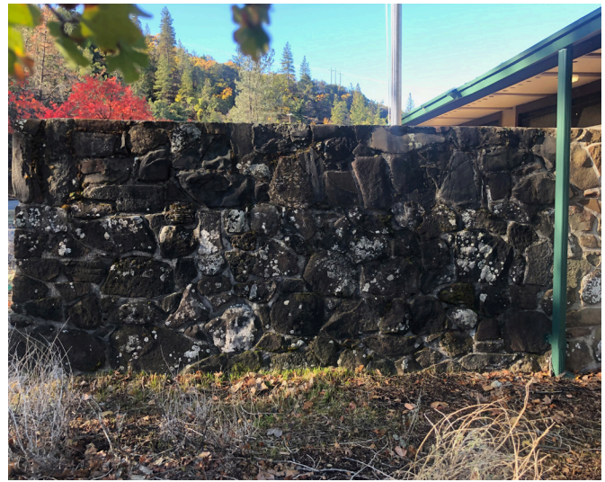
Figure 21 The western portion of the northern rubble wall is very dirty with excessive bio growth.
