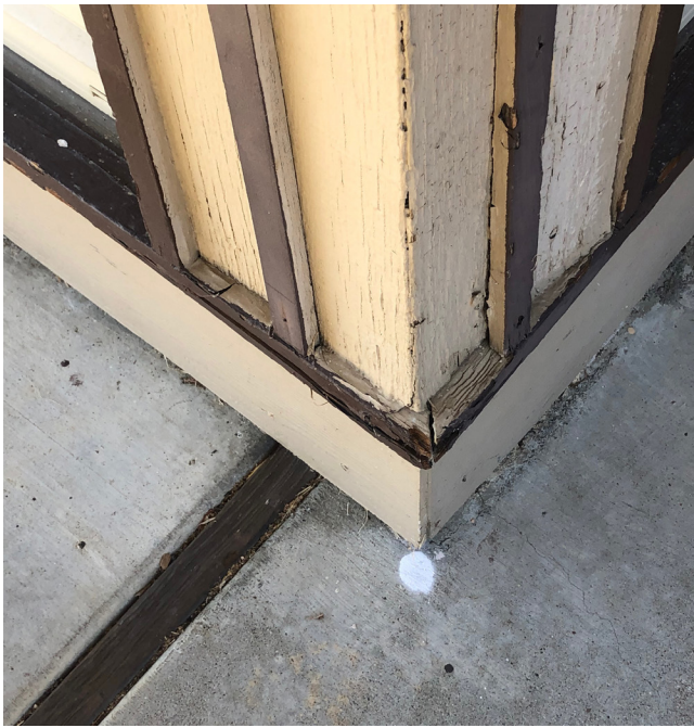
Figure 23 Typical deteriorated redwood window trim.
