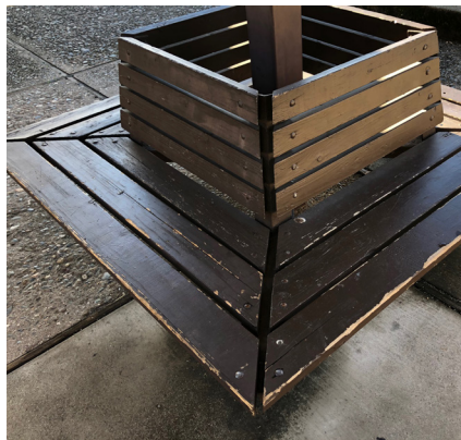
Figure 9 Typical worn edges and paint at an original built-in redwood bench
