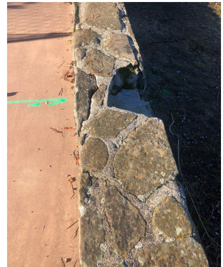
Figure 5 A large stone is missing at the west side of the rubble wall.
