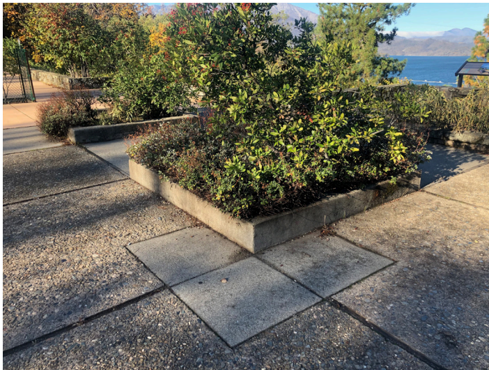
Figure 1 Portions of the original exposed aggregate concrete have been replaced.
