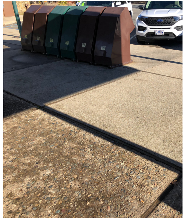
Figure 19 The bear-proof garbage bins at the north end of the promenade and an example of the replacement concrete that does not match the original concrete aggregate used throughout the promenade.
