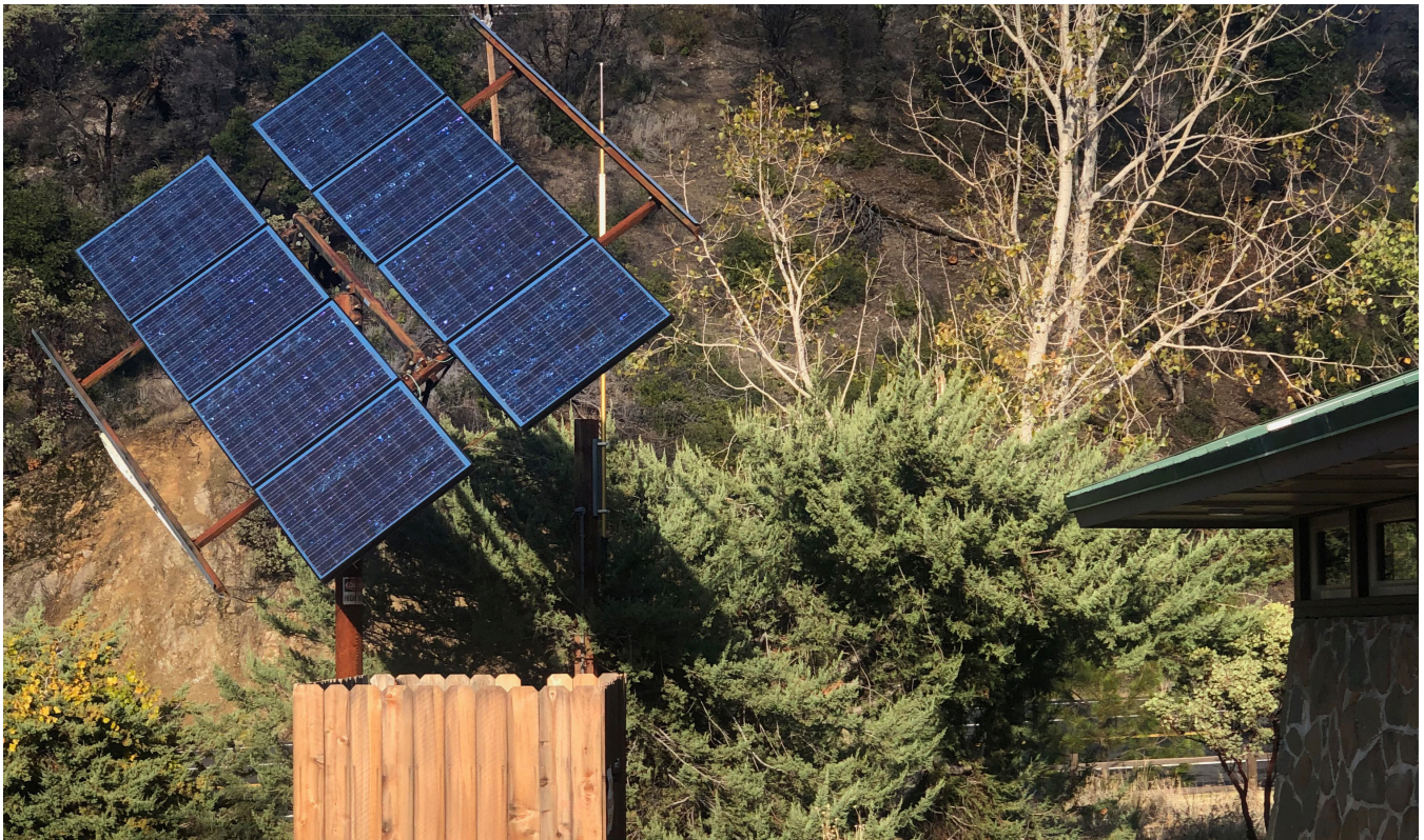
Figure 10 The solar panels at the northwest corner of the Visitor Center site, looking north.
