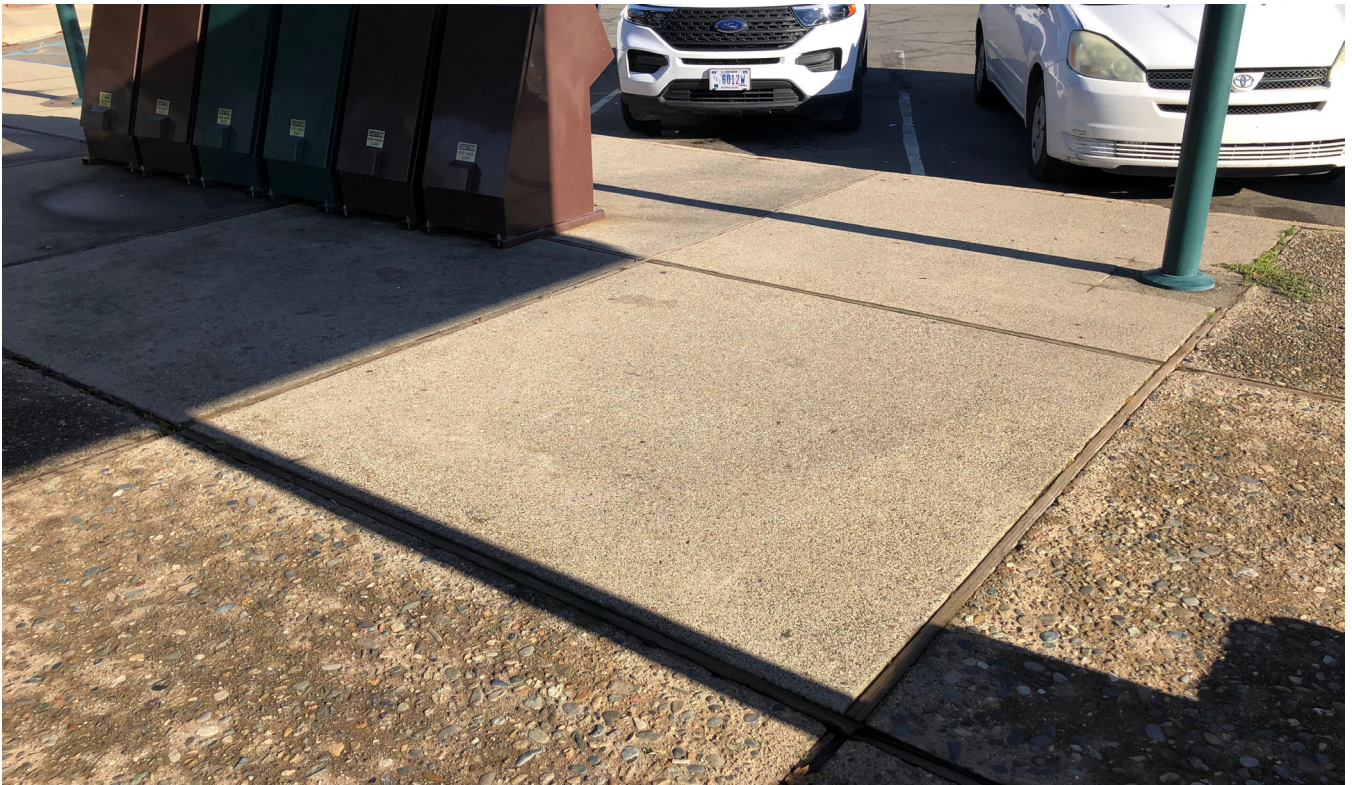
Figure 12 Example of the replacement paving at the promenade which does have the same aggregate quality as the original.
