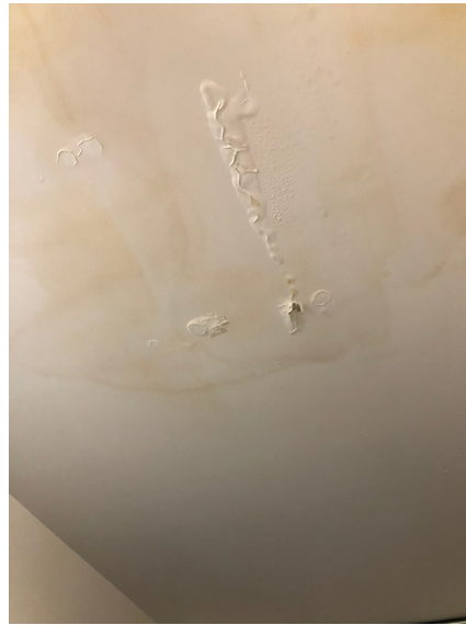
Figure 15 Ceiling staining is indicative of water failure at converging roof valleys above.
