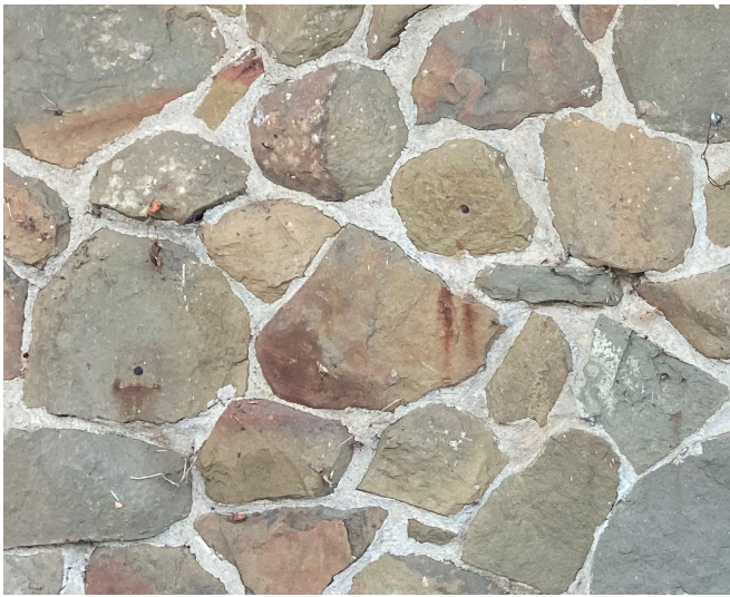
Figure 20 Small holes remain where items were previously attached to the rubble stone wall.
