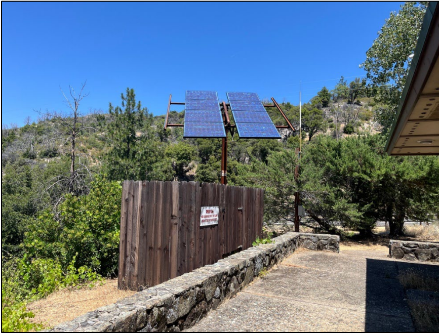
Figure 49. Photovoltaic panels and propane tank fence, camera facing north (NPS 2025).
