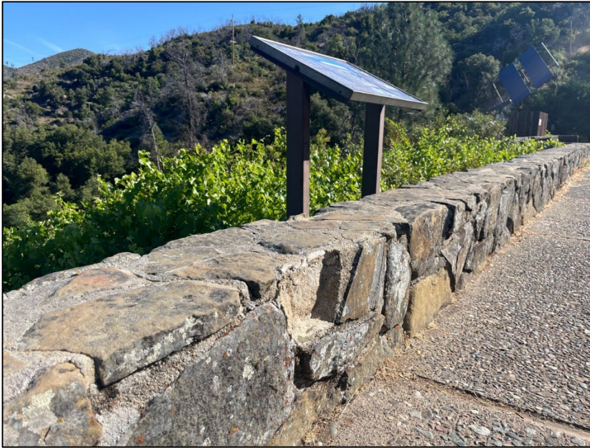
Figure 37. Missing masonry on the perimeter rubble masonry wall, camera facing north (NPS 2025).
