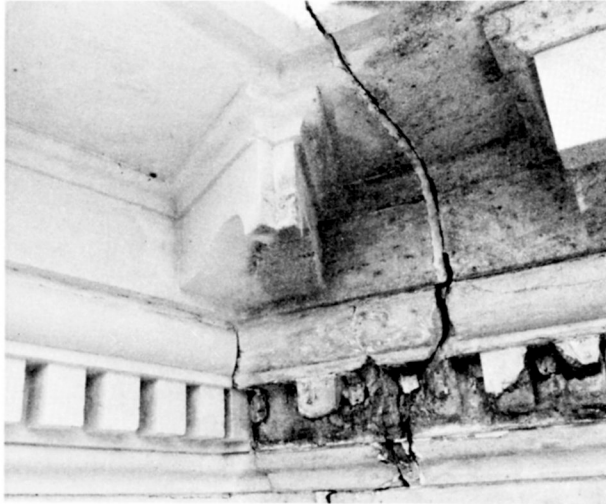
Fig. 25 One of the major cracks in the entablature of the south wall. This view also shows the results of environmental damage where the protected stone dentils absorbed airborne pollutants that could not be washed off by rainwater. Over the past 200 years, many of the dentils have been destroyed or damaged in this way. photo: Bill Allman, Office of the Curator, The White House.
