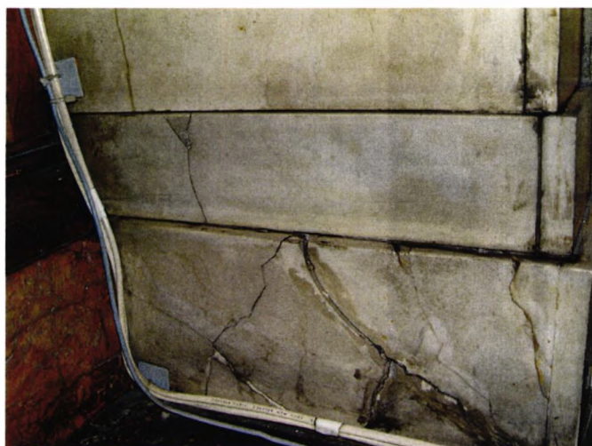
Figure 14. Various cracks are apparent, and chips were repaired at the bottom proper right of the side panels.
