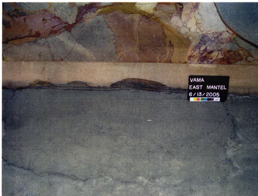
Figure 2. The top of the fascia and frieze panel consists of plaster/cement over metal mesh.
