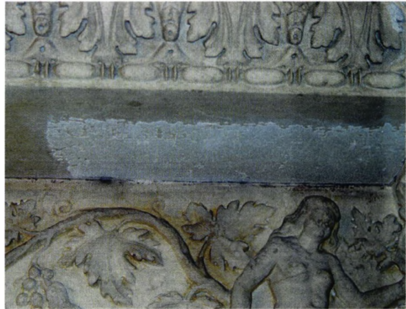
White, powdery accretions on underside of mantel.
