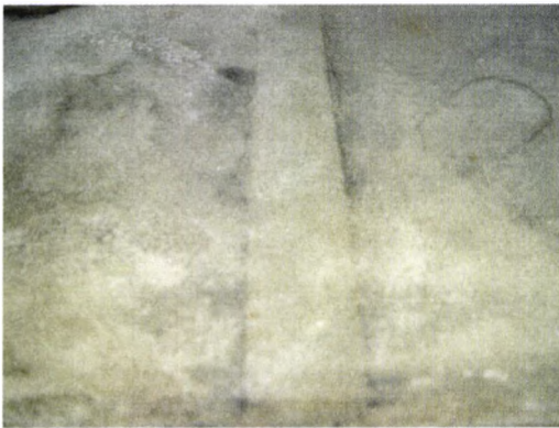
Staining on balustrade.
