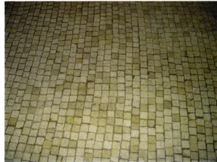
Grout is becoming loose, dislodging tiles in some areas.
