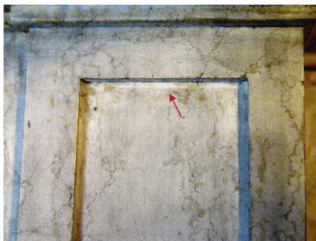
Figure 15. Toning was also apparent on the fireplace surround. The natural, white color of the marble can be seen between the molding and inset piece.
