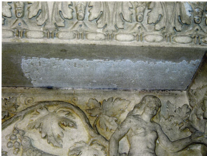
Figure 11. White, powdery accretion on the underside of the mantelpiece.
