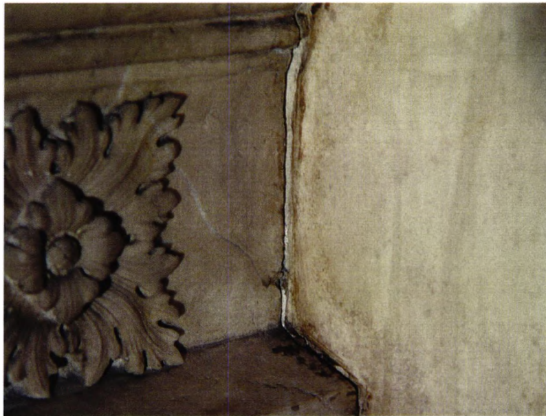
Figure 11. Accumulated brown toning is apparent in the gaps between the flat marble panels and the fireplace surround.
