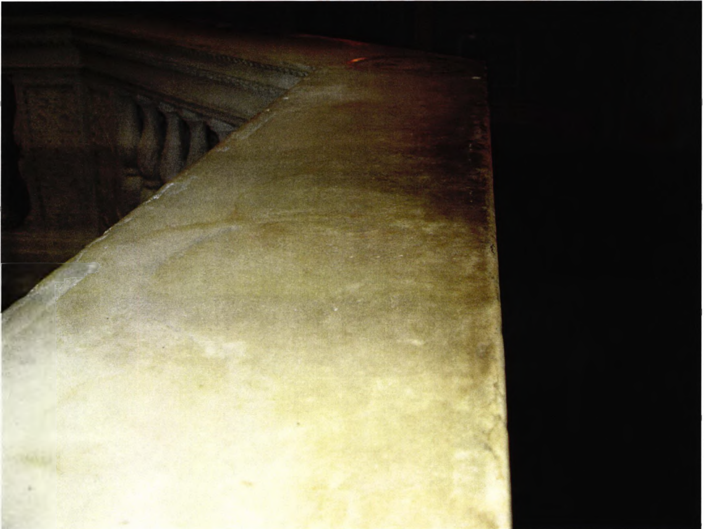
The top of the balustrade before treatment showing dirt and lipids from visitors.
