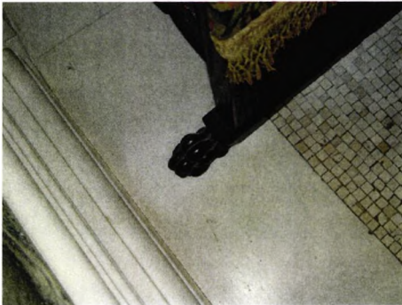
The floor appears lighter under furniture, suggesting a yellowed floor coating.
