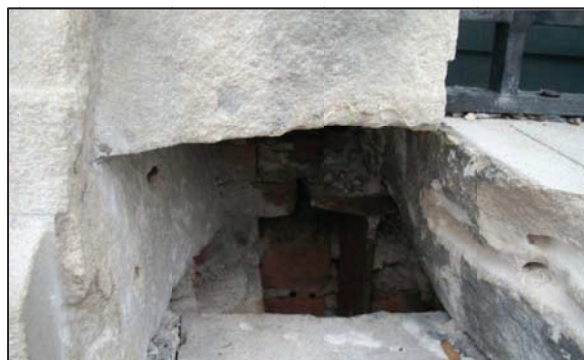
Photo 4 – Probe at Window Sill
