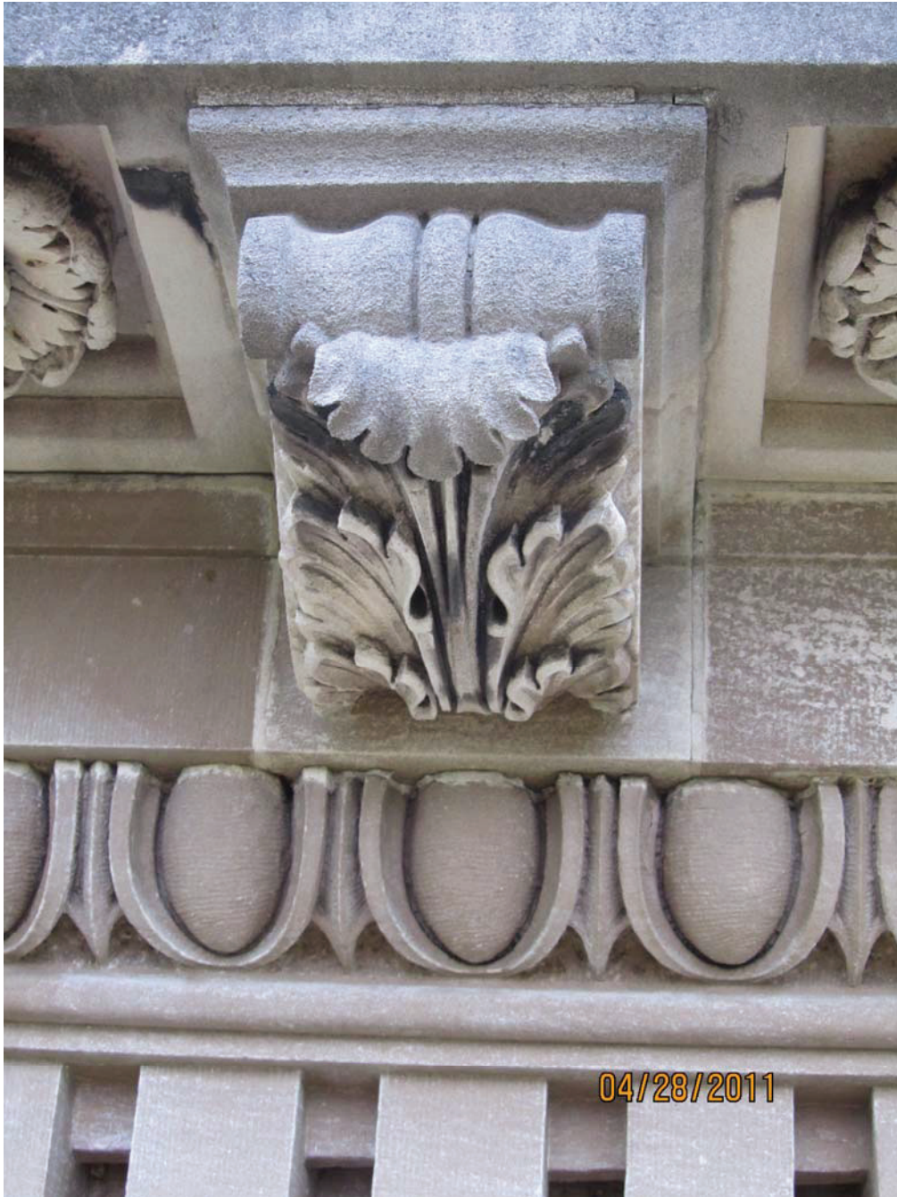
Test area #4, cornice modillion conditions with black crust in protected area
