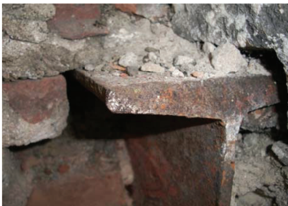
Photo 5 – Steel Framing Exposed at Window Sill Probe
