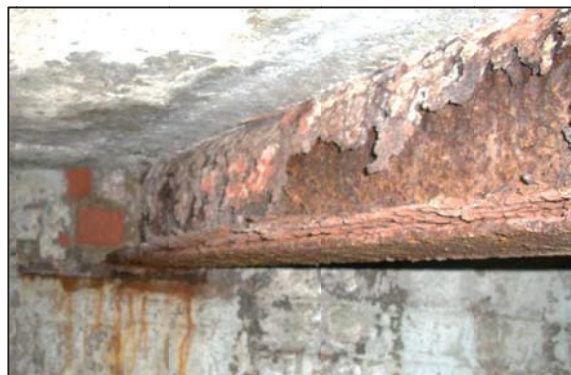
Figure 5: Deterioration at West Portico Steel Wide Flanges
