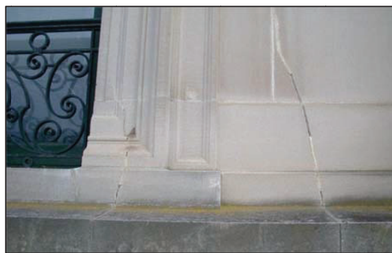
Figure 13: Stone Cracking Near Window on West Façade
