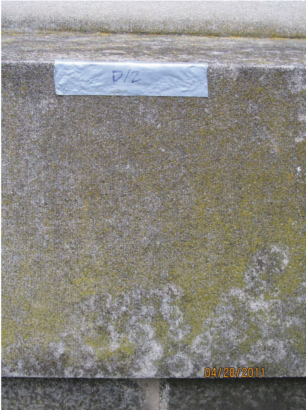
Test area #1, biological growth before cleaning with D/2
