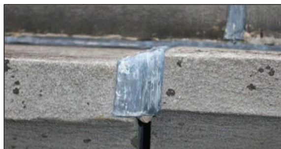
Figure 11: Rotation and Displacement at Cornice Joint
