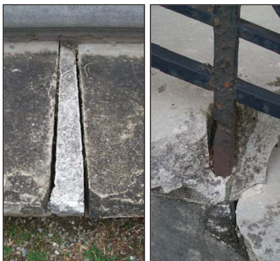
Figure 16: Joint Separation & Spalling at Portico Stairs
