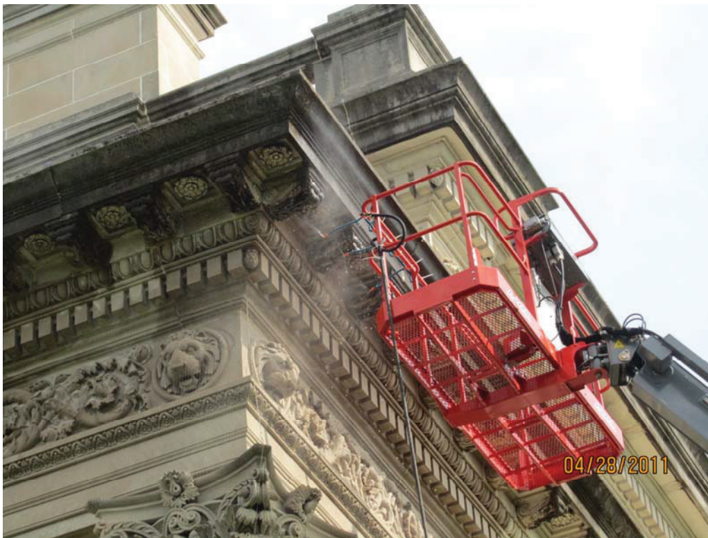
Test area #4, intermittent misting set-up
