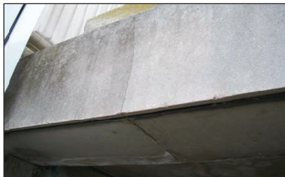
Photo 8 – Crack at Stone Lintel
