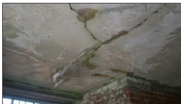
Photo 7 – Cracking in Ceiling Below North Portico
