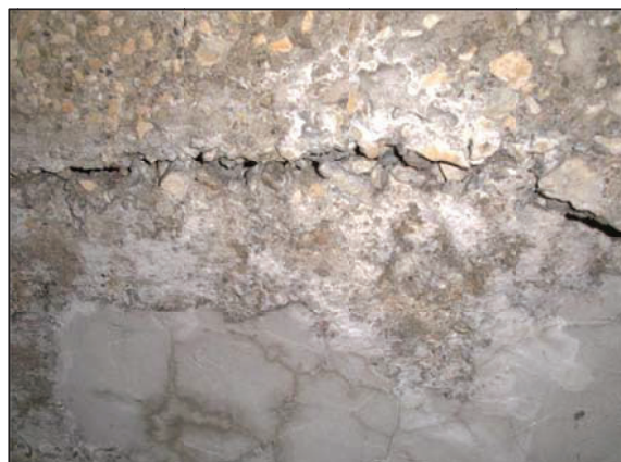
Figure 6: Spalling at the Underside of South Portico
