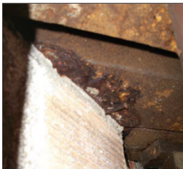
Photo 14 – Corrosion at Bearing of Steel Lintels
