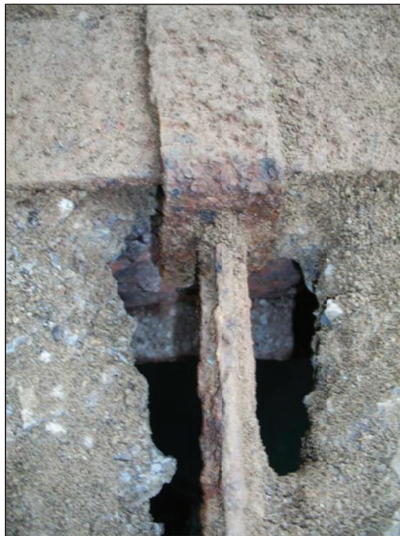
Photo 3 – Exposed Concrete Slab Reinforcement
