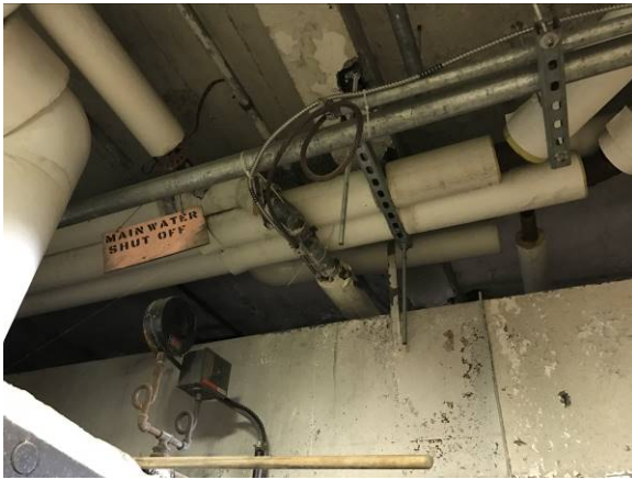
Domestic water main entering room SB02. [KR, 2017]
