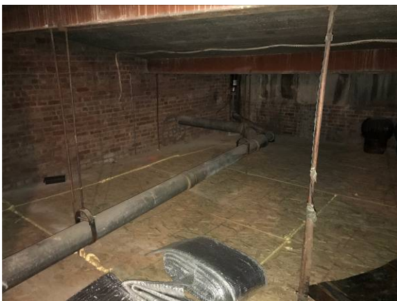
Roof drain leaders collected in the attic. [KR, 2017]
