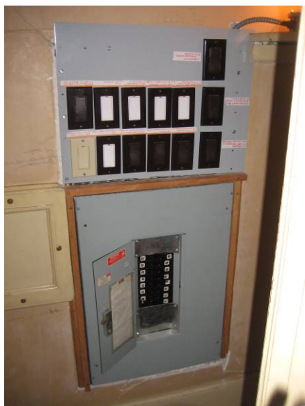
Lighting Control relays with bypass manual switches. [KR, 2017]
