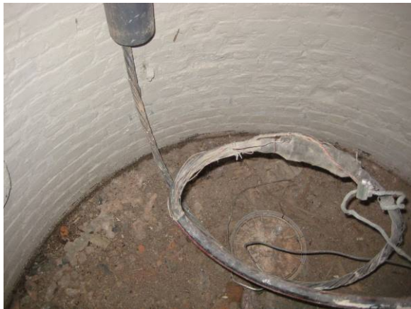
2,500 volt entrance in room adjacent to room SB03. [KR, 2017]
