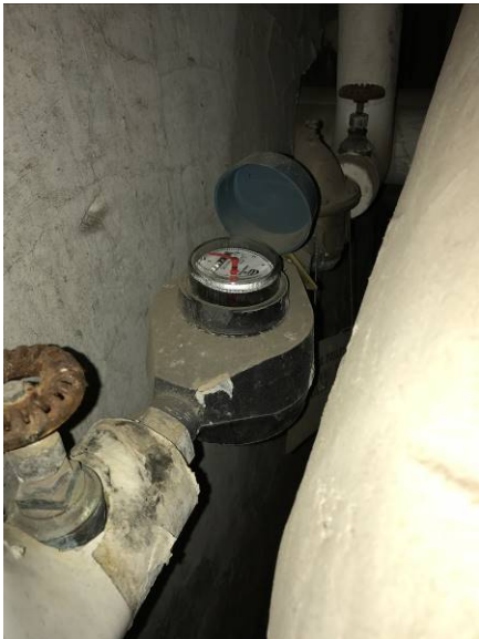
Domestic water meter and pressure reducing valve in room SB02. [KR, 2017]
