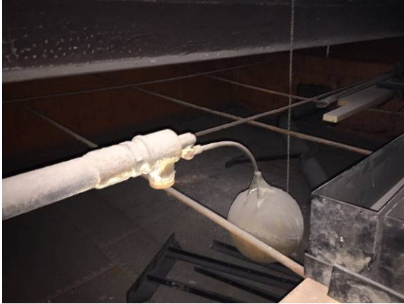
Abandoned domestic water storage tank in attic room 402. [KR, 2017]
