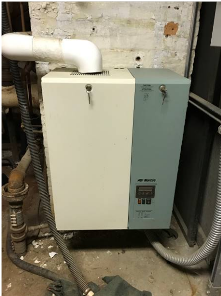
Electric humidifier located in room SB02. [KR, 2017]
