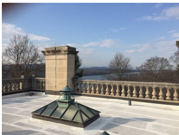
Lightning protection air terminals on parapet. [KR, 2017]
