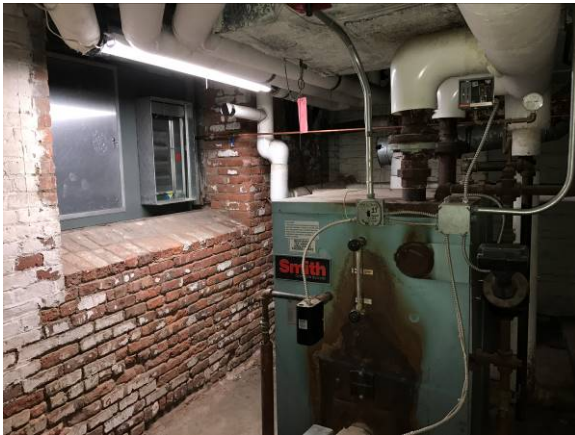
Combustion air louver and areaway access in room SB03, adjacent to Boiler #1. [KR, 2017]
