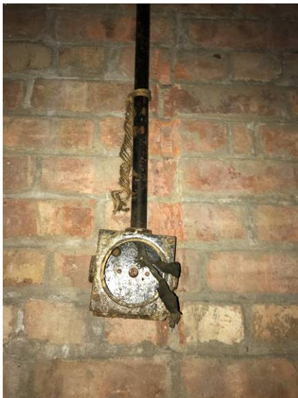
Original abandoned wiring, conduit and box in room SB06. [KR, 2017]
