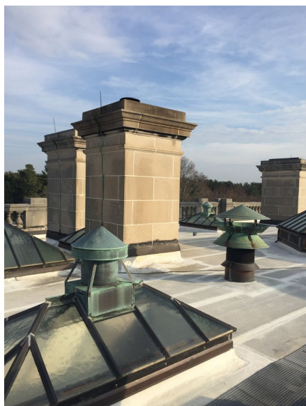
Lightning protection air terminal on boiler flue chimney. [KR, 2017]
