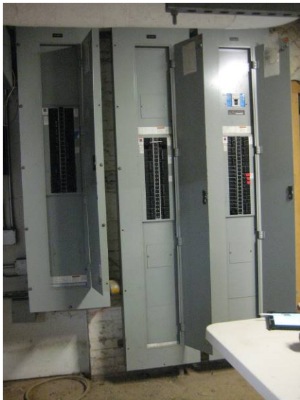
3 section panelboard in room SB03. [KR, 2017]
