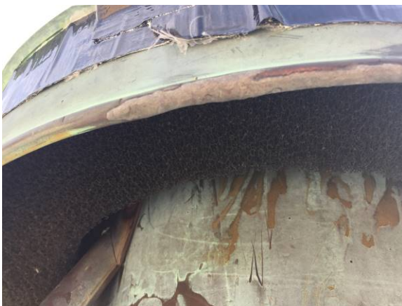
Insect mesh in skylight vent. [KR, 2017]
