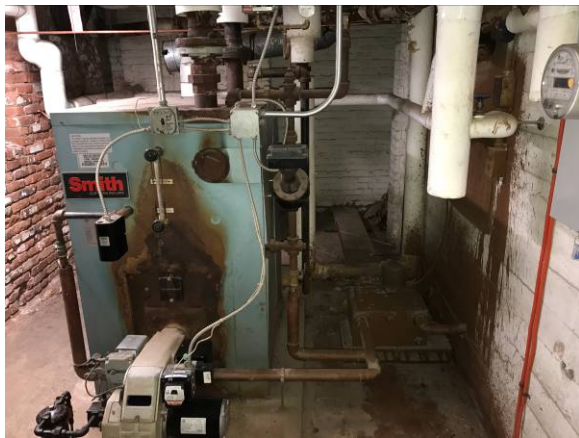
Oil fired boiler; Boiler #1; and condensate receiver in room SB03. [KR, 2017]
