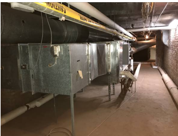
Air handling unit in room SB06. [KR, 2017]
