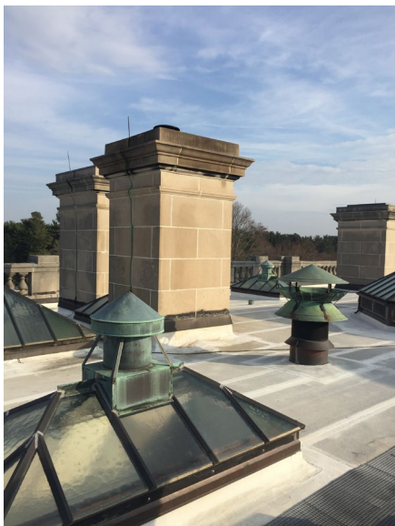
Boiler flue termination through masonry chimney (center of picture). [KR, 2017]
