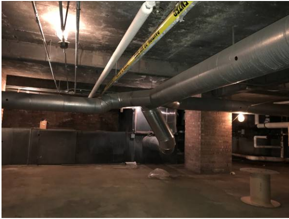
Air handling unit outdoor air intake ductwork connected to the outdoor air intake plenum and areaway in room SB14. [KR, 2017]
