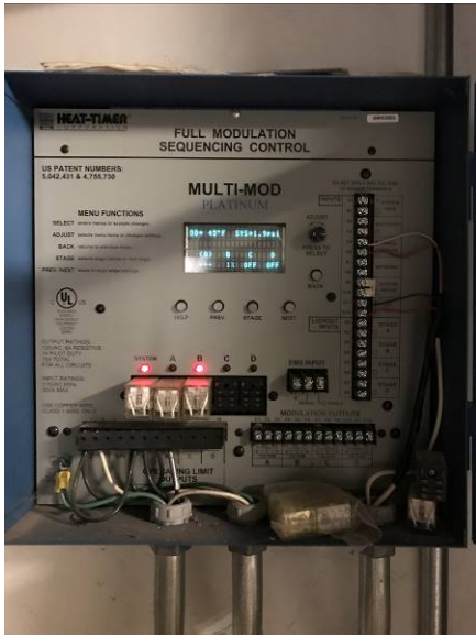
Sequencing modulating boiler controller in room SB03. [KR, 2017]
