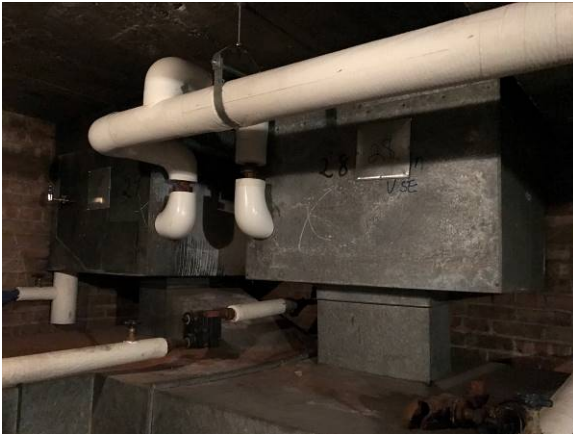
Gravity steam convector ducted to architectural grilles. [KR, 2017]
