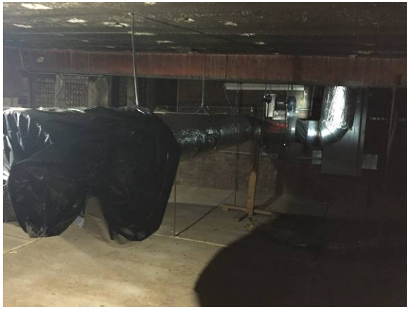
Toilet exhaust fan in the attic room 402. [KR, 2017]
