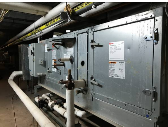
Air handling unit in room SB06. [KR, 2017]
