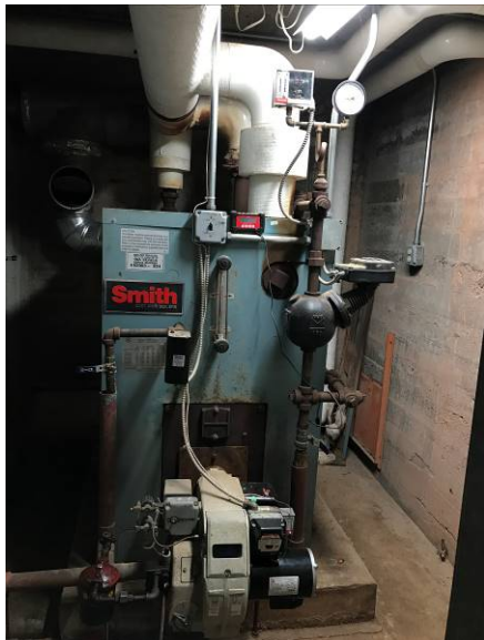
Oil fired boiler; Boiler #2; in room SB03. [KR, 2017]
