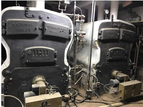
Abandoned boilers and oil burners in room SB02. [KR, 2017]
