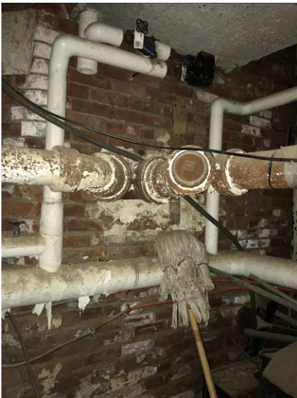
Sanitary mains combining with cleanout, leaving room SB02. [KR, 2017]
