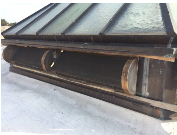
Hall Well skylight vents and screens. [KR, 2017]
