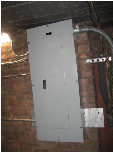
Panelboard located in the attic. [KR, 2017]
