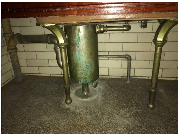
The Tucker Grease Trap in Scullery room B02. [KR, 2017]
