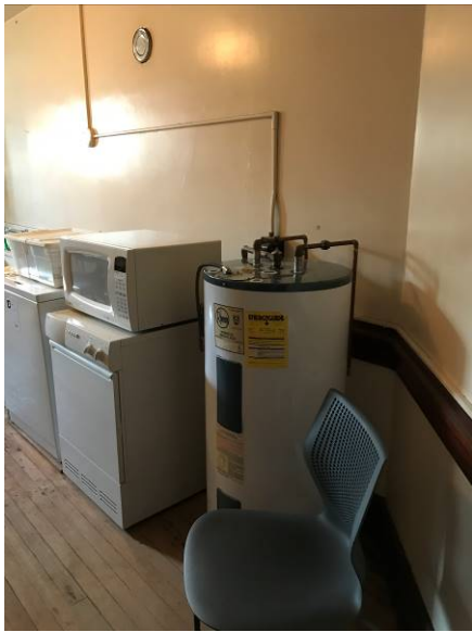
Electric water heater in Service Laundry room B06. [KR, 2017]
