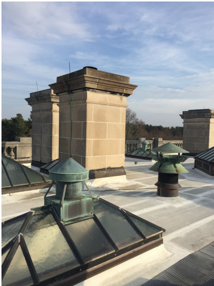
Skylight vents and exhaust fan discharge terminations from roof. [KR, 2017]
