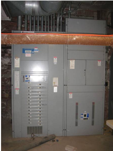
Main Switchboard in sub-basement room SB03. [KR, 2017]
