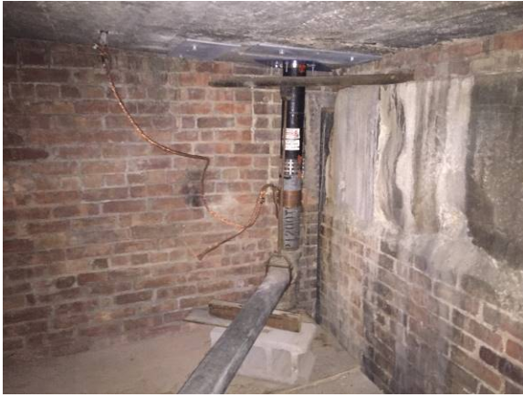
Lightning protection conductor connected to roof drain pipe in attic. [KR, 2017]
