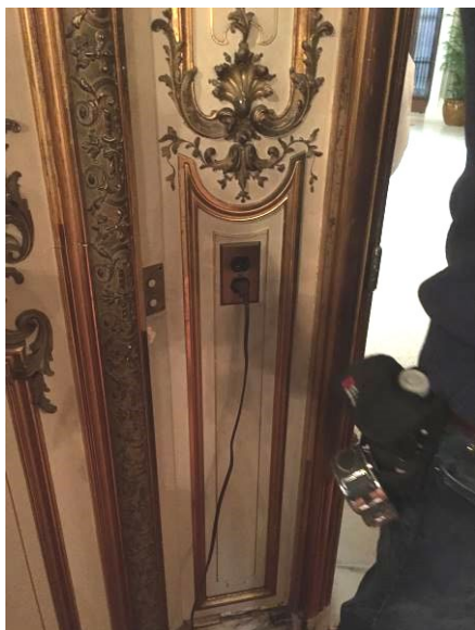
Convenience receptacle located in Reception Room 105 [KR, 2107]
