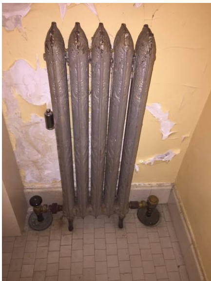
Original cast iron radiator with angle valve, thermostatic trap and air vent. [KR, 2017]
