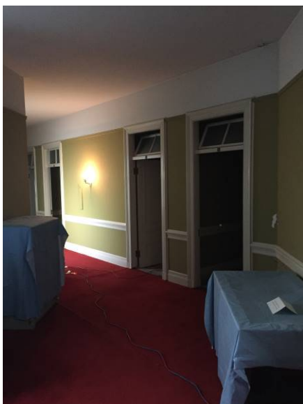
Operable transoms over the doors to promote air movement. [KR, 2017]
