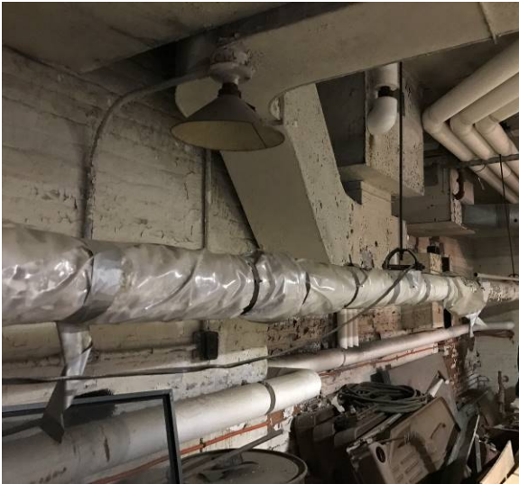
Sanitary running east/west in room SB02. [KR, 2017]
