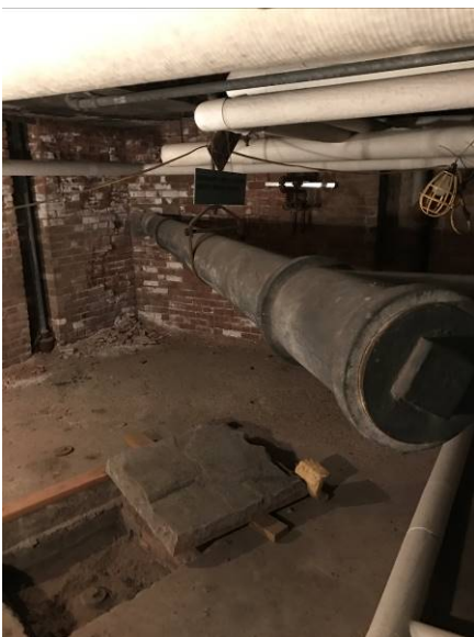
Roof drain main leaving SB17. [KR, 2017]
