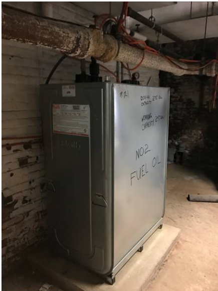
275-gallon no. 2 fuel oil day tank in room SB03. [KR, 2017]
