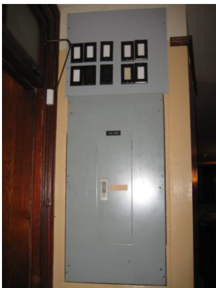
Panelboard located on the floors [KR, 2017]
