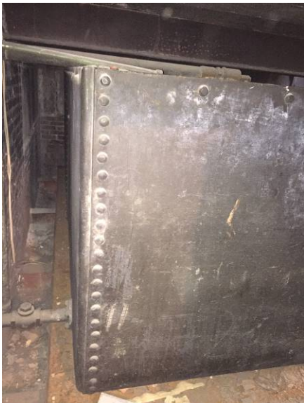
Abandoned domestic water storage tank in attic room 402. [KR, 2017]
