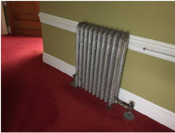
Original cast iron radiator with angle valves and air vent. [KR, 2017]
