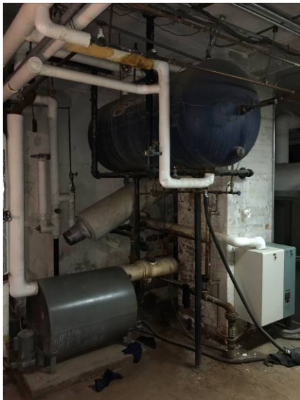
Duplex condensate receiver and pumps in room SB02. [KR, 2017]
