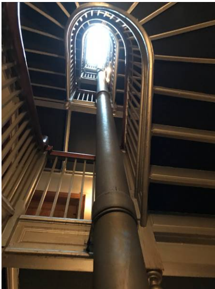
Roof drain main in the attic room 404 down to room SB07. [KR, 2017]
