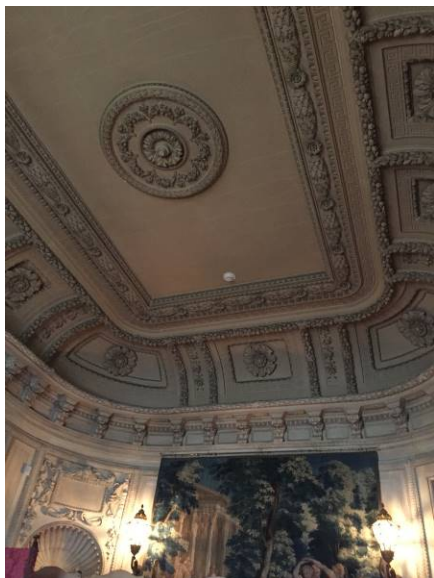
Smoke Detector at Main Stair and abandoned smoke detector in center of the medallion. [KR, 2017]
