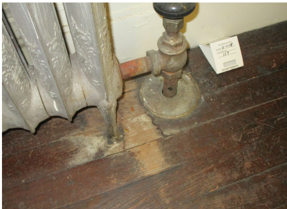
Figure 44. (Upper image) Many of the historic light fixtures were damaged in an effort to retrofit them to work with a modern system of exposed wire conduit. This is particularly prevalent at the third floor. (Lower image) In several locations steam radiators have leaked as a result of deteriorated steam release valves. This image shows surface rust and floor damage that resulted from such a leak. JGWA, 2018.
