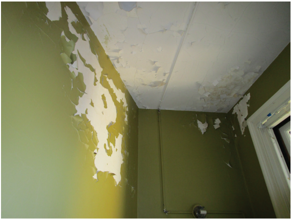
Figure 42. Numerous areas of plaster and paint deterioration exist at the third floor level. These areas are concentrated near, but are not limited to, the exterior walls. A second common condition at the third floor level is cracking across the plaster ceilings. The upper image shows a location where water has migrated along the course of a crack. These are largely unrelated issues, but the course of water through cracks has worsened the deterioration of the plaster in numerous locations. JGWA, 2018.
