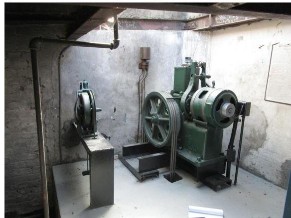
Figure 56. Water tank (upper image) and elevator equipment (lower image) in 404. JGWA, 2017.
