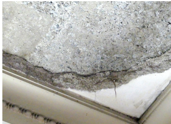
Figure 41. The guest quarters at the third floor level have suffered moisture damage. Fabric wall coverings have deteriorated in several rooms at the south end of the third floor, such as the silk in the Empire Room; and a large section of finish plaster recently became dislodged from the southwest corner of the room. JGWA, 2018.
