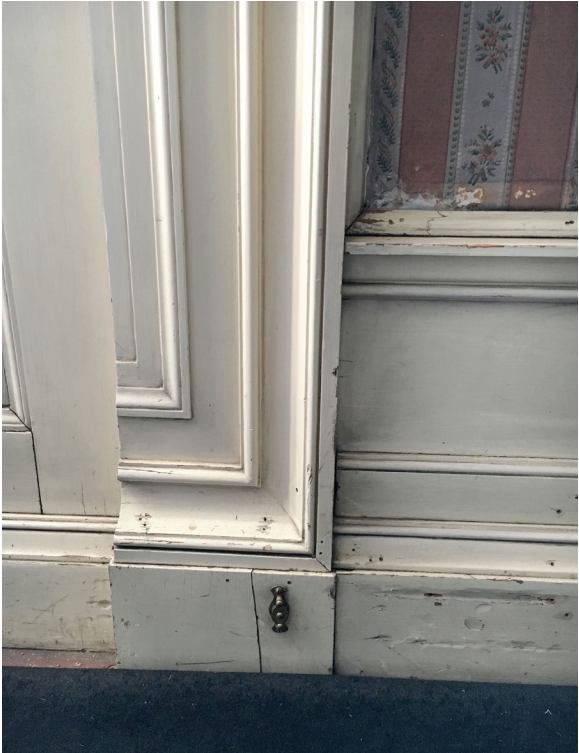
Figure 40. (Upper image) This section of wallpaper in the Small Pink Room is another example of damage from moisture infiltration. (Lower image) As is the case with many surfaces in the mansion, this section of baseboard near the east window retains its original painted finish. Although the early finish is still in sound condition it has been compromised by impact damage and holes from removed anchors. (Upper right) A large offset crack can be seen on the north wall. JGWA, 2018.
