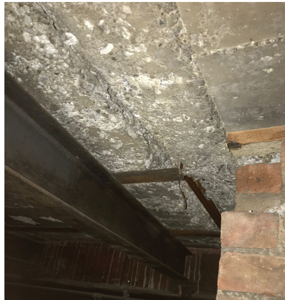
Figure 60. (Upper image) Evidence of leaks, or water pooling as a result of condensation, can be seen on the plywood flooring under several roof vents. (Lower image) A large offset crack exists through the roof deck to the south of the central skylight. This damage to the roof deck appears to have occurred a long time ago. JGWA, 2018.
