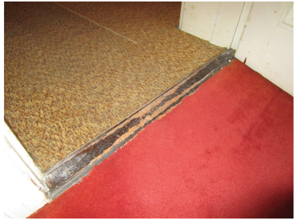
Figure 43. The floors on the third floor have suffered from water and sun-related deterioration, but other conditions have had an impact. Wear and cracking of the floorboards can be seen in several areas, as can patches that were likely necessitated by water damage. The lower image shows a threshold worn to bare wood. This condition will only worsen without a protective coating on the wood. JGWA, 2018.
