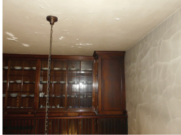
Figure 65. The upper mezzanine level of the Butler's Pantry exhibits several problems that are common to the interior. The soot staining on the east wall of the room serves to highlight the extensive network of hairline cracks through the wall plaster. The ceiling exhibits signs of extensive paint failure. JGWA, 2018.
