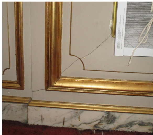
Figure 61. The decorative plaster in the Reception Room (105) was produced off site and installed in panels. In some areas plaster cracking appears at the junction of panels (lower image), while in others a network of apparently random cracking extends through panels (upper image). Conditions like this are common on both the first and second floor levels, and in most locations are little more than hairline cracks. JGWA, 2018.
