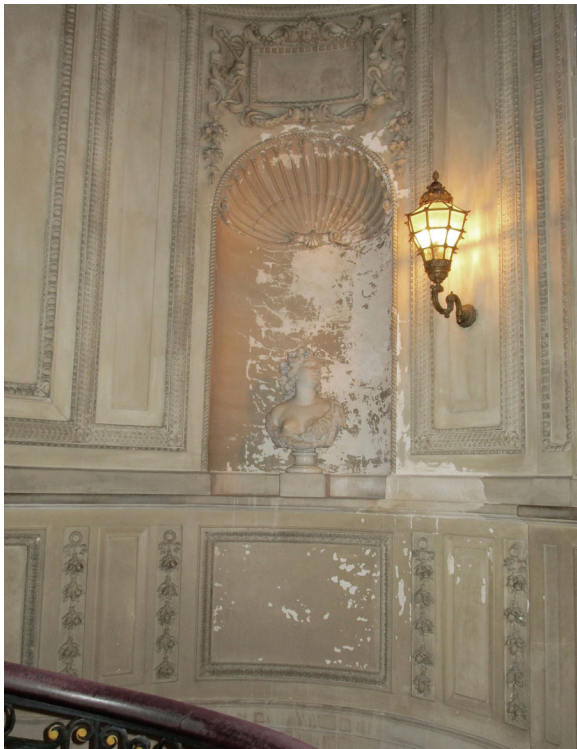
Figure 62. Moisture ingress at the west portico roof level has led to damage around the niche on an intermediate landing of the main staircase. The stone stringers at both of the intermediate landings of the main staircase have cracks through mortar joints or a combination of the joints and adjacent masonry units. JGWA, 2018.
