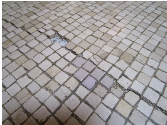
Figure 60. The mosaic floor in the entrance Hall (101) has a network of cracks that extend in a pattern radiating from the center of the room to its perimeter. Loss of original mosaic tiles extends along the largest of these cracks. Replacement materials do not match the original mosaic and are not set flush with the original surface. JGWA, 2018.
