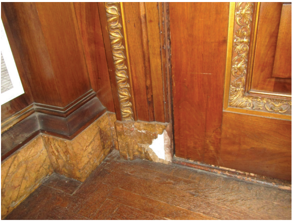
Figure 63. In some of the most formal rooms in the house, marble baseboards exist in conjunction with wood or plaster paneling or trim. Loss of sections of this baseboard can be seen in the Dining Room (lower image), where the underlying plaster can be seen. White plaster can also be seen behind several of the cracked wood panels at the upper level of the Dining Room walls (upper image), and paneled wood ceiling. JGWA, 2018.
