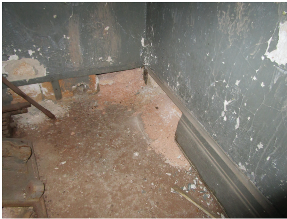
Figure 34. In the upper image, rising damp has severely compromised the terra cotta block wall surrounding the stair to the subbasement. This underlying condition has also adversely effected the paint at the landing level of the stairs, and surface rust covers much of the metal components of the stairs. In the lower image, the terra cotta block wall to the south of Room SB02 is severely compromised by rising damp, and the adjacent wood trim is also deteriorated. JGWA, 2018.
