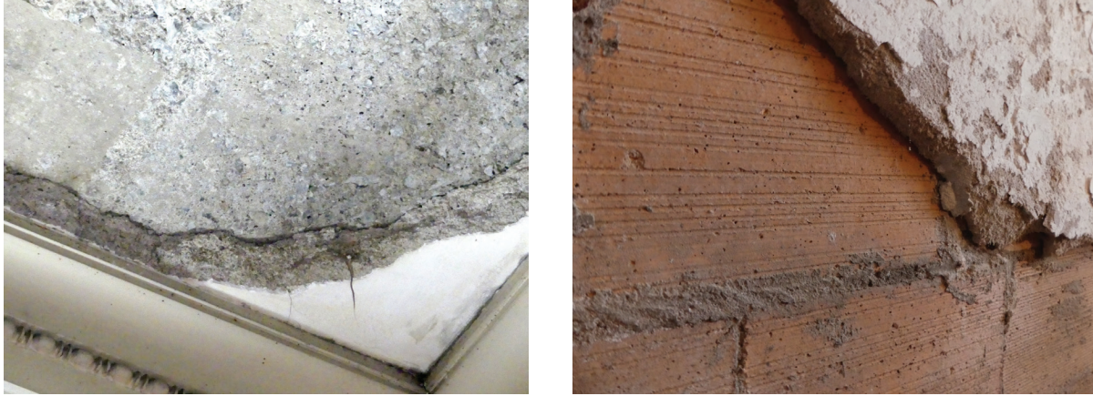
Figure 4. Areas of plaster damage reveal show the plaster layers applied directly to the masonry substrate: in the Empire Room (304) (left), the plaster is applied to the concrete roof slab; and in the Butler's Room (B13) (right), it is applied to the fireproof terra cotta tiles. JGWA, 2018.
