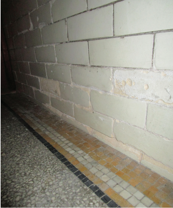
Figure 73. The glazed wall brick at the northeast corner of the Kitchen (B01) is substantially deteriorated as a result of rising damp, which is likely related to heavy salt use on the adjacent paved surface and stairs. JGWA, 2018.
