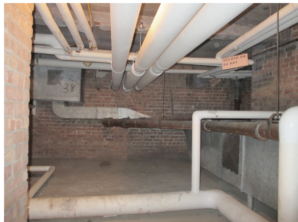
Figure 30. In SB10 (upper image), the east area of the elliptical section, the telephone panel for Franklin D. Roosevelt's World War II switchboard remains on the west wall; view of SB11, looking south (lower image). JGWA, 2017.
