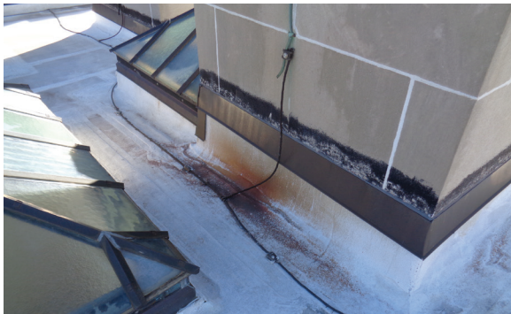
Figure 19. Given the recent extensive exterior restoration, most of the remaining problem conditions are at the roof, and in particular are related to the various roof penetrations such as skylights and vents (upper image). In the lower image, there is tar residue on the chimney stone. JGWA, 2018.
