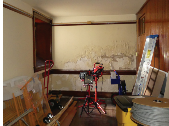
Figure 77. Plaster failure covers the entire lower half of the west wall of room B11. This extensive moisture-based deterioration is immediately adjacent to the south stair of the west portico. The recent repairs to this stair, and elimination of open mortar joint, has corrected the moisture ingress problem. JGWA, 2018.
