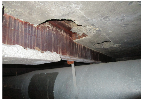
Figure 35. (Upper image) Evidence of moisture in the sub-basement can be seen on perimeter walls, where efflorescence and related mortar and brick deterioration are present, and in the center of the floors in some rooms. Evidence of standing water at low points in the floor (center image) are often accompanied by salt deposits around their perimeter. Rising damp can be seen at the base of some of the central piers.
