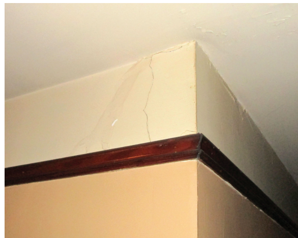
Figure 75. Paint and plaster deterioration can be seen on the perimeter of the basement level where site water has soaked through the foundation in some locations, but paint and plaster problems can also be seen on the walls of the interior corridor (B08). The paint and finish coat of plaster deterioration seen in the upper image are prevalent problems at the basement level. A substantial offset crack in the South Hall, adjacent to the northwest corner of the laundry room drying racks, was successfully patched at some point in the past (lower image). JGWA, 2018.
