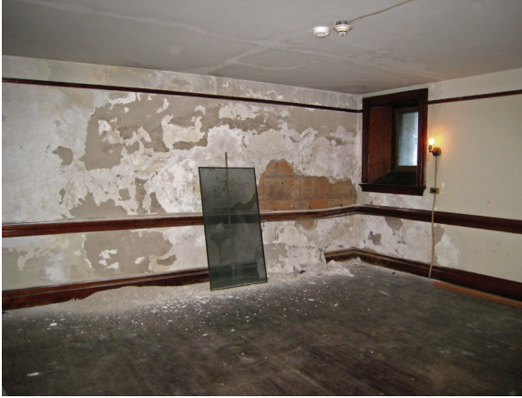
Figure 76. Extensive plaster damage extends along the east and north walls of the Chef's Room. The chair rail on the west wall is buckling, and the baseboard is pulling off of the wall. The recent exterior restoration eliminated the water infiltration that caused the damage. JGWA, 2017.
