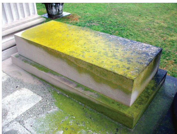
Figure 20. One of the primary issues with the stone was staining from several types of biological growth. JGWA, 2010.
