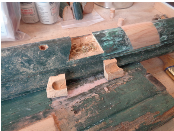
Figure 35. (Upper image) The woodwork was damaged from insects and woodpeckers. (Center and bottom image) Mock-up to develop techniques for dutchman repair on the windows' wood brick molds. Brick mold this damaged was typically replaced. JGWA, 2017.
