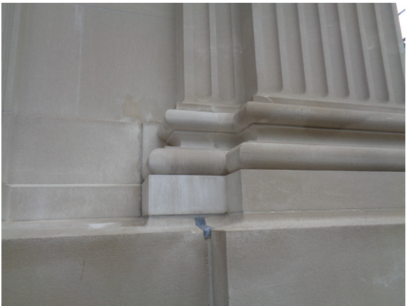
Figure 37. Example of a carved stone dutchman repair. The bottom image also shows one of the lead tee caps that replaced sealant on the skyward joints of the water table and belt course. JGWA, 2017.
