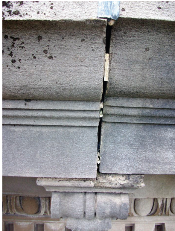
Figure 23. The corner stones in the north and south portico cornices were displaced and rotating out. JGWA, 2010.
