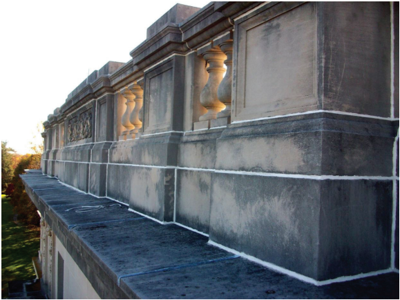
Figure 22. (Upper image) The original mortar joints are very thin; the original workmanship was meticulous and difficult to replicate. (Lower image) Repointed mortar joints on the balustrade did not match the original. JGWA, 2010.
