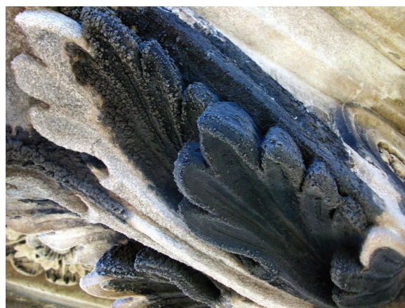
Figure 21. Stone deterioration was also attributed to gypsum crust. On the left, the window lintel is stained with biological growth and damaged by gypsum crust; below, gypsum crust has developed on one of the modillions. JGWA, 2010.
