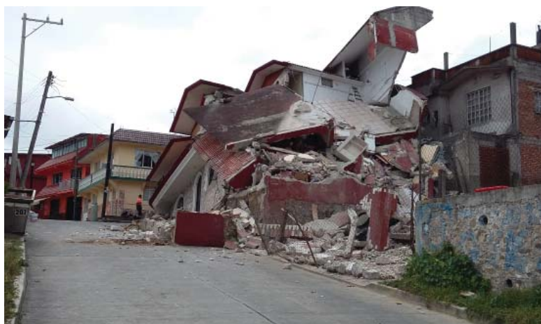
Teziutlán. Collapse of a house triggered by intense rainfall. The house was located on a drainage area! Took place in August 10th, 2015. Photo: Rubén Acebo-Zárate.
