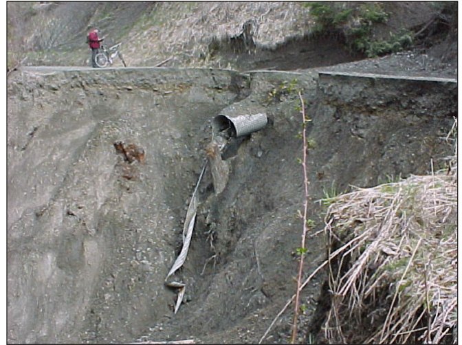
Increased flooding would affect water quality, fisheries, and recreation. It would also require road and drainage infrastructures that can handle increased flows.
