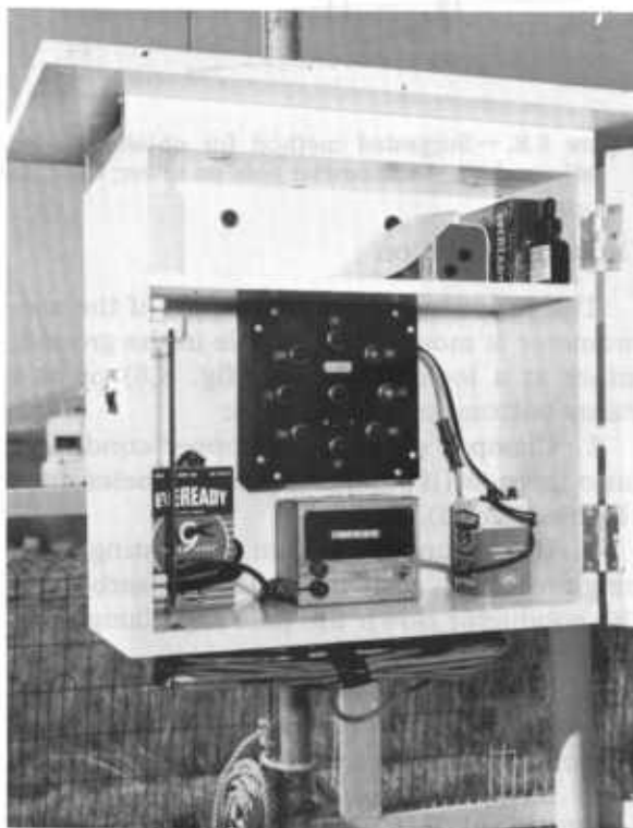
Figure 8.11. — A small accessory cabinet for installation of wind counter and wind direction readout device. The upper part of the cabinet can be used for tools and supplies.
