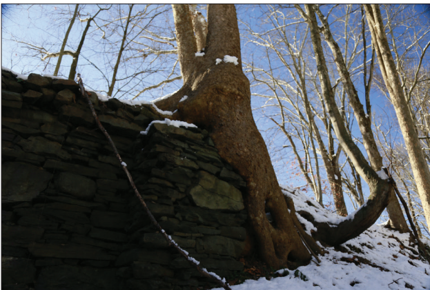
Figure 3.3e. View of a mature tree anchored in the canal wall. (OCLP 2022, IMG_1878)
