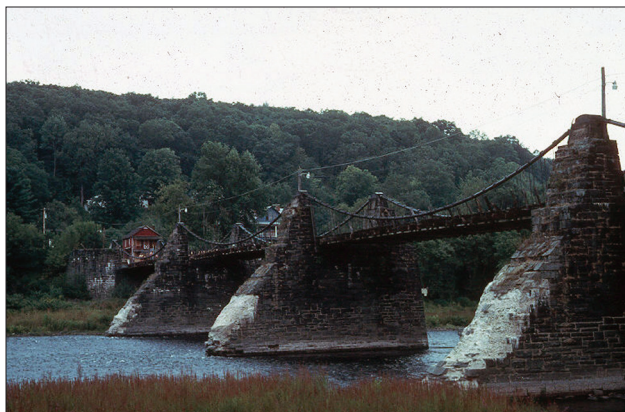
Figure 1.62. View looking southeast at the deteriorated aqueduct/bridge, 1980. (National Park Service, Photo Gallery, "48 Roebling Aqueduct in 1980." From https://www.nps.gov/media/photo/gallery-item )
