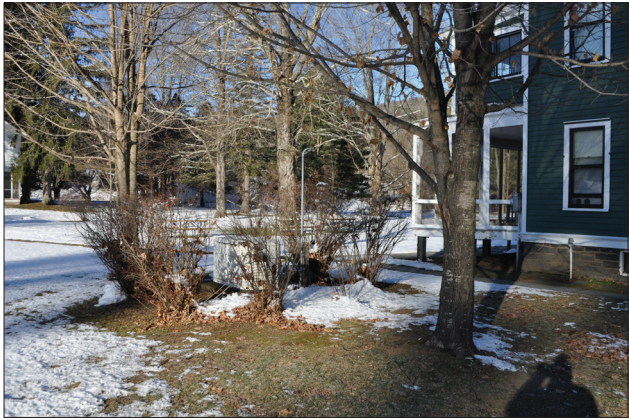
Figure 2.58. View looking northwest at the generator. (OCLP 2022, DSC_7381)
