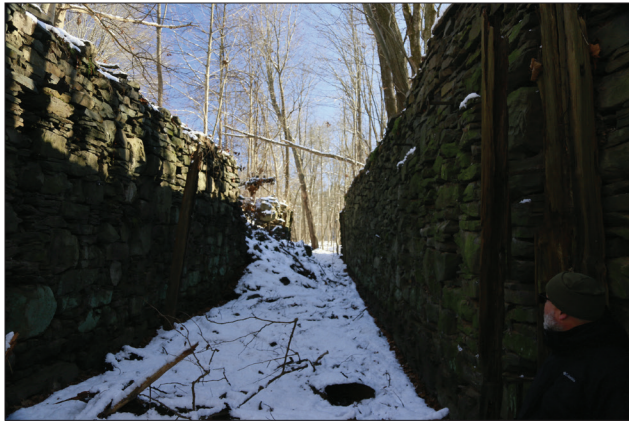
Figure 2.11. A section of Lock 71 has collapsed due to stormwater associated with a culvert on State Highway 97. (OCLP 2022, IMG_1877)
