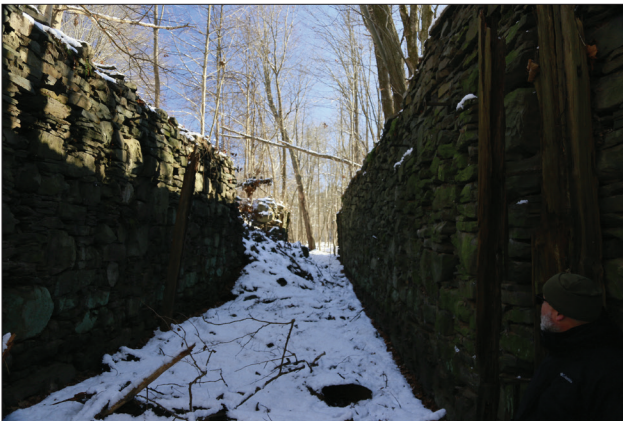
Figure 3.3d. View looking southeast from the interior of Lock 71. Note the collapsed section of the lock wall (image left). (OCLP 2022, IMG_1877)
