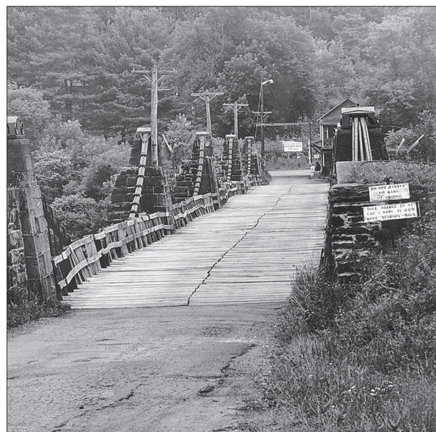
Figure 1.53. View looking east at the aqueduct/bridge, c.1969. The structure’s decking and railings are in poor condition. (Historic American Engineering Record, HAER PA-1, 1969, #140679pv)
