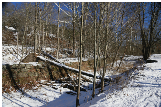
Figure 3.1d. View looking east at canal prism wall damage from a fallen tree. (OCLP 2022, IMG_1856)
