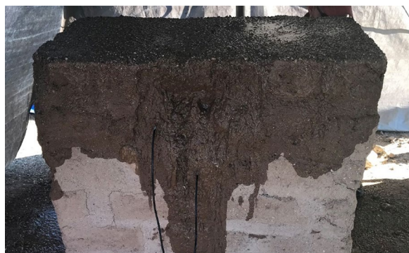
Fig. 8 Wall S with erosion near the EC-5 sensor
