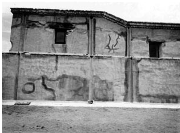
West wall of nave/sanctuary exterior in 1972. Note the jigsaw like appearance.
