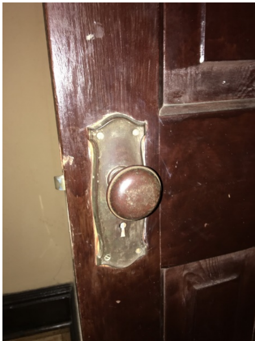
FIGURE 158. Worn finish on latch set.
