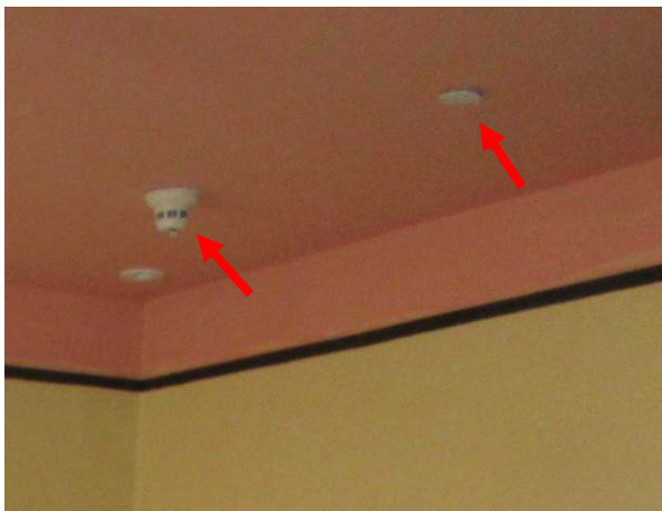
FIGURE 204. Typical smoke and fire detector (left) and concealed sprinkler head (right).
