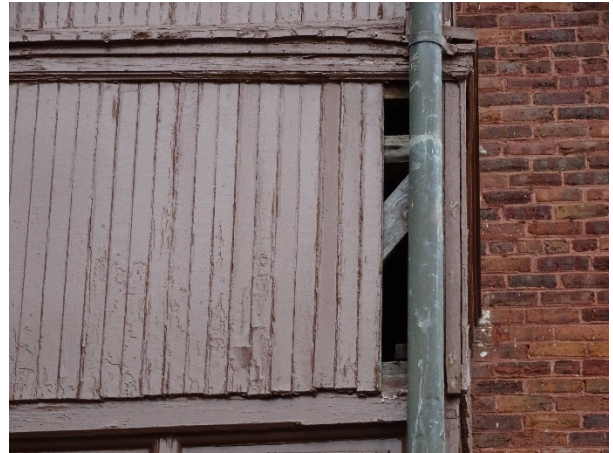
FIGURE 106. Missing wood cladding at south two-story porch.
