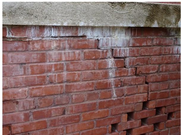
FIGURE 86. Step cracking and efflorescence at the porch walls.
