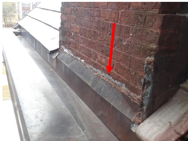
FIGURE 129. Deteriorated sealant at regletted flashing joint.
