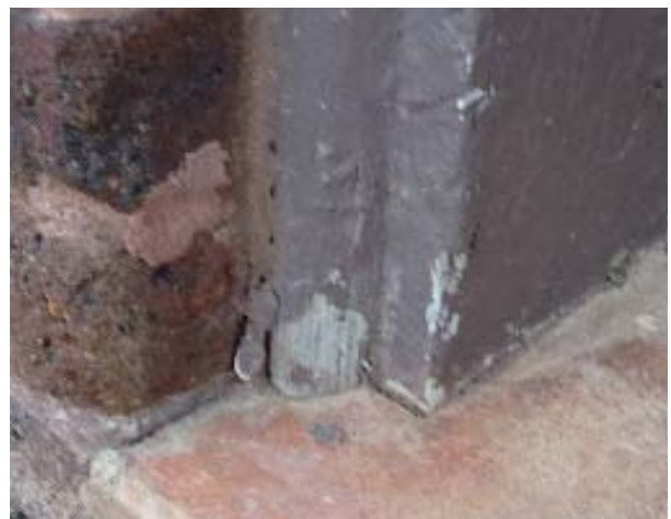
FIGURE 108. Peeling paint at door and window framing members.
