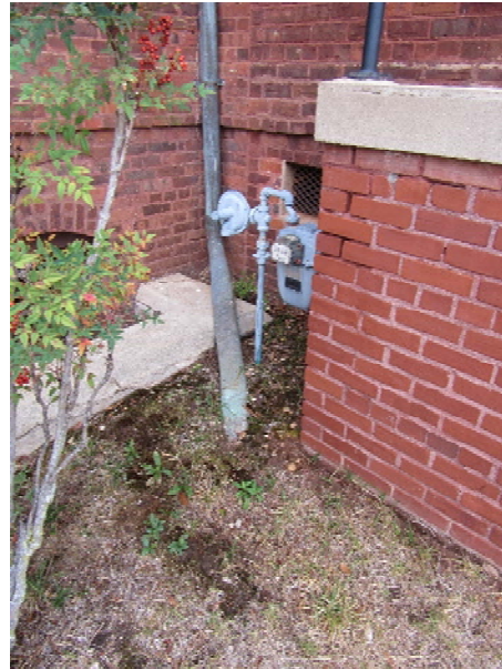
FIGURE 37. Gas meter in front of the south elevation of the dining room addition.
