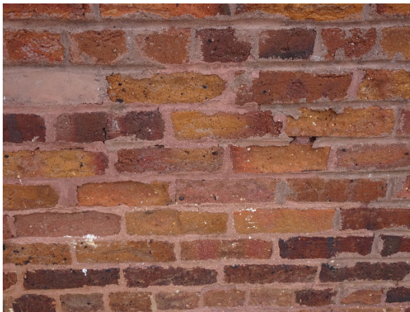
FIGURE 88. Face spalling of brick.
