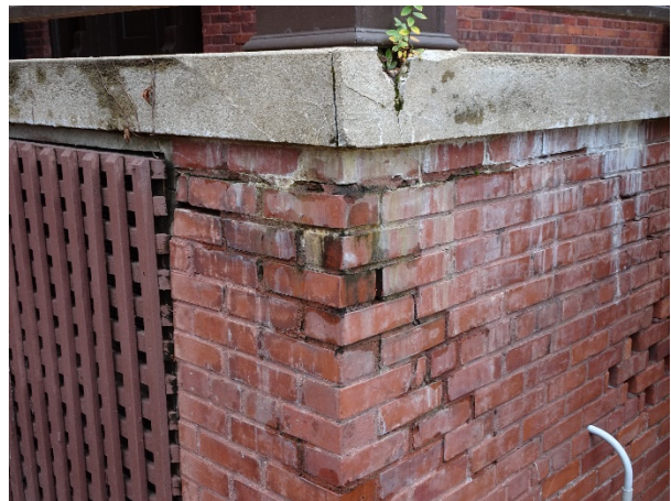
FIGURE 85. Step cracking, open joints, and evidence of water infiltration at the porch walls.
