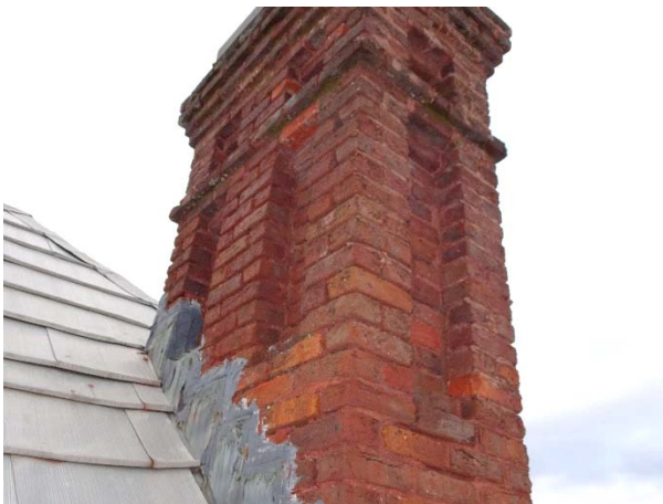
FIGURE 83. Deteriorated mortar joints and evidence of previous repointing efforts visible at the chimney.
