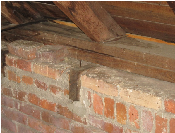
FIGURE 234. Typical wood kicker found in the attic of the south wing.
