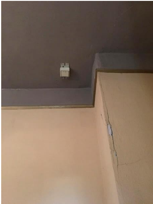
FIGURE 135. Detail of plaster cracking.
