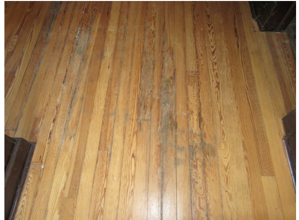
FIGURE 197. Third-floor hall – discoloration from moisture on wood-strip flooring.
