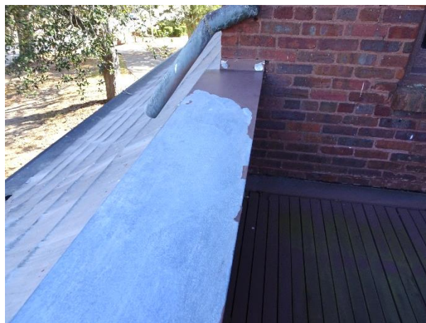
FIGURE 112. Peeling paint at the sheet-metal flashing at second-floor balcony.
