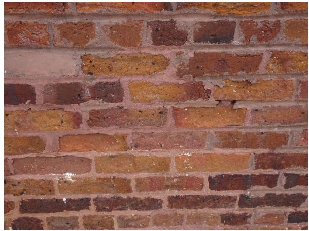
FIGURE 84. Evidence of previous mortar repointing in the field of the wall.
