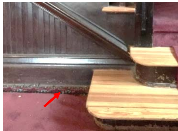
FIGURE 215. Common damage to woodwork and trim.
