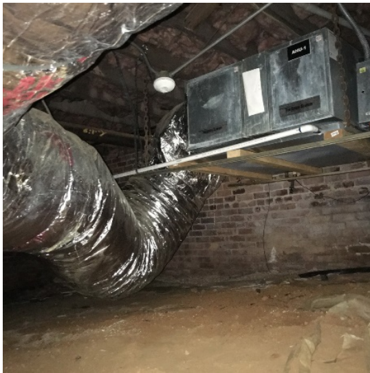
FIGURE 220. Air-handling unit in crawl space.
