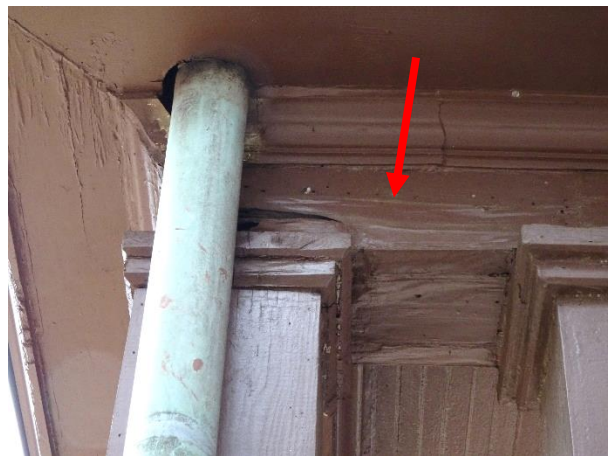
FIGURE 101. Blistering paint at wood porch members.
