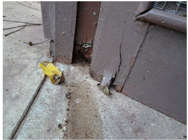
FIGURE 115. Deteriorated wood door sash.
