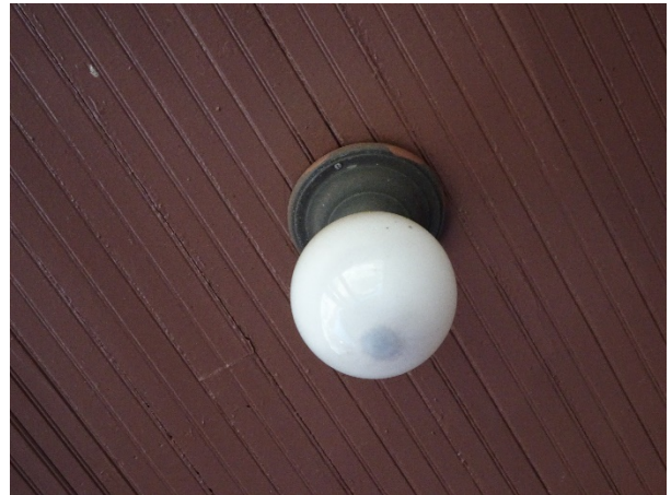
FIGURE 55. Light fixture on ceiling of the recessed porch.
