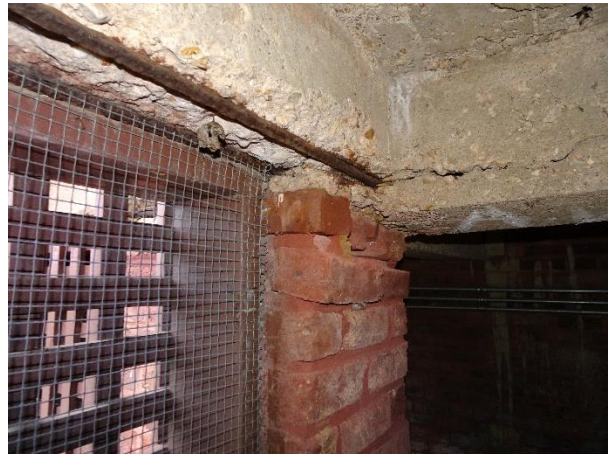
FIGURE 94. Spalled concrete bond beam at porch wall.
