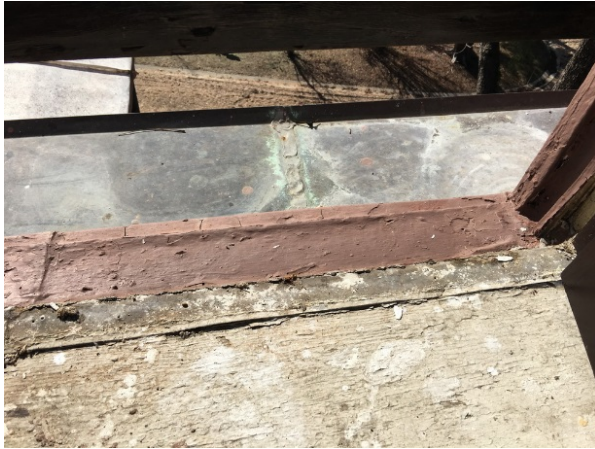
FIGURE 216. Third-floor bathroom – severely deteriorated window and wood sill.
