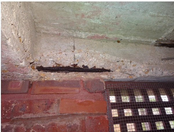
FIGURE 92. Spalled concrete bond beam at porch wall.
