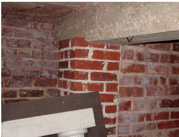
FIGURE 229. Brick support pier and concrete beam at porch foundation.
