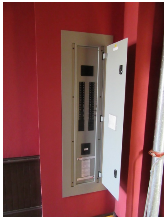
FIGURE 224. Electrical sub-panel at west bedroom.
