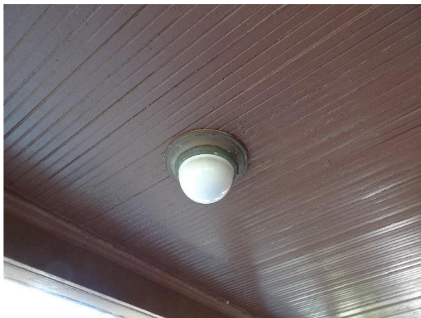
FIGURE 50. Typical porch ceiling light fixture.
