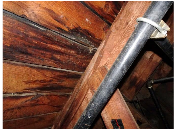
FIGURE 126. Moisture staining at wood sheathing.
