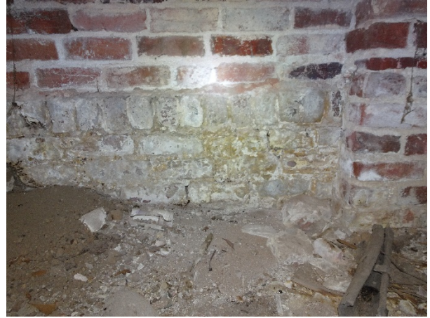
FIGURE 89. Accumulation of efflorescence at base courses of porch walls.
