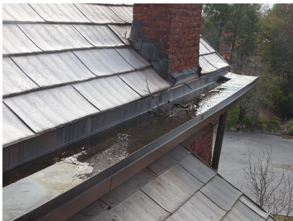
FIGURE 119. Gutter overflowing with water. Note branches in the gutter.
