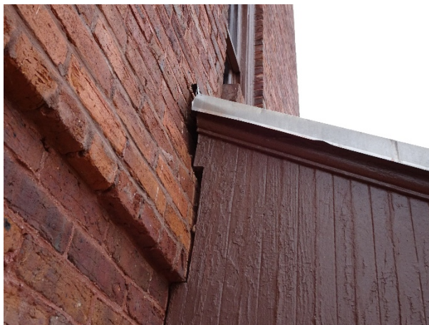
FIGURE 109. Displaced roof framing over south entrance.
