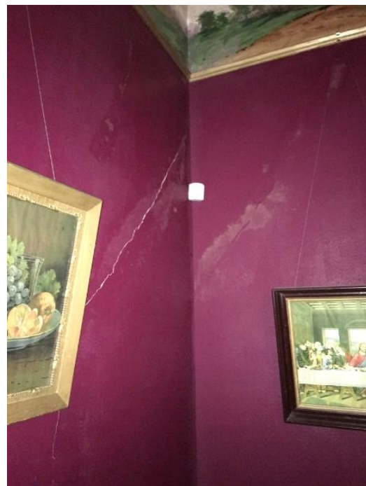
FIGURE 134. Detail of plaster cracking.
