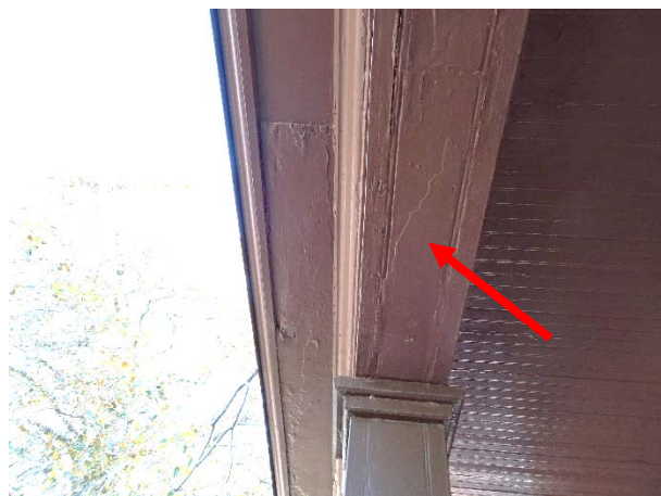
FIGURE 102. Previous paint coatings at wood porch members were not completely removed prior to repainting.
