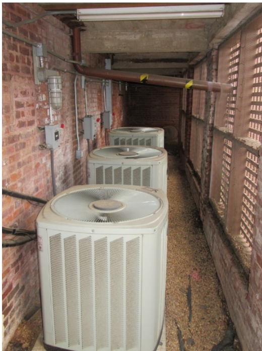
FIGURE 221. Condensing units at porch crawl space.
