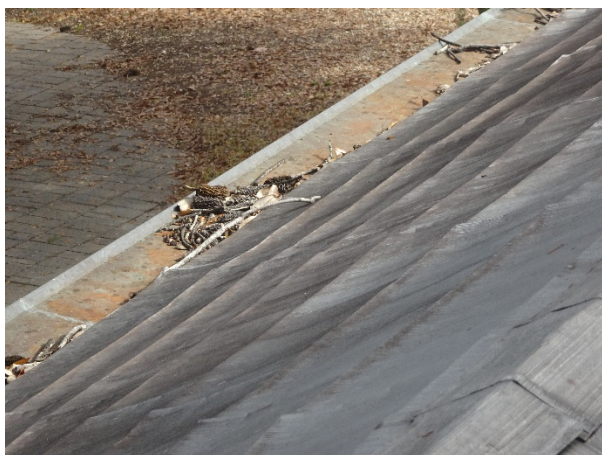
FIGURE 118. Debris and organic matter at gutter.
