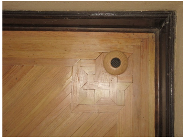
FIGURE 218. Typical Unico distribution nozzle in the parquet floor.
