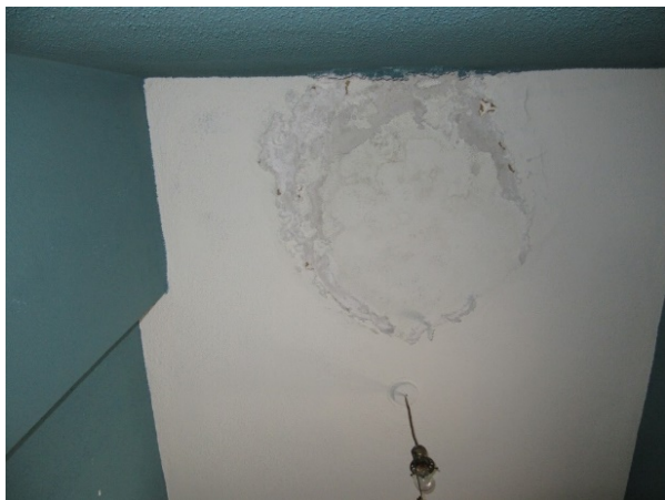
FIGURE 178. Plaster damage at ceiling of Portia's shower room.
