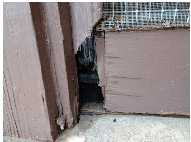
FIGURE 116. Severely deteriorated wood door sash.
