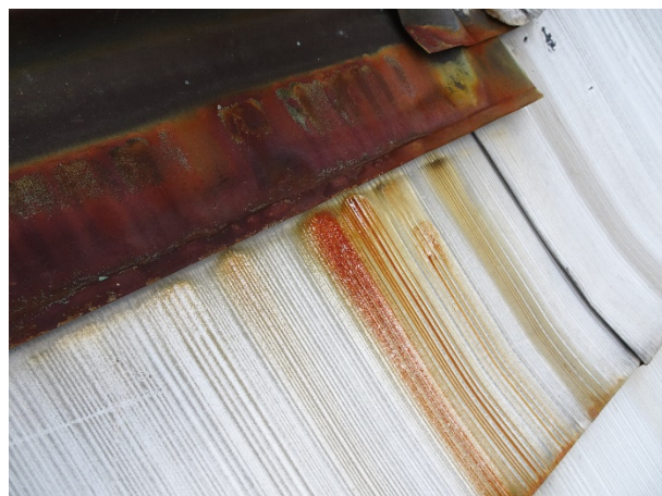
FIGURE 130. Corrosion staining at interface of flashing with roof cladding.
