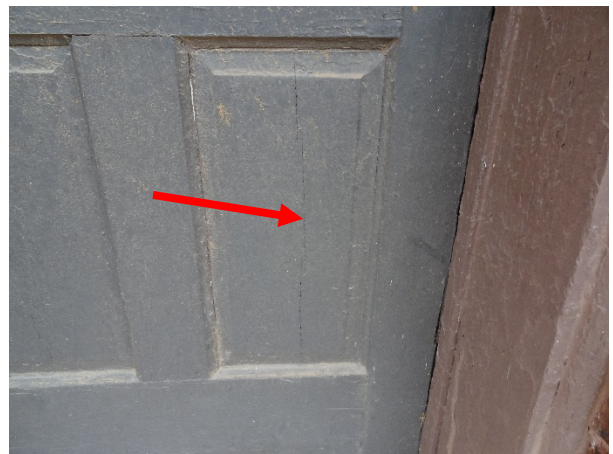
FIGURE 107. Vertical crack in recessed panel.
