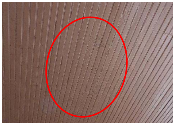
FIGURE 103. Dark spots of biological growth on face of ceiling boards at porch.
