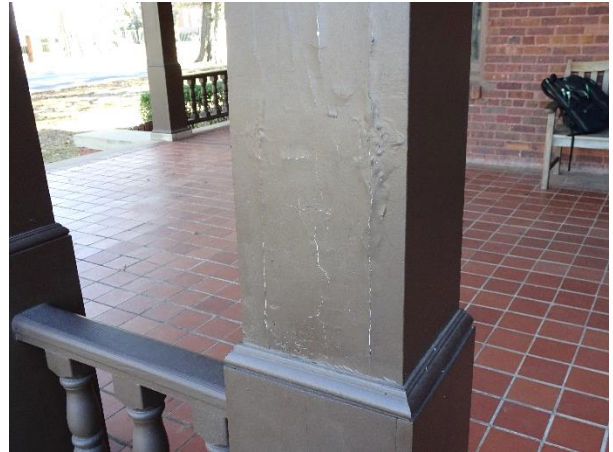
FIGURE 98. Debonded paint and plaster coating at columns.
