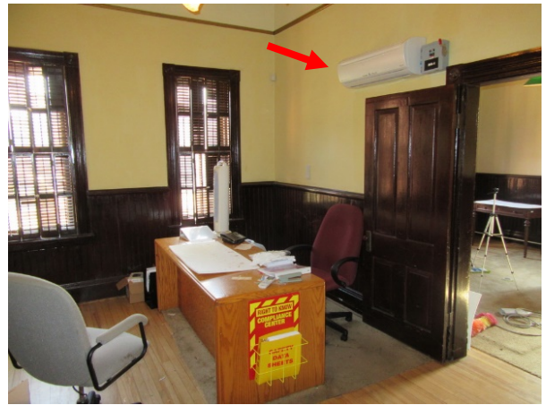
FIGURE 222. Wall-mounted VRF unit in the breakfast room.
