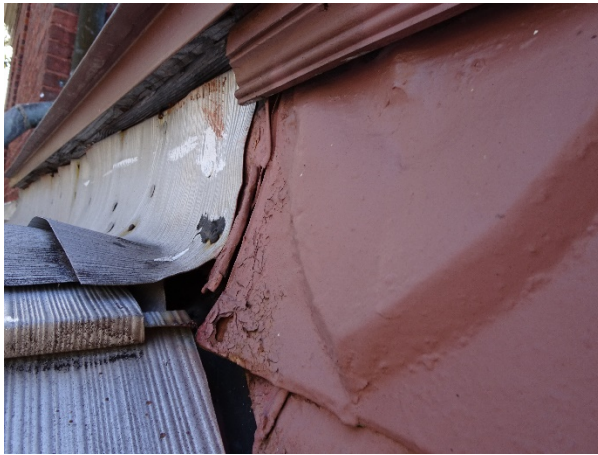
FIGURE 123. Gap at interface between the sheet-metal roof and wall cladding.
