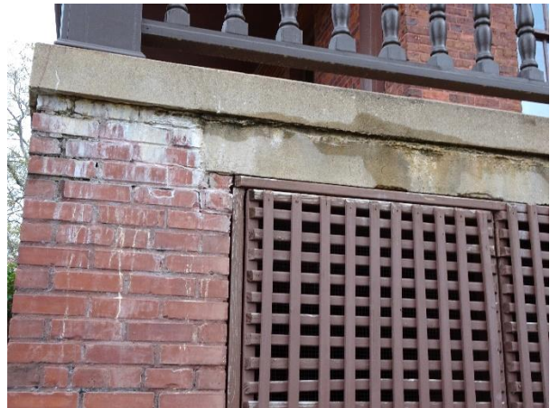
FIGURE 95. Moisture staining and evidence of moisture infiltration at concrete bond beam.
