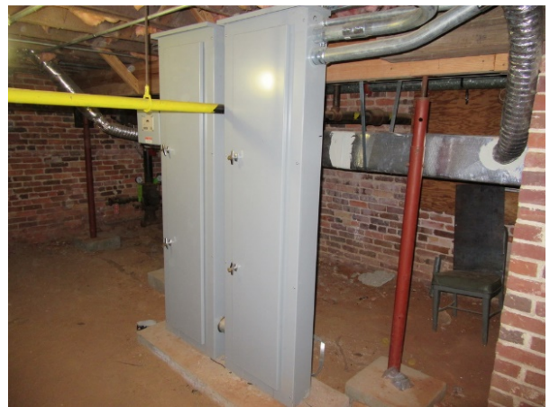
FIGURE 223. Electrical panels in the crawl space.
