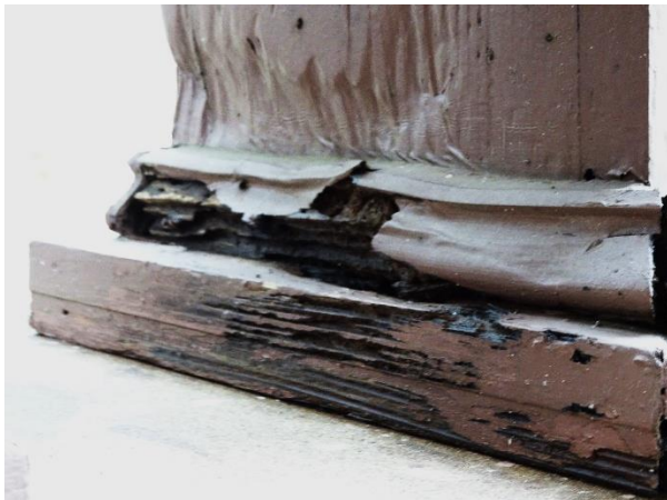
FIGURE 97. Deteriorated wood at base of columns.
