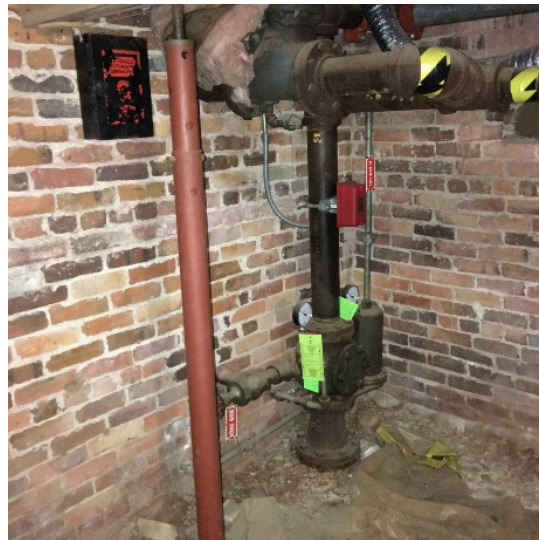
FIGURE 226. Fire sprinkler standpipe in basement.
