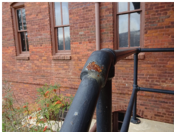
FIGURE 111. Surface corrosion and paint loss at metal handrail.
