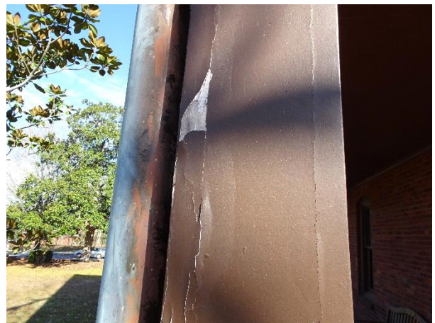
FIGURE 99. Cracking and flaking paint at columns.
