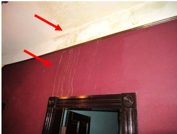
FIGURE 170. Plaster damage from water in second-floor front hall.
