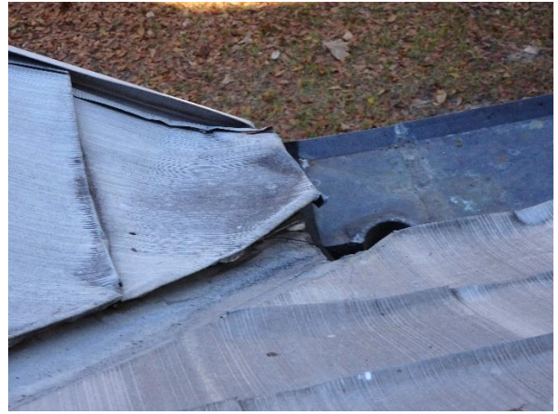
FIGURE 124. Damaged sheet-metal roof cladding near the gutter.
