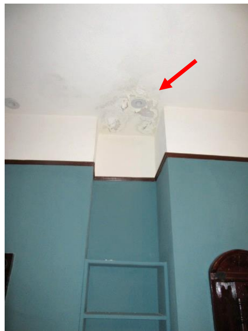
FIGURE 177. Plaster degradation and water damage at ceiling, Margaret Washington's bedroom.
