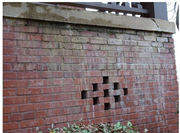
FIGURE 90. Moisture staining at porch walls.
