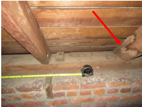
FIGURE 127. Moisture staining at roof rafters.
