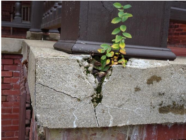
FIGURE 96. Spalling and cracking of concrete at northwest corner of porch.
