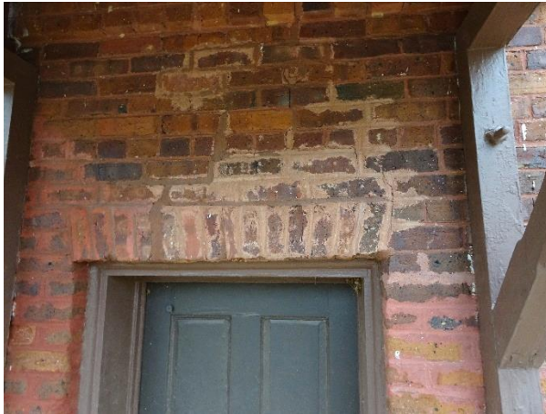
FIGURE 87. Cracking and open mortar joints above flat arch opening.
