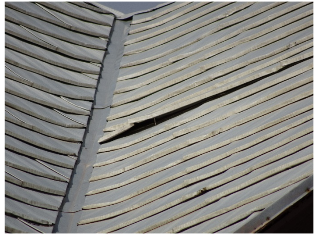
FIGURE 125. Bowed and displaced sheet metal at field of roof.
