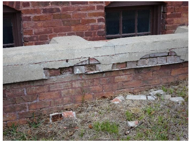
FIGURE 81. Spalling of the brick and cementitious parge coating at the light well walls.
