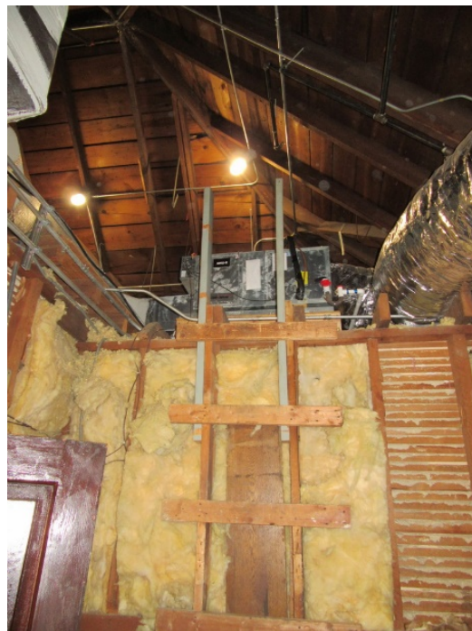
Figure 219. Air-handling unit in the attic.
