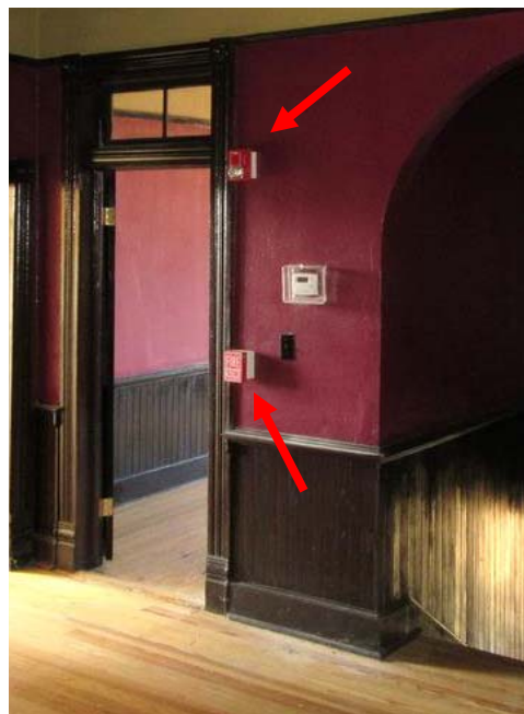
FIGURE 227. Typical alarm pull-station (bottom) and strobe (top).
