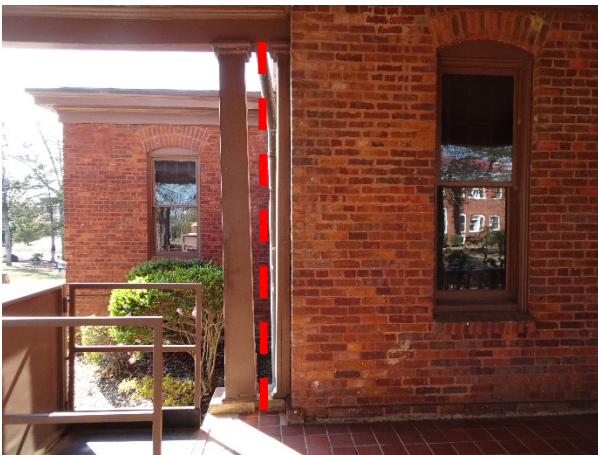
FIGURE 105. Tilted and displaced porch column.
