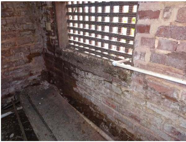
FIGURE 91. Evidence of moisture infiltration at northwest corner of porch.
