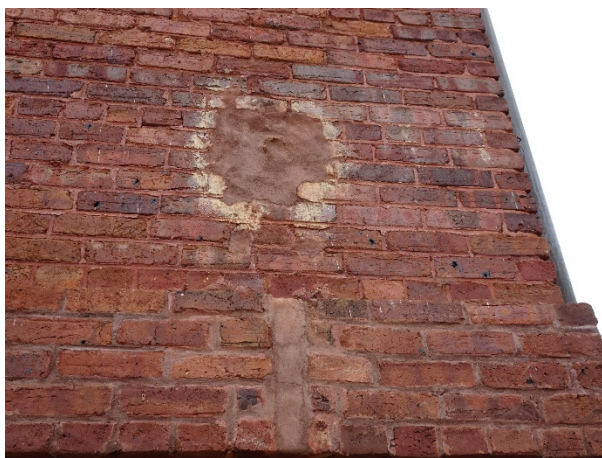
FIGURE 110. Previous cementitious patch repair at abandoned utility openings.
