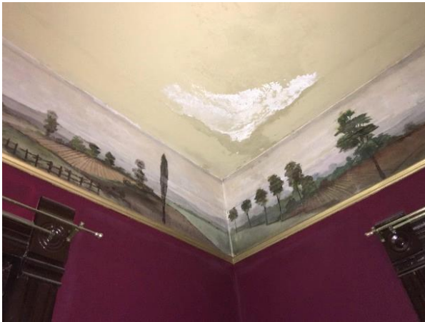
FIGURE 139. Water damage at ceiling.
