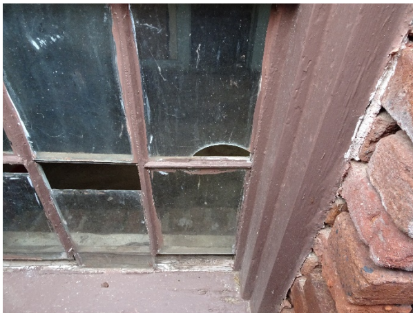
FIGURE 114. Broken and displaced glass at basement windows.
