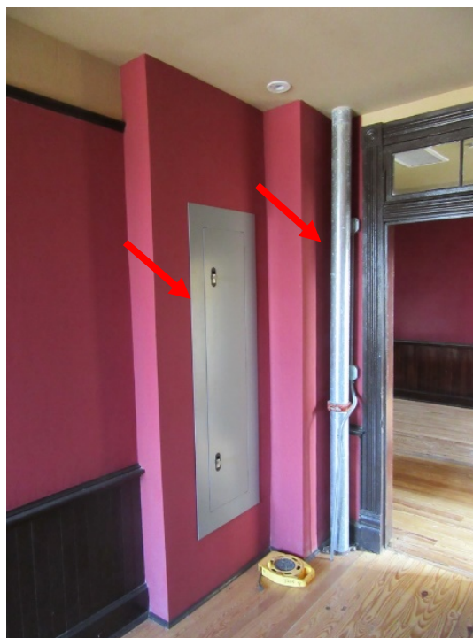
FIGURE 202. Electrical panel and sprinkler standpipe at west bedroom.
