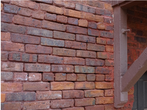
FIGURE 82. Eroded mortar joints at the field of the wall.
