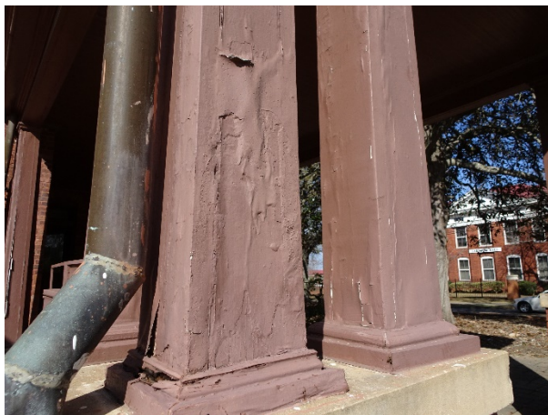
FIGURE 100. Deteriorated paint and underlying plaster coating at columns.
