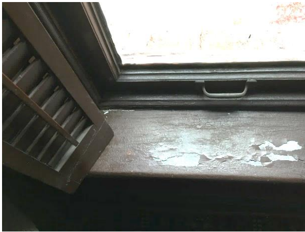
FIGURE 217. Dining room extension – blistering and peeling paint on the window sill.
