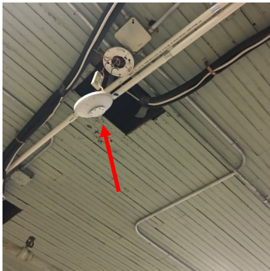
FIGURE 225. Disconnected smoke and fire detectors in basement.
