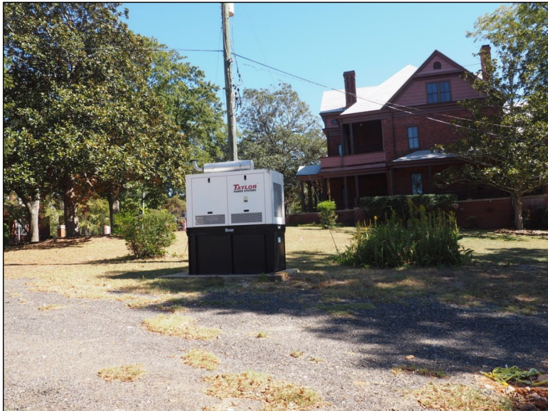
Fig 8-22. Power generator, photo by author
