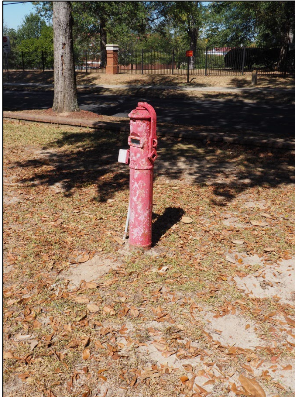
Fig 8-31. Post indicator valve, photo by author
