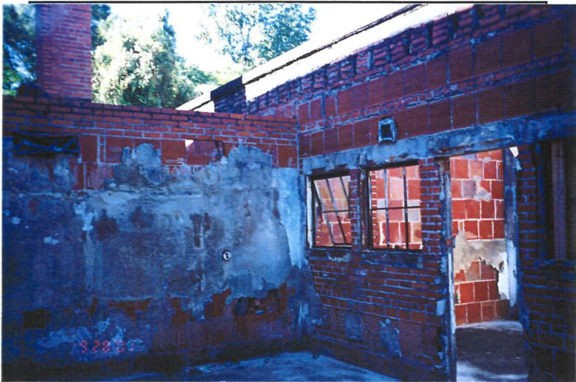
Photo 10. Hangar No. 1, Interior – Parge coat mortar observed on structural clay tile and masonry surfaces.
