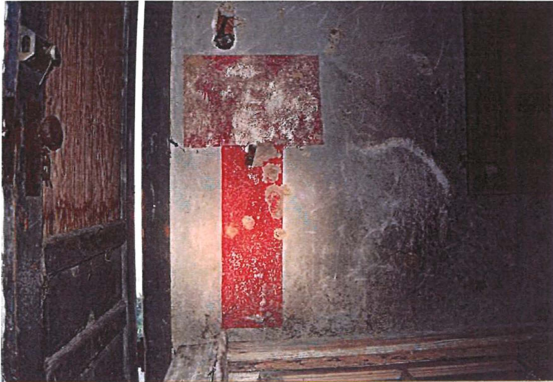
Figure 13: Evidence of fire safety system on the north interior wall of the heater room.
