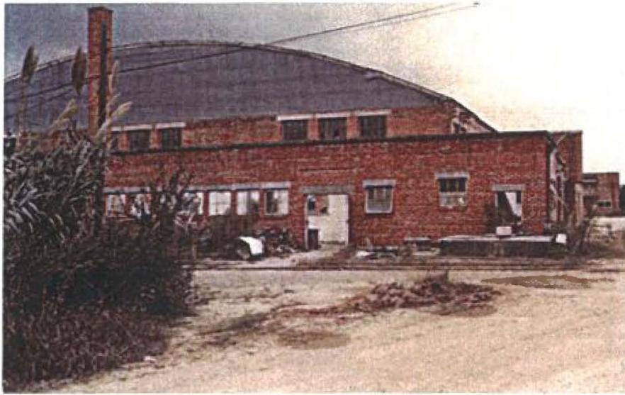
Figure 22: Post-War Deterioration of Hangars and Landscape. From Booker Conley's Photograph Collection.
