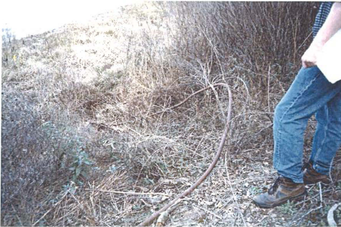
Figure 53: Exposed Water Pipe on slope.
