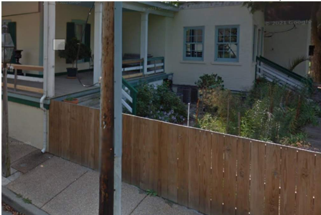
Figure 300.. Older air-cooled condensing units which resided at the north side of the house. (Source: Google Street View, 2013)
