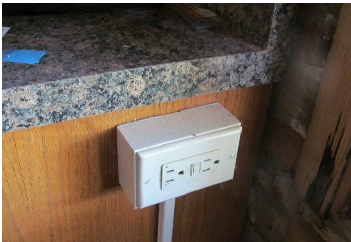
Figure 366. Double-duplex, GFCI receptacle in kitchen on first floor. (Source: Alvine, 2022)
