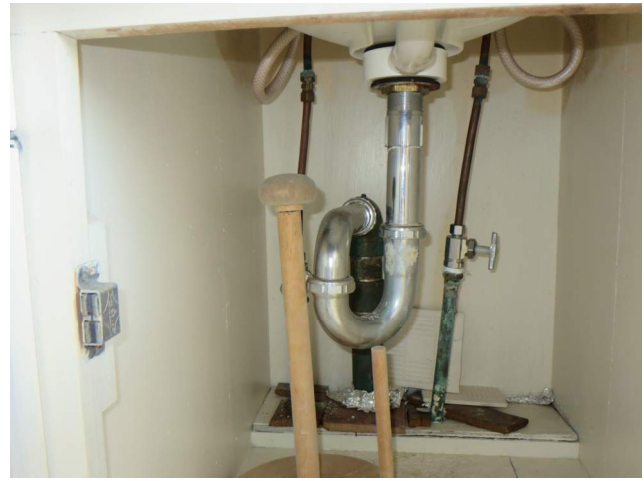
Figure 280. Existing copper water piping below restroom cabinet serving lavatory. (Source: Alvine, 2022)
