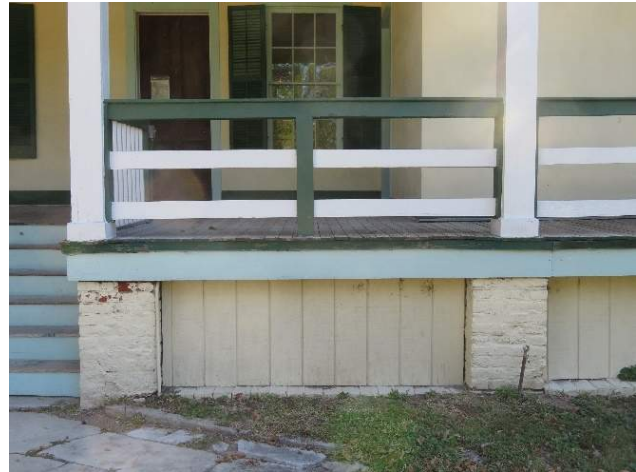
Figure 86. Exterior Panelboard Covering Basement Windows (Source: RRJ, 2022)
