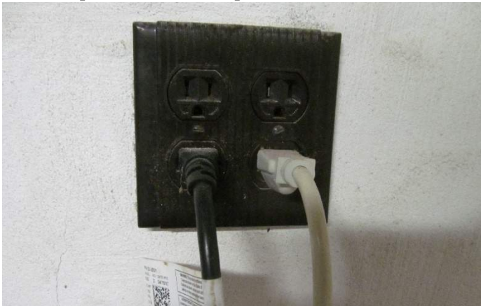
Figure 364. Double-duplex, grounded, 120-volt receptacles northwest storage room in basement. (Source: Alvine, 2022)
