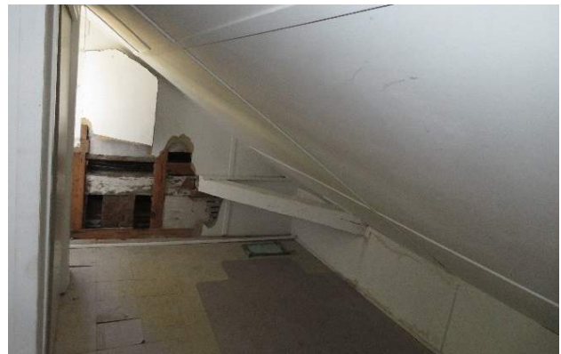
Figure 242. Overview of Room 208 facing north showing failed flooring and water staining. (Source: RRJ, 2022)
