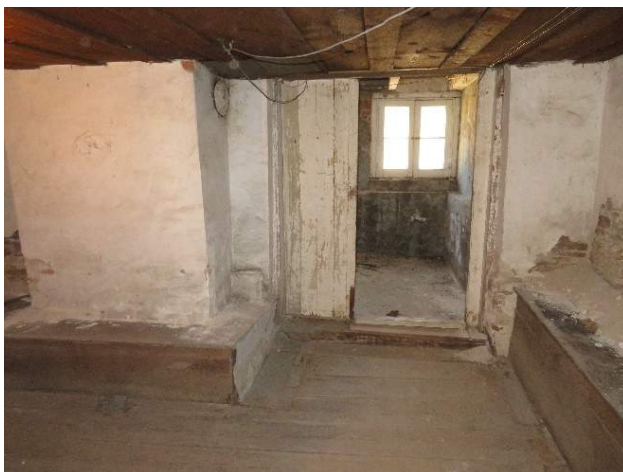
Figure 250. Door D010 has been removed since 1985 HABS documentation. (Source: RRJ, 2022)
