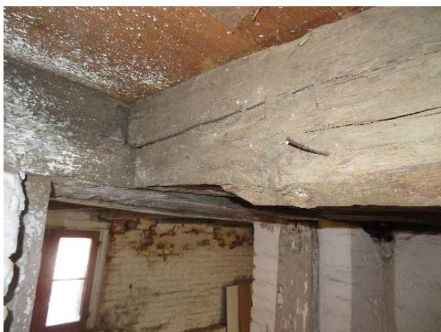
Figure 162. Split joist at southeast. (Source: RRJ, 2022).
