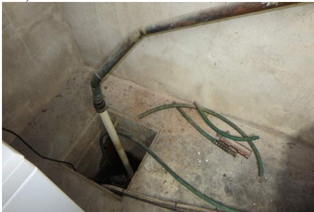
Figure 296. The sump pump has a PVC discharge pipe which is connected to copper DWV piping. (Source: Alvine, 2022)
