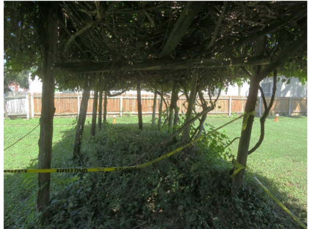
Figure 52. North end of grape arbor exhibiting failed members (Source: RRJ, 2022).
