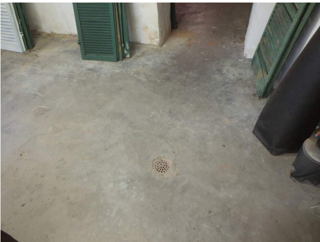
Figure 277. Existing floor drain in the far southwest room of the basement level. The drain grate appears to be dirty and partially clogged with debris. (Source: Alvine, 2022)
