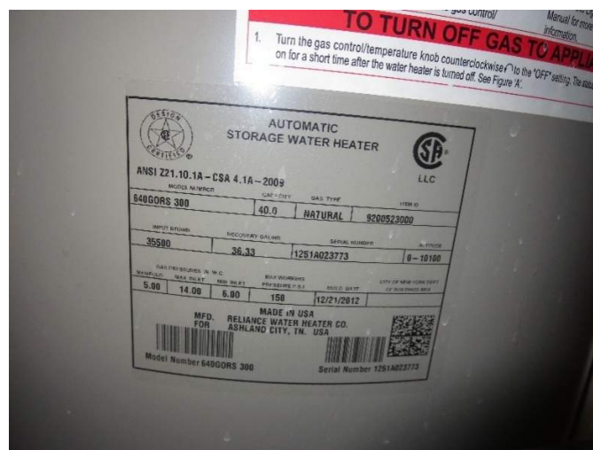
Figure 283. The water heater has a 40-gallon storage capacity and 36.33 GPH recovery. (Source: Alvine, 2022)
