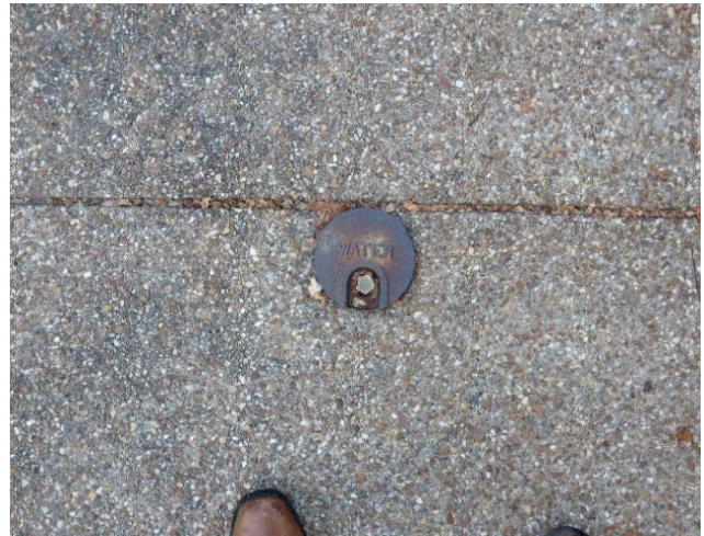
Figure 259. Existing water stop valve in sidewalk south of property with the water service originating at Market Street. (Source: Alvine, 2022)
