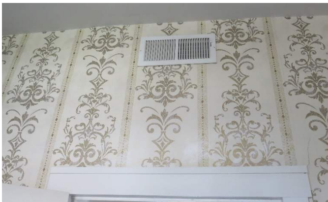
Figure 327. Typical sidewall supply air registers located up high on the walls of the second level rooms. (Source: Alvine, 2022)
