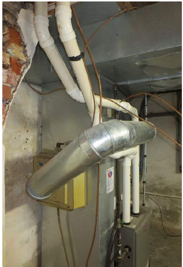
Figure 305. Existing flue and combustion air PVC piping routing through basement level from northwest furnace. (Source: Alvine, 2022)
