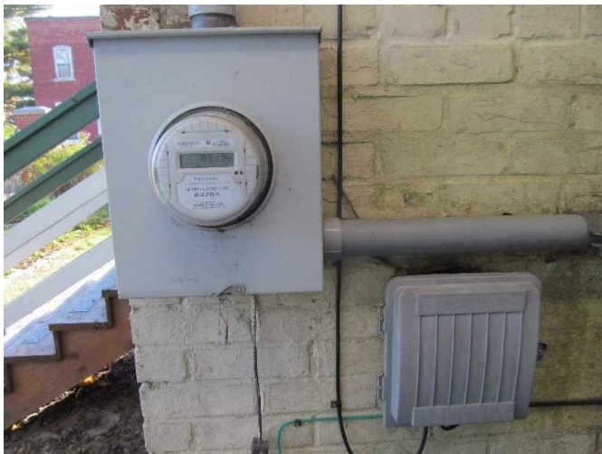
Figure 340. 200-amp, 240/120-volt, single-phase meter socket on left side; telephone cable termination box on right side. (Source: Alvine, 2022)
