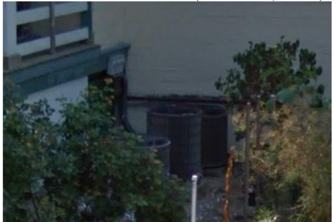
Figure 301. Close-up view of older air-cooled condensing units which resided at the north side of the house. (Source: Google Street View, 2013)
