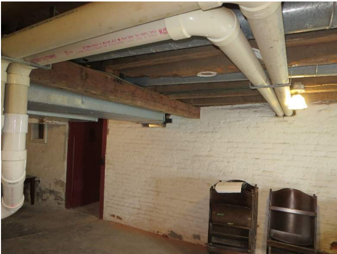
Figure 304. Existing flue and combustion air PVC piping routing through basement level from central furnace. (Source: Alvine, 2022)
