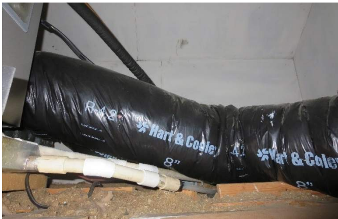
Figure 325. Typical insulated flexible supply air ductwork located up above the ceiling within the attic serving sidewall supply air registers at the Second level spaces. (Source: Alvine, 2022)
