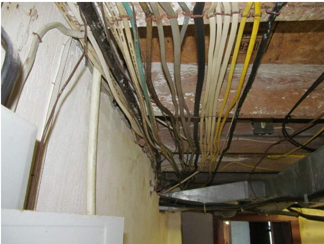
Figure 348. Branch circuit, non-metallic sheathed (NM) cable routed horizontally along basement ceiling. (Source: Alvine, 2022)
