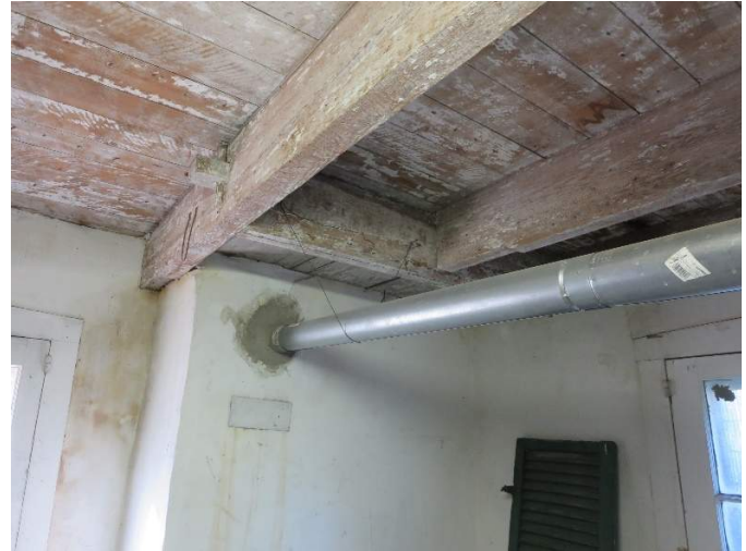
Figure 285. The water heater flue continues to the south where it connects to an existing chimney. (Source: Alvine, 2022)
