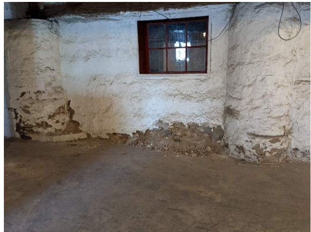
Figure 191. Moisture related masonry decay at basement foundation between Rooms 005 and 009. (Source: RRJ, 2022).
