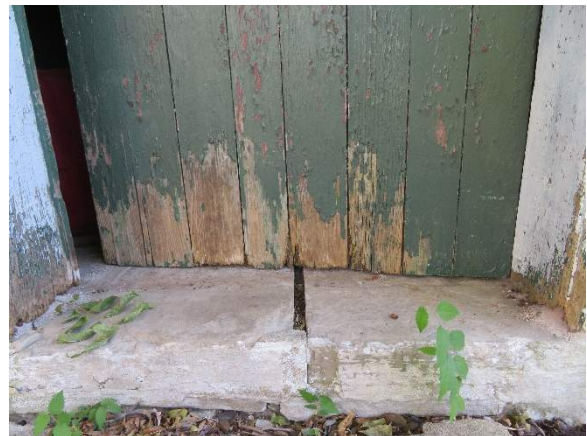
Figure 111. Weathered paint and wood at base of Door D110. (Source: RRJ, 2022)
