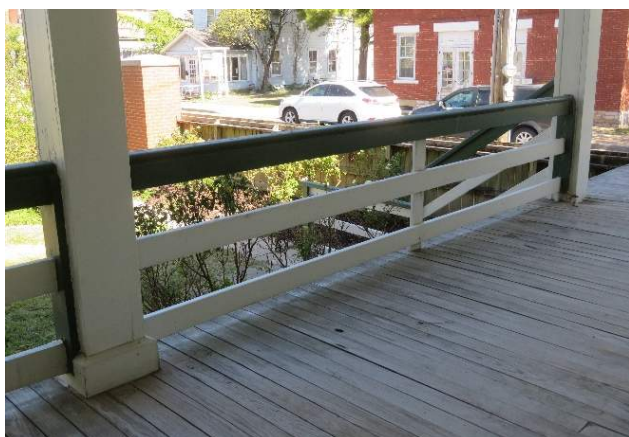
Figure 119. Typical gallery handrails which do not comply with IBC safety provisions (Source: : RRJ, 2022)
