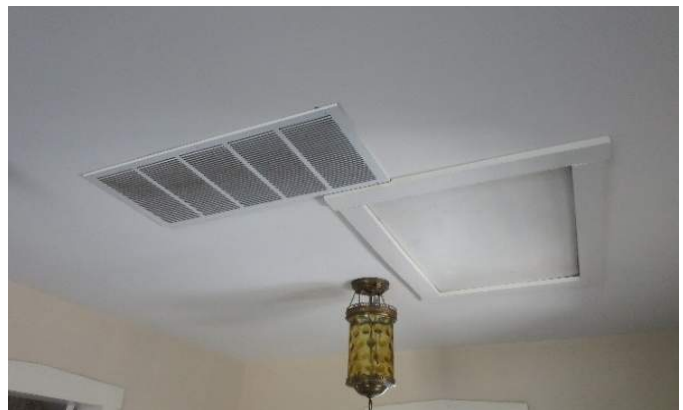
Figure 328. Central ceiling-located return air grille serving second level located adjacent to the attic equipment access hatch. (Source: Alvine, 2022)
