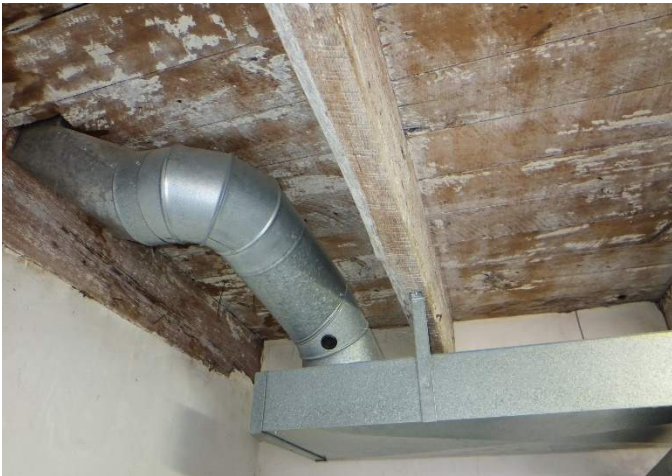
Figure 322. Typical supply air ductwork located at the basement level which serves the First level spaces. (Source: Alvine, 2022)
