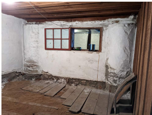
Figure 131. Overview of missing floor planking and remaining sleepers within Room 009 (Source: RRJ, 2022)
