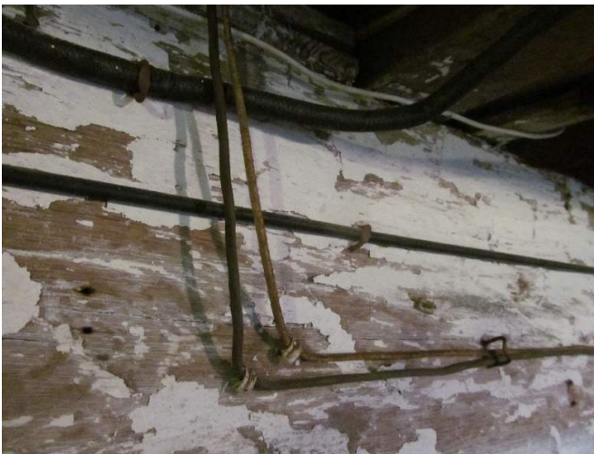
Figure 351. An older, cloth-covered cable in the basement. (Source: Alvine, 2022)
