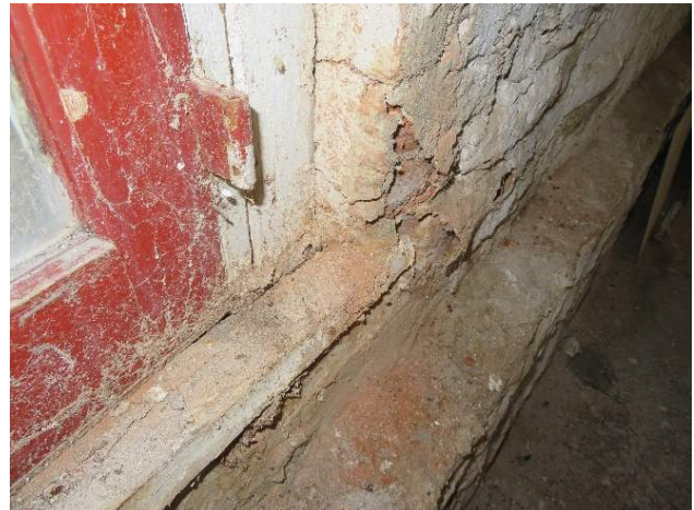
Figure 190. Moisture related brick decay at basement window; typical along east wall. (Source: RRJ, 2022)
