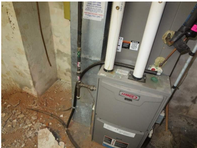
Figure 290. The gas piping serving each of the Basement furnaces is Schedule 40 black steel. (Source: Alvine, 2022)
