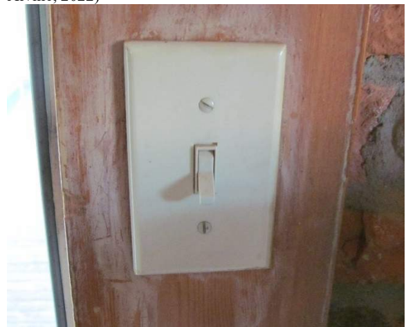
Figure 367. Single-pole, toggle switch in kitchen on first floor. (Source: Alvine, 2022)
