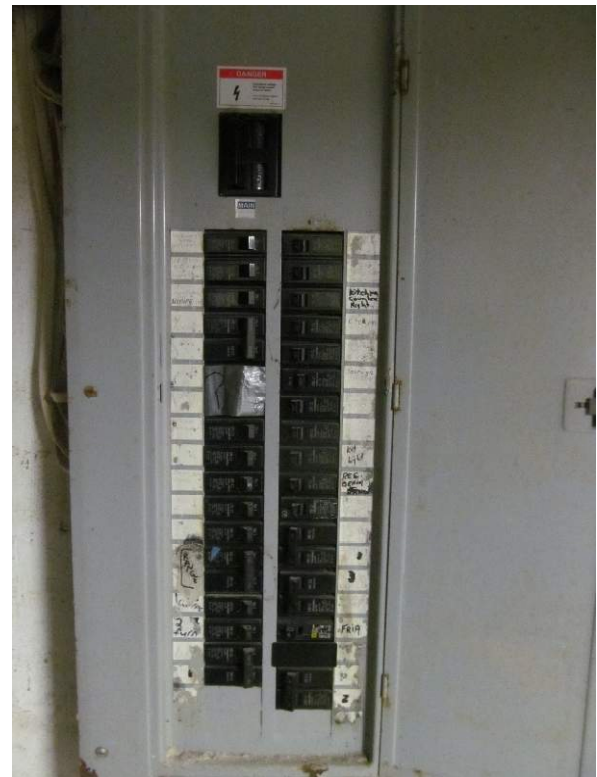
Figure 344. Load center circuit breakers and circuit directory. (Source: Alvine, 2022)
