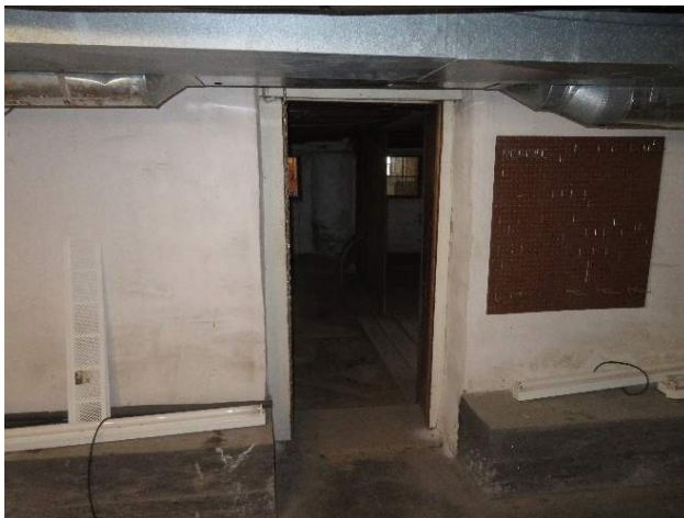
Figure 249. Door D009 has been removed since 1985 HABS documentation. (Source: RRJ, 2022)
