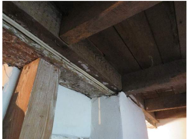
Figure 171. Supplemental post below sill plate, viewed from Room 007. (Source: RRJ, 2022)
