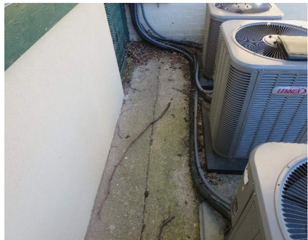
Figure 320. Existing refrigerant piping routes along top of concrete slab to grade-mounted second level condensing unit. (Source: Alvine, 2022)
