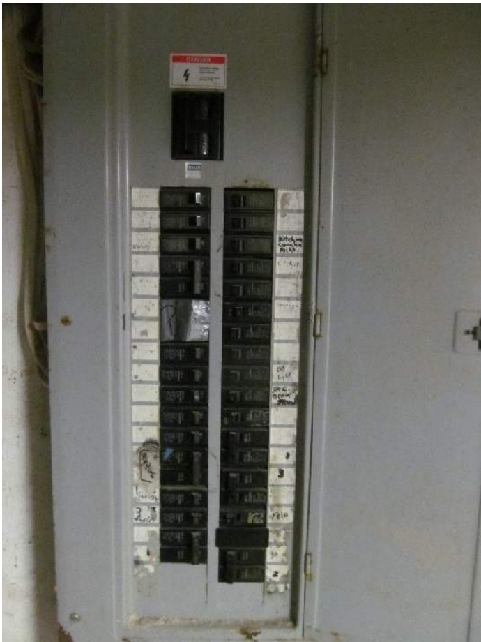
Figure 345. Circuit load marked next to each circuit breaker in load center. (Source: Alvine, 2022)
