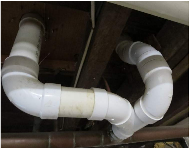
Figure 287. There are portions of the building which have PVC sanitary waste piping connected to the copper DWV piping as indicated in the above photo. (Source: Alvine, 2022)
