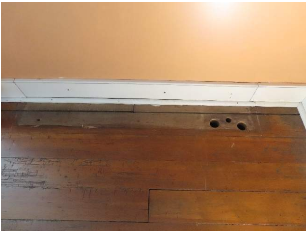
Figure 201. Penetrations in flooring likely from previous radiator. (Source: RRJ, 2022).
