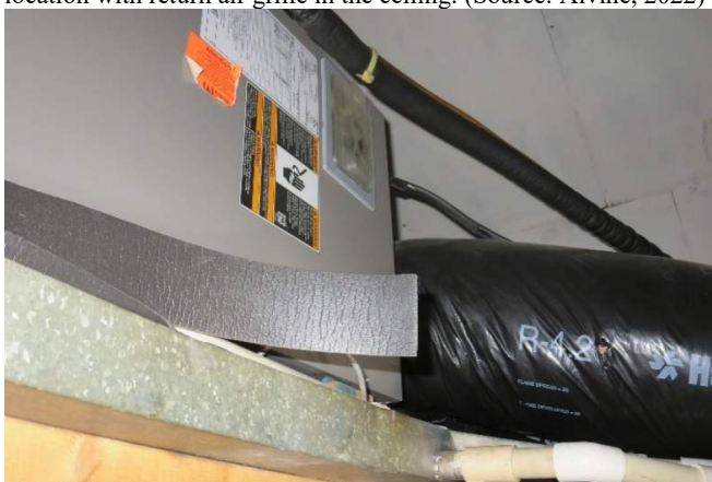
Figure 312. Existing Second level electric furnace with sheet metal pan below. Note the PVC drain line from the pan. (Source: Alvine, 2022)
