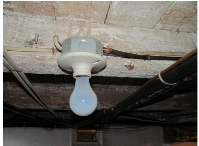
Figure 353. Incandescent lamp holder in basement. (Source: Alvine, 2022)
