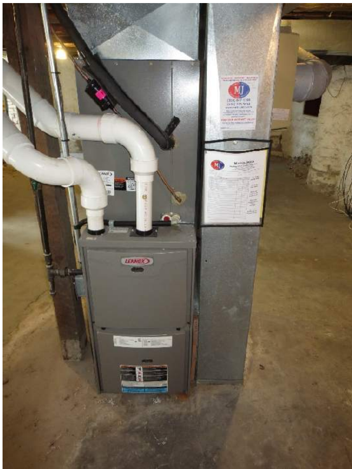
Figure 302. Existing 66,000 Btuh input and 64,000 Btuh output (95% efficient), gas-fired furnace located at center of basement level. (Source: Alvine, 2022)
