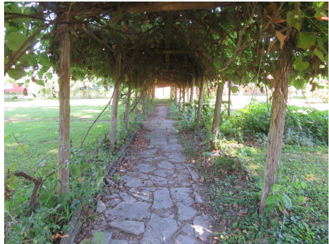
Figure 389. The pathway under the arbor, looking north, prior to the arbor being stabilized and the walkway closed. (Source: RRJ, 2022)
