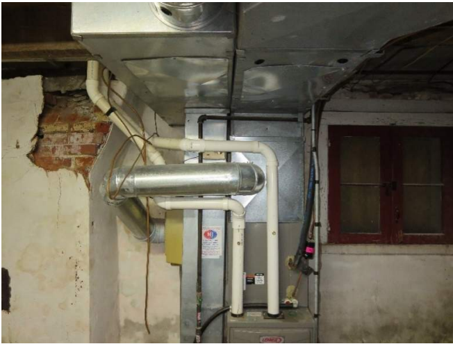
Figure 292. The gas piping serving each of the Basement furnaces is Schedule 40 black steel. (Source: Alvine, 2022)
