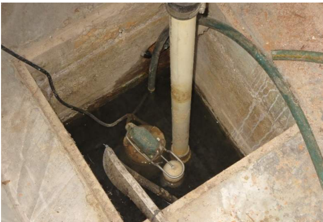
Figure 295. The PVC standpipe routes under the floor to a concrete pit where a sump pump is located. (Source: Alvine, 2022)
