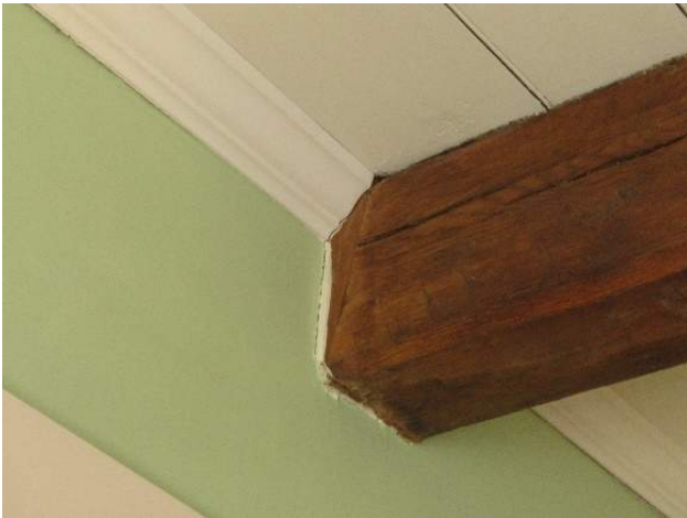
Figure 180. Exposed joist in Room 104 with fill at bearing end. (Source: RRJ, 2022)
