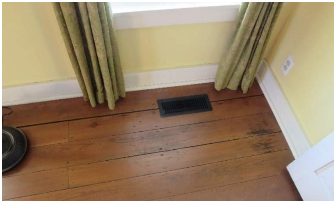
Figure 323. Typical floor supply air register located at the floor of the first level. (Source: Alvine, 2022)
