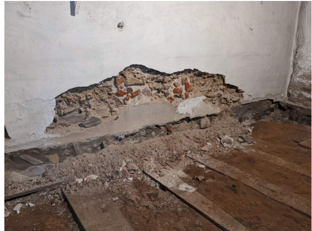
Figure 127. Stone masonry distress including spalling and mortar loss in room 009. (Source: RRJ, 2022)
