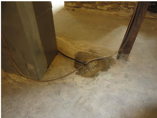
Figure 275. Existing floor drain in the center of the basement level adjacent to the furnace. The drain grate appears to be dirty and partially clogged with debris. (Source: Alvine, 2022).
