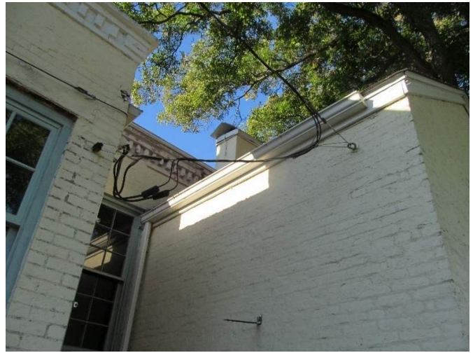
Figure 337. Overhead 240/120-volt secondary electrical attachment to building. (Source: Alvine, 2022)
