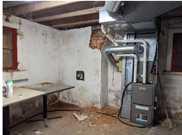
Figure 125. Brick spalling in room 002. (Source: RRJ, 2022).
