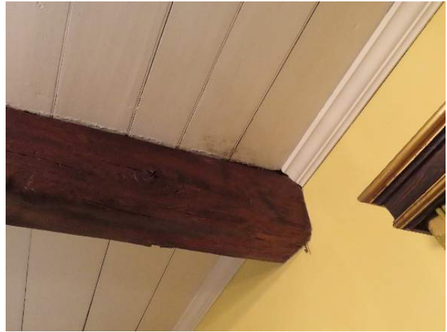
Figure 181. Exposed joist separating from finishes in Room 106. (Source: RRJ, 2022).
