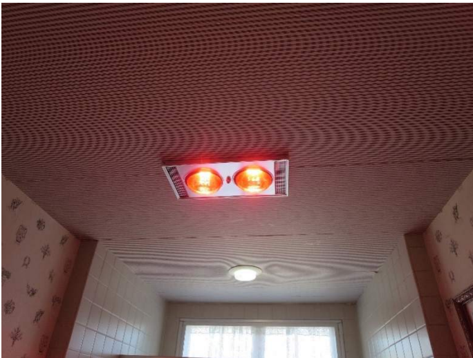
Figure 330. Second level restroom ceiling exhaust fan/heat lamp. (Source: Alvine, 2022)
