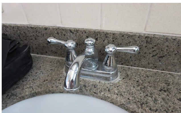
Figure 270. Existing lavatory faucet with two handles at First level restroom. (Source: Alvine, 2022).
