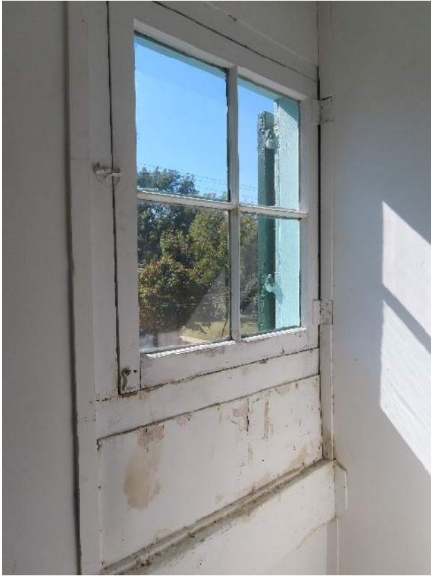
Figure 233. Staining and water damage below window in Room 203. (Source: RRJ, 2022)
