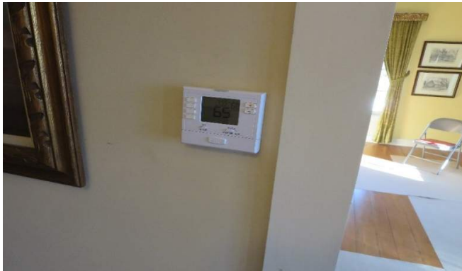
Figure 331. First level furnace system control thermostat located in entry hallway of the first level. This thermostat controls the central basement furnace. (Source: Alvine, 2022)
