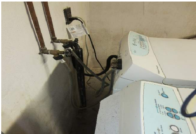
Figure 294. Existing washing machine waste piping discharging into a PVC standpipe behind the washing machine. (Source: Alvine, 2022)
