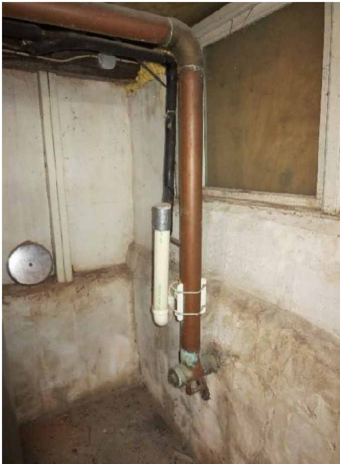
Figure 286. The main sanitary sewer piping exiting the building is copper DWV piping as indicated in the above photo. (Source: Alvine, 2022)
