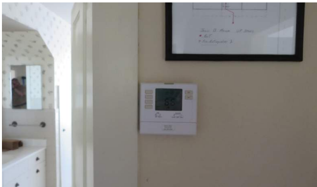
Figure 333. Second level furnace system control thermostat located in the central hallway outside the restroom at the second level. This thermostat controls the Second level furnace. (Source: Alvine, 2022)
