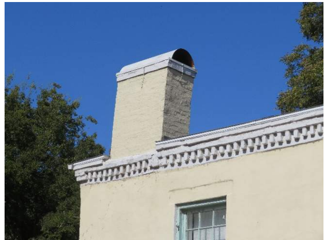
Figure 84. Office Chimney leaning toward the north . (Source: Source: RRJ, 2022)
