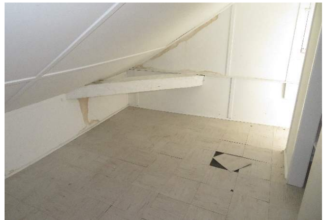
Figure 231. Debonded linoleum tile flooring in Room 203. (Source: RRJ, 2022)
