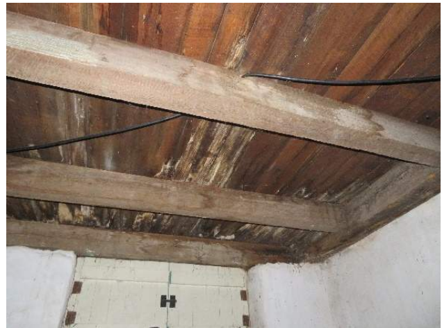
Figure 134. Evidence of past water infiltration near window. (Source: RRJ, 2022).
