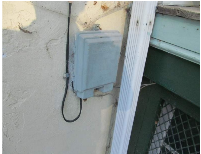
Figure 371. Cable television junction box on south side of building. (Source: Alvine, 2022)
