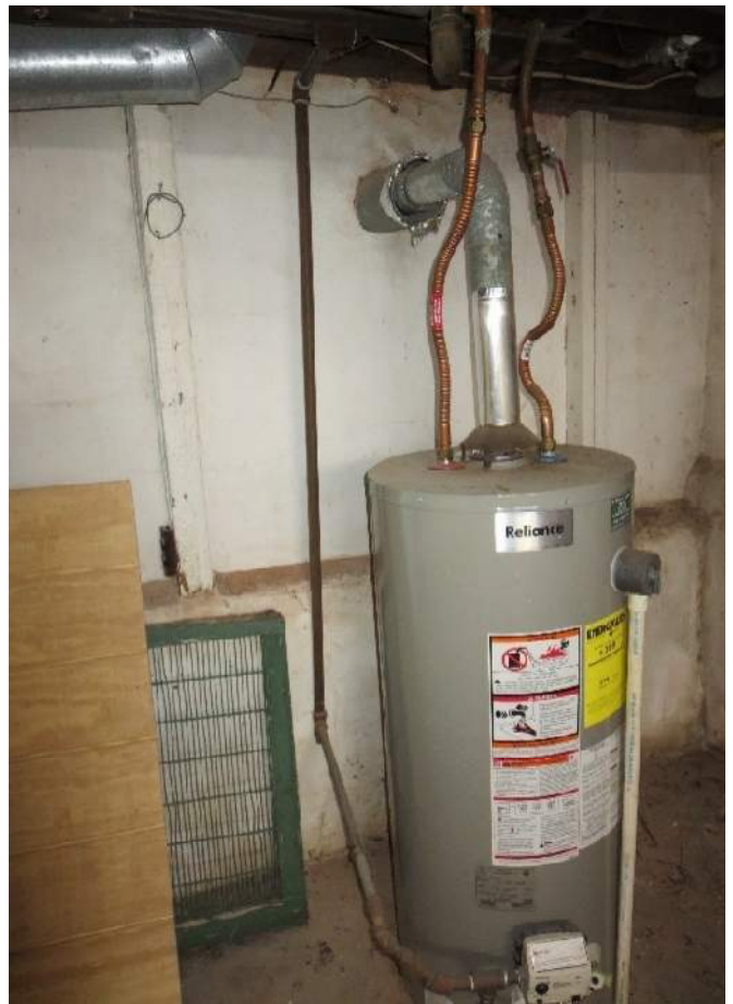
Figure 293. The gas piping serving the water heater in the basement level is Schedule 40 black steel before transitioning to flexible copper pipe at the water heater. (Source: Alvine, 2022)
