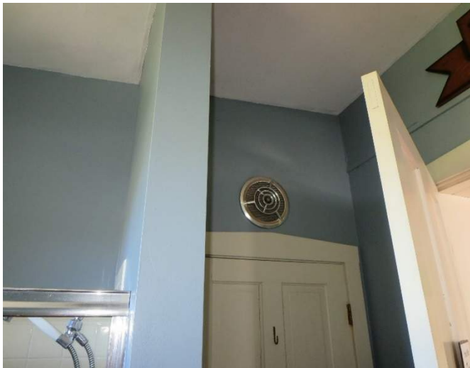
Figure 329. First level restroom wall exhaust fan. (Source: Alvine, 2022)
