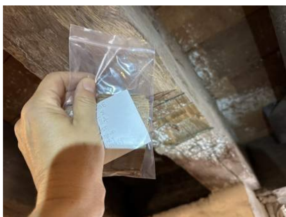
Figure 11. Sample 8. Room 11A, beam, white oak.
