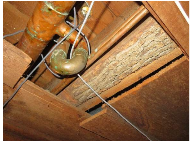
Figure 154. Bottom face of joist exhibiting tree bark at opening in the ceiling. (Source: RRJ, 2022)
