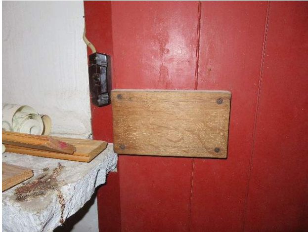
Figure 248. Hardware at Door D006. (Source: RRJ, 2022)
