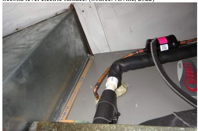
Figure 313. Existing Second level electric furnace with refrigerant coil. Note sheet metal pan below unit. (Source: Alvine, 2022)
