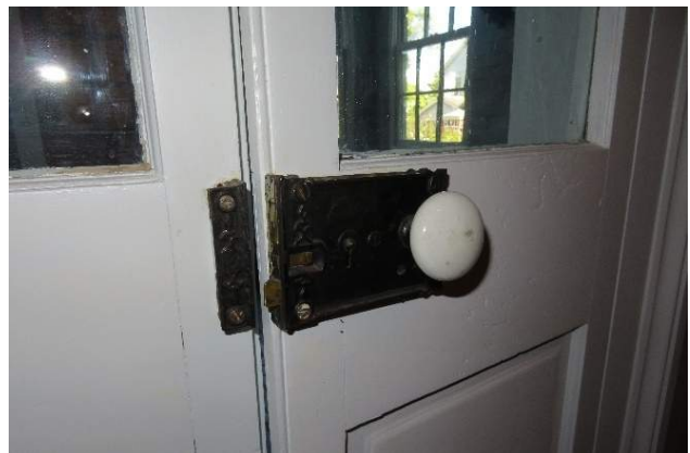
Figure 255. Rim lock and door knob at Door D107B. (Source: RRJ, 2022)
