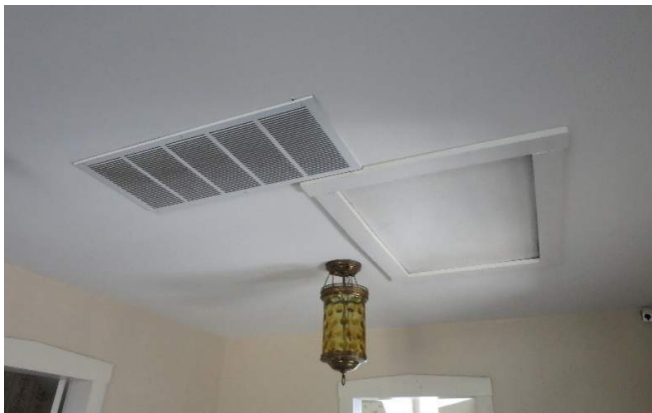
Figure 310. Existing ceiling area below Second level electric furnace location with return air grille in the ceiling. (Source: Alvine, 2022)
