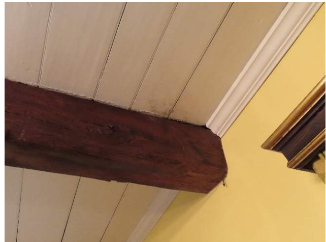
Figure 210. Mild mildew and moisture damage at west wall at ceiling beam. (Source: RRJ, 2022).
