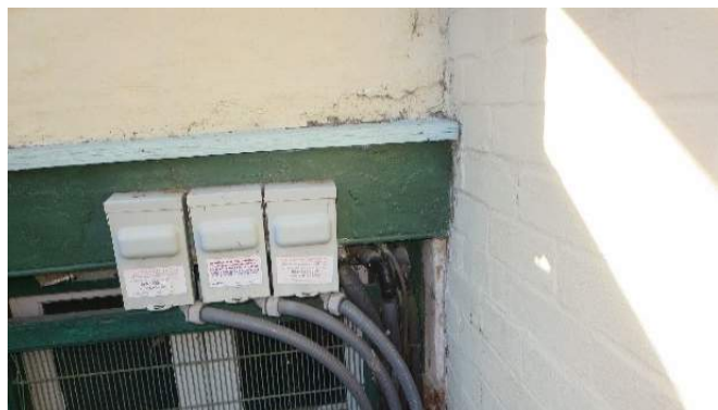
Figure 317. Existing refrigerant piping routing through exterior wall above corner of basement window. (Source: Alvine, 2022)
