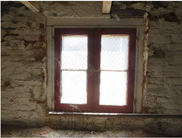
Figure 89. Interior view of typical basement level Casement Window with metal mesh covering (Source: RRJ, 2022).
