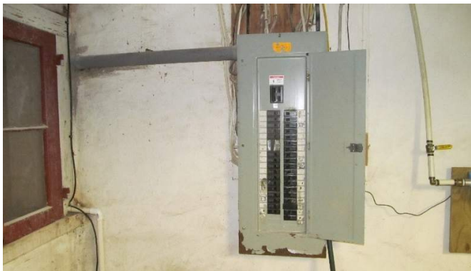
Figure 342. 240/120-volt, 200-amp load center in basement. (Source: Alvine, 2022)
