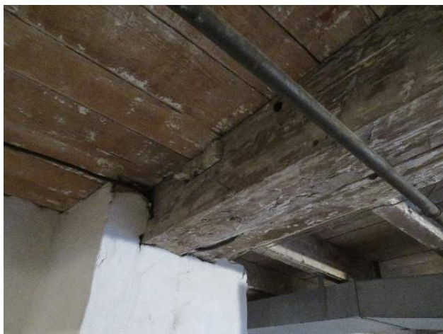
Figure 148. Missing diagonal brace within timber beam at north. (Source: RRJ, 2022)
