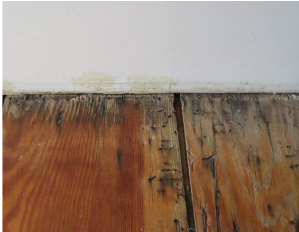
Figure 196. Mild moisture damage of flooring in Room 101. (Source: RRJ, 2022).
