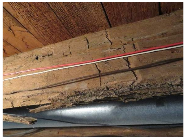
Figure 146. Hand hewn joist with tree bark and powder post beetle exit holes. (Source: RRJ, 2022).
