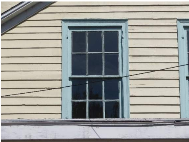
Figure 82. Weatherboard siding at the second floor (Source: RRJ, 2022).
