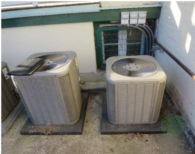
Figure 318. Existing condensing unit (on the left) which serves the Second level electric furnace located in the attic. This unit is a 2-ton unit. (Source: Alvine, 2022)
