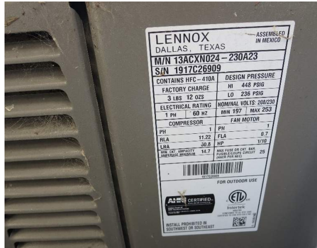
Figure 319. Existing 2-ton condensing unit serving Second level furnace. (Source: Alvine, 2022)
