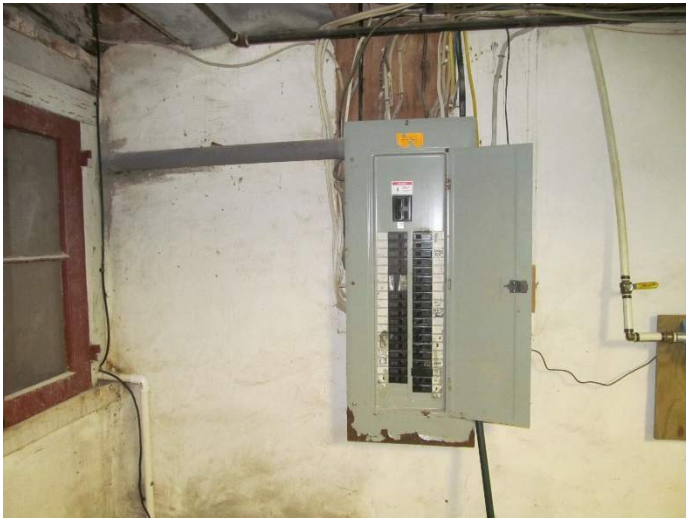
Figure 346. There is no visible grounding electrode connection visible from load center. (Source: Alvine, 2022)
