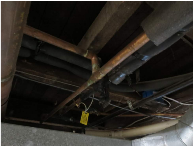
Figure 279. Existing copper water piping with closed cell insulation in basement level. (Source: Alvine, 2022).
