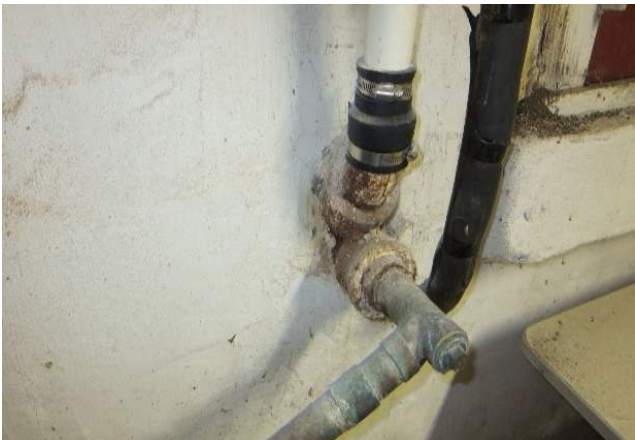
Figure 297. The existing copper DWV waste piping then connects to a cast iron hub and spigot drain line which exits the west wall of the basement level. (Source: Alvine, 2022)
