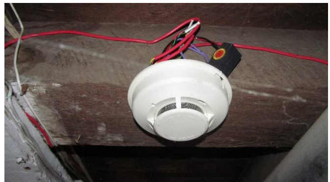
Figure 373. Fire alarm/smoke detector in basement. (Source: Alvine, 2022)
