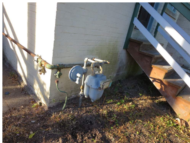
Figure 264. Existing gas utility meter location near the northeast corner of the building. (Source: Alvine, 2022).
