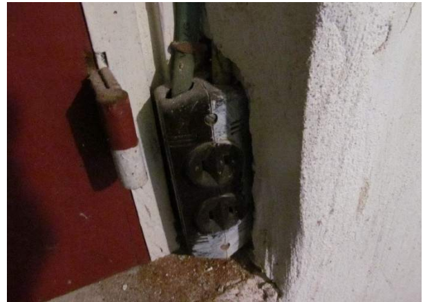
Figure 365. Double-duplex, non-grounded, 120-volt receptacle in north storage room in basement. (Source: Alvine, 2022)
