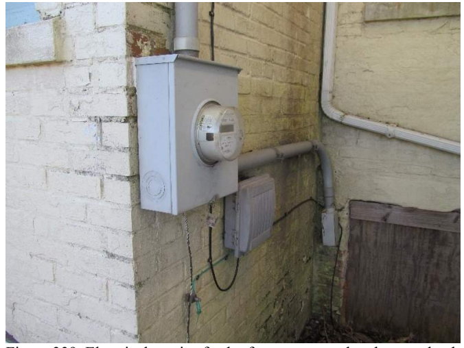
Figure 339. Electrical service feeder from meter socket down to load center in basement. (Source: Alvine, 2022)
