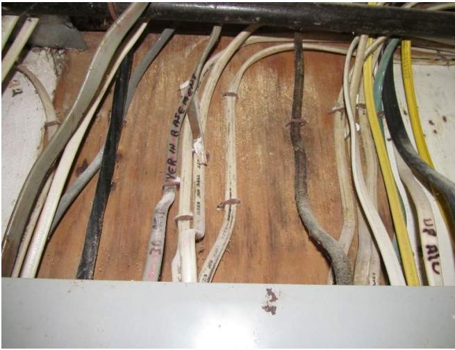
Figure 349. Non-metallic sheathed (NM) cable and cloth covered NC cable originating from top of load center. (Source: Alvine, 2022)
