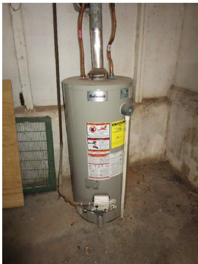
Figure 282. Existing gas-fired water heater located at the basement level. (Source: Alvine, 2022)
