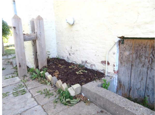
Figure 83. Masonry Foundation wall with peeling finishes and missing mortar (Source: RRJ, 2022)
