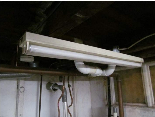
Figure 352. Fluorescent 4-ft. strip light in basement. (Source: Alvine, 2022)
