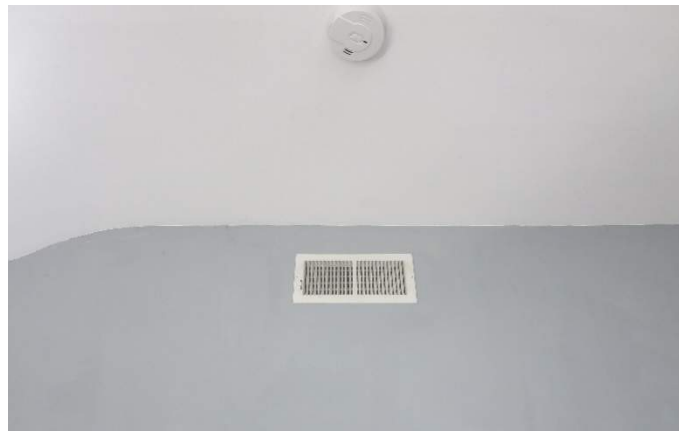
Figure 326. Typical sidewall supply air registers located up high on the walls of the Second level rooms. (Source: Alvine, 2022)
