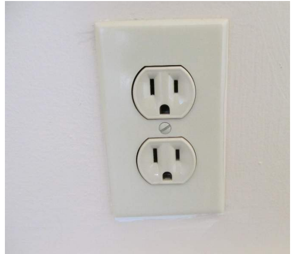
Figure 369. Double-duplex, 120-volt, 15-amp receptacle in living room on first floor. (Source: Alvine, 2022)
