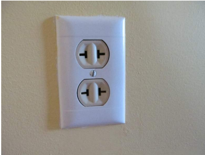
Figure 368. Double-duplex, non-grounding, 120-volt receptacle in the living room on first floor. (Source: Alvine, 2022)
