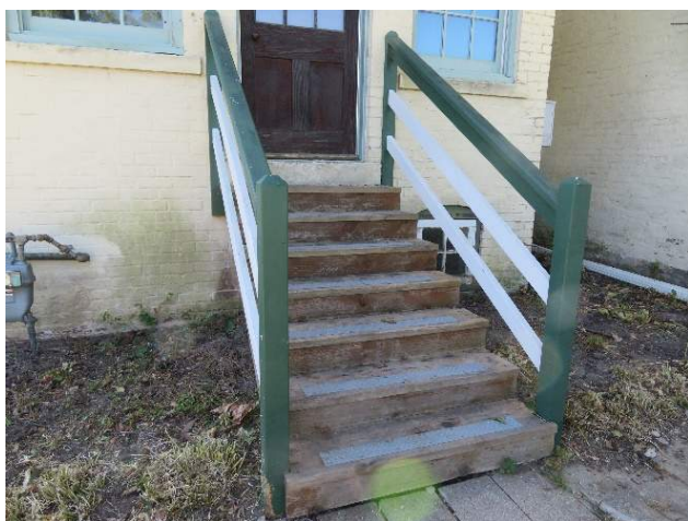
Figure 118. Stairs and handrails to sunroom; the treads have since been replaced. (Source: : RRJ, 2022)
