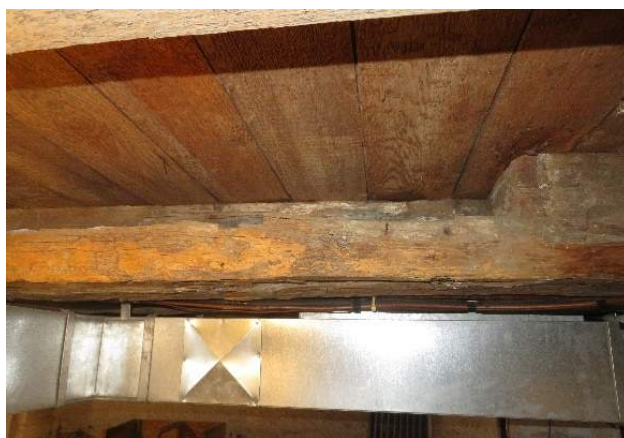
Figure 163. Notched joist at former fireplace location. (Source: RRJ, 2022)
