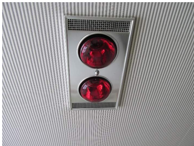
Figure 361. Heat/vent light in bathroom on second floor. (Source: Alvine, 2022)
