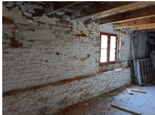
Figure 126. Brick distress including spalling in room 013. (Source: RRJ, 2022)
