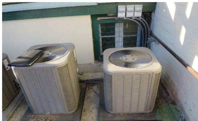
Figure 314. Existing condensing units for basement level furnaces. The unit capacities are 3-ton (left) and 2-ton (right). (Source: Alvine, 2022)
