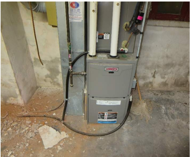
Figure 303. Existing 66,000 Btuh input and 64,000 Btuh output (95% efficient), gas-fired furnace located at northwest end of basement level. (Source: Alvine, 2022)
