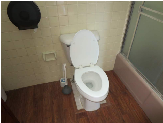
Figure 265. Existing floor-mounted, bottom-outlet, pressure-assisted, water closet at First Floor restroom. (Source: Alvine, 2022)
