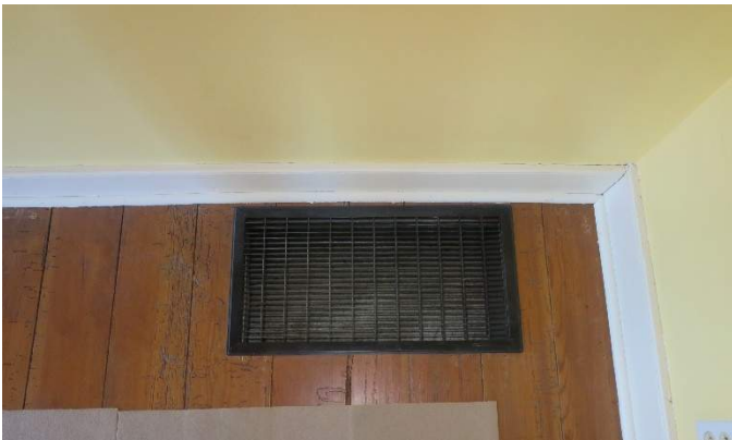
Figure 324. Typical floor return air grille located at the floor of the first level. (Source: Alvine, 2022)
