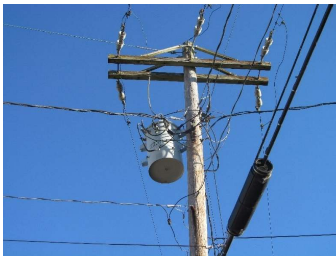
Figure 335. Citizen Electric Corporation oil-filled, pole-mounted transformer. (Source: Alvine, 2022)
