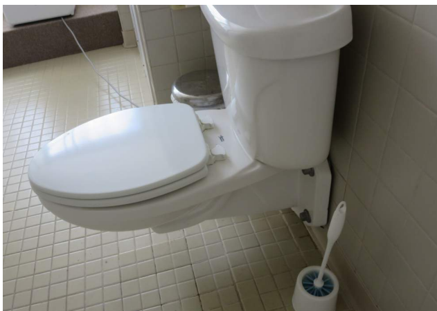
Figure 266. Existing wall-mounted, back-outlet, pressure assisted, water closet at Second level restroom. (Source: Alvine, 2022).
