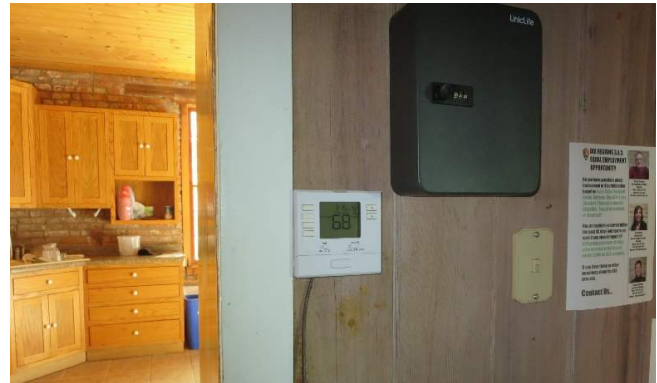
Figure 332. First level furnace system control thermostat located at the entry of the kitchen of the first level. This thermostat controls the northwest basement furnace. (Source: Alvine, 2022)
