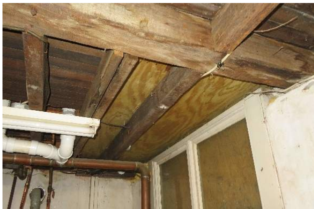
Figure 140. Plywood at room southwest. (Source: RRJ, 2022)
