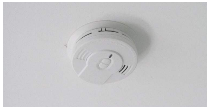
Figure 374. Fire alarm/smoke detector in hallway on second floor. (Source: Alvine, 2022)
