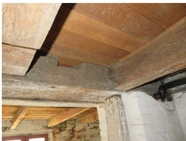
Figure 165. Un-used half dovetail lap joint at southeast corner. (Source: RRJ, 2022).
