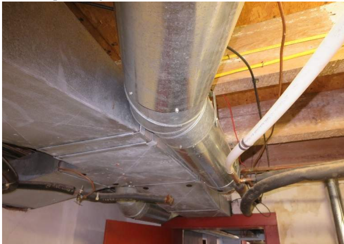
Figure 321. Typical supply air ductwork located at the basement level which serves the First level spaces. (Source: Alvine, 2022)
