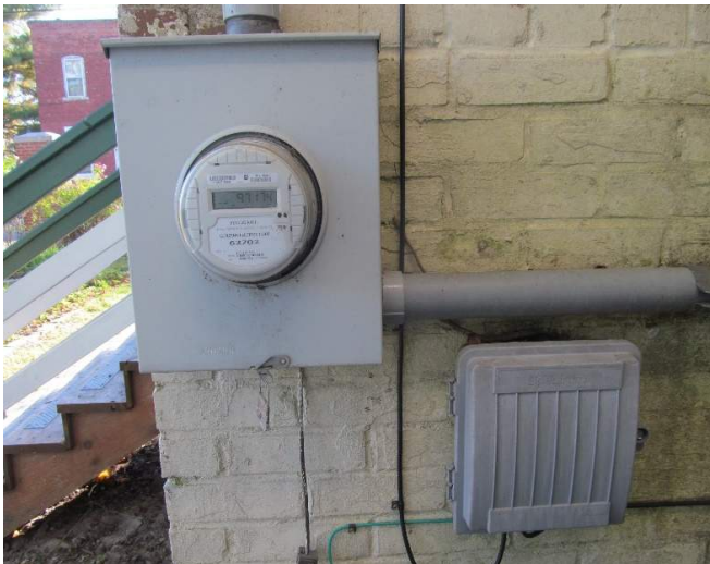
Figure 370. Telephone cable junction box on the right side; electrical meter on left side on north side of building. (Source: Alvine, 2022)
