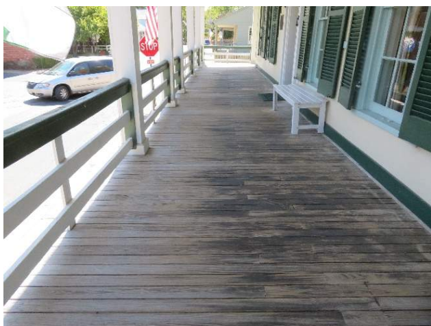
Figure 120. Weathered decking at east gallery; this has since been replaced with new decking (Source: : RRJ, 2022)
