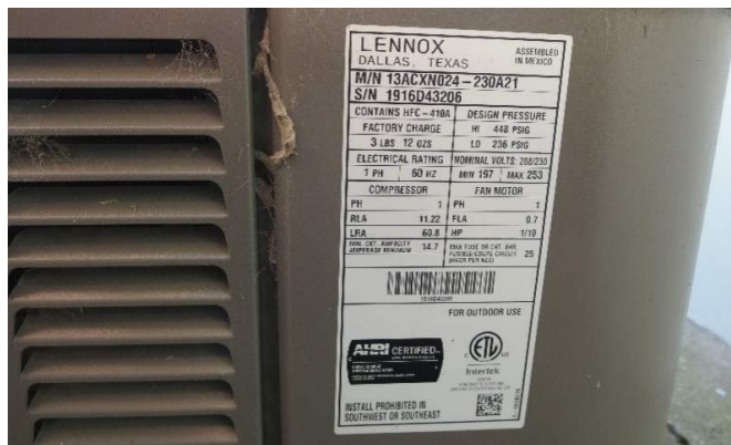
Figure 315. Existing 2-ton condensing unit serving NW basement level furnace. (Source: Alvine, 2022)
