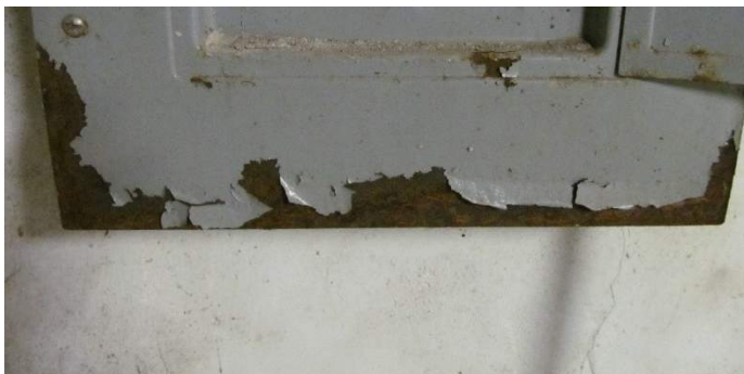
Figure 343. Rusting on load center. (Source: Alvine, 2022)
