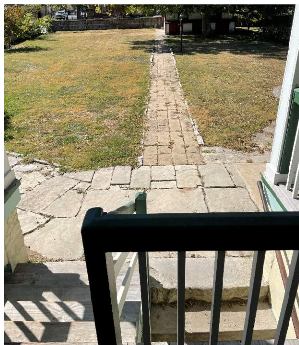
Figure 384. View of the intersection of the cut-stone walkways, their deteriorated condition, and the staircase leading to the west porch. The existing conditions interfere with an accessible route to the west entrance of the house. (Source: LSHLA, 2022)
