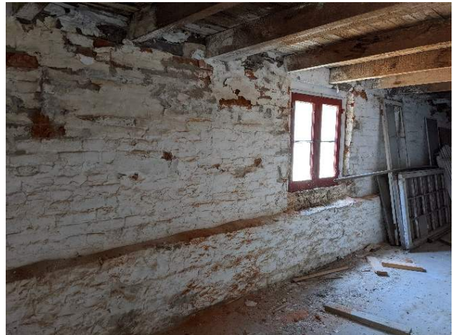
Figure 192. Failed plaster and brick decay at east wall of basement. (Source: RRJ, 2022)
