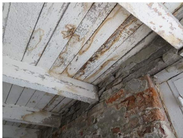
Figure 157. Planking and joists exhibiting staining related to water infiltration along the south exterior wall. (Source: RRJ, 2022).
