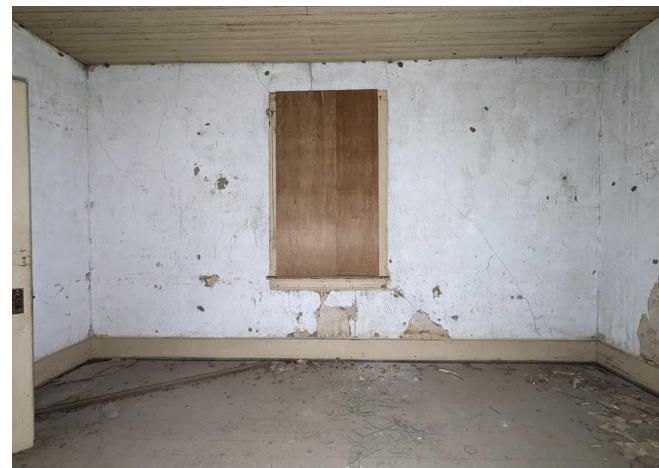
Figure 186. Room 201, looking east, showing damage to the plaster under the failed window. (Source: RRJ 2023)
