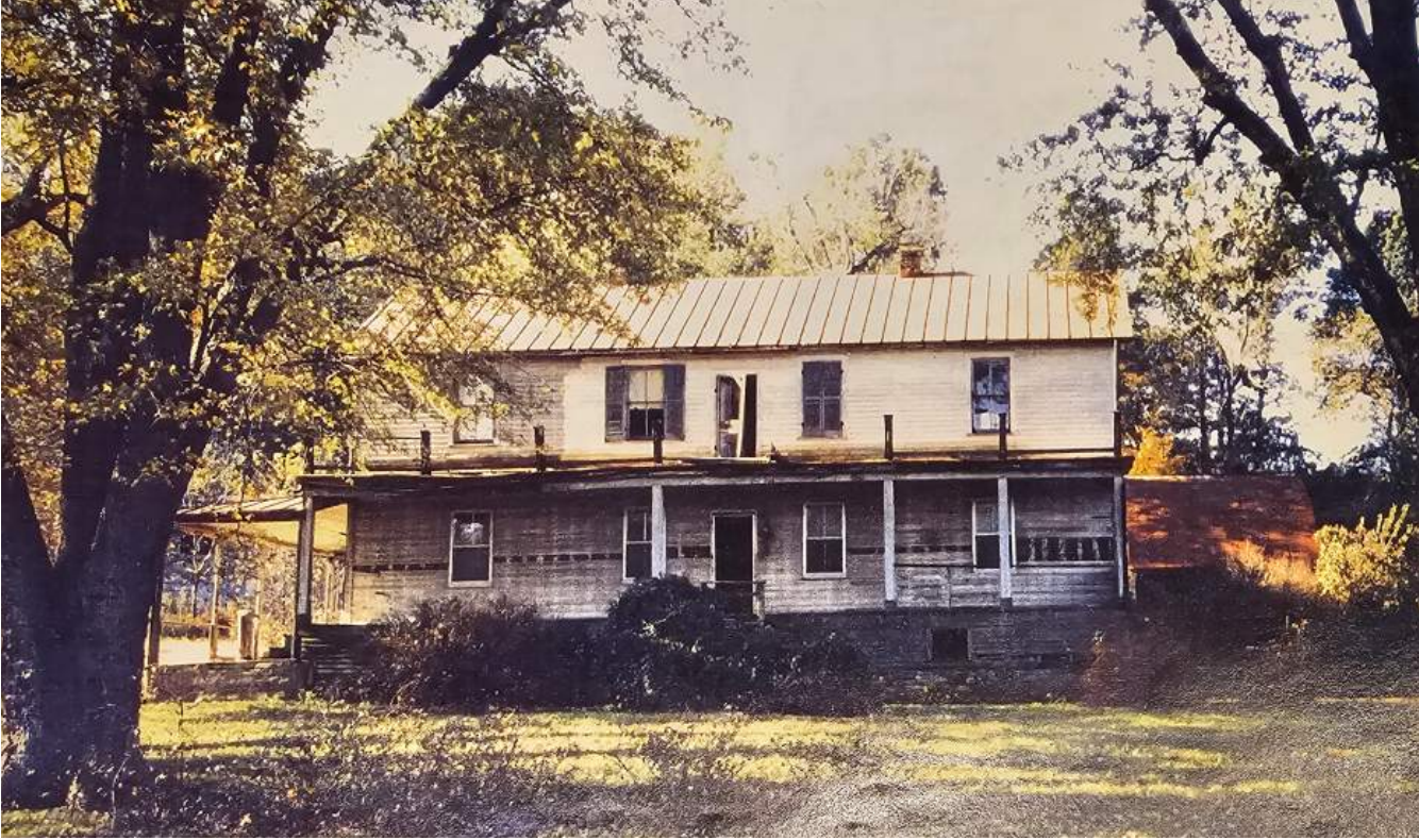
Figure 26. The east exterior in 1990, showing continued deterioration of the exterior. (Source: Volz and Associates, "Pierre Delassus de Luziere House (Kern House) Condition Assessment Report").
