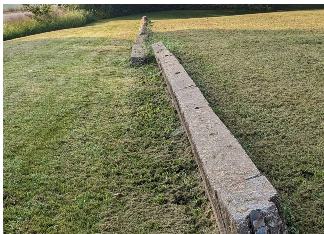
Figure 90. Displacement and distress to the concrete retaining wall, looking south. (Source: LSHLA 2023)
