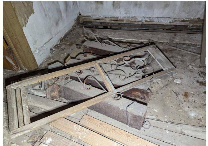
Figure 120. Damaged louvered shutter in the debris in Room 204 (Source: RRJ 2023)
