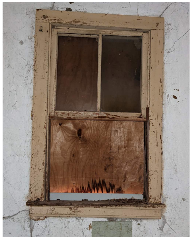
Figure 116. W201B, with missing lower sash. (Source: RRJ 2023)
