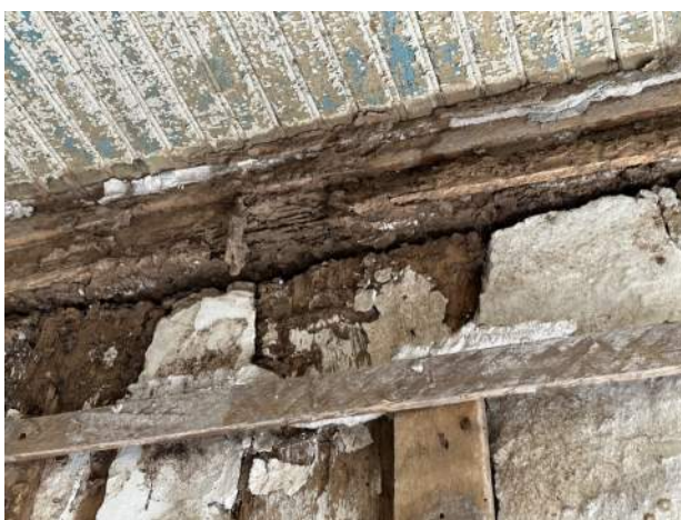
Figure 6. Termite damage in the top sill and vertical logs. Room I.
