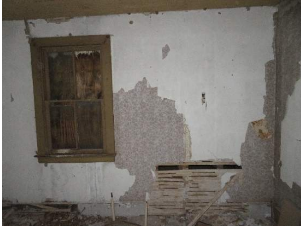
Photo 50. Second-floor stud wall framing visible within areas of missing plaster finishes.
