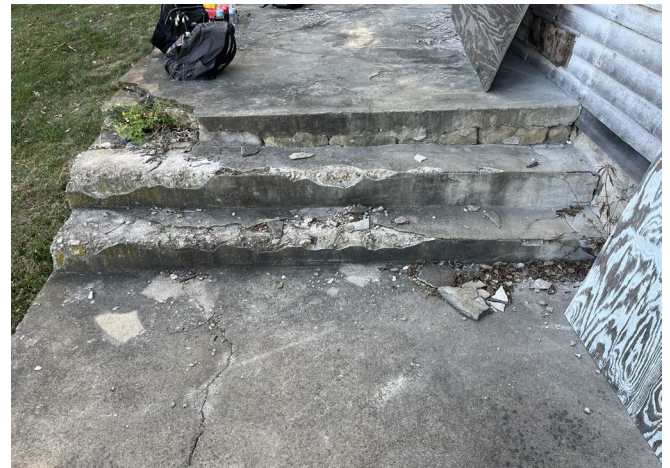
Figure 88. Deteriorated concrete steps. (Source: RRJ 2023)
