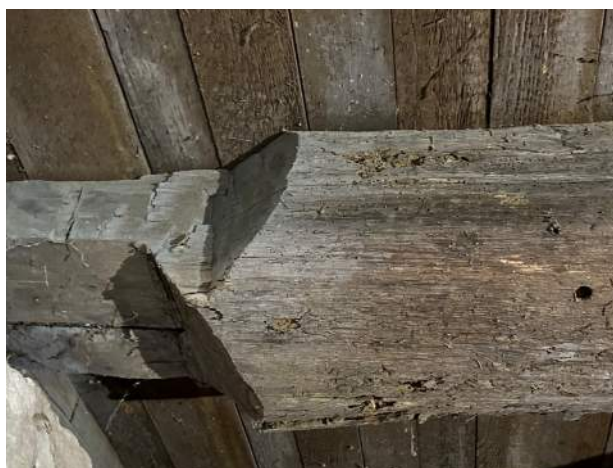
Figure 12. Pin-size powderpost beetle emergence holes on the wood surface.
