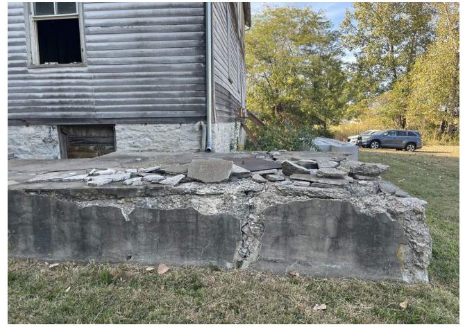
Figure 87. Deteriorated concrete landing. (Source: RRJ 2023)
