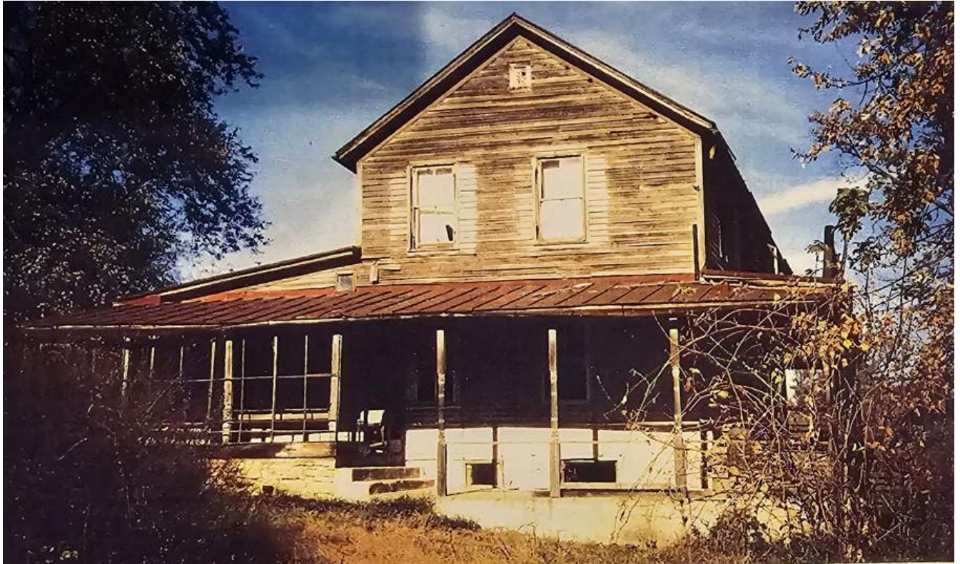
Figure 28. The south exterior wall in 1990, showing continued deterioration of the exterior. (Source: Volz and Associates, "Pierre Delassus de Luziere House (Kern House) Condition Assessment Report").
