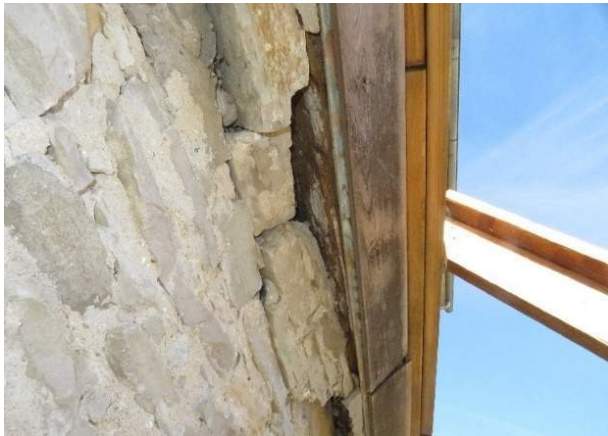
Photo 31. Underside of east wall bottom plate visible from exterior where the log wall and top course of stones have moved out of plane. The exposed log surface shows evidence of moisture and pest damage.
