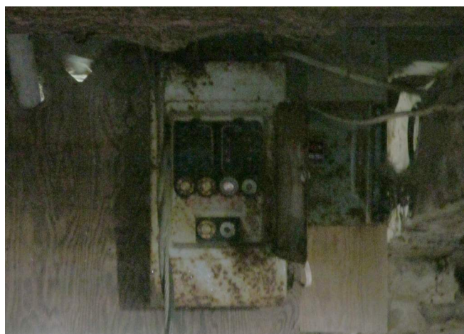
Figure 228. Photograph of existing, not-active 240/120-volt, 1-phase, 6-circuit, plug-fuse panel in basement. (Source: Alvine 2023)
