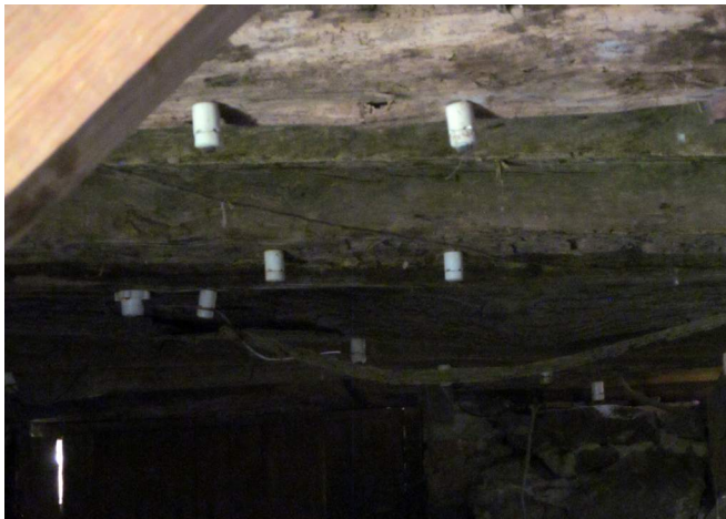
Figure 224. Photograph of remaining know-and-tube wiring. (Source: Alvine 2023)
