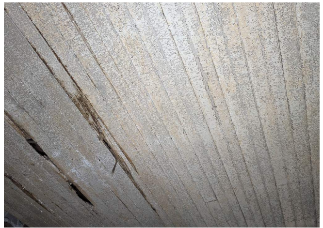
Figure 179. Distress to beadboard ceiling in Room 105. (Source: RRJ 2023)
