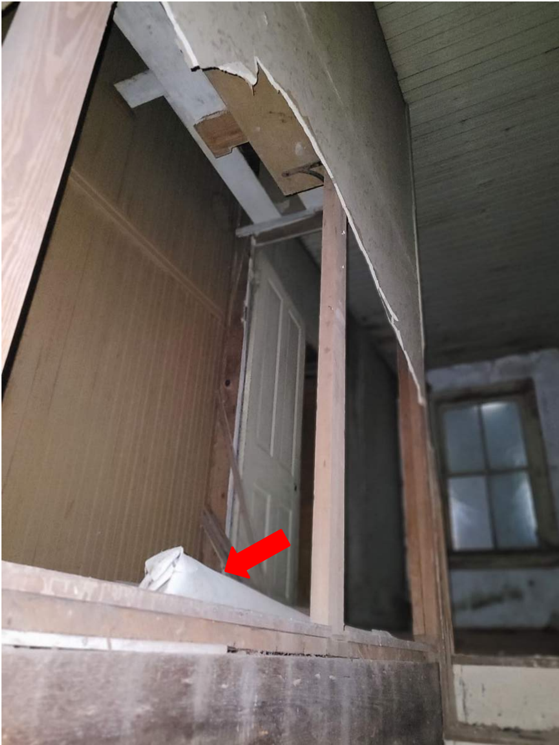
Photograph 18: LBP closet door (white), closet wall (brown), and asbestos linoleum Room 202.
