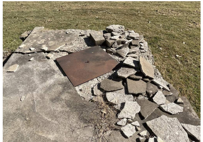
Figure 80. Porch cistern, showing deteriorated concrete and loose metal plate cover. (Source: RRJ 2023)
