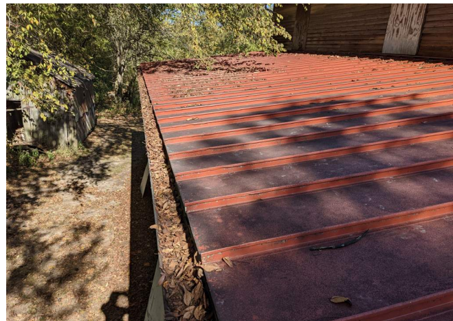
Figure 96. View of the standing seam metal panel roofing from the west, showing the gutters full of leaves. (Source: RRJ 2023)
