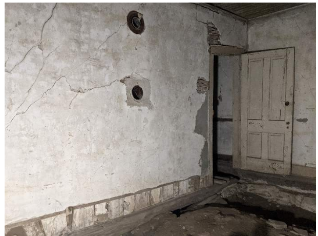
Photo 19. Remaining interior finishes at the south interior wall of Room 103.
