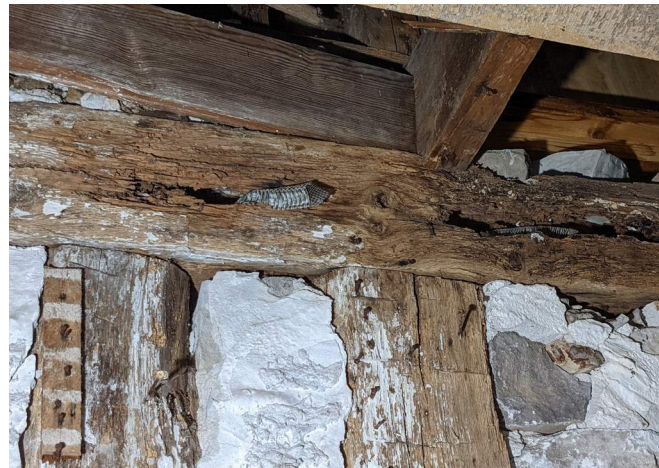
Figure 140. Deterioration of the top plate in Room 105. (Source: RRJ 2023)
