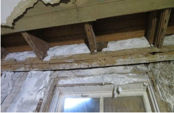
Photo 27. East wall top plate distress within room 104. The top plate has split through its mid-height, and is crushing and rotating. The lower face of the top plate is visible.
