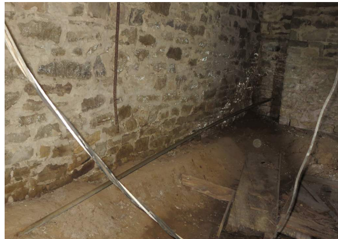
Figure 212. Existing 1-inch galvanized water piping along the west wall where piping is laying on the dirt floor from where it has been disconnected at the vertical pipe offsetting down to the pump at the center of the Basement space. (Source: Alvine 2023)
