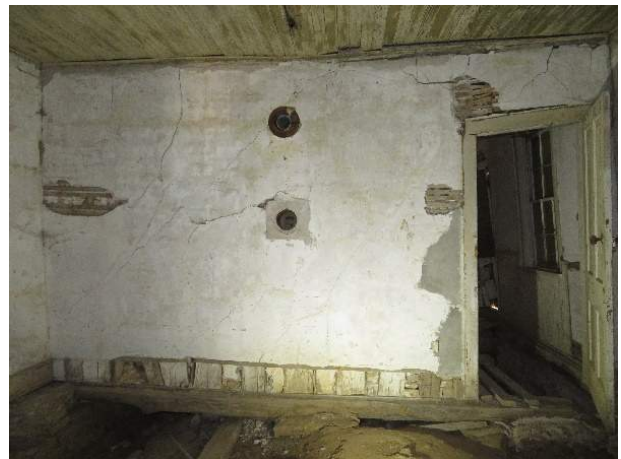
Photo 33. Rotated door framing and cracked interior finishes observed within the south wall of room 103.
