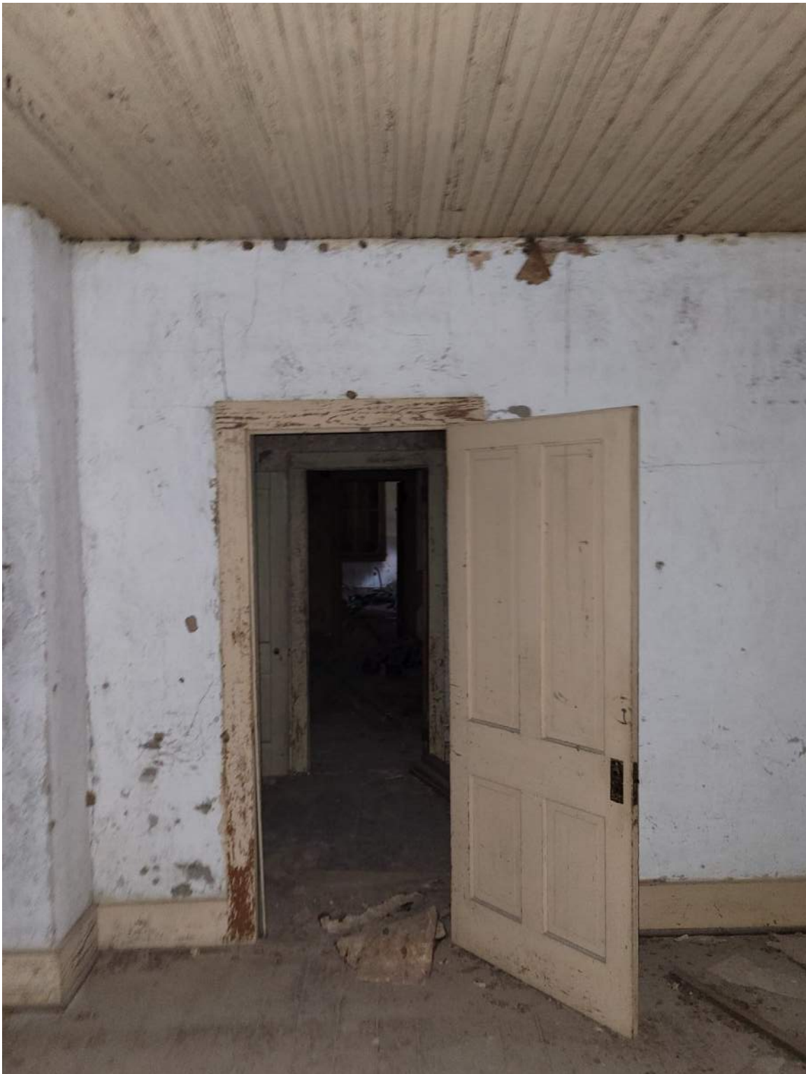
Photograph 16: LBP door and door frame Room 201.
