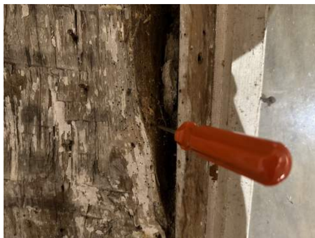
Figure 7. Powderpost beetle pin-size emergence holes and damage restricted to the sapwood of oak.
