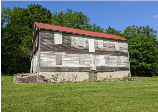
Figure 67. The east exterior wall before shoring installation. (Source: RRJ 2022)
