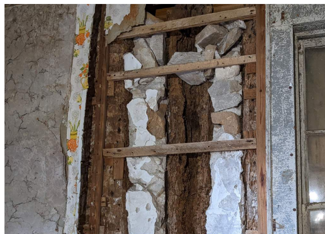
Figure 135. Termite and water damage to logs on the west wall of Room 101. (Source: RRJ 2023)
