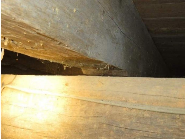
Photo 44. Gap observed between joist 9 and girder.
