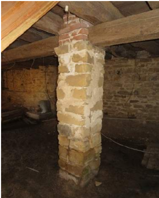
Photo 38. Masonry pier in the basement. Note mortar loss at base and transition from stone to brick masonry at the bottom face of the wood girder.
