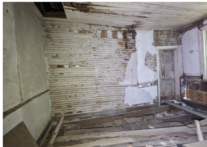
Figure 164. Room 102, looking south, note the loss of plaster on the south interior wall. (Source: RRJ 2023)
