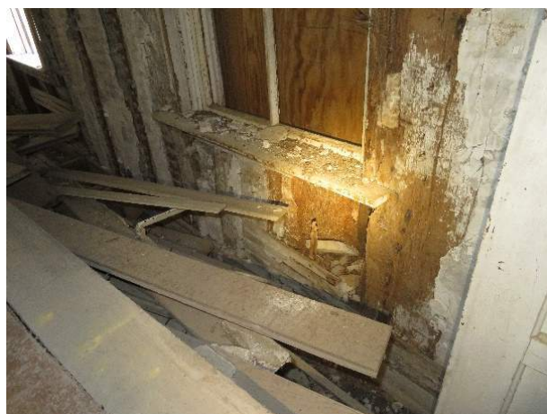
Photo 76. Animal damage to vertical log near a hole in exterior cladding below window W104B.
