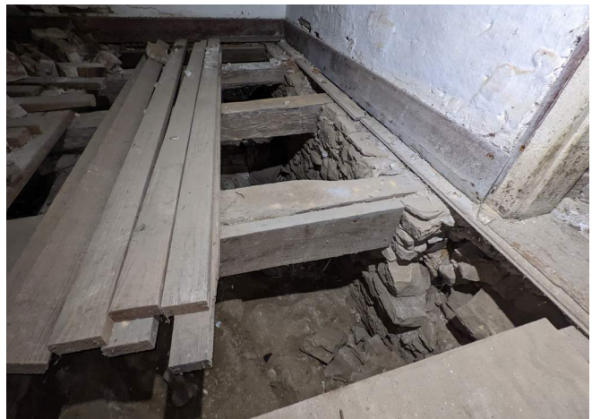
Figure 144. Damaged floor framing in Room 102. (Source: RRJ 2023)
