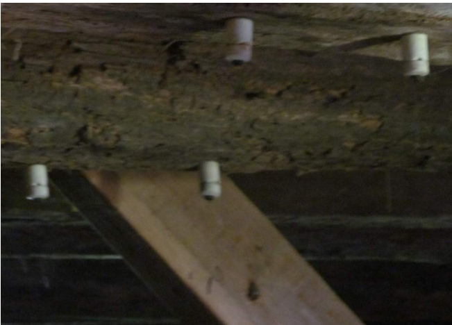
Figure 225. Photograph of remaining know-and-tube wiring. (Source: Alvine 2023)
