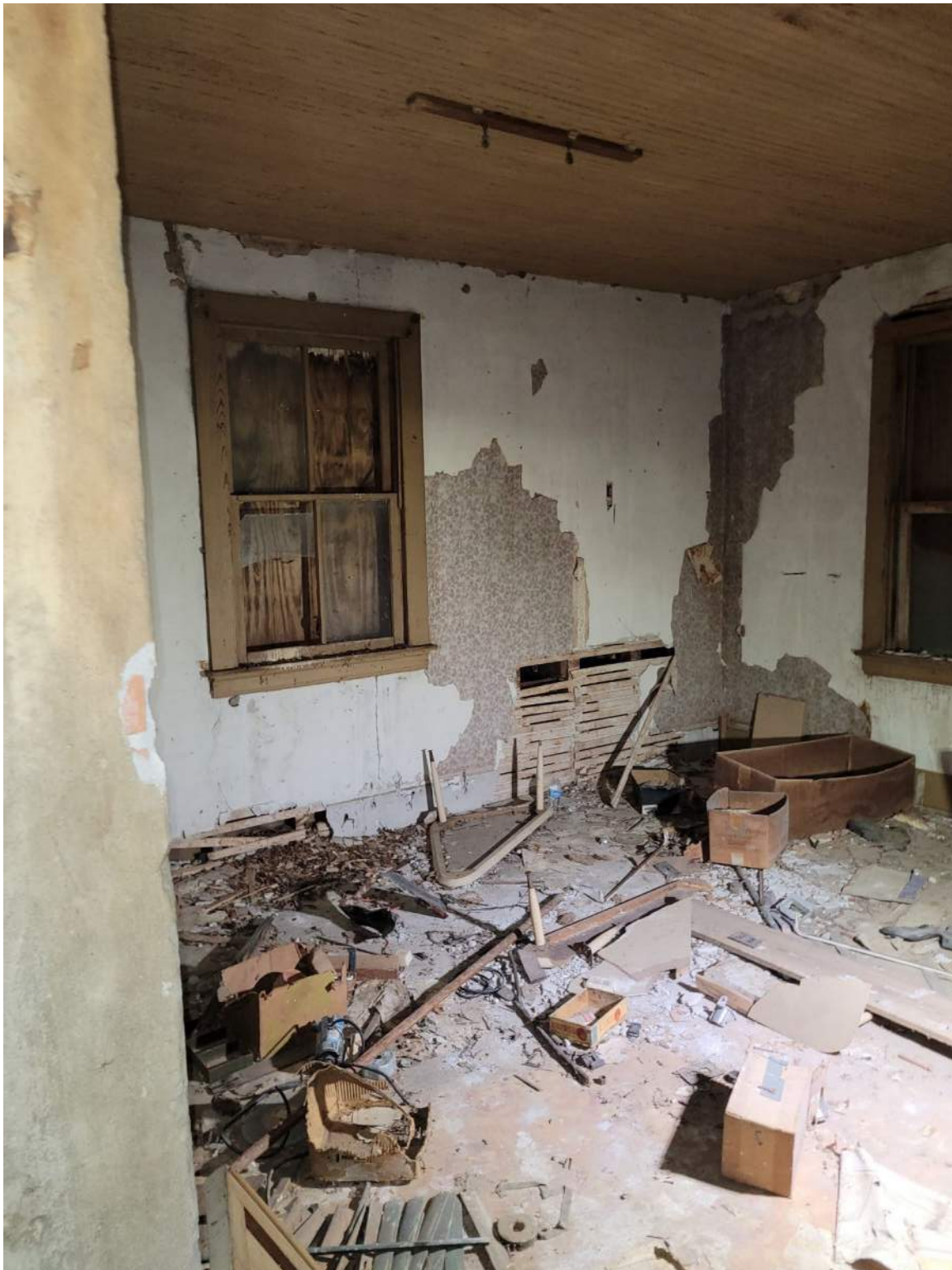
Photograph 20: LBP window, window frame, and baseboard Room 203.
