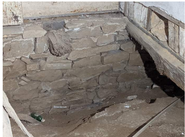
Photo 36. Missing mortar within interior masonry wall west face as viewed from room 103.
