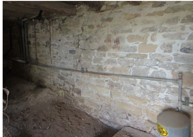
Figure 211. Existing 1-inch galvanized water line along the west all of the Basement level where the line extends through the south exterior wall. Note the offset in the piping down to the abandoned pump at the center of the room. (Source: Alvine 2023)
