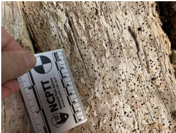
Figure 29. Powderpost beetle emergence holes on the interior wall log.
