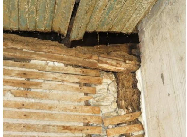
Photo 32. Failed top plate within the wall separating rooms 101 and 102 at room centerline.
