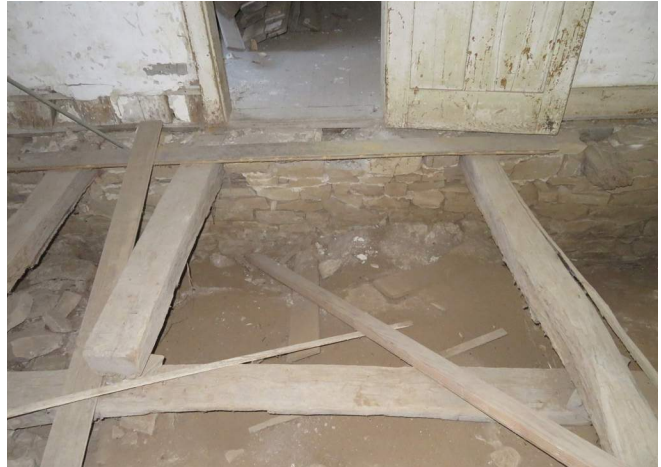
Figure 143. Damaged floor framing in Room 103. (Source: RRJ 2023)
