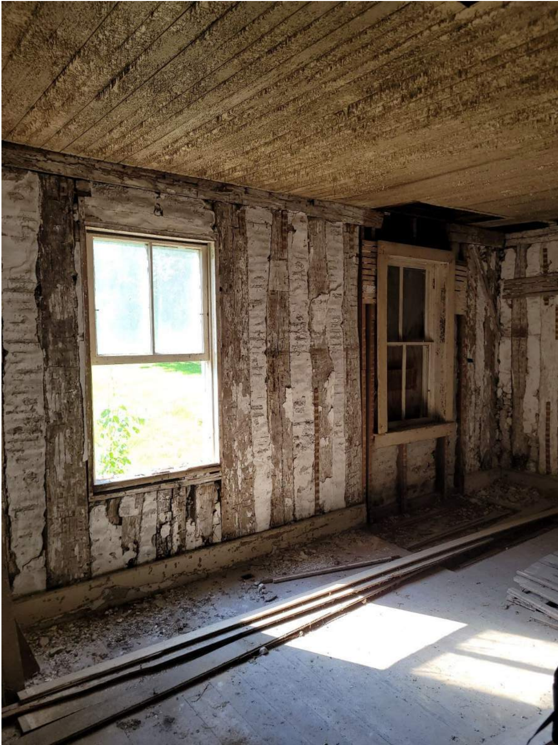
Photograph 11: LBP baseboard, window, window frame, and ceiling Room 102.
