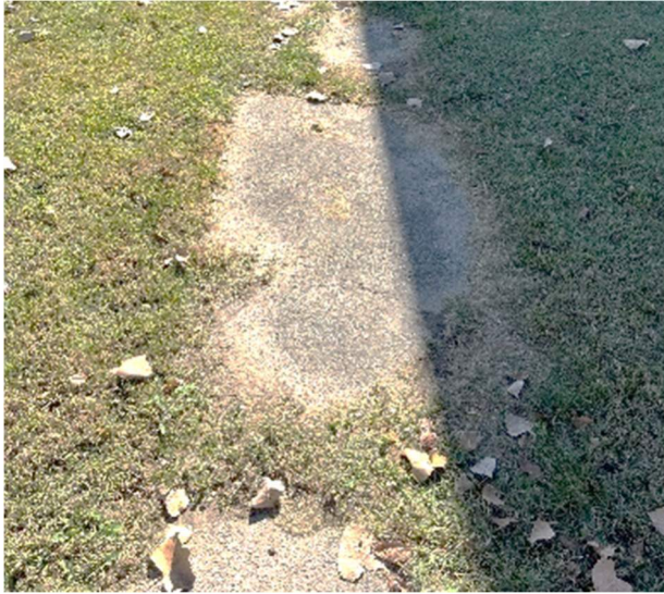
Photo 56. Deteriorated concrete walkway.
