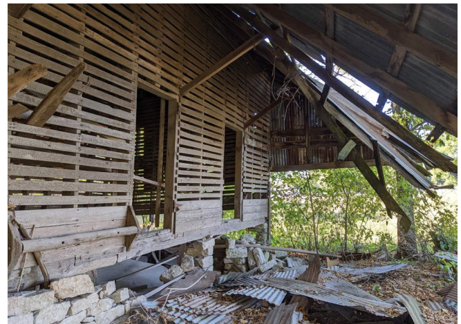
Figure 72. East exterior wall of the corn crib, showing deterioration of the foundation and roof overhang. (Source: RRJ 2023)
