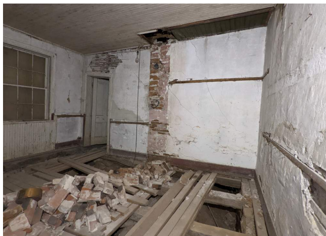
Figure 122. Collapsed chimney in Room 102, with brick rubble still present in room. (Source: RRJ 2023)
