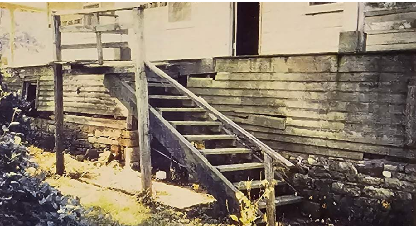
Figure 27. 2000 photograph of the east porch stairs; note that the left flight is now missing. (Source: Volz and Associates, "Pierre Delassus de Luziere House (Kern House) Condition Assessment Report").
