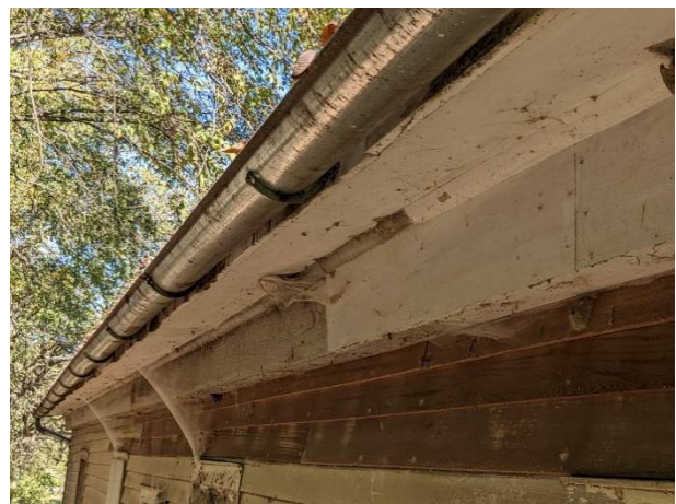
Photo 79. West gutter showing anchored gutter hangers and visible corrosion on gutter.
