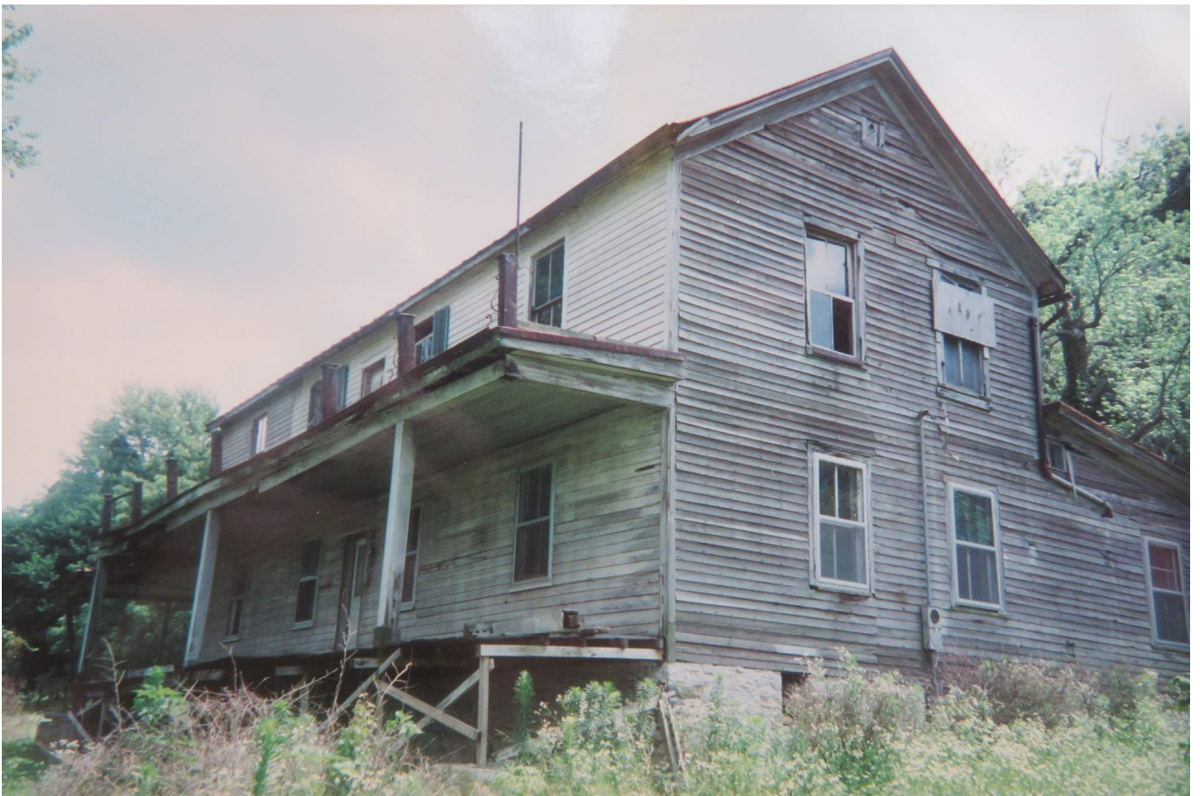
Figure 29. Photograph c. 1995, looking southwest, showing the poor condition of the house and the collapsing double porch. (Source: MoDNR Felix Vallé House archives)
