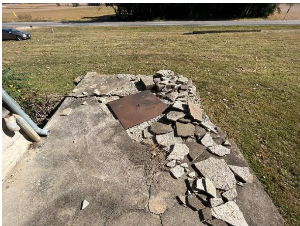
Photo 58. Cistern at the southeast corner of the house, with a metal cap and distressed concrete.
