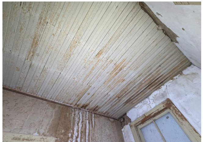
Figure 194. Beadboard ceilings with water damage in Room 202. (Source: RRJ 2023)
