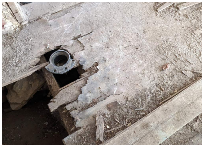
Figure 160. Failed flooring around plumbing riser. (Source: RRJ 2023)
