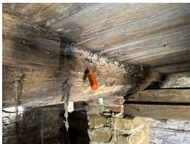
Figure 11. Floor beam B15. Note moisture stains on the flooring boards and the beam. Surface wood decay is confirmed by probing with an awl.
