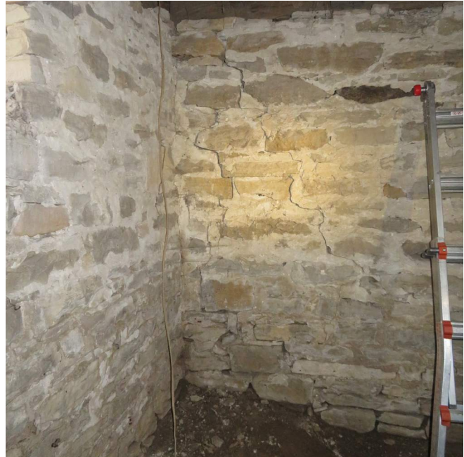
Figure 129. Step cracking and mortar deterioration at the northwest corner of the basement limestone foundation wall. (Source: RRJ 2023)
