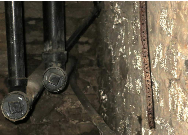
Figure 216. Existing sanitary pipes routing along west wall to the south existing wall where lines extend through foundation wall. (Source: Alvine 2023)
