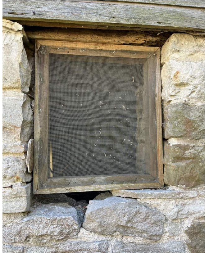
Figure 107. W001B, a basement level window on the north exterior wall, showing deterioration of the frame and masonry. (Source: RRJ 2023)
