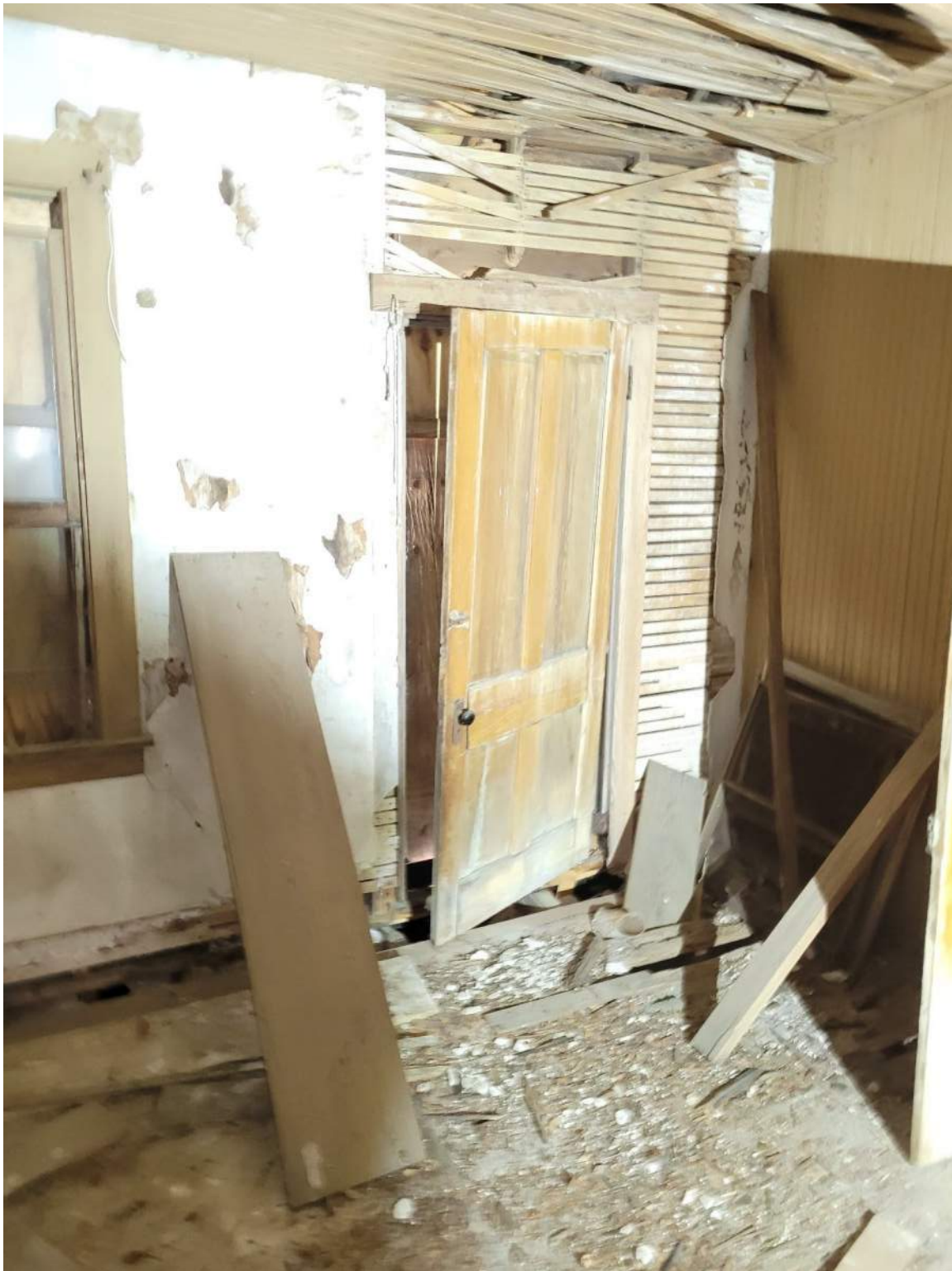
Photograph 5: LBP door, door frame, and ceiling Room 101.
