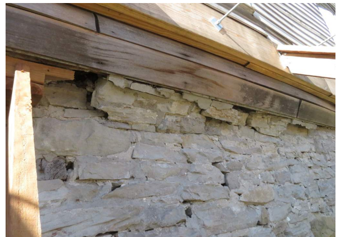
Figure 128. Displacement of the top course of stone masonry due to distress of the east log wall. (Source: RRJ 2023)
