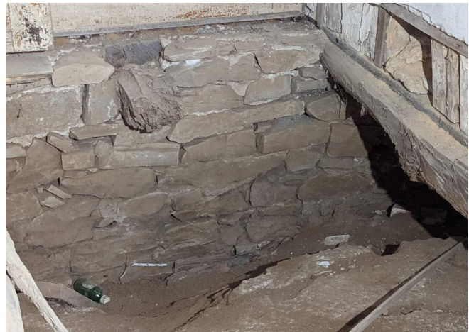
Figure 130. Deterioration of mortar joints at the west foundation wall/demising wall between Rooms 103 and 104 (Source: RRJ 2023)
