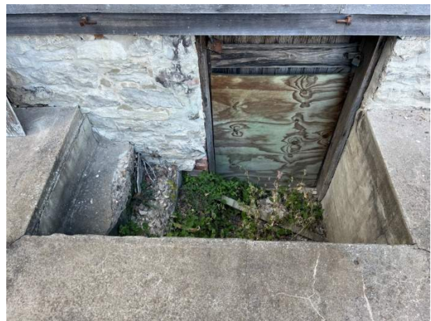
Photo 55. Deteriorated concrete topping at steps to south basement entrance.
