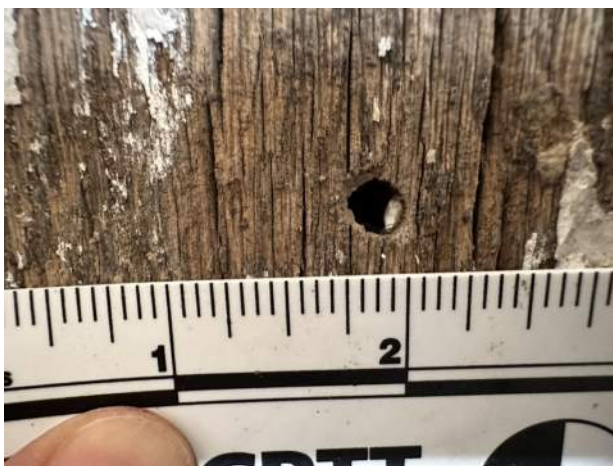
Figure 8. Large wood-boring beetle emergence holes measuring 1/4 inch in diameter.
