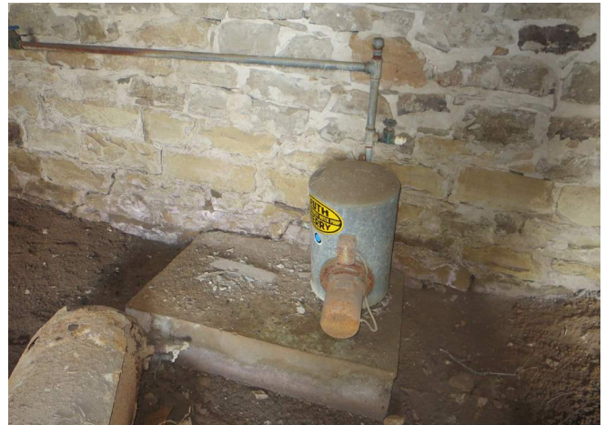
Figure 213. Photo of existing abandoned water pump located on concrete pad in Basement level in house.. (Source: Alvine 2023)
