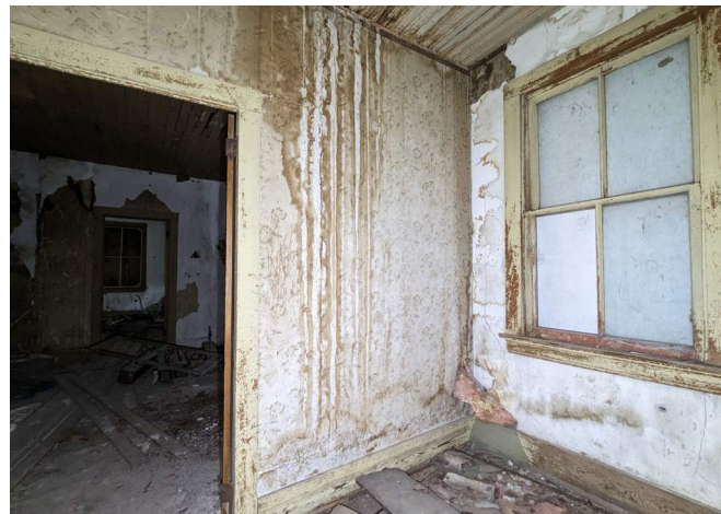
Figure 191. Room 202, looking northeast, showing the damage to the walls and flooring from the previous roof leak. (Source: RRJ 2023)
