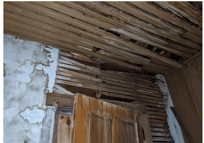
Figure 137. Damage to roof framing and wall framing in Room 202. (Source: RRJ 2023)
