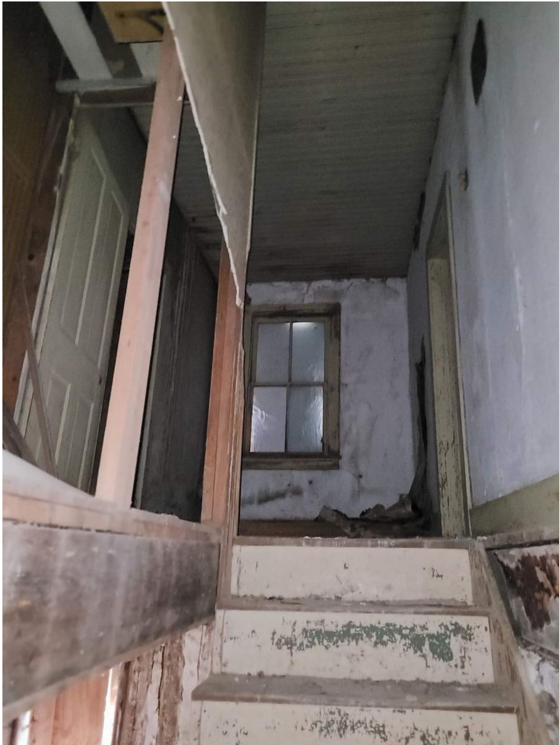
Photograph 17: LBP tread, riser, window, window frame, baseboard, and closet wall Room 202.
