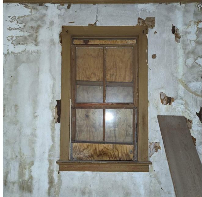
Figure 117. W203B, a second floor window on the east wall with damaged but intact upper and lower sashes with glazing. (Source: RRJ 2023)
