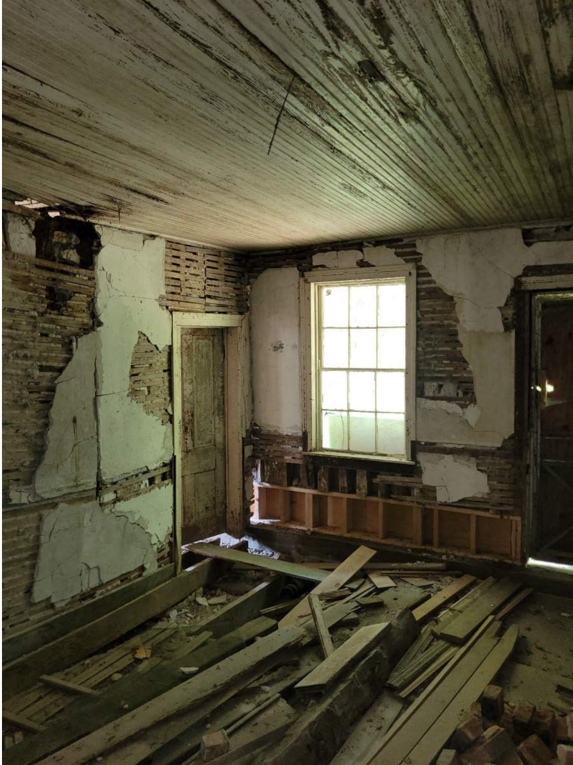
Photograph 12: LBP baseboard, window, window frame, and ceiling Room102.
