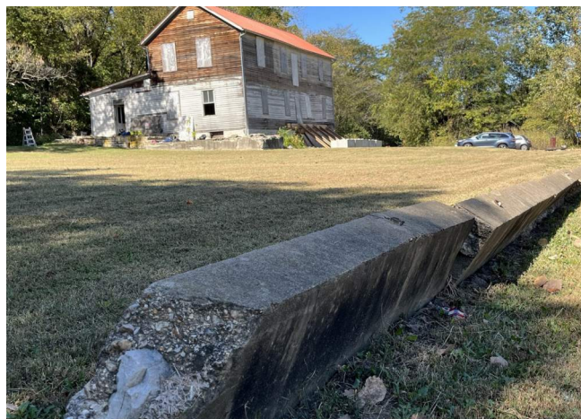
Figure 89. Displacement and distress to the concrete retaining wall, looking north. (Source: RRJ 2023)
