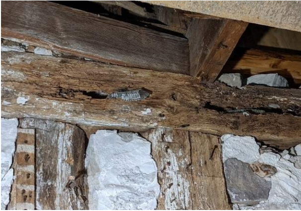
Photo 28. East wall top plate distress within room 105. Pest and water damage to the top plate has created large voids in the timber section, allowing for further animal-related deterioration as evidenced by snakeskin caught between rough surfaces.
