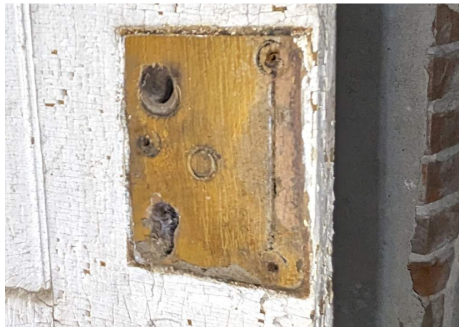
Figure 153. Faux graining exposed on the north face of D104. (Source: RRJ 2023)
