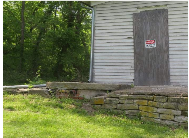
Photo 59. Cistern at the southwest corner of the house, with a stone cover and distressed stone and brick masonry.
