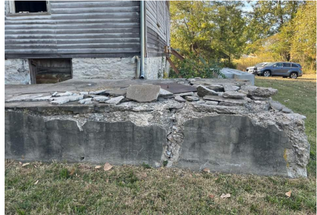
Photo 53. South view of deteriorated concrete topping at south elevation.
