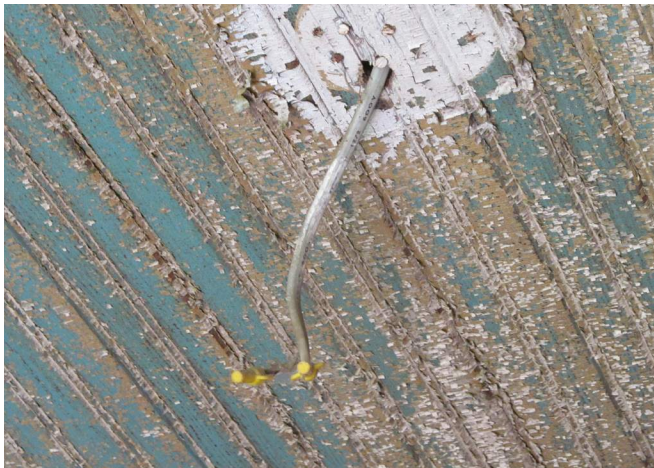
Figure 226. Photograph of remaining non-metallic sheathed cable. (Source: Alvine 2023)
