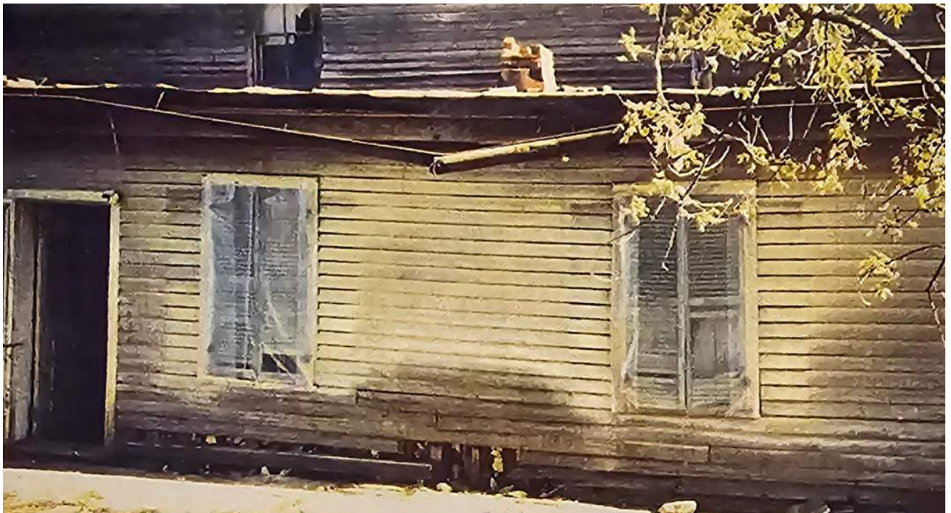
Figure 29. 2000 photograph of the west exterior, showing the deterioration and deformation of the sill plate in Rooms 101 and 102 prior to the stud wall repairs. (Source: Volz and Associates, "Pierre Delassus de Luziere House (Kern House) Condition Assessment Report").
