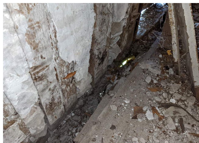
Figure 136. Displacement of the east wall of Room 105, looking at base of wall at failed sill plate. (Source: RRJ 2023)
