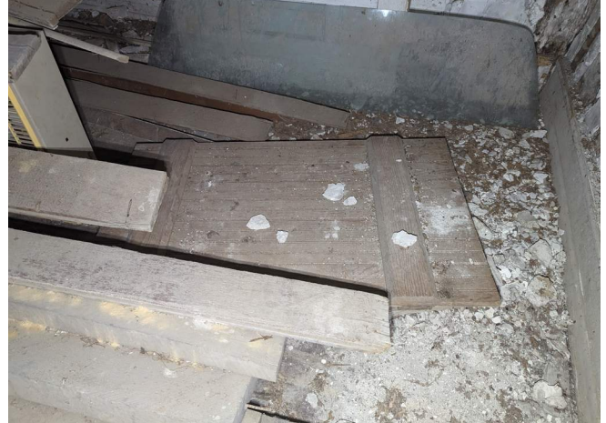
Figure 119. Small batten-style shutter in the debris in Room 104 (Source: RRJ 2023)
