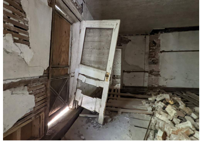
Figure 103. Door D201A, the back door, in a failed condition. (Source: RRJ 2023)
