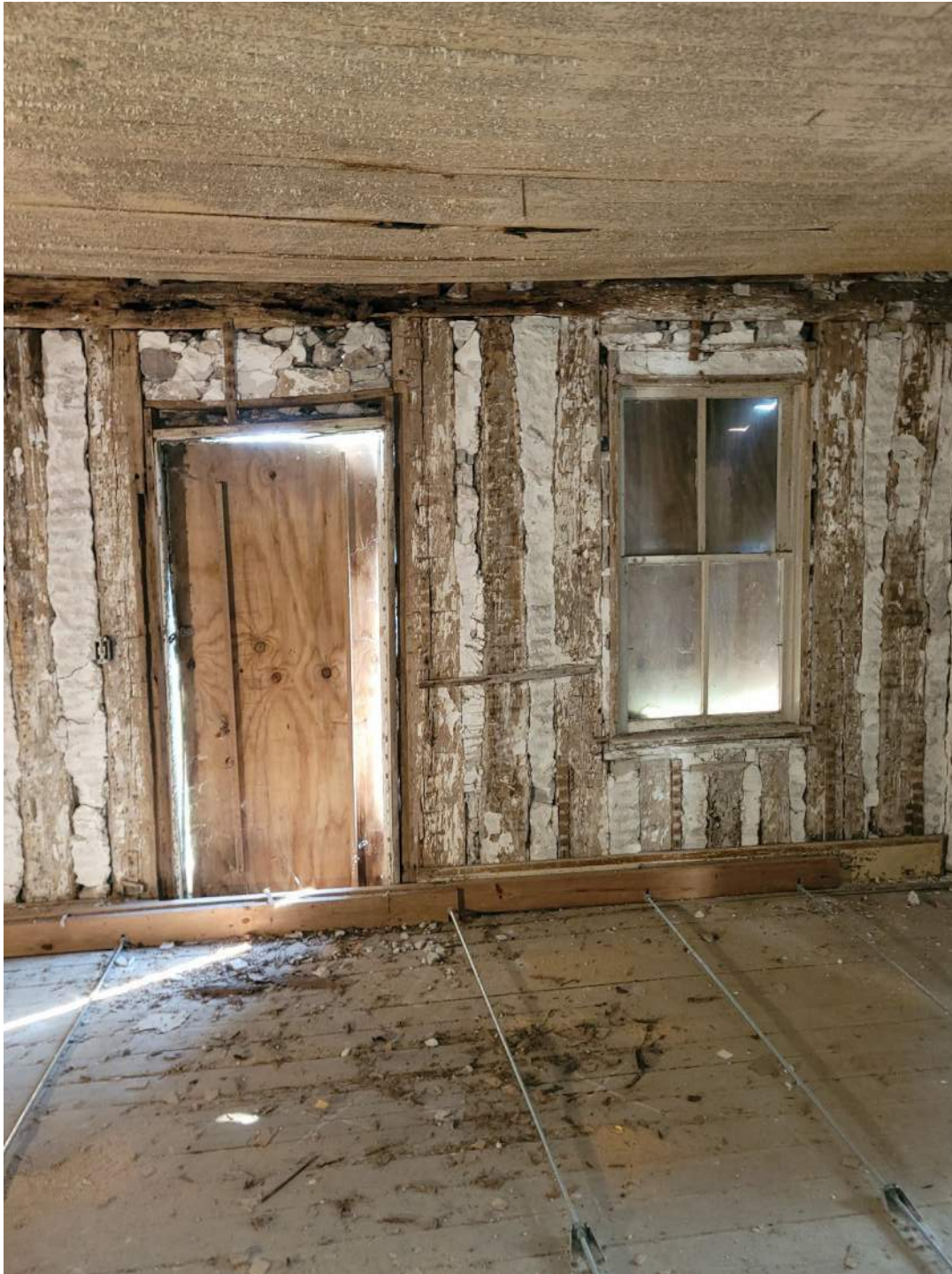
Photograph 10: LBP baseboard, window, window frame, ceiling Room 105.
