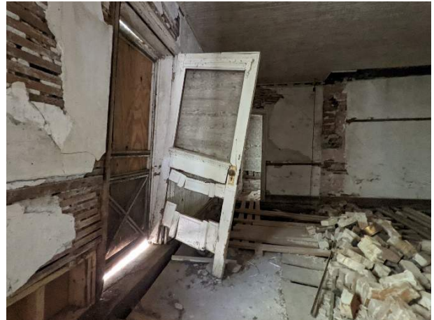
Photo 87. Door 102A with ornamental panels in failed condition.
