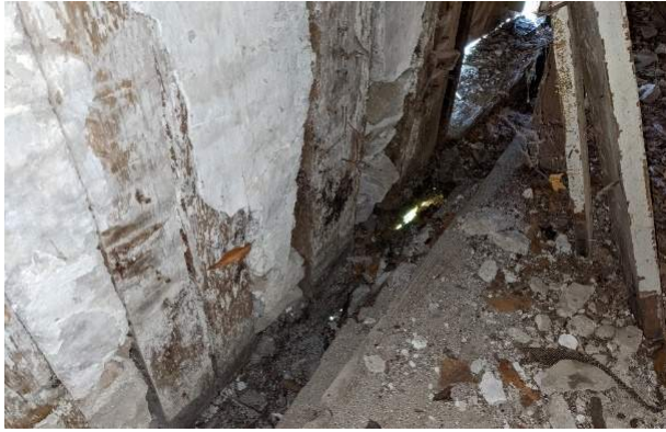
Photo 30. East wall bottom plate distress near exterior door within room 105. The bottom plate has split vertically, crushed, rotated, and deteriorated as the vertical log wall moved out of plane, exposing the notched lower ends of vertical logs. Daylight is visible below the door threshold.
