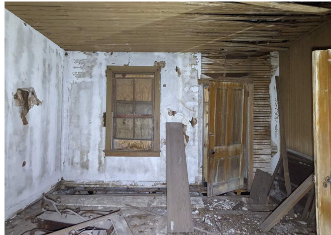
Figure 196. Room 203, looking east towards the water damage to the ceiling, walls, and flooring around the door. (Source: RRJ 2023)
