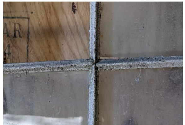
Photo 84. Delicate muntins at the 6-over-6 windows. Further research is needed to determine an approximate age of these window units compared to the 2-over-2 units.
