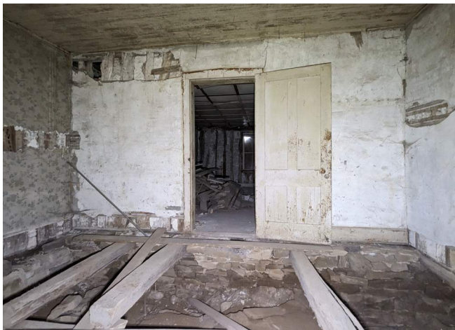
Figure 46. Room 103, looking east, showing missing floor framing. (Source: RRJ 2023)
