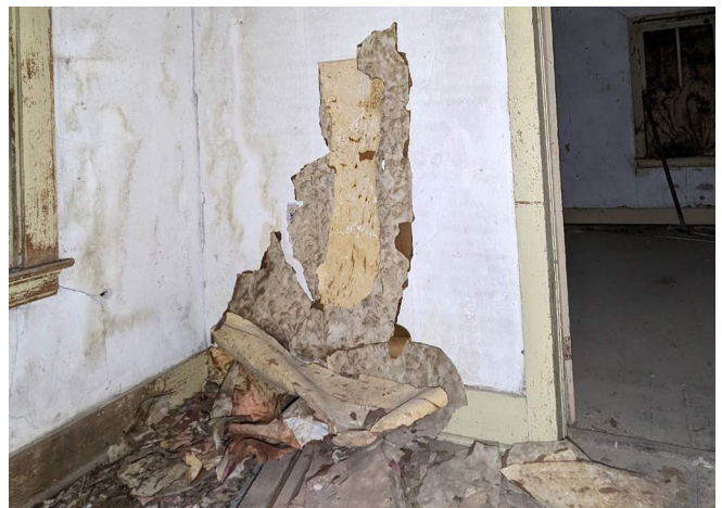
Figure 195. Multiple layers of wallpaper were present in the southeast corner of Room 202. (Source: RRJ 2023)
