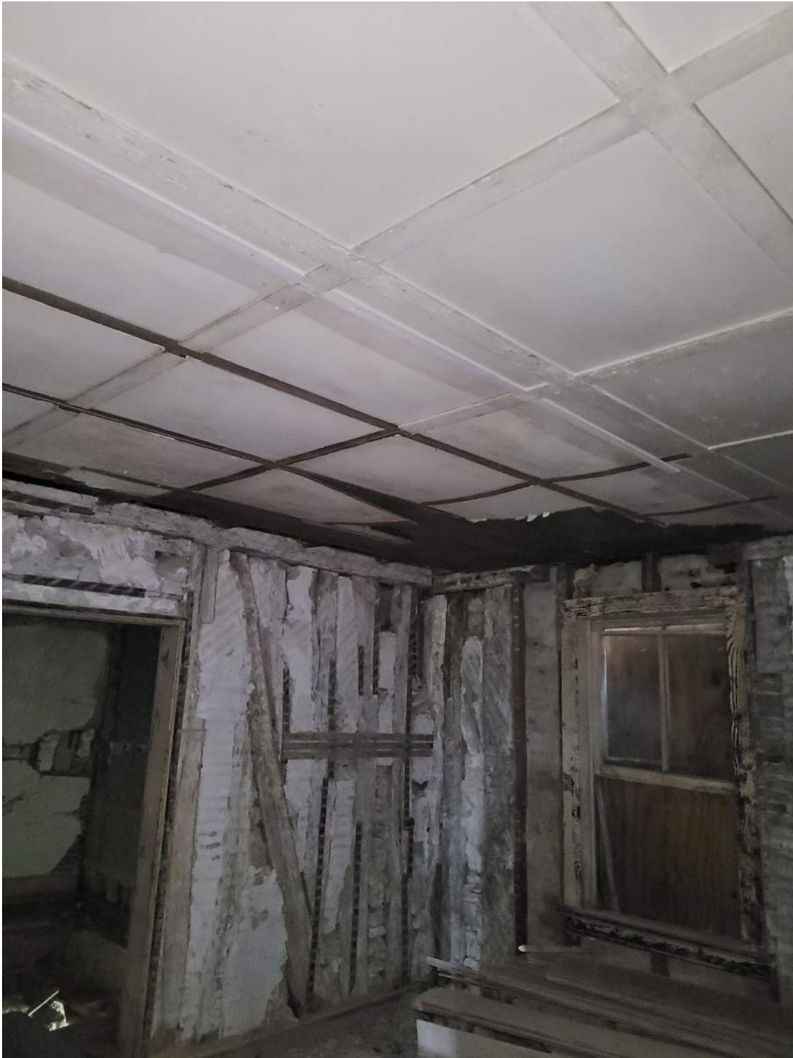
Photograph 14: LBP door frame, door, window, window frame, ceiling board and ceiling Room 106.
