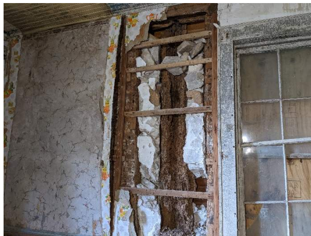
Photo 75. Termite damage to vertical logs in Room 101.
