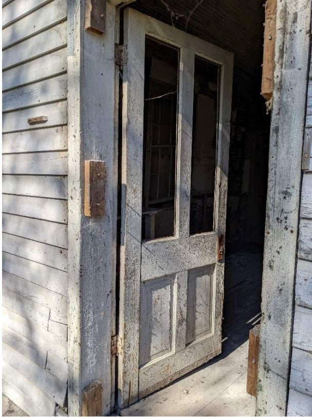
Photo 85. Door 101A, missing hardware and glass.
