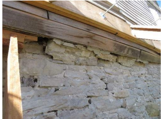
Photo 35. Lateral displacement of the outer course of the east masonry foundation wall near the middle of the wall.
