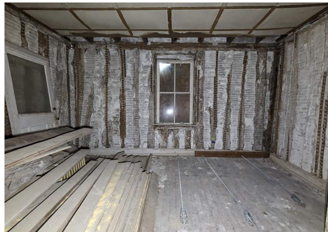
Figure 171. Room 104, looking east towards the distressed east wall. (Source: RRJ 2023)
