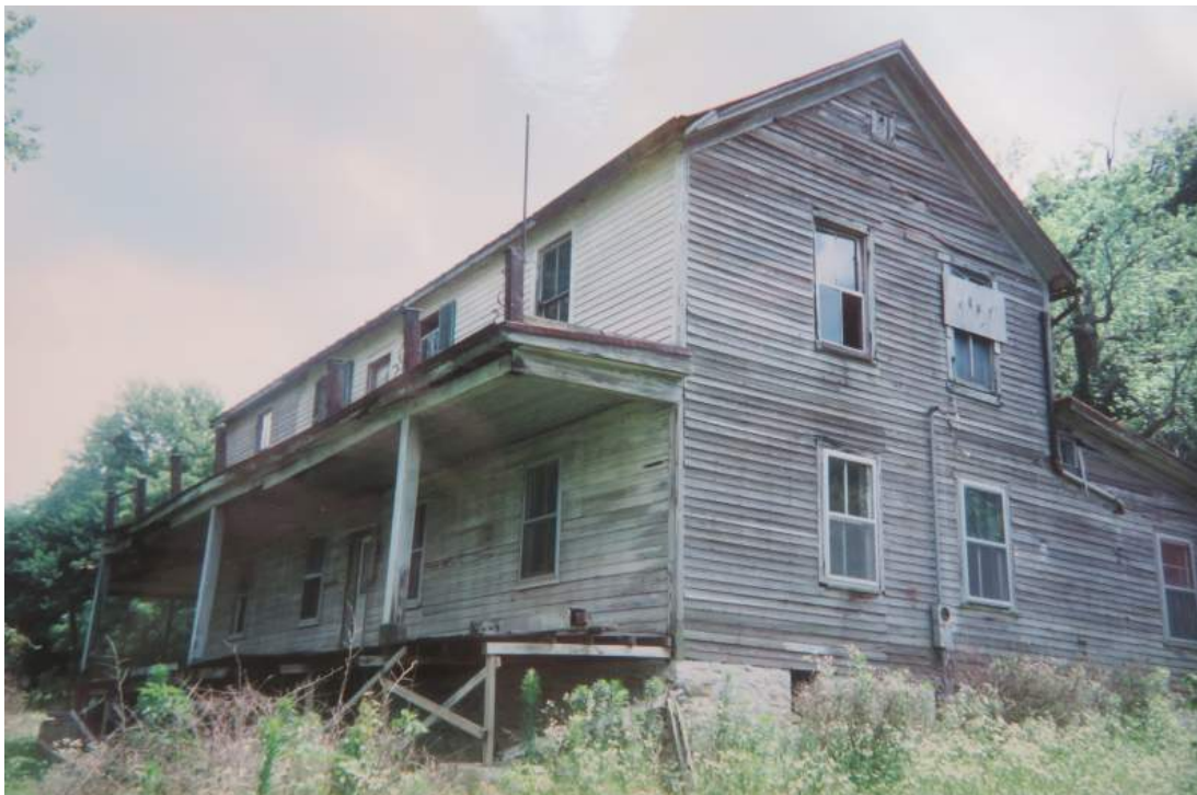
Figure 31. Photograph c. 1995, looking southwest, showing the poor condition of the house and the collapsing double porch. (Source: MoDNR Felix Vallé House archives)
