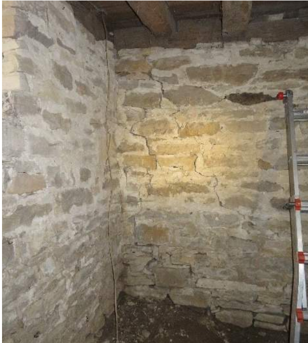
Photo 37. Step cracking at northeast corner, east wall viewed from basement.
