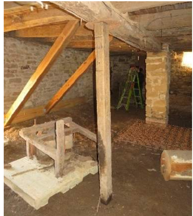
Photo 47. Timber post at girder center exhibits some wood decay at the post/soil intersection.
