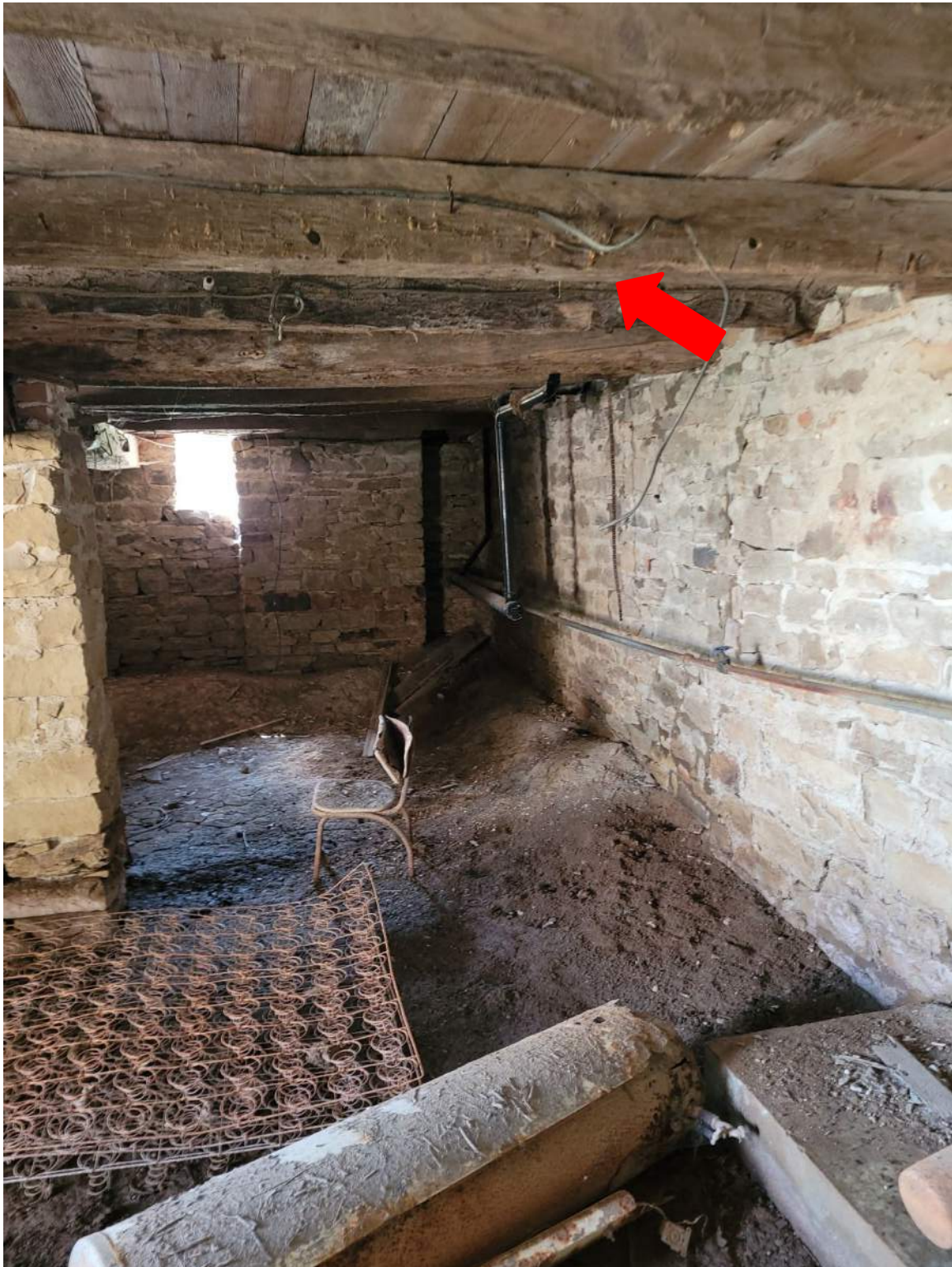
Photograph 23: Non asbestos electrical wiring in basement Room 001.
