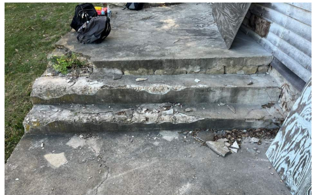
Photo 54. Deteriorated concrete topping at steps to south entrance.
