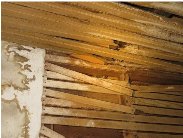
Photo 51. Top plate distress above exterior wall at second floor.
