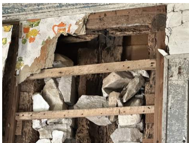
Figure 5. Severe deterioration and void in the vertical wall logs and top plate on the west wall. Room I.
