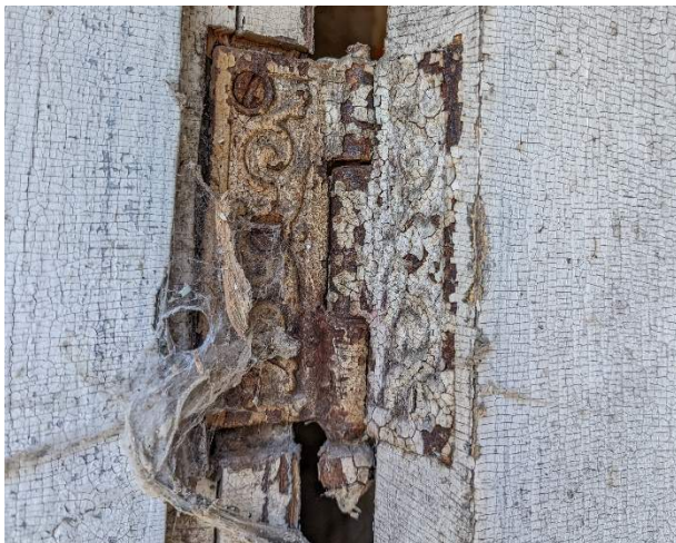
Photo 86. Historic but not original hinge at Door 101A.
