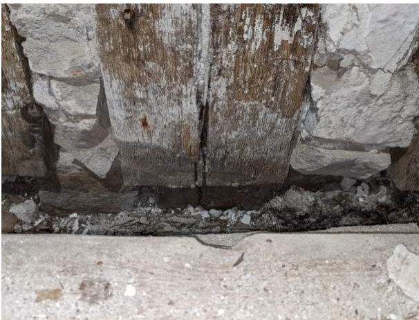
Photo 24. Lower termination of vertical log walls within room 105. The tenon at the log end is visible where the sill plate has heavily deteriorated.
