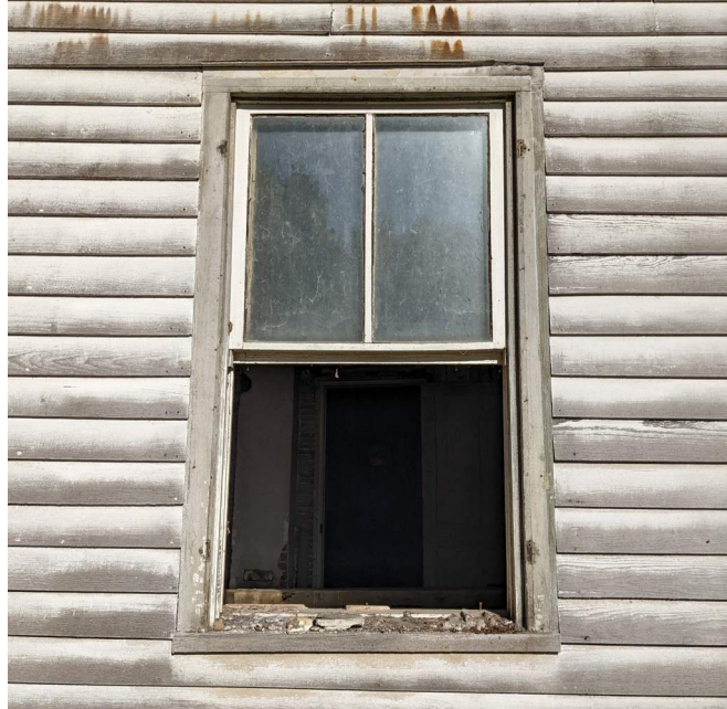
Figure 113. W106B, a first floor window on the south wall with a missing lower sash but intact upper sash, dating to the 1903 alterations to the house. (Source: RRJ 2023)
