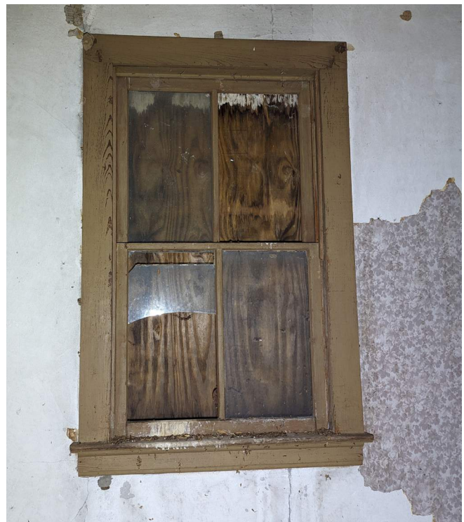
Figure 118. W204A, a second floor window on the west wall with relativelyt intact upper and lower sashes with damaged glazing. (Source: RRJ 2023)
