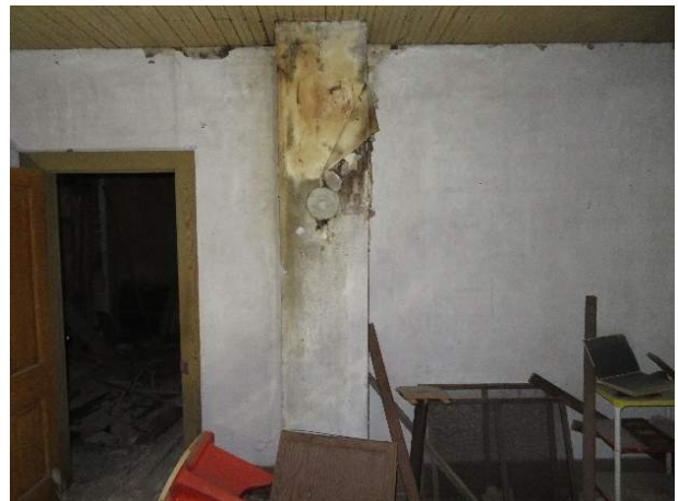
Photo 40. Interior chimney within Room 204 exhibiting moisture-related deterioration to finishes.
