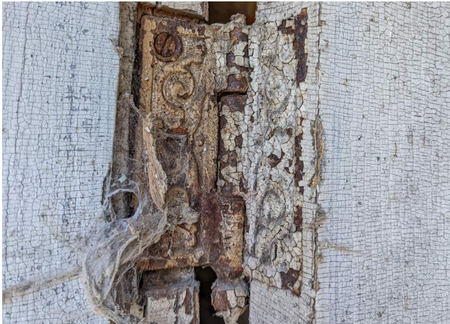
Figure 102. Replacement hinge on Door D101A. (Source: RRJ 2023)
