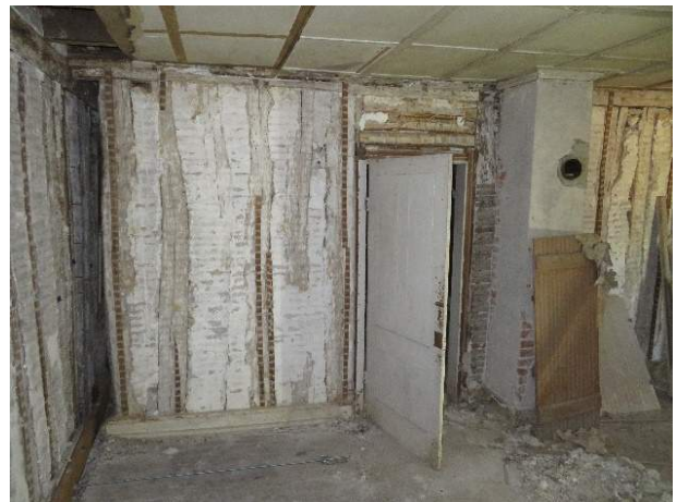
Photo 29. Pierrotage has dislodged where the east-west interior wall separating rooms 104 and 105 abuts the laterally displaced east exterior wall (gap at left).
