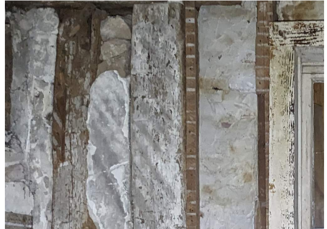
Figure 173. Marks from now missing diagonal lath, possibly an earlier plaster application, which would have been to the left side of the stone masonry chimney (now missing). (Source: RRJ 2023)
