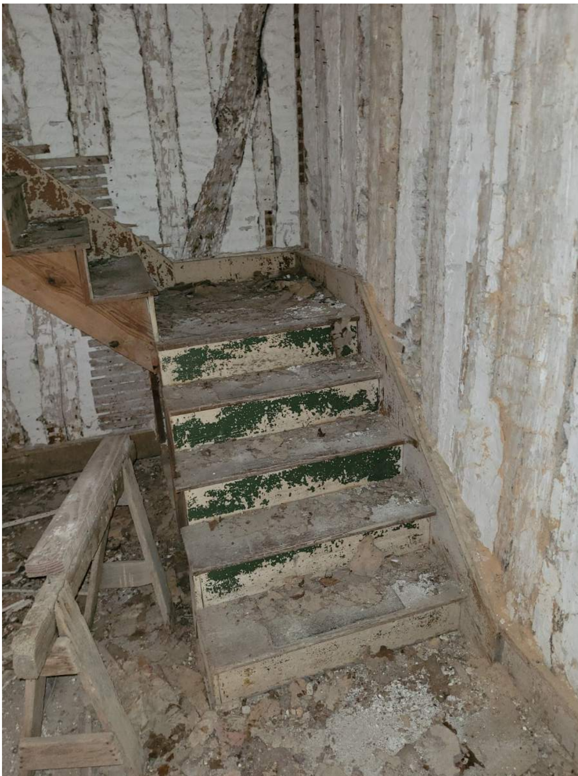
Photograph 9: LBP stair, tread, and stringer Room 105.
