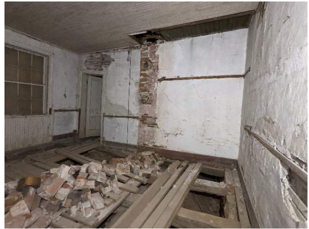
Photo 39. The interior chimney within Room 102 has collapsed or been disassembled.
