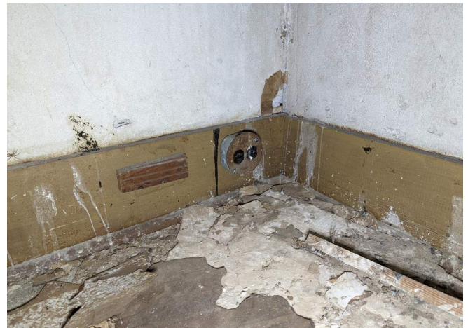
Figure 200. Baseboard with an old electrical receptacle. (Source: RRJ 2023)
