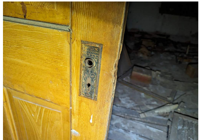
Figure 155. Faux graining and ornamental escutcheon on D204. (Source: RRJ 2023)
