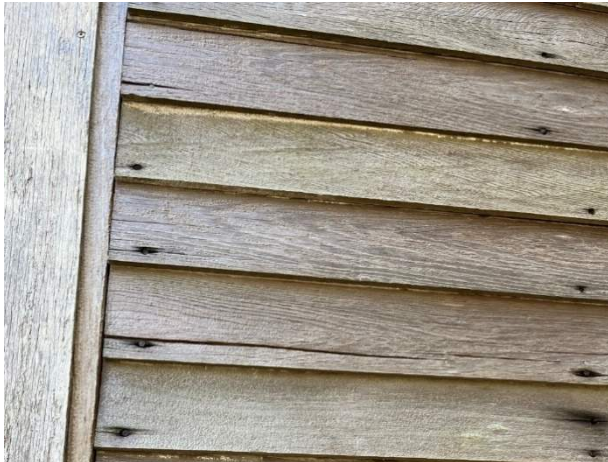
Photo 81. General weathering of lap siding and one split board of siding at north wall.
