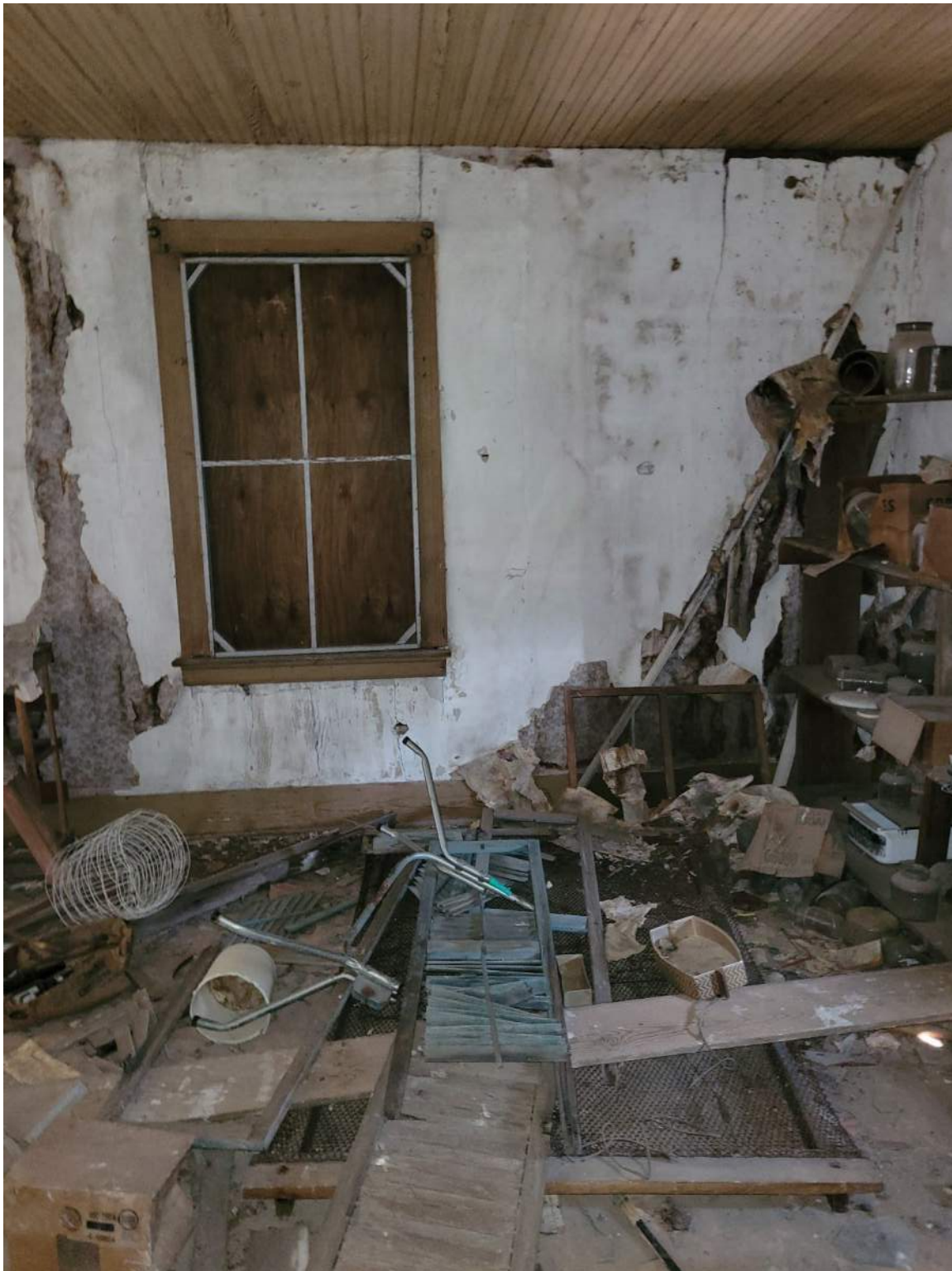
Photograph 21: LBP window, window frame, and baseboard Room 204.
