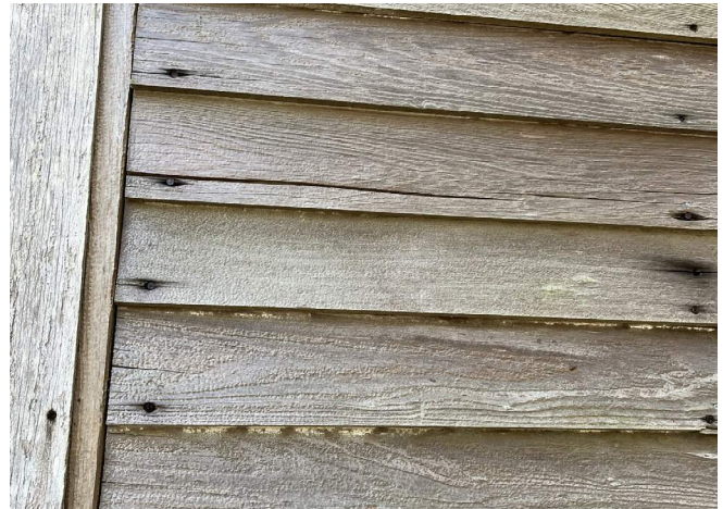
Figure 97. Weatherboard siding, showing exposed nails, along with splits in the wood boards. (Source: RRJ 2023)
