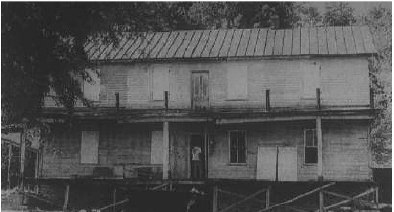
Figure 33. October 1998, showing the continued deterioration of the exterior. (Source: Evans, Mark. "DNR Ties to Unravel Mystery of De Luziere House," Ste. Genevieve Herald (October 9, 1996): 1B.)
