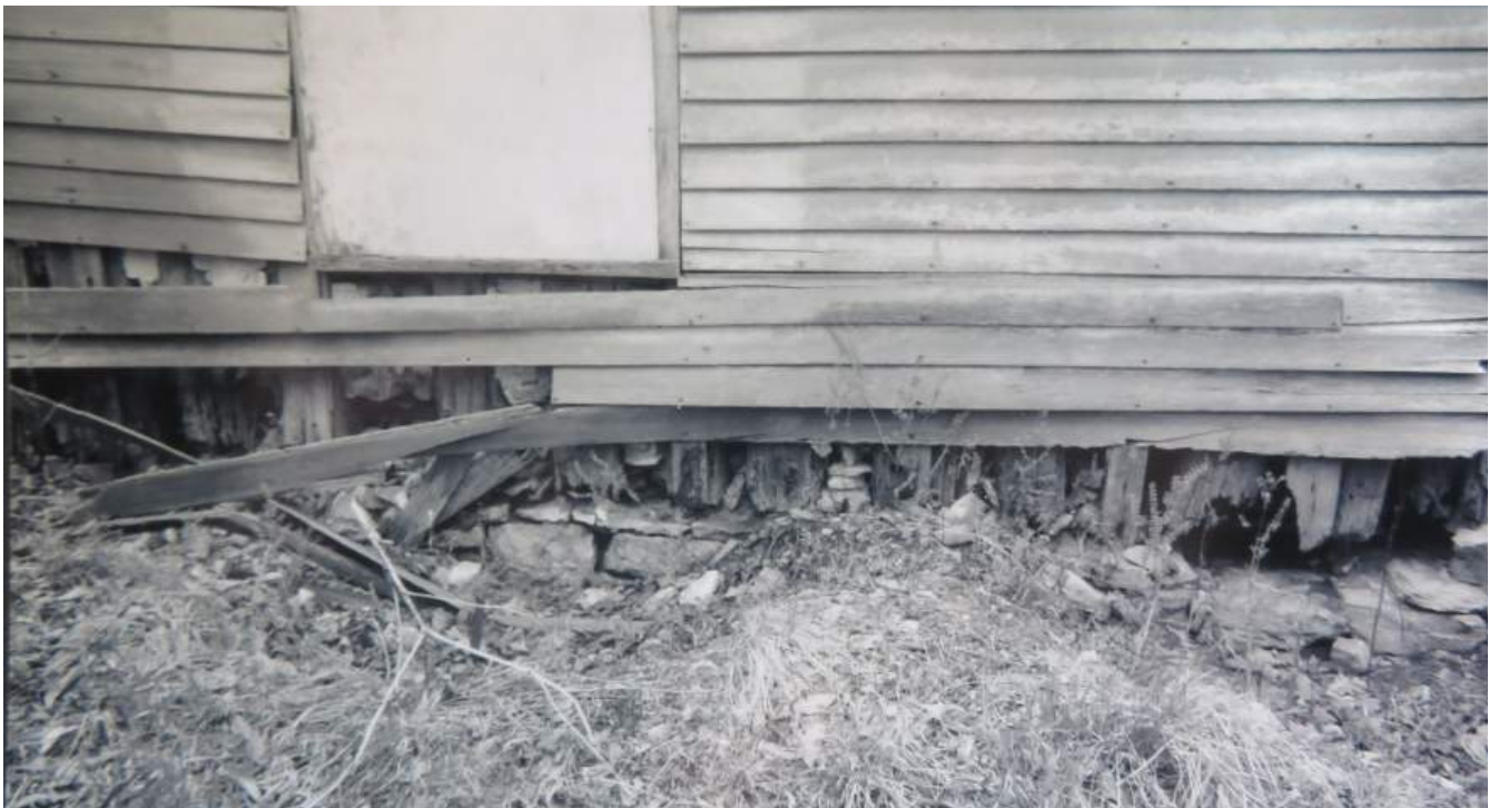
Figure 35. April 2007 photograph, showing the deterioration of the west wall sill plate and bottom of the vertical logs at Room 102. (Source: MoDNR Felix Vallé House archives)
