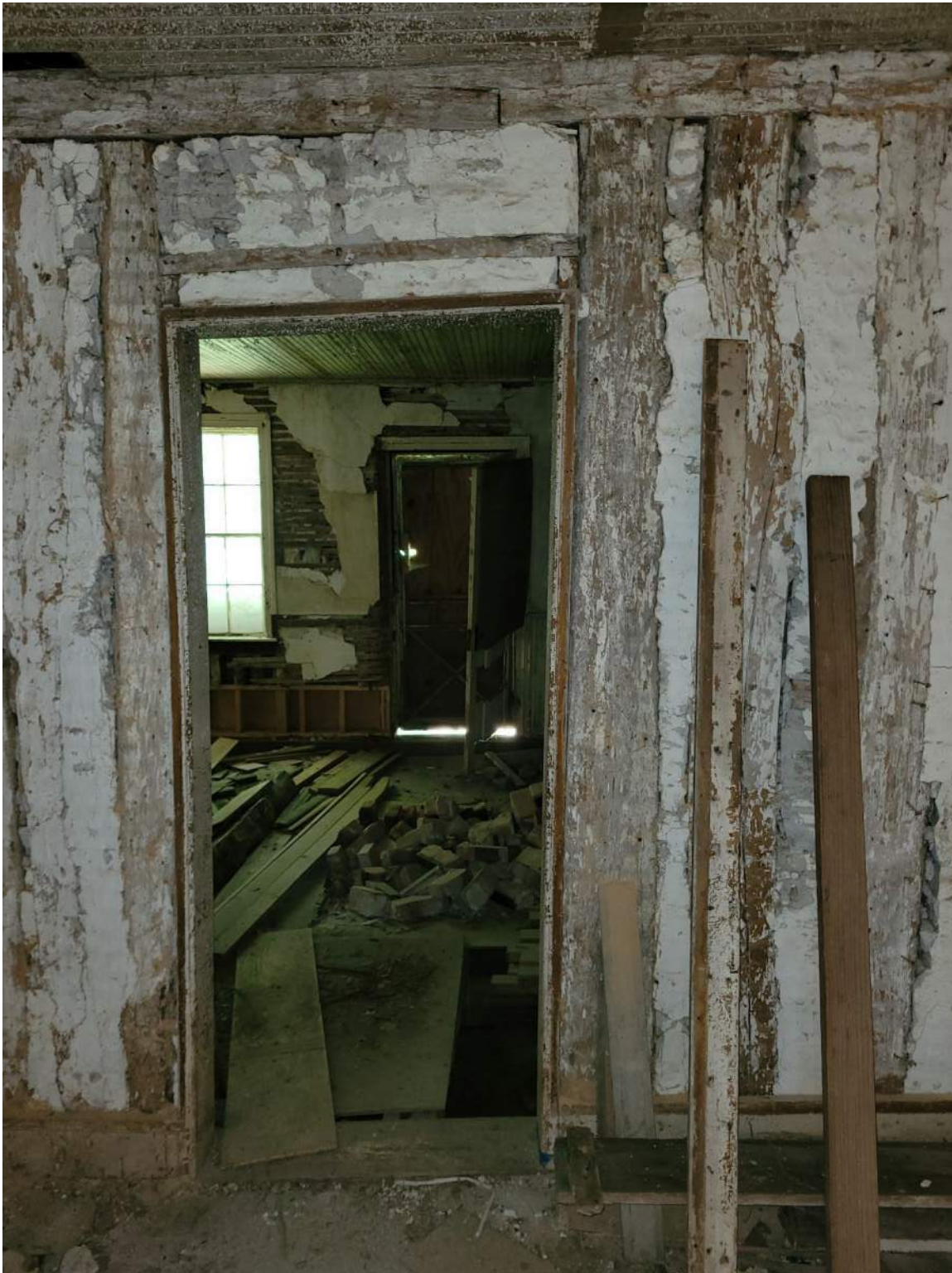
Photograph 13: LBP door frame, ceiling, baseboard Rooms 105 and 102.
