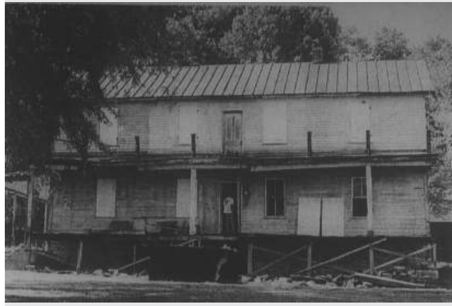
Figure 66. An image of the house from 1996 that shows the poor condition of the house from the flood damage. (Source: Ste. Genevieve Herald , October 9, 1996, p. H)
