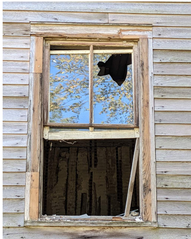
Figure 110. W104A, a first floor window on the east wall in failed condition, dating to the 1903 alterations to the house. (Source: RRJ 2023)
