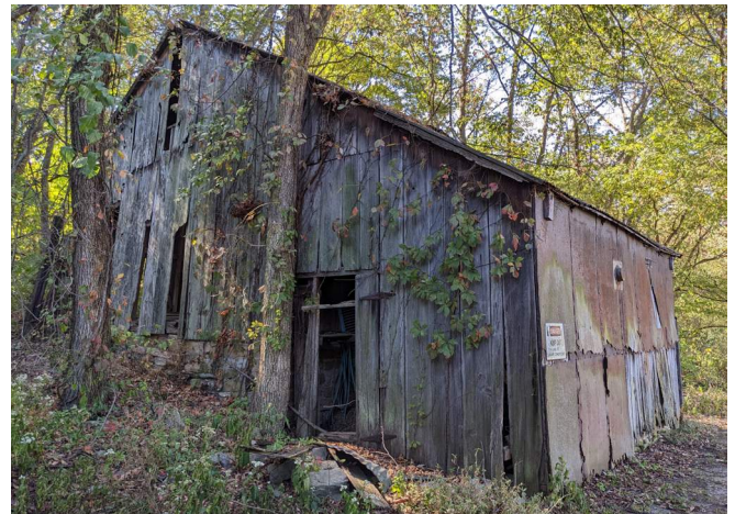
Figure 68. The woodshed from the south, showing deterioration of the wood siding and structure. (Source: RRJ 2023)
