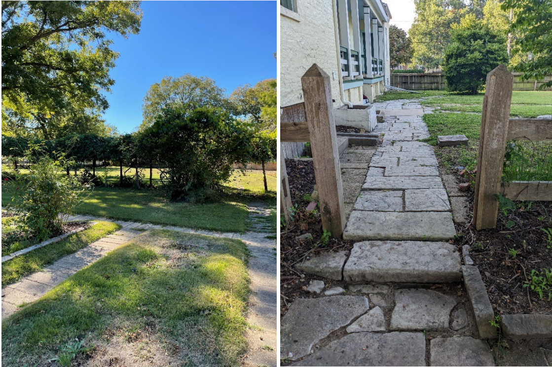
FIGURES 140 AND 141. Landscape pathways vary in dimensions and condition of materials. (Source: LSHLA, October 2022)
