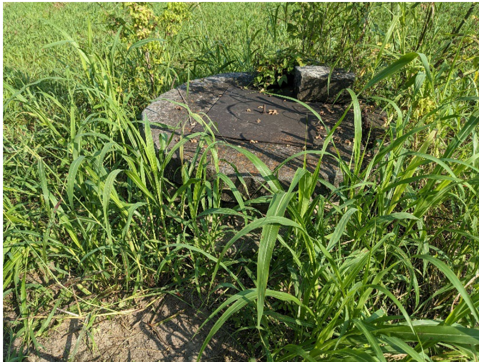
FIGURE 249. View of the well in the field north of the house.
