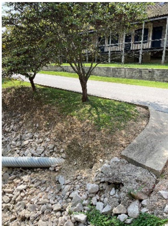
FIGURE 121. Riprap has been used along the banks of South Gabouri Creek to mitigate erosion and undercutting resulting from regular flooding. Drainage infrastructure empties into the creek from adjacent St. Marys Road.
