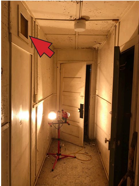
Figure 4.48. R107 looking east, February 25, 2020. Note closed-up door opening below mesh screen on north wall. (Image by author)
