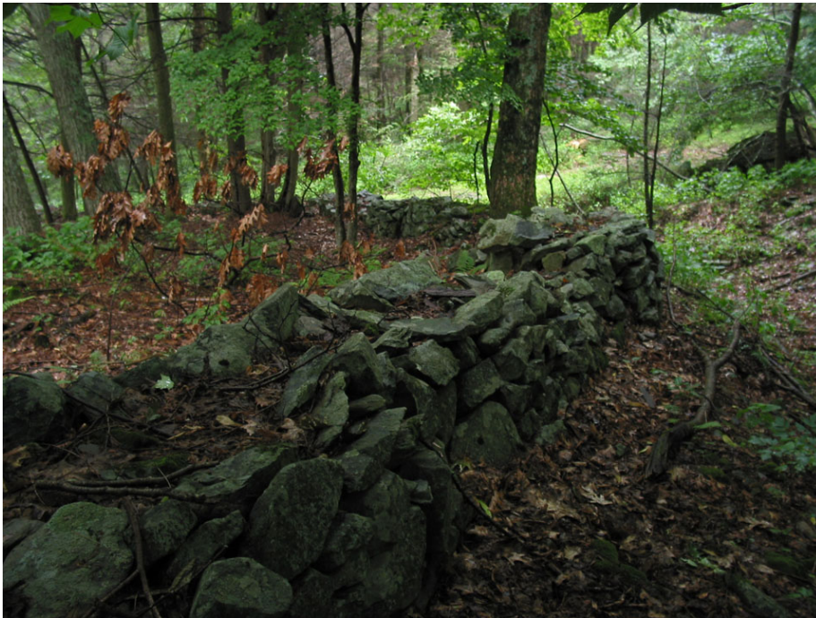
Figure 21: Stone walls and planting areas at the Judd Gardens are in poor condition (OCLP, 2006).
