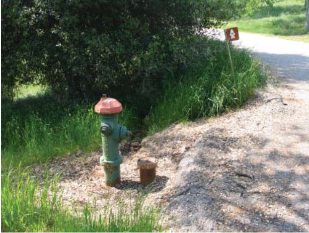
Buckeye Fire Hydrant (typical) (Undetermined)
