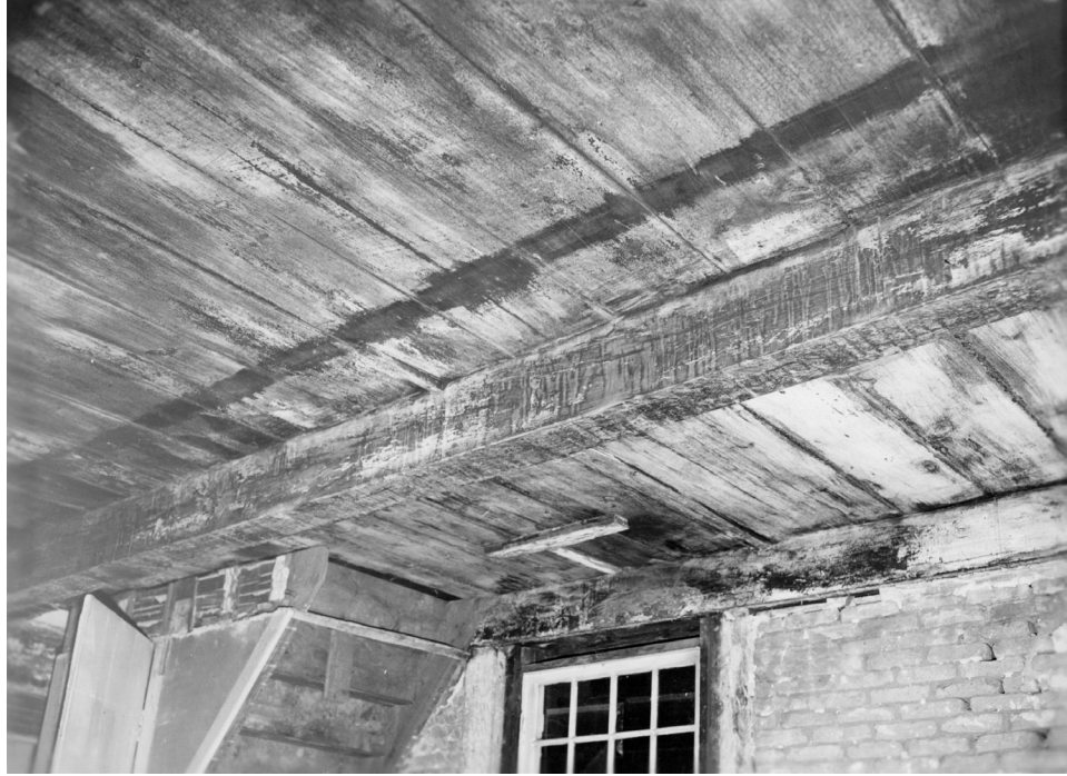
Figure 38. View of the kitchen ceiling, looking southwest, with a clear ghost of a partition that extends southward beyond the door to the enclosed stair to the garret. Photograph by Charles Hutchins, 1958. SARA.
