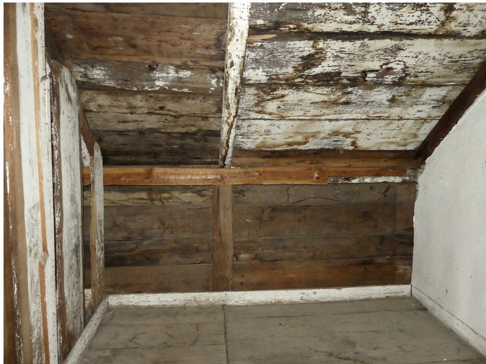
Figure 112. South room (207), looking south. Note the original brick nogging has been removed (compare with Figure 46). JGWA, 2019.
