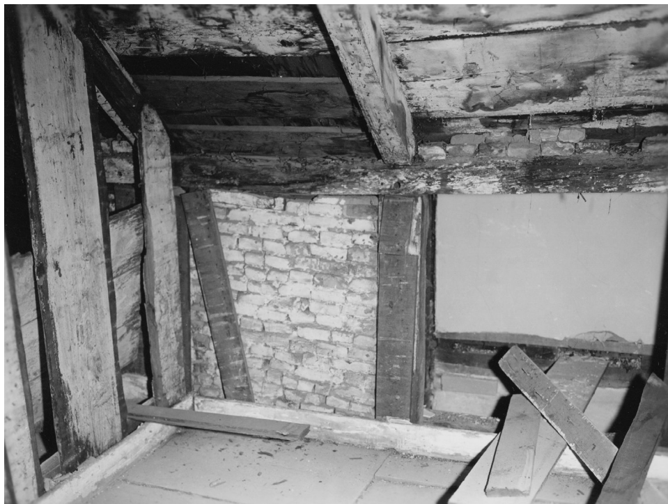
Figure 47. The kitchen plate and rafters below the south cricket in 1958. The deterioration was such that Judd recommended replacing these members. The brick nogging was removed in the 1963 restoration work. Photograph by Henry Judd. SARA.
