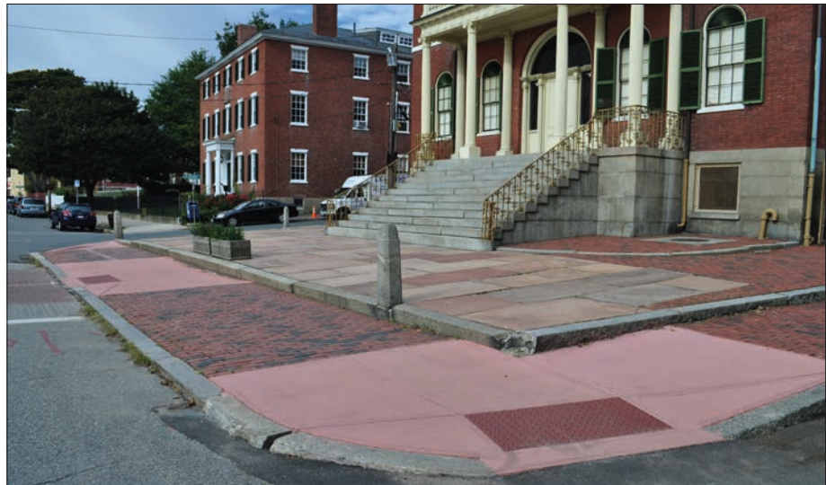
Figure 144. Existing condition of a hazard created by the city's sidewalk modifications in 2012. The step between the Custom House terrace and Derby Street sidewalk drops ten inches and is unsafe. The park placed planter boxes at the edge of the terrace to protect pedestrians, June 2015 (OCLP).
