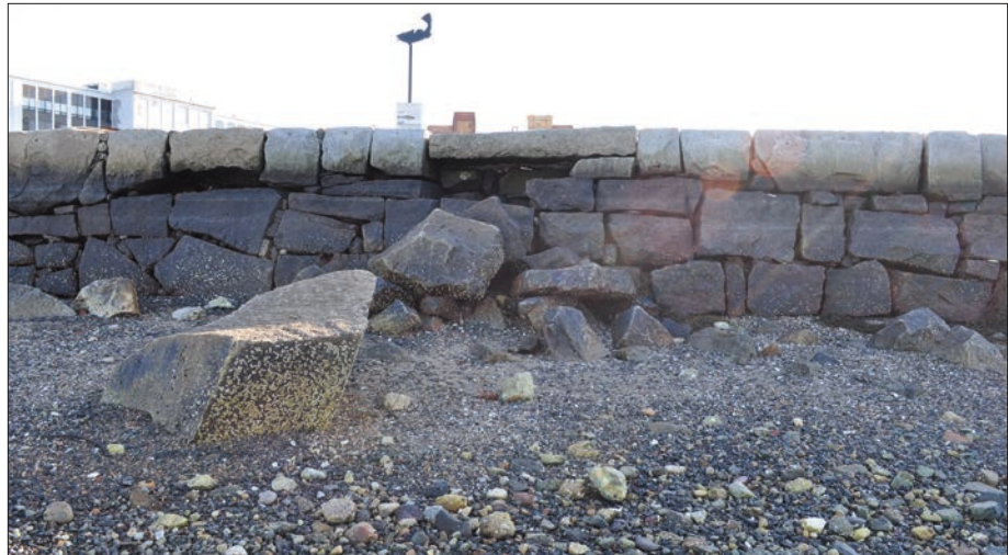
Figure 185. View looking west of granite blocks pulled out of Derby Wharf seawall by storm waves in section that is 700 feet from Derby Street. The top course remains intact due to the steel pins, June 2015 (OCLP).
