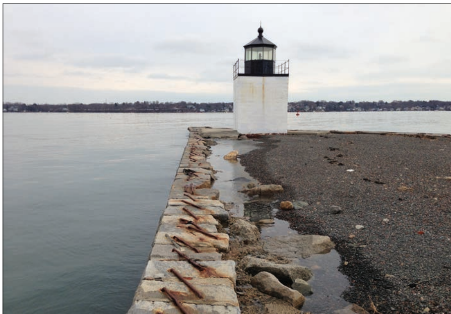
Figure A.28. Looking south at erosion and over-wash damage on the eastern side of Derby Wharf near the lighthouse during an exceptionally high tide, February 2013 (OCLP).
