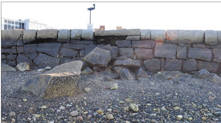
Figure A.06. View looking west of granite blocks pulled out of Derby Wharf seawall by storm waves in section that is 700 feet from Derby Street. The top course remains intact due to the steel pins, June 2015 (OCLP).
