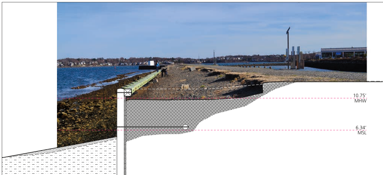
Figure A.22. Existing condition of eastern side of Derby Wharf showing erosion (OCLP).
