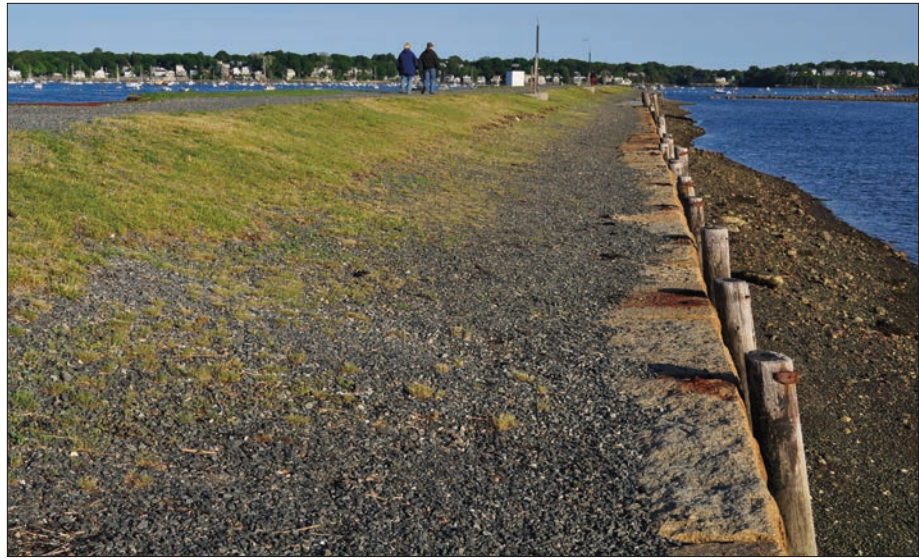
Figure A.16. View looking south along west side of Derby Wharf about 1,500 feet from Derby Street. Timber piles aid in retaining the granite block retaining wall. Gravel washed from the access road during storm surges settles above the wall, June 3, 2015 (OCLP).
