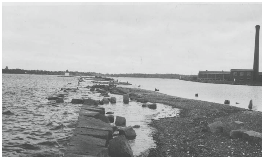
Figure A.26. Looking south at Derby Wharf in poor condition in April 1937 prior to rehabilitation by the National Park Service in 1938–39. Without maintenance or rehabilitation, the wharf will return to this condition (Allan Rinehart, National Park Service Collections, SAMA 14B-003).
