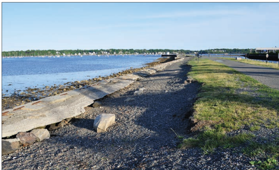
Figure A.27. Looking south at erosion and over-wash damage on the eastern side of Derby Wharf, June 2015 (OCLP).
