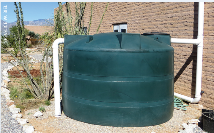
Rainwater harvesting tank at the Desert Research Learning Center.
