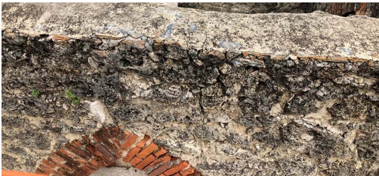
Figure 6.B.247: 203 S—West wall, exterior façade. Disintegrating edges, with associated detachment, and three cracks extended to the vertical wall.
