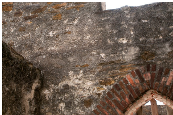
Figure 6.B.63: Room HS 203 D—South wall. Detail above the right bottom lancet arch features vegetation growth and erosion.
