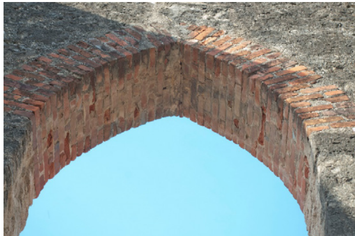
Figure 6.B.9: Room HS 203 S—South wall, upper-level lancet arch. Fragmentation of the bricks composing the arch.
