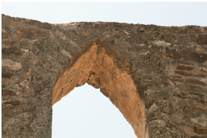
Figure 6.B.196: Exterior walls—North wall. Detail of the window W09 leading to room 203 D. It shows that the crack visible from the inside is not passing through the whole thickness of the wall.
