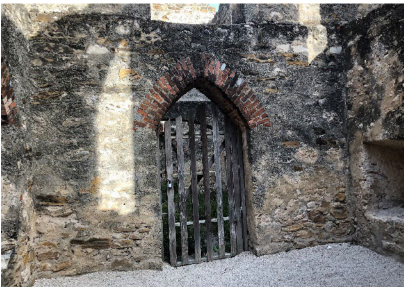
Figure 6.B.104: Room HS 203 B—West wall. Lower level general view, which exhibits biological growth in the upper part and erosion and missing parts in the lower part.
