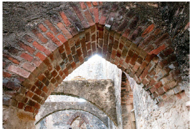
Figure 6.B.41: Room HS 203 A—East wall. Detail of the brick lancet arch, which features vegetation growth above and efflorescence in the intrados.
