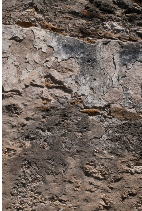
Figure 6.B.54: Room HS 203 D—North wall. Detail of the historic plaster remains just to the right of the window. The historic plaster features vegetation growth and detachment of edges.
