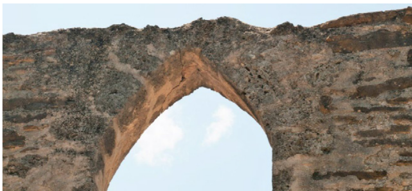
Figure 6.B.207: Exterior walls—North wall. Part corresponding to room 203 B. Left window (W12). Features the crack near the keystone that passes through all the thickness of the wall.
