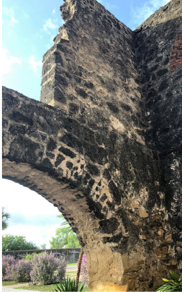
Figure 6.B.7: Room HS 203 S—East wall. The southeast corner has a thick layer of biological growth.
