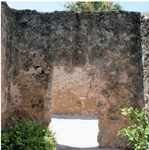
Figure 6.B.156: Room HS 203 H—South wall. General view. Features vegetation growth in the upper part of the wall and erosion in the lower part.
