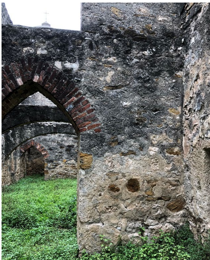
Figure 6.B.86: Room HS 203 C—West wall. Bottom right corner features biological growth, inconsistency in type of mortar used for repointing, erosion of the bottom part, and loss of mortar joints.
