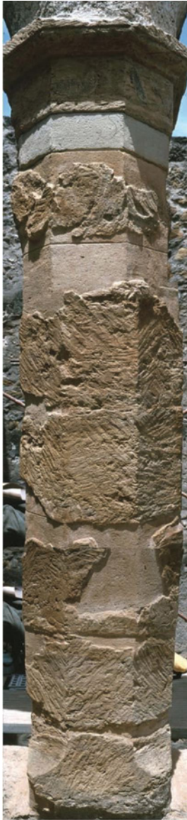
Figure 6.A.3 Reprinted from Evaluation of Proposed Consolidation Treatments for the San José Convento Column , by Kalen McNabb, 2012, p. 13.
