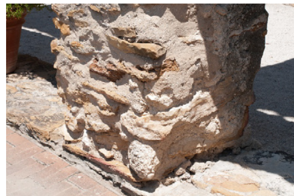
Figure 6.B.232: Exterior walls—Cloister south wall. Detail of the erosion and loss of mortar in the lower part of the pillars.
