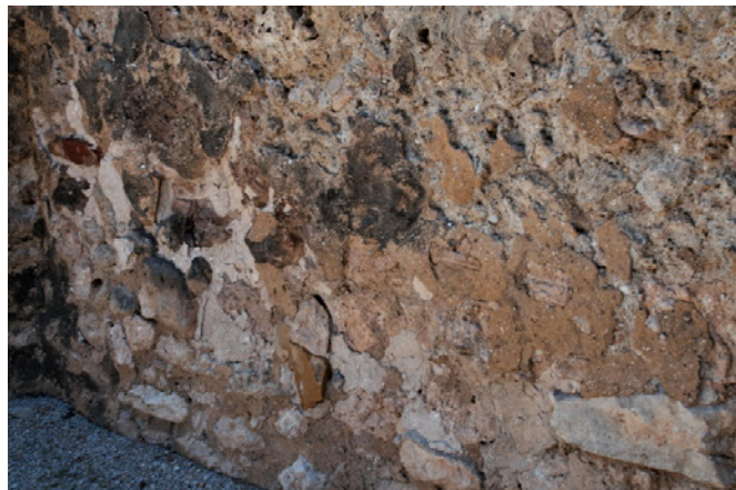
Figure 6.B.182: Room HS 203 R—East wall. Detail of the bottom part of the wall. Exhibits a high level of erosion of the wall and detachment of the patching.
