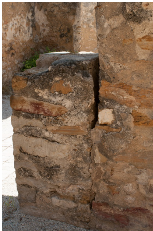
Figure 6.B.125: Room HS 203 E—South wall. Detail of the fracture in the connection of the south arcade and the parapet.
