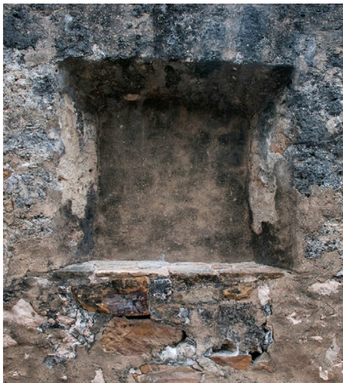
Figure 6.B.184: Room HS 203 R—South wall. Detail of the niche N05. Features biological growth surrounding it and erosion of the masonry wall, numerous holes and detachment of the patching in the area below the niche.
