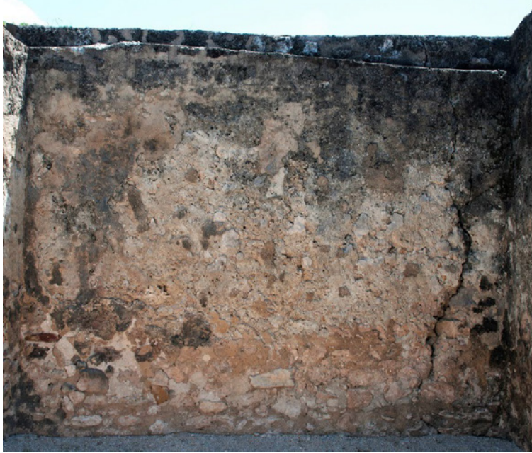
Figure 6.B.179: Room HS 203 R—East wall. General view. Exhibits a big fracture, biological growth in the upper part, erosion and roughly executed patching.
