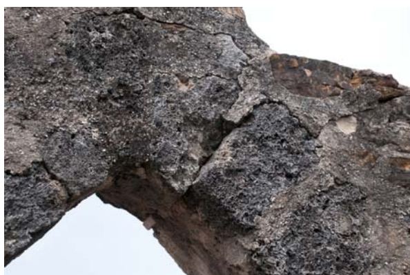
Figure 6.B.256: 203 B—North wall, Window 12. Fracture, with associated loss of restoration joint mortar.
