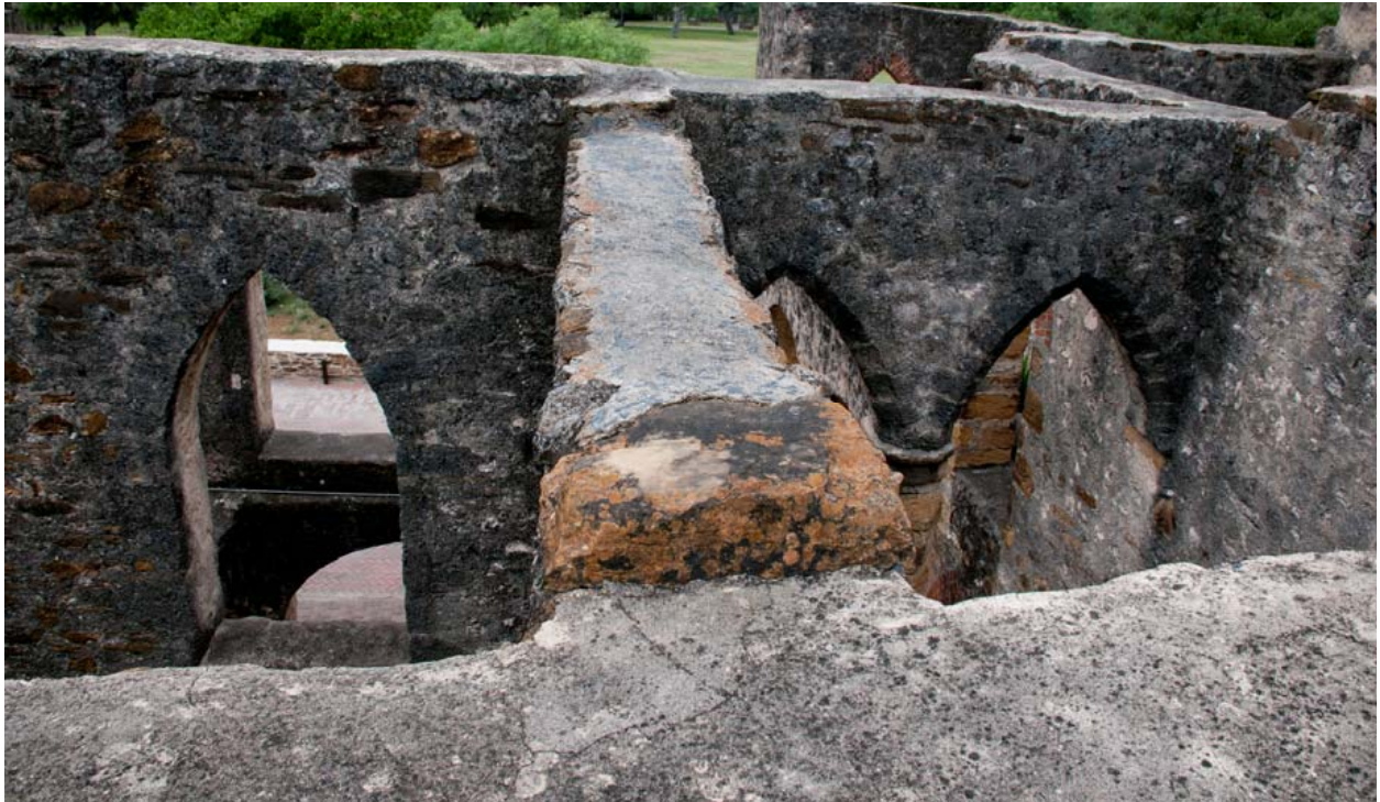
Figure 6.B.246: Wall between 203 A and 203 D—Disintegrating capping with detachment of the edges.
