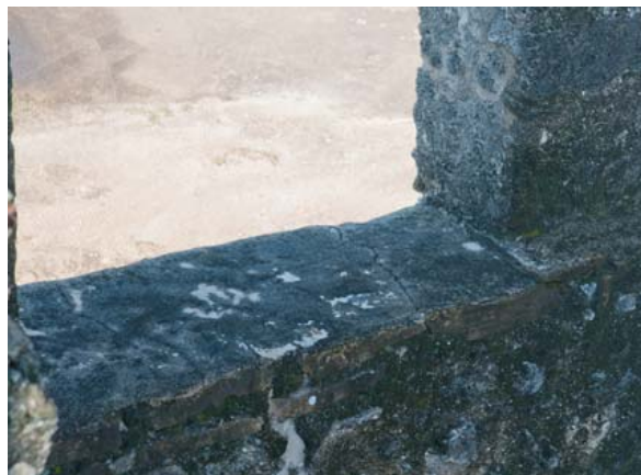
Figure 6.B.248: 203 S—South wall. Detail of the crack in the sill of window W21.
