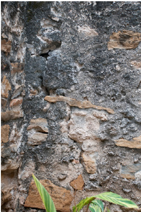
Figure 6.B.8: Room HS 203 S—South wall, south corner. Diagonal crack is located on the east corner of the south wall.
