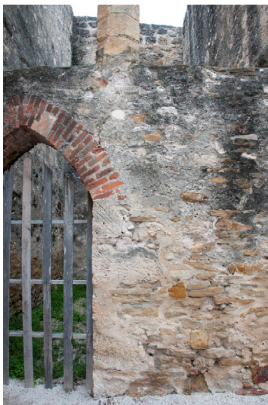
Figure 6.B.110: Room HS 203 E—North wall. Area under the octagonal column, which features several cracks and erosion in the bottom part of the wall.
