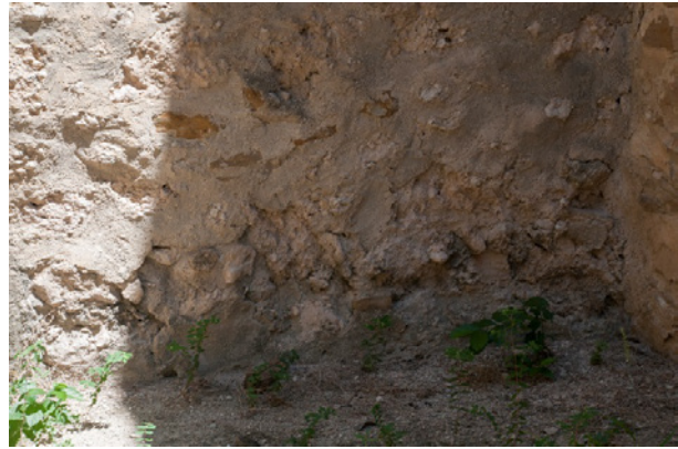
Figure 6.B.40: Room HS 203 A—North wall, detail of the bottom part of the wall showing erosion of the masonry wall and detachment of edges of the mortar patching.
