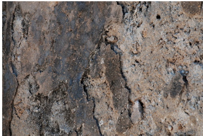
Figure 6.B.181: Room HS 203 R—East wall. Detail showing the biological growth and the detachment of the patching.
