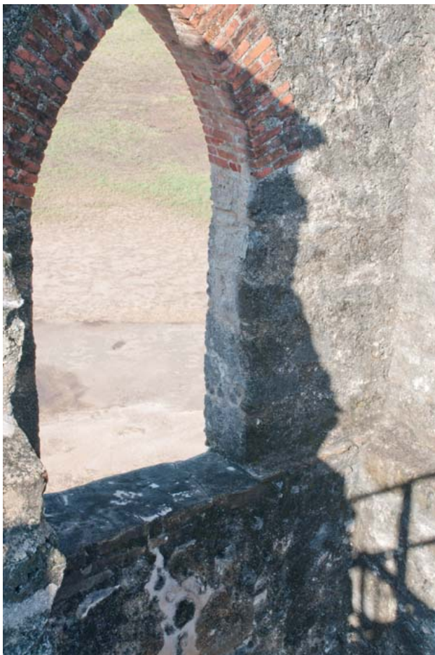
Figure 6.B.249: 203 S—South wall, featuring several cracks. There is evidence of a large filled area.
