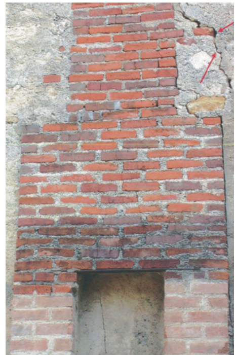
Figures 6.A.16, 6.A.17: Kitchen—Northern Wall in 2002. Large crack from the uttermost section of the wall extending down to the oven height. Reprinted from Mission San José y San Miguel de Aguayo—Inventory & Condition Assessment Survey and Documentation Report of Spanish Colonial Plasters and Mortars , by Restoration Associates Limited, LLC, 2002, pp. 96–97.
