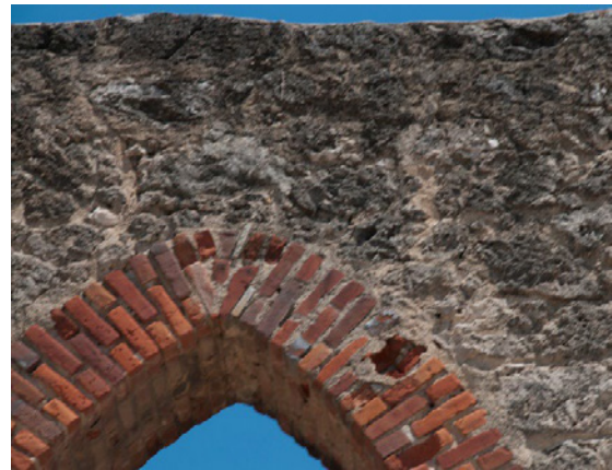
Figure 6.B.238: Exterior walls—South wall. Detail of the brick lancet arch of window W21. Features several missing parts, fragmentation of the bricks and efflorescence.
