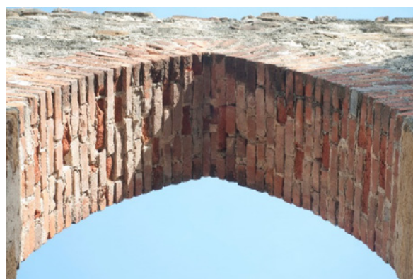
Figure 6.B.135: Room HS 203 E—West wall. Detail of arch at door D24 (upper-level) which features efflorescence, fragmentation, and powdering in the intrado.
