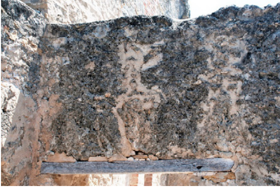
Figure 6.B.152: Room HS 203 H—East wall. Detail above the door D05. Features erosion of the masonry wall and a crack starting in the middle of the wooden architrave that has been filled with mortar.
