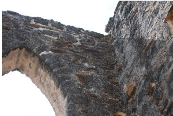
Figure 6.B.83: Room HS 203 C—South wall. Detail of the southwest corner, which exhibits a thick black layer of biological growth and erosion.
