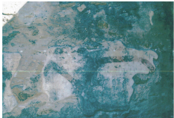
Figure 6.A.12: Room HS 203 C—North wall. Detail of decorated Spanish Colonial plaster with biological growth. Reprinted from Mission San José y San Miguel de Aguayo—Inventory & Condition Assessment Survey and Documentation Report of Spanish Colonial Plasters and Mortars , by Restoration Associates Limited, LLC, 2002, p. 66.
