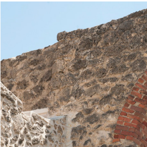
Figure 6.B.243: Exterior walls—West wall. Features a crack starting in the connection with the sacristy and going until the coping of the wall.
