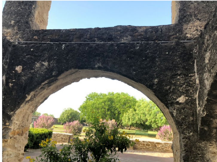
Figure 6.B.124: Room HS 203 E—South wall. Detail of the thick black layer of biological growth.
