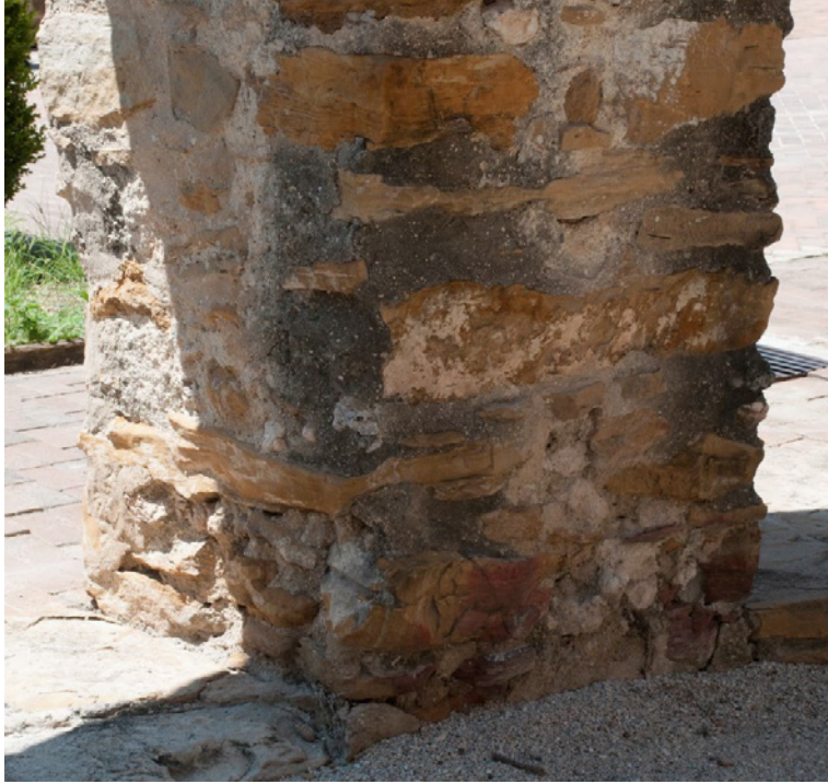
Figure 6.B.129: Room HS 203 E—South wall. Detail of one pillar, which features erosion of the masonry wall and encrustations in the stones.
