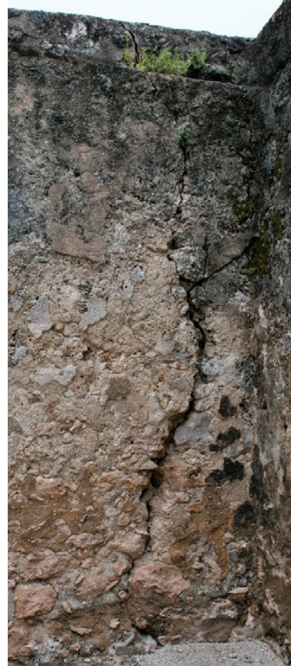
Figure 6.B.180: Room HS 203 R—East wall. Detail of the fracture in the southern end of the wall.
