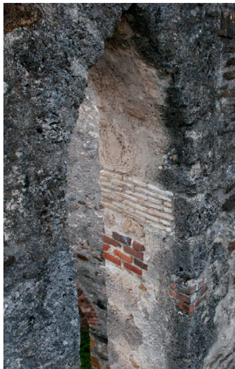
Figure 6.B.197: Exterior walls—North wall. Detail of the window W09 leading to room 203 D. Features additions of different types of bricks, probably used for repairs.
