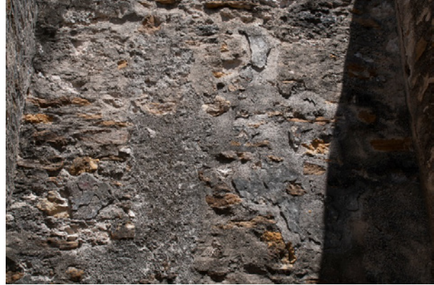
Figure 6.B.39: Room HS 203 A—North wall, detail of the middle part of the wall. Features remnants of historic plaster. Exhibits erosion and vegetation growth.
