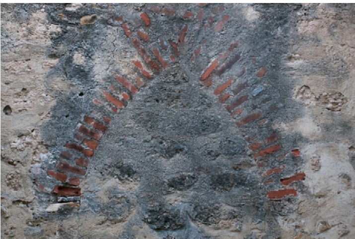
Figure 6.B.75: Room HS 203 C—North wall. Detail of the closed door in the right part of the wall, which features vegetation growth and detachment of edges of the repointing mortar.
