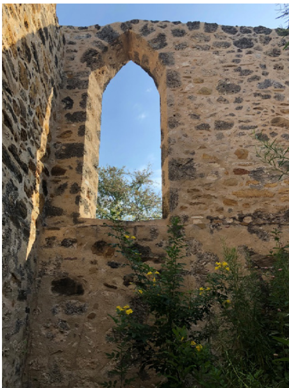
Figure 6.B.137: Room HS 203 P—North wall. The wall has been repointed recently. The limestones show a layer of biological growth.
