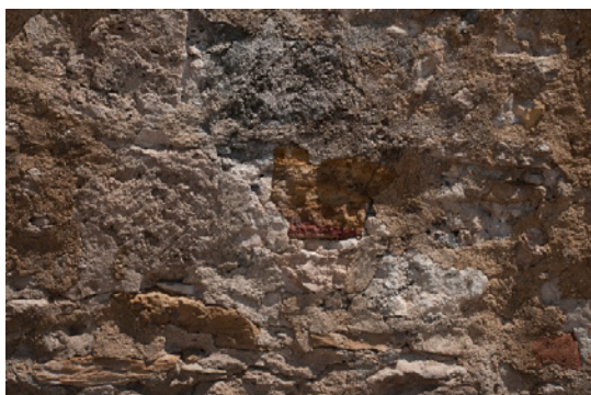
Figure 6.B.217: Exterior walls—South wall. Detail of the mid bottom part of the wall. Features delamination in the stones and erosion of the masonry wall.
