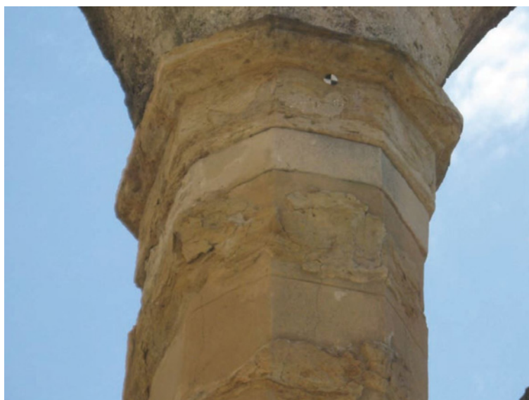
Figure 6.A.2: The column: microcracking observed during the 2011 assessment attributed to the swelling of clays inherent within the stone. The resulting 2012 thesis investigates also the effects of an elastified ethyl silicate consolidant with a swelling inhibitor.
