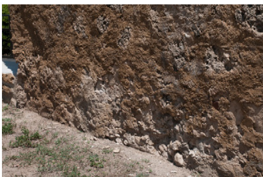
Figure 6.B.219: Exterior walls—South wall. Detail of the west bottom end of the wall. Exhibits erosion of the masonry wall and detachment of the visually intrusive patching.
