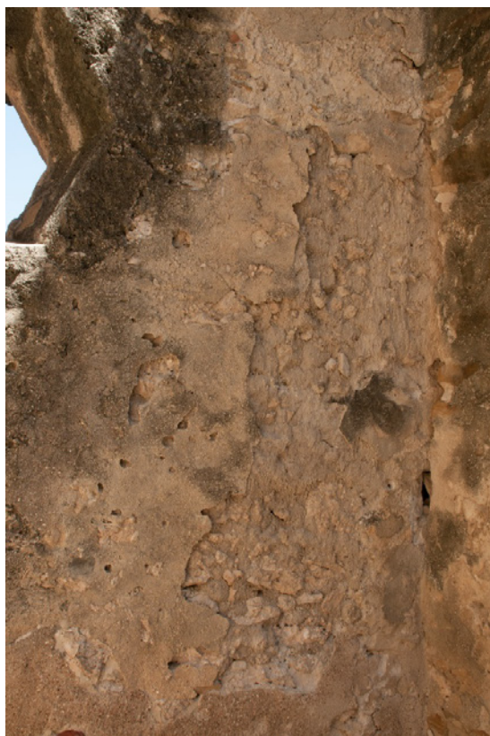
Figure 6.B.15: Room HS 203 F—North wall. The wall features detachment of edges and erosion.
