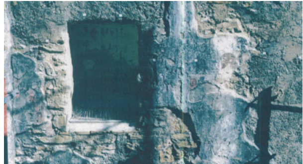
Figure 6.A.11: Room HS 203 C—North wall. Detail of Spanish Colonial plaster with heavy biological growth. Reprinted from Mission San José y San Miguel de Aguayo—Inventory & Condition Assessment Survey and Documentation Report of Spanish Colonial Plasters and Mortars , by Restoration Associates Limited, LLC, 2002, p. 65.
