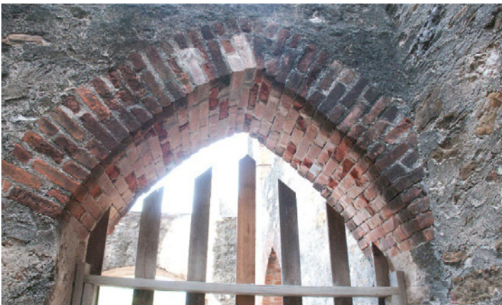
Figure 6.B.45: Room HS 203 A—South wall. Detail of the lancet arch that leads to HS 203 E features fragmentation of the bricks in the intrados.
