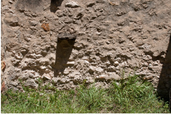
Figure 6.B.52: Room HS 203 D—North wall. Bottom left corner features erosion and missing parts.
