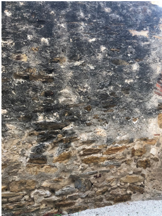
Figure 6.B.20: Room HS 203 F—East wall. Erosion and loss of mortar joint in the bottom part of the wall.
