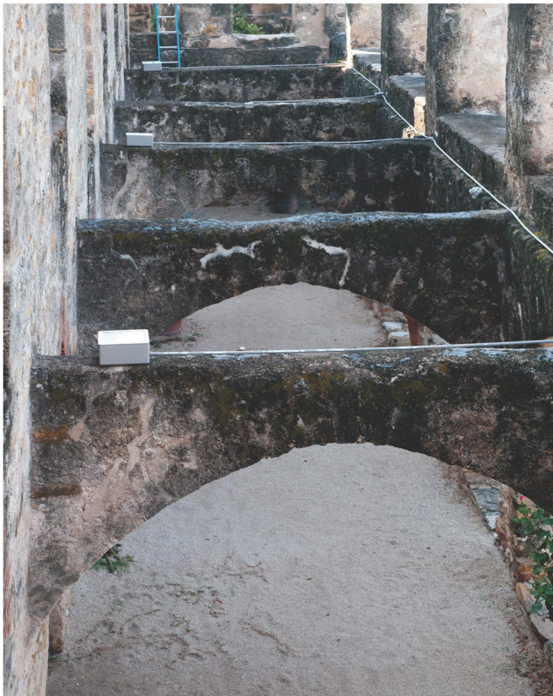
Figure 6.B.262: Room 203 E— Transverse arches. View from toward the east wing. The transverse arches feature an area with higher level of disintegration of the thin coping.
