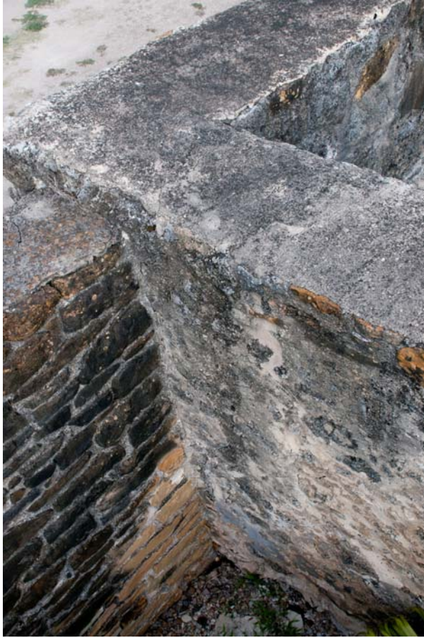
Figure 6.B.260: 203 R—East wall. View of the exterior side of the west wall. Close to the corner, the coping exhibits two cracks, continuing on the exterior wall as a sub-vertical crack.
