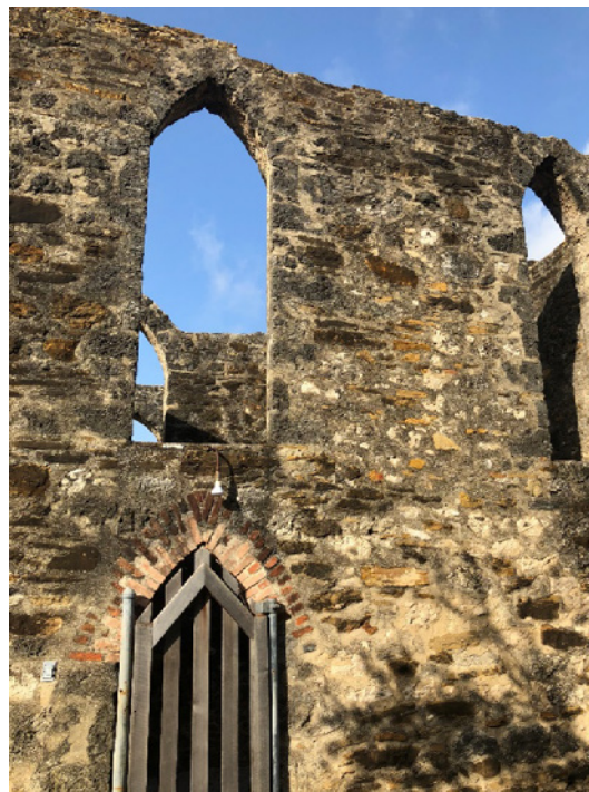
Figure 6.B.205: Exterior walls—North wall. Part corresponding to room 203 B. Features erosion in the bottom area, fragmentation of stones and fractures in the windows W12 and W11.
