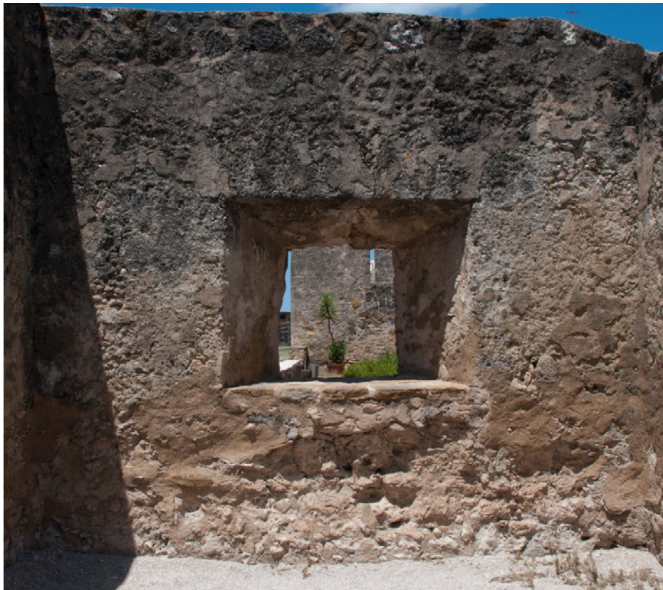
Figure 6.188: Room HS 203 R—West wall. General view. Features severe erosion below the window W03, biological growth in the upper part of the wall and cracks in the architrave of the window.
