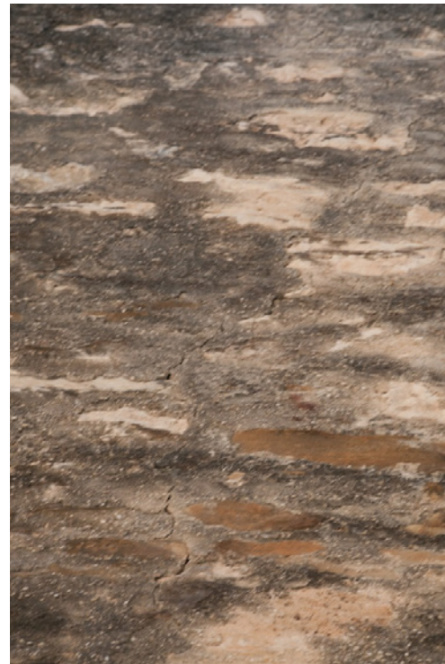
Figure 6.B.21: Room HS 203 F—East wall. Hair crack that becomes a fracture in the higher part of the wall. Corresponds to the location of the perpendicular wall of the adjacent room.
