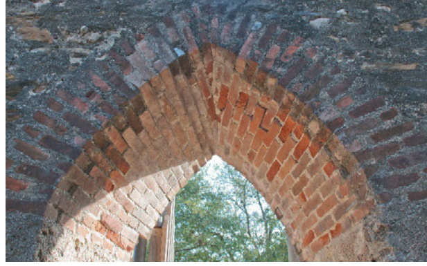
Figure 6.B.93: Room HS 203 B—North wall. Detail of the brick lancet door D03 in the right part of the wall, which features several holes in the masonry wall, and efflorescence and powdering of the bricks.
