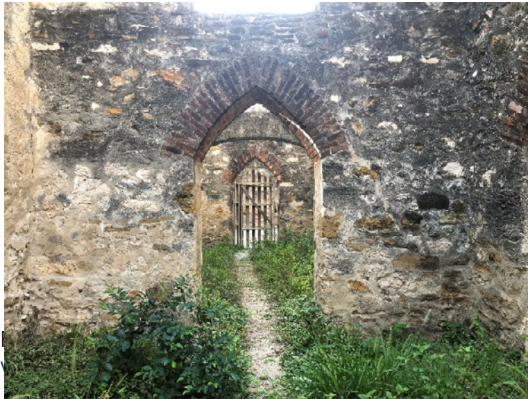
Figure 6.B.61: Room HS 203 D—East wall, bottom part features a crack to the left of the lancet brick arch, erosion in the bottom part of the wall and vegetation growth in the higher part.
