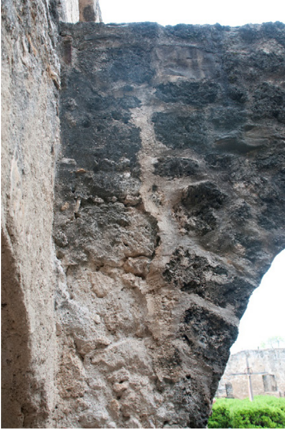
Figure 6.B.6: Room HS 203 S—East wall. Filled crack on the arcade north section.
