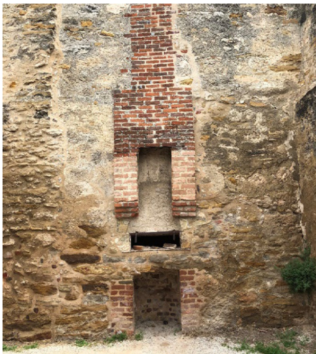
Figure 6.B.160: Room HS 203 K—North wall. General view. Features two filled cracks, one between the south arcade and the wall (left of the photo) and another in the right side of the chimney.
