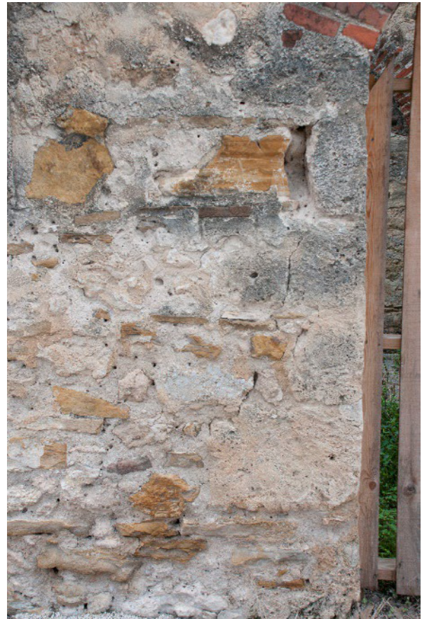
Figure 6.B.115: Room HS 203 E—North wall. Fracture at the ground floor, located left of the second door (D08) staring from the west. Erosion is also occurring at the bottom part of the wall.
