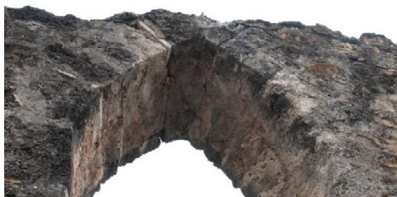
Figure 6.B.89: Room HS 203 B—North wall. Right upper window W12 also showing a fracture near the keystone of the lancet arch.
