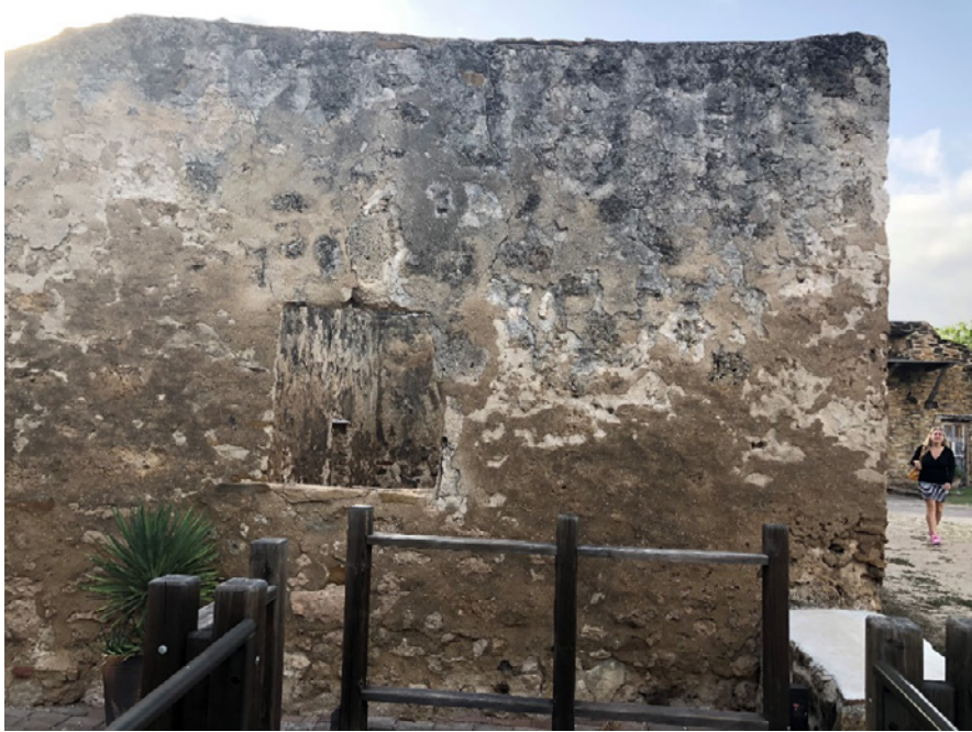
Figure 6..B.224: Exterior walls—West wall. Area corresponding to room 203 R. General view. Features vegetation growth in the upper part, multiple cracks near the window and detachment of edges of the visually contrasting patching.
