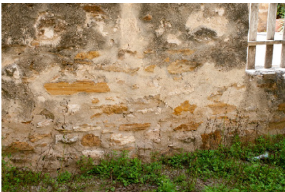
Figure 6.B.62: Room HS 203 D—South wall. Detail under the left transverse arch features vegetation growth in the higher parts and detachment of the mortar repointing edges.
