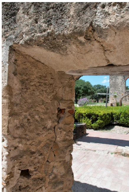
Figure 6.B.172: Room HS 203 K—West wall. Left jamb of the door D05. Features a diagonal fracture that starts under the wooden architrave.
