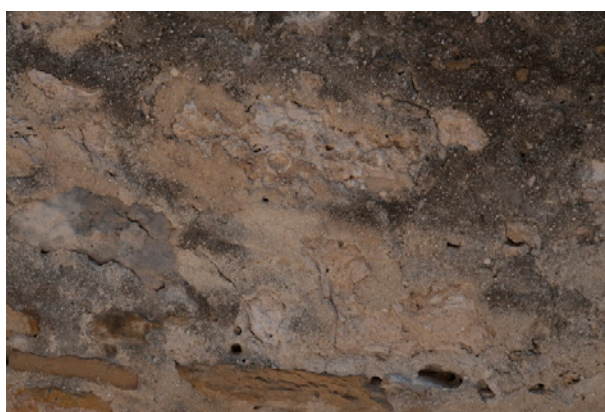
Figure 6.B.97: Room HS 203 B—East wall. Detail of the bottom part of the wall, which features vegetation growth and differential erosion of the stone blocks.
