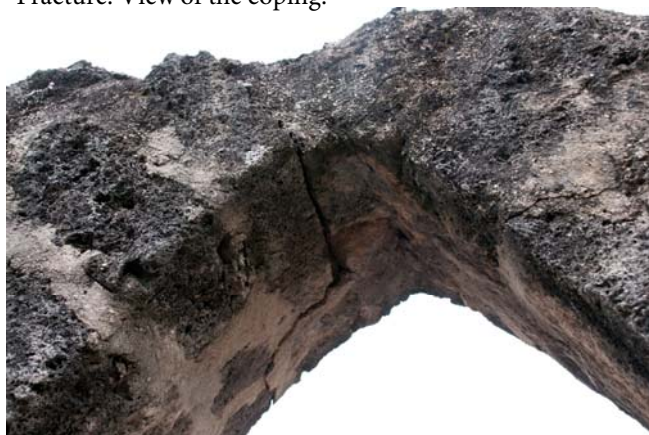
Figure 6.B.257: 203 B—North wall, Window 11. Fracture. View of the intrados of the arch.
