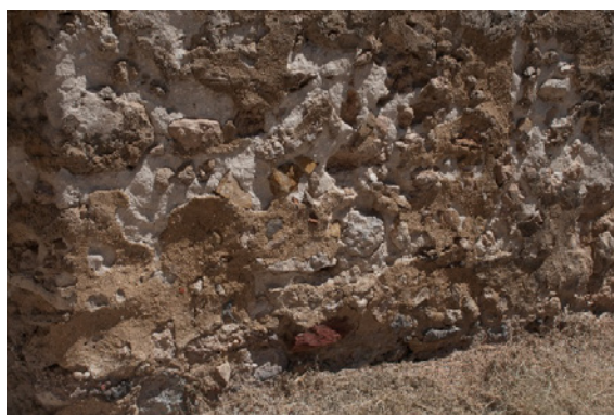
Figure 6.B.176: Room HS 203 R—North wall. Detail of the bottom part of the wall. Features erosion, missing parts and detachment of the patching.
