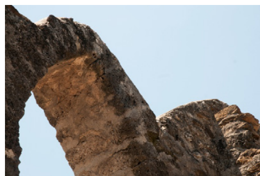
Figure 6.B.99: Room HS 203 B—South wall. Detail of the upper right window W12, which features a small crack and cement-based mortar repointing in the intrados of the arch.
