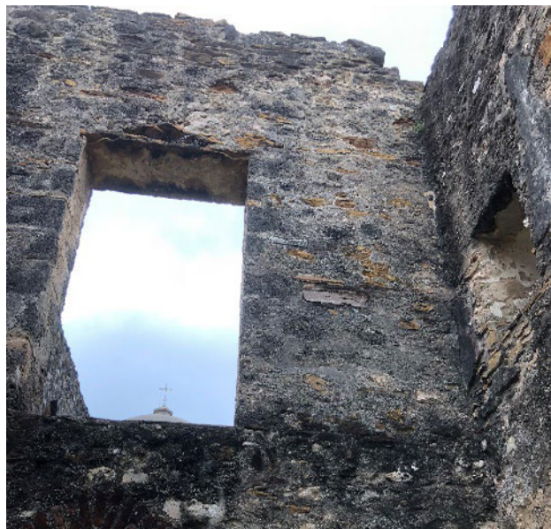
Figure 6.B.85: Room HS 203 C—West wall. Upper level exhibits erosion and delamination of stones in its upper right corner.
