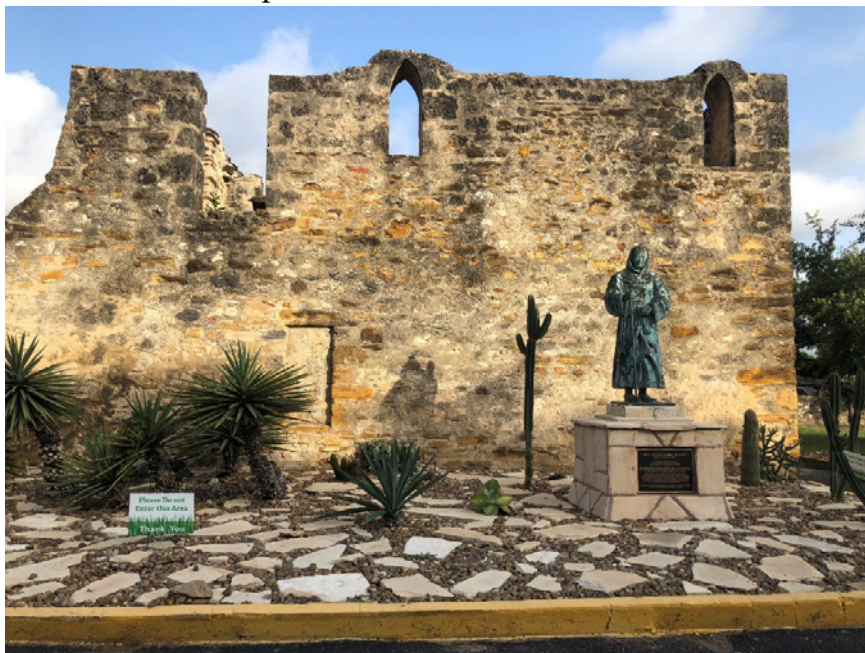
Figure 6.B.208: Exterior walls—East wall. Norther end of the wall. General view. Features vegetation growth in its upper part, erosion in the bottom and delamination in the stones.
