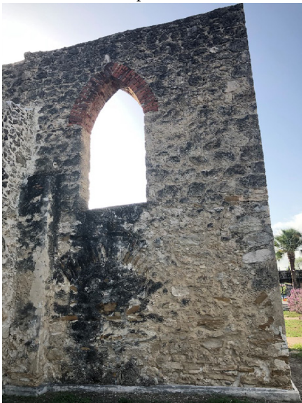
Figure 6.B.244: Exterior walls—West wall. General view. Features an accumulation of vegetation growth in the upper part and in the area below the window.
