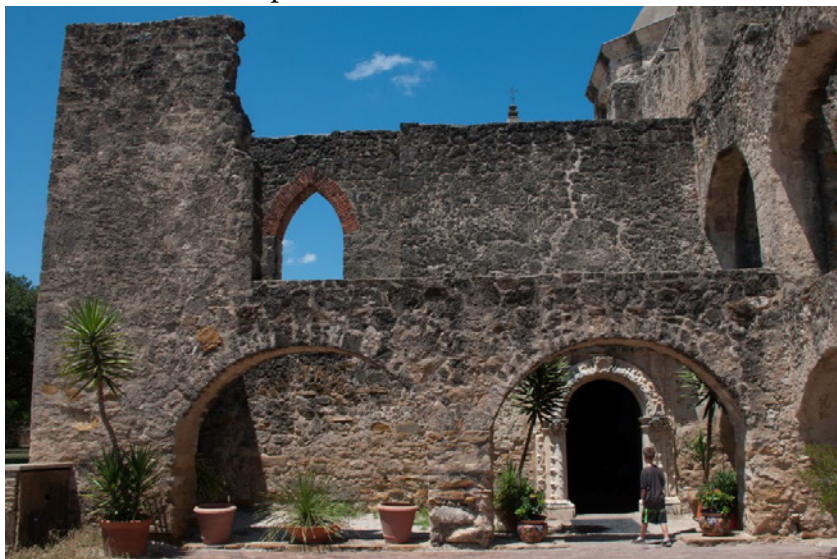
Figure 6.B.233: Exterior walls—Cloister west wall. General view. Features vegetation growth and erosion in the lower part of the pillars.
