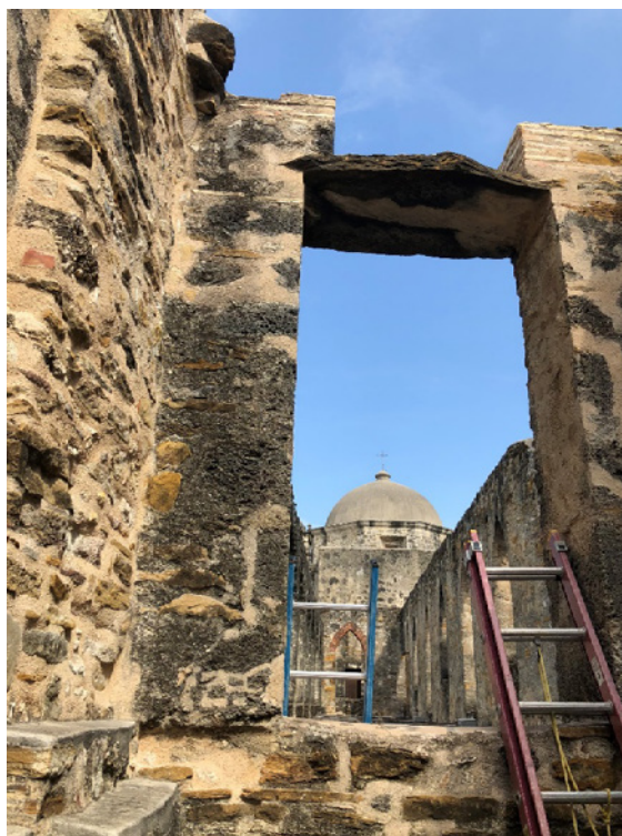
Figure 6.B.145: Room HS 203 O—West wall, which exhibits biological growth and fragmentation in some sandstones.
