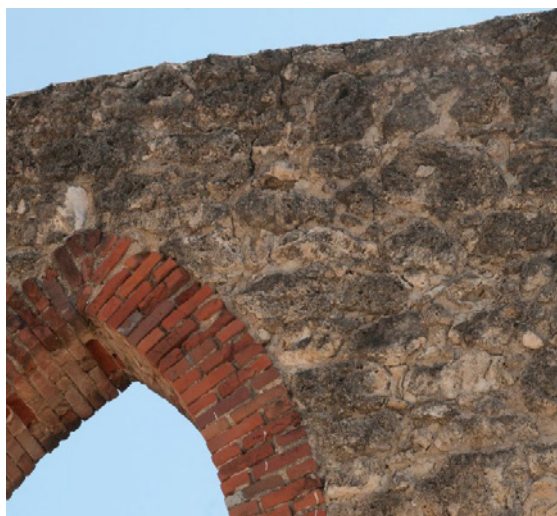
Figure 6.B.241: Exterior walls—West wall. Crack from the brick arch going until the coping of the wall.
