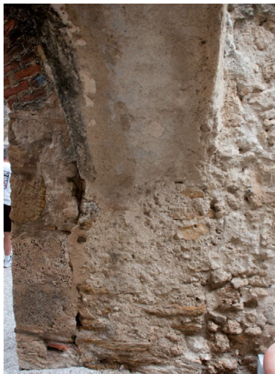
Figure 6.B.25: Room HS 203 F—East wall. The wall features a deep fracture at the corner with the south arcade.
