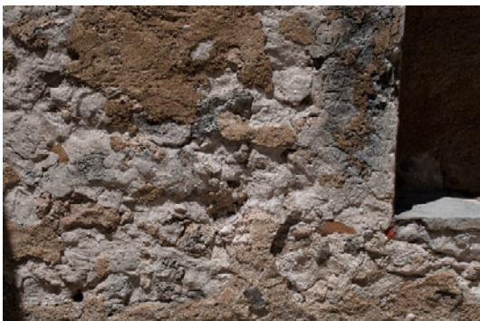
Figure 6.B.173: Room HS 203 K—West wall. Area left of the niche. Features erosion and detachment of edges of the mortar patching.
