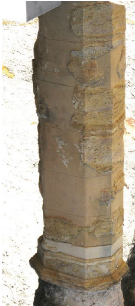
Figure 6.A.4 Reprinted from Evaluation of Proposed Consolidation Treatments for the San José Convento Column , by Kalen McNabb, 2012, p. 14.
