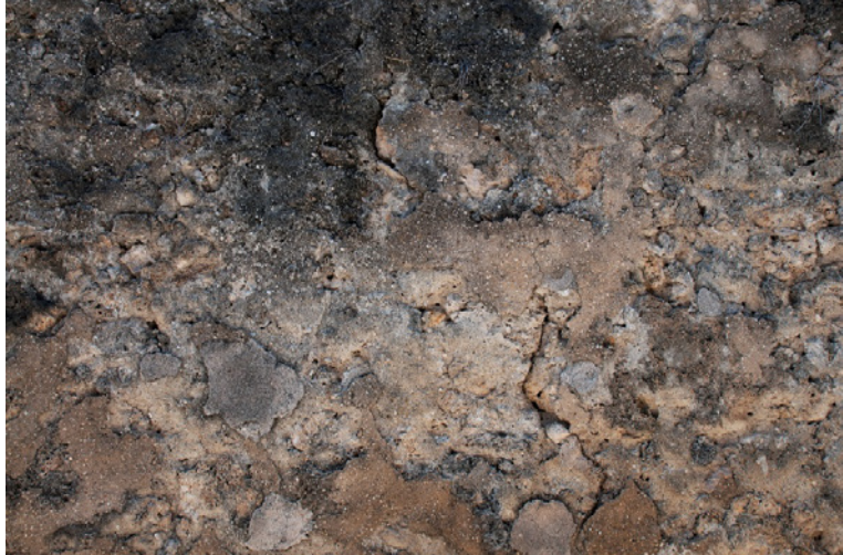
Figure 6.B.187: Room HS 203 R—South wall. Detail of the middle part of the wall. Exhibits cracks, biological growth, dry plants, erosion and different visually disturbing patching that show detachment of edges.
