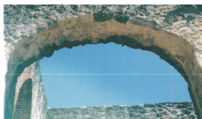
Figure 6.A.19: Arch 2 A—Detail of existing condition of remnants of Spanish Colonial mortar. Reprinted from Mission San José y San Miguel de Aguayo—Inventory & Condition Assessment Survey and Documentation Report of Spanish Colonial Plasters and Mortars , by Restoration Associates Limited, LLC, 2002, p. 121.
