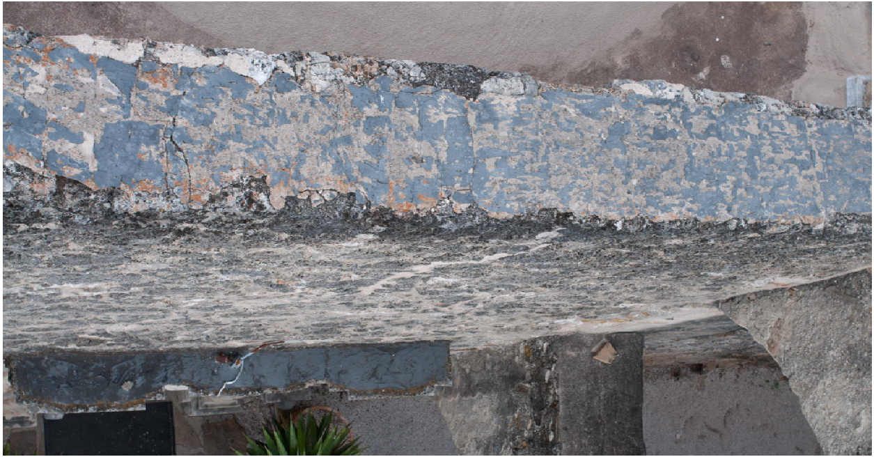
Figure 6.B.245: 203 S—West wall, disintegrating capping, with loss of material on the edges. Fragmented waterproof layer. This photo shows four cracks.
