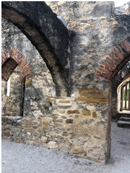
Figure 6.B.114: Room HS 203 E—North wall deterioration pattern.
