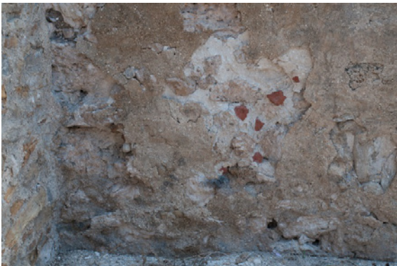
Figure 6.B.167: Room HS 203 K—East wall. Detail of the lower north corner. Features erosion, missing parts and detachment of the mortar patching.
