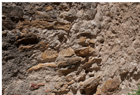
Figure 6.B.33: Room HS 203 F—West wall. Detail of the bottom part of the wall, which exhibits erosion and loss of the mortar joints.
