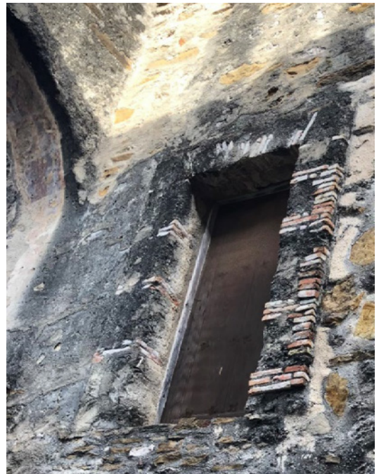
Figure 6.B.27: Room HS 203 F—West wall. Note the painted finish plaster under the arch and the biological growth on and around the door.
