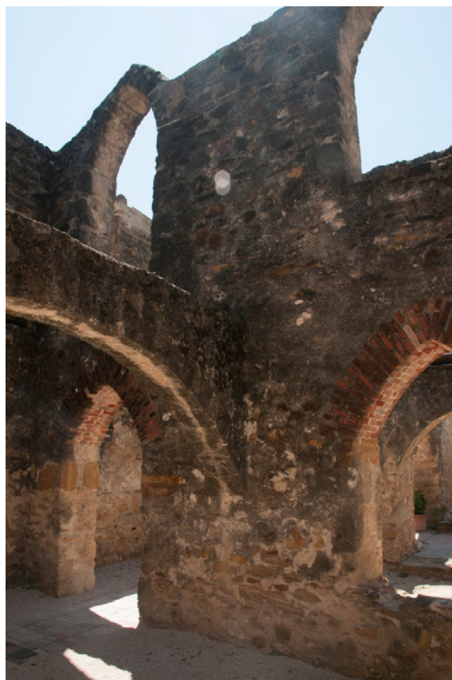
Figure 6.B.100: Room HS 203 B—South wall. General view. Vegetation growth and erosion in the lower part of the wall.
