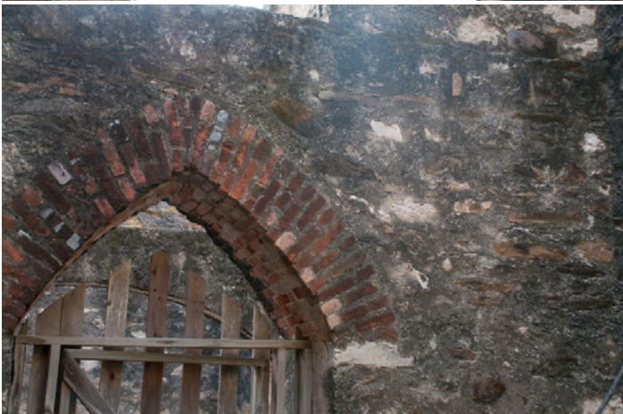
Figure 6.B.79: Room HS 203 C—East wall. Detail of the lower-level door D14, which features delamination of stones and fragmentation and efflorescence in the bricks.
