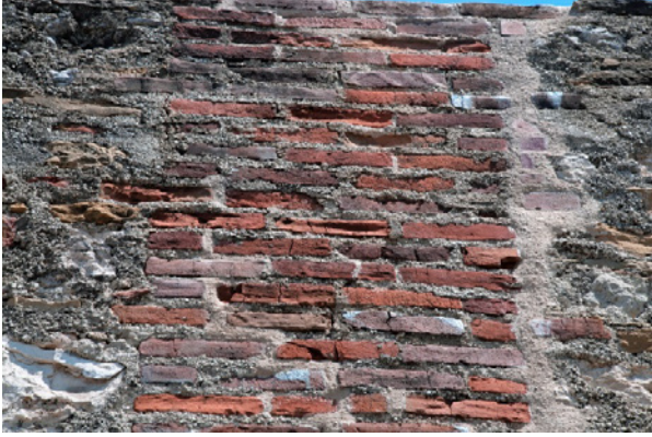
Figure 6.B.164: Room HS 203 K—North wall. Detail of the higher part of the chimney. Features cracks, efflorescence and fragmentation of the bricks.
