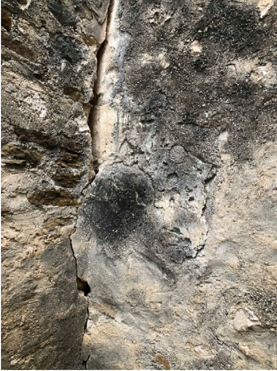
Figure 6.B.43: Room HS 203 A—North wall. The northwest corner is characterized by a vertical fracture/separation extending for the entire wall height. Remnants of historic plaster are visible on the north wall inside the fracture, indicating the west wall was added in a latter phase of construction.
