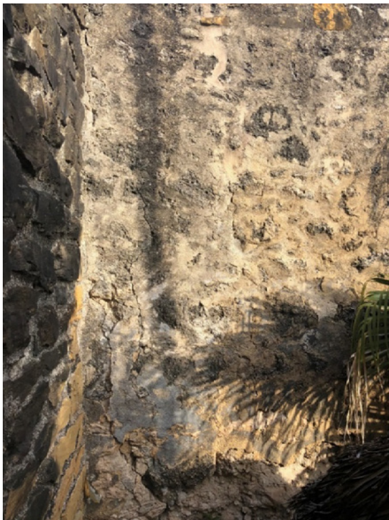
Figure 6.B.213: Exterior walls—East wall. South corner. Detail of the deep fracture, also visible from the inside.
