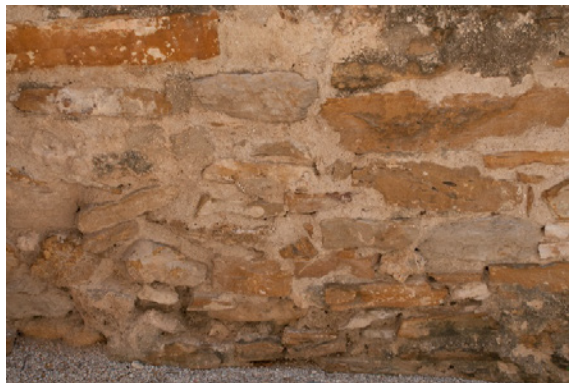
Figure 6.B.22: Room HS 203 F—East wall. Detail of the bottom part of the wall. Unlike the rest of the wall, it does not feature vegetation growth, but it exhibits erosion and loss of the mortar joints.
