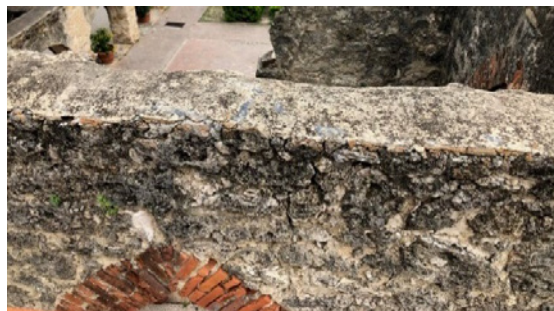
Figure 6.B.240: Exterior walls—West wall. The top of the wall features numerous hair cracks and disintegration of the wall capping.
