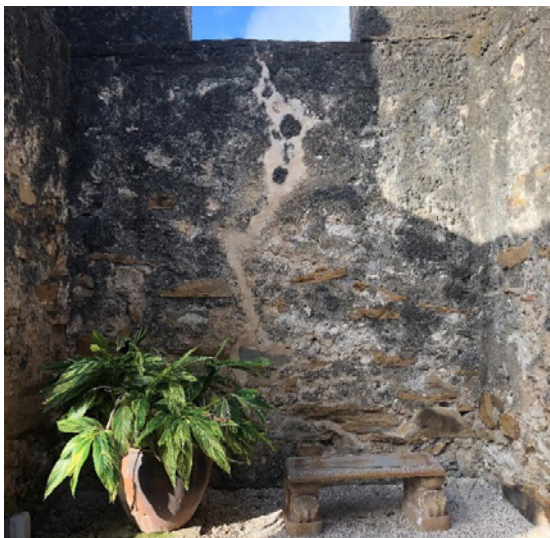
Figure 6.B.10: Room HS 203 S—South wall lower level. General view exhibiting a big crack that has been filled and a thick layer of vegetation growth.
