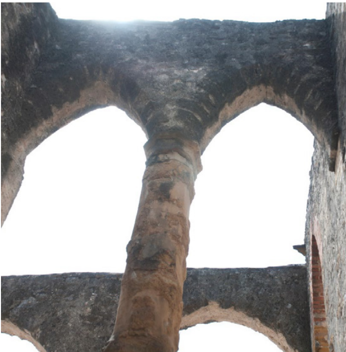
Figure 6.B.44: Room HS 203 A—South wall. Upper level. The thick layer of biological growth alters substantially the color of the tufa and sandstone. The octagonal column exhibits fragmentation and missing parts in its upper portion.
