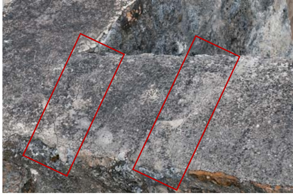
Figure 6.B.259: 203 R—East wall. Detail of the coping with the two cracks highlighted.
