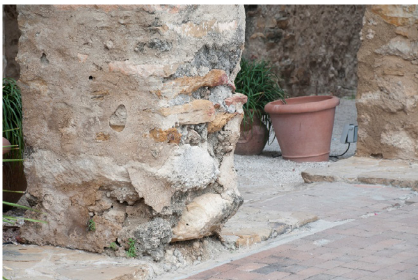
Figure 6.B.235: Exterior walls—Cloister west wall. Detail of erosion and loss of mortar in the middle pillar.
