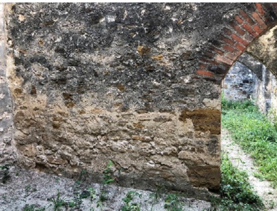
Figure 6.B.42: Room HS 203 A—East wall, which features erosion and loss of mortar joints in the bottom part and vegetation growth in the upper part.
