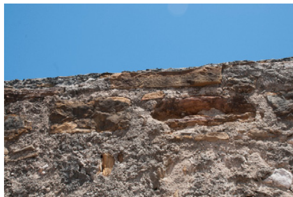
Figure 6.B.230: Exterior walls—Cloister south wall. Detail of the higher part of the lower level showing fragmentation in the stones.
