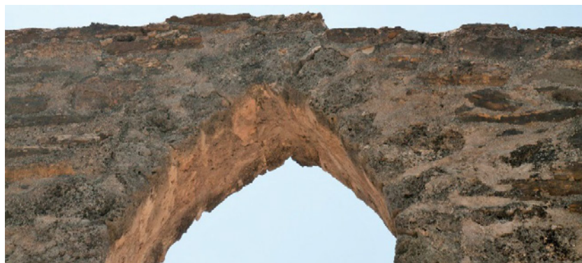
Figure 6.B.206: Exterior walls—North wall. Part corresponding to room 203 B. Right window (W11). Features the crack near the keystone that passes through all the thickness of the wall.
