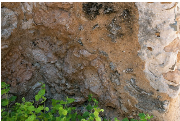
Figure 6.B.158: Room HS 203 H—South wall. Detail of the bottom left corner of the wall. Exhibits visually contrasting mortar patchings, erosion of the stone blocks and missing mortar joints.
