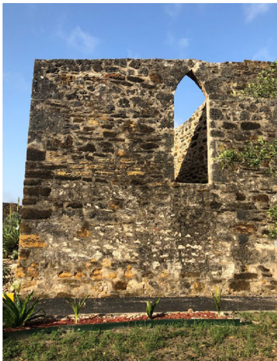
Figure 6.B.204: Exterior walls—North wall. Eastern end of the wall. Features erosion in the bottom part of the wall and multiple fragmented stones caused by the use of a repointing mortar stronger than the stone.
