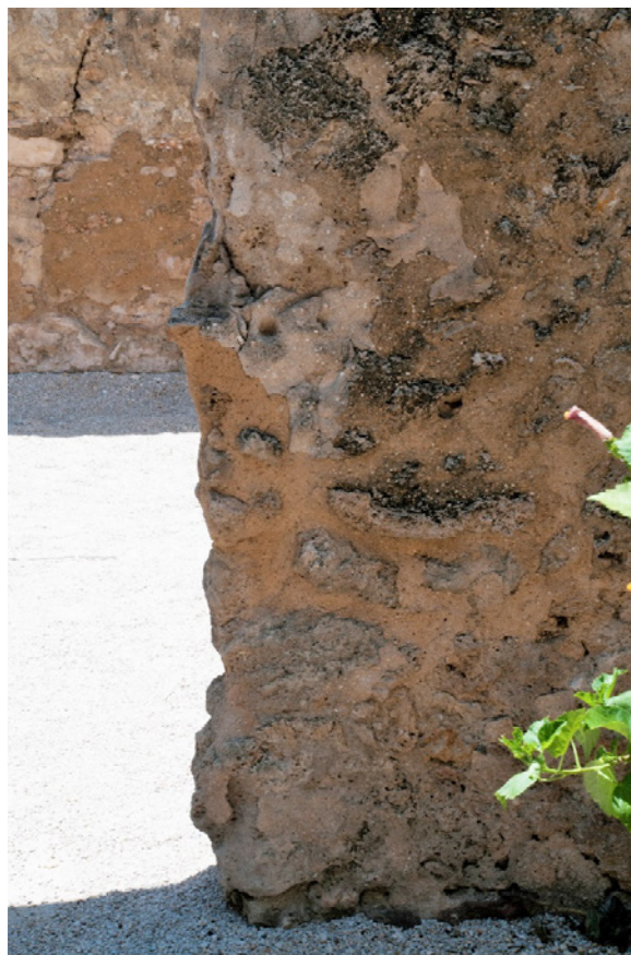
Figure 6.B.159: Room HS 203 H—South wall. Detail of the right jamb of the door D04. Features vegetation growth, different types of visually contrasting mortar patchings and erosion of the wall.
