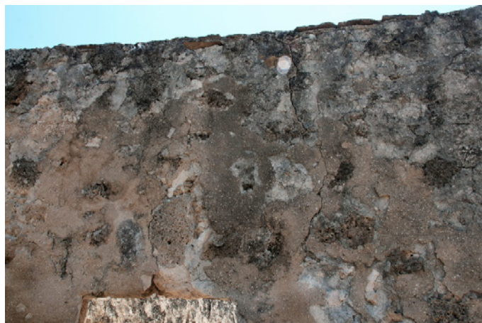
Figure 6.B.227: Exterior walls —West wall. Detail of the area above the window W03, featuring multiple cracks and detachment of the visually contrasting patching.
