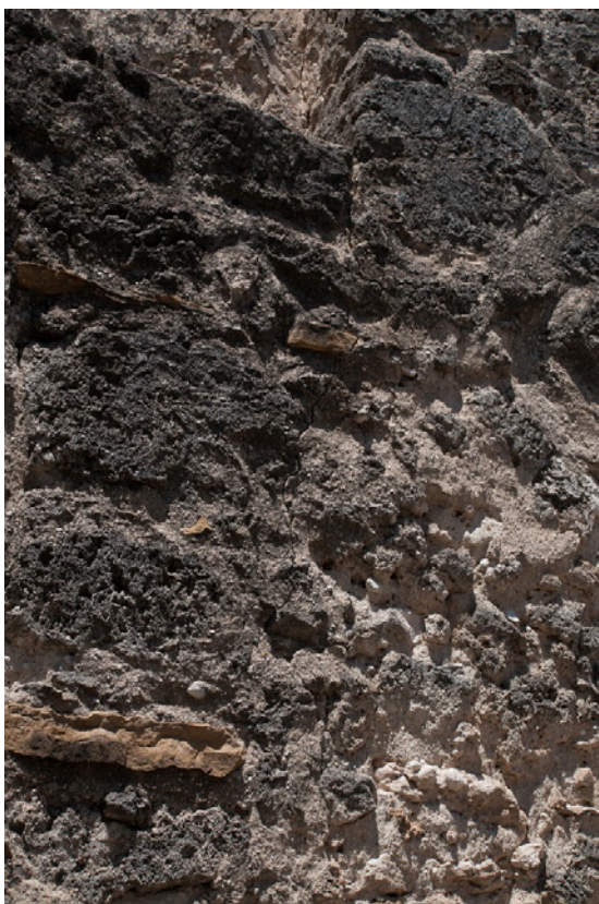
Figure 6.B.12: Room HS 203 S—West wall. Detail showing a crack in the corner where the wall's thickness changes.
