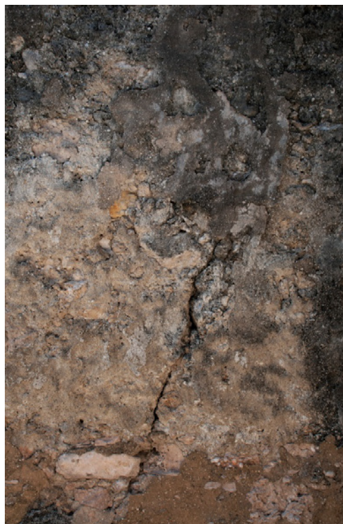
Figure 6.B.185: Room HS 203 R—South wall. Detail of the crack in the right part of the wall. Features different types of patching and erosion in the lower area of the wall.
