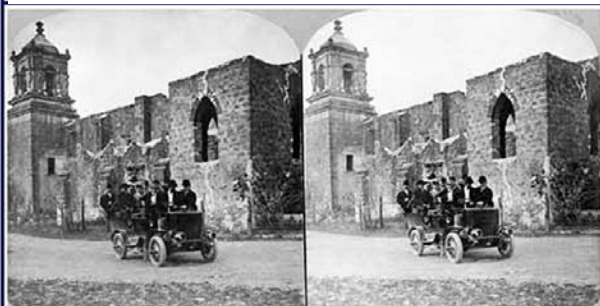
Figure 4.53: South view. Several cracks are visible in the south and east walls of the portería. Stereo-Ti:avel Co. photograph, 1909 (SMU Library).
