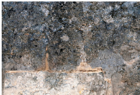
Figure 6.B.157: Room HS 203 H—South wall. Detail of the architrave of the door D04. Features two cracks in the middle and middle right of the architrave, mortar patching with graffiti and detachment of the mortar below the door.
