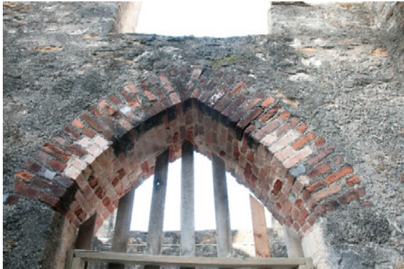
Figure 6.B.82: Room HS 203 C—South wall. Detail of the right bottom lancet arch W05, which features fragmentation and efflorescence in the intrados of the arch.
