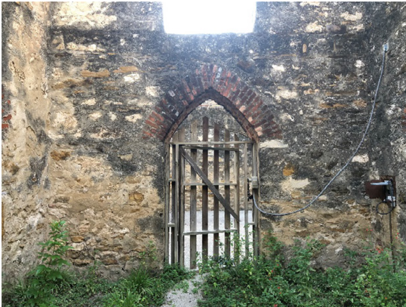
Figure 6.B.81: Room HS 203 C —East wall. General view of the lower level, which exhibits a layer of vegetation growth except in the bottom part where erosion of the masonry wall is occurring.
