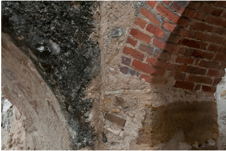
Figure 6.B.130: Room HS 203 E—Southwest corner, which features a thick layer of biological growth.
