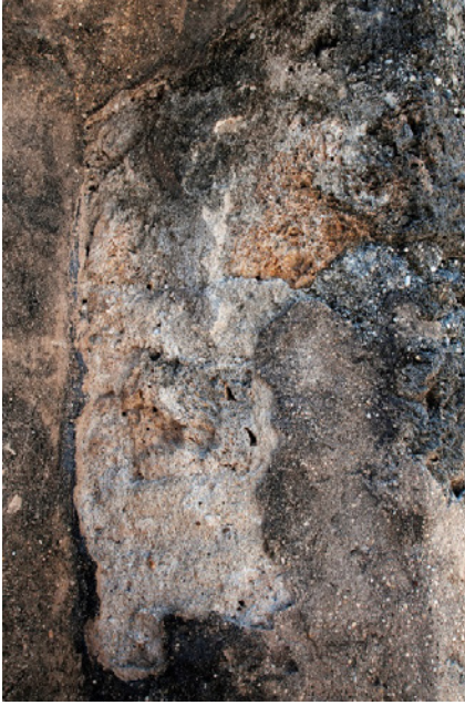
Figure 6.B.186: Room HS 203 R—South wall. Detail of the right jamb of the niche. Features biological growth and detachment of mortar patching.
