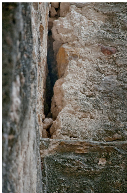
Figures 6.B.16 and 6.B.17: Room HS 203 F—East wall. Separation of 18 th -century north wall from 19 th -century perpendicular wall at the northern corner shows a stratigraphic sequence in the construction phases.
