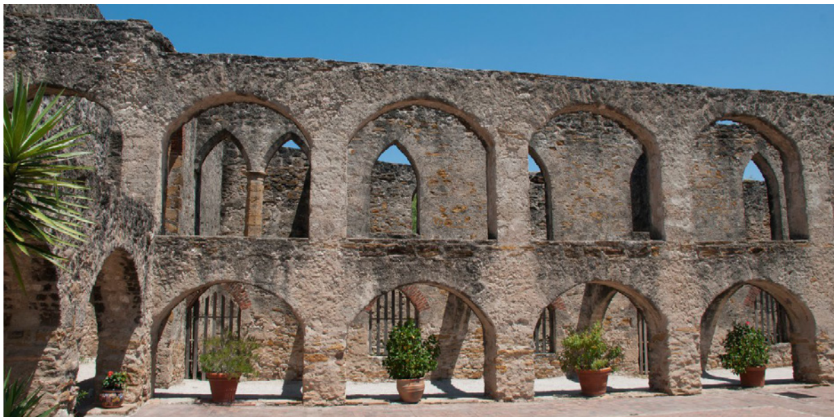
Figure 6.B.228: Exterior walls—Cloister south wall. General view. Features vegetation growth concentrated in the higher part of the wall and under the upper level arches. It also exhibits a high level of erosion in the bottom part of the pillars.
