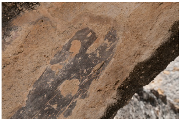
Figure 6.B.231: Exterior walls—Cloister south wall. Detail of the intrados of a lower level arch. Features detachment of the painted plaster remains.
