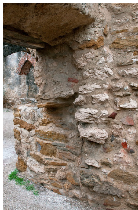
Figure 6.B.161: Room HS 203 K—North wall. Detail of the left corner of the wall. Features a crack in the middle of the door D05, erosion of the wall and fragmentation of stones.
