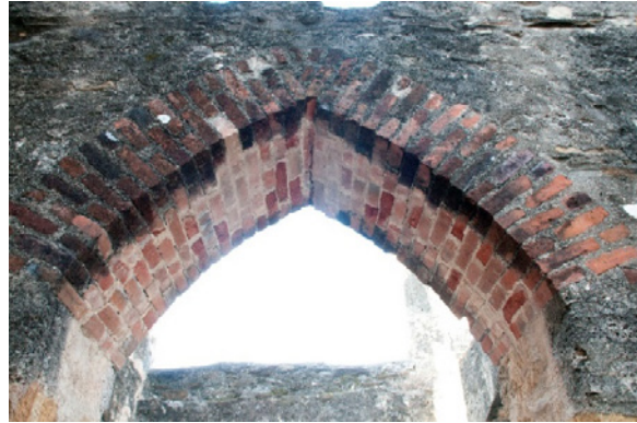
Figure 6.B.102: Room HS 203 B—South wall. Detail of the lower left arch (door D06), which features biological growth and fragmentation of the bricks.
