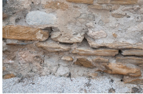
Figure 6.B.113: Room HS 203 E—North wall. Erosion of the masonry. Detail showing loss of joint mortar.
