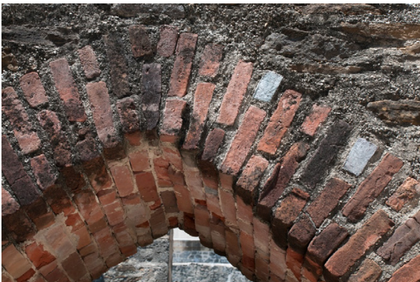
Figure 6.B.106: Room HS 203 B—West wall. Detail of the lower-level door D14, which features biological growth, fragmentation, and efflorescence.
