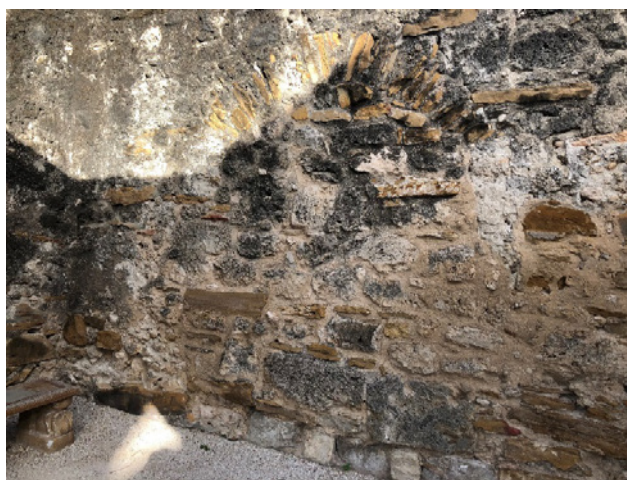
Figure 6.B.13: Room HS 203 S—West wall, south corner. Cracks are visible above the sandstone arch line. Biological growth is more developed in the upper corner.
