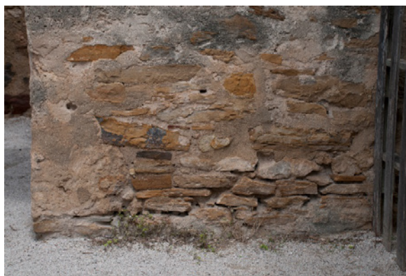
Figure 6.B.136: Room HS 203 E—West wall. Detail of the lower right area of the wall, which features erosion of the masonry wall and loss of mortar joints.
