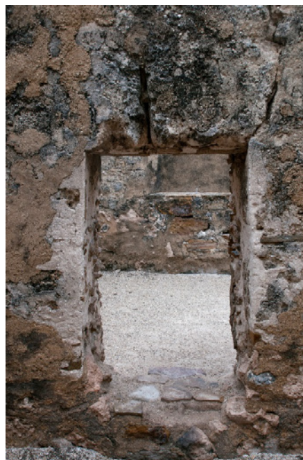
Figure 6.B.170: Room HS 203 K—South wall. Detail of the door D13 featuring a fracture starting in its upper right corner.
