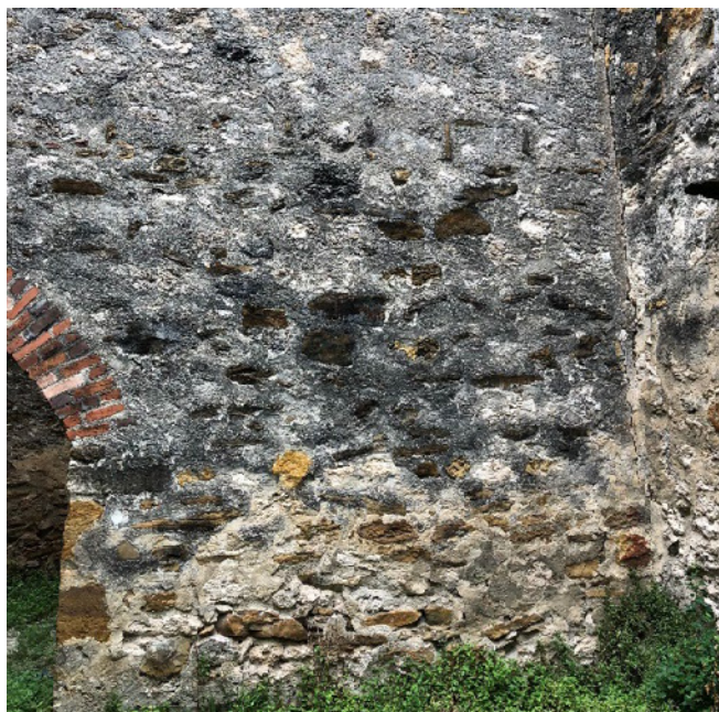
Figure 6.B.67: Room HS 203 D—West wall, bottom area exhibits erosion of the masonry due to rising damp and loss of mortar joints. In the northwest corner there is a fracture that goes all the way to the top of the wall and causes discontinuity in the structure.
