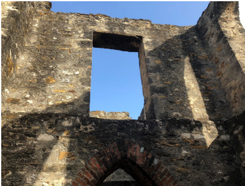
Figure 6.B.103: Room HS 203 B—West wall. Upper level general view, which exhibits a homogeneous layer of biological growth.
