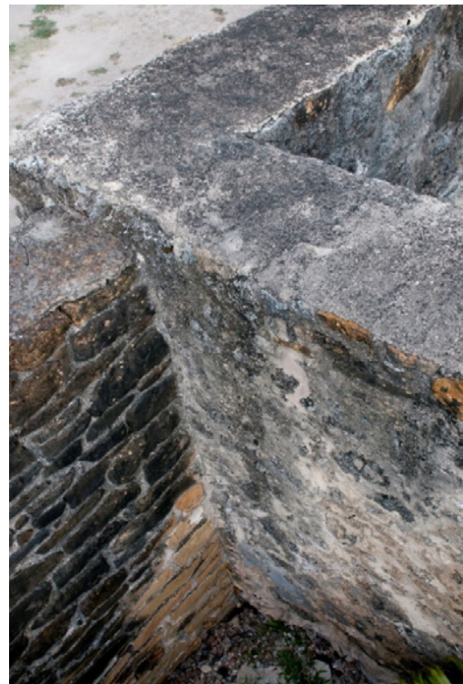
Figure 6.B.214: Exterior walls—East wall. South corner. Detail of the capping, featuring the fracture also visible on the vertical walls.
