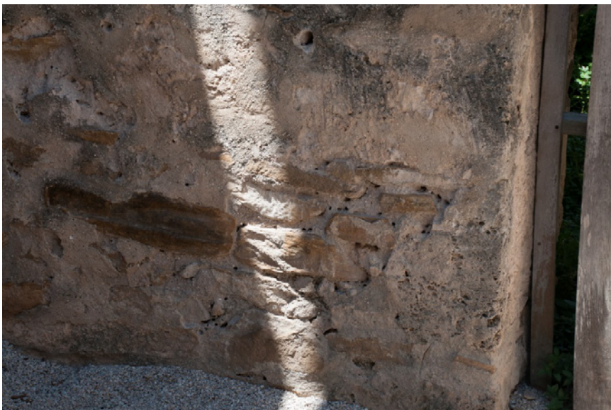
Figure 6.B.107: Room HS 203 B—West wall. Detail of the area left of the lower-level door D14, which exhibits numerous holes and loss of mortar joints.
