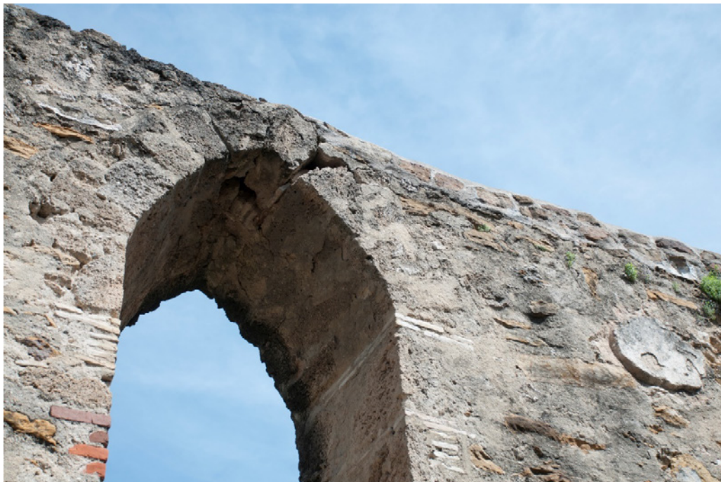
Figure 6.B.57: Room HS 203 D—North wall. Detail of the upper part of the window. A structural crack can be seen at the right of the keystone, and also additions of bricks in the construction or reparation of the window.
