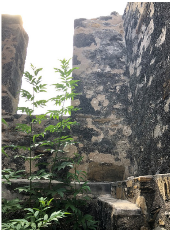
Figure 6.B.143: Room HS 203 O—East wall, which features biological growth and some fragmentation in the sandstones.
