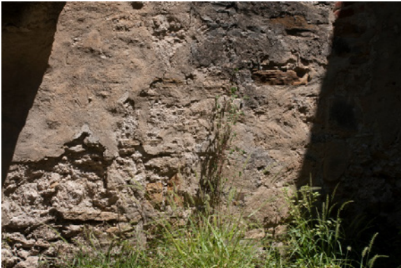
Figure 6.B.53: Room HS 203 D—North wall. Bottom right area exhibits erosion of the bottom part of the wall due to rising damp and detachment of edges of the arriccio.
