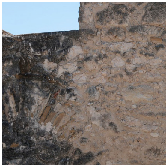
Figure 6.B.242: Exterior walls—West wall. Note the crack above the sandstone voussoirs shaping the arch line of former door D12.
