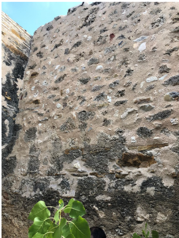
Figure 6.B.142: Room HS 203 O—North wall. The walls in this room have been recently repointed. Biological growth is present.
