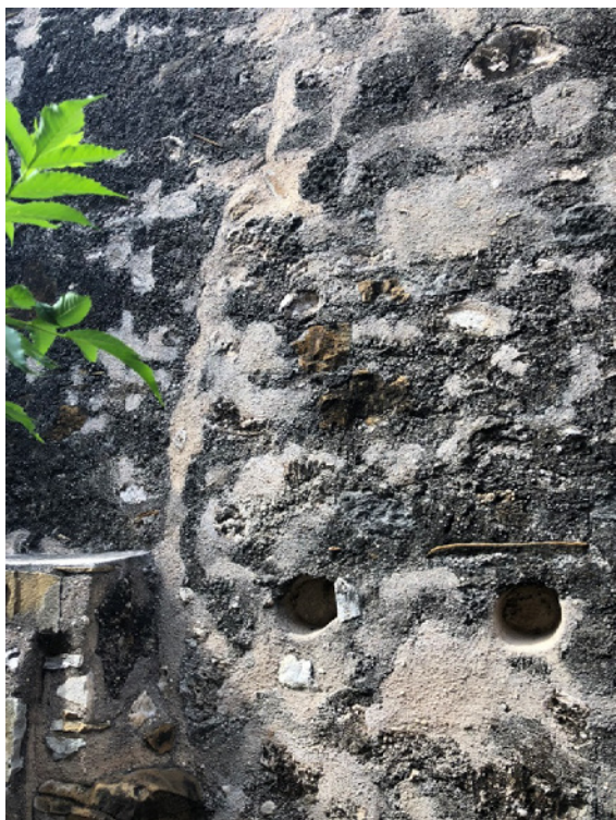
Figure 6.B.144: Room HS 203 O—South wall, which features biological growth and regular holes that might have been the location of wooden beams.
