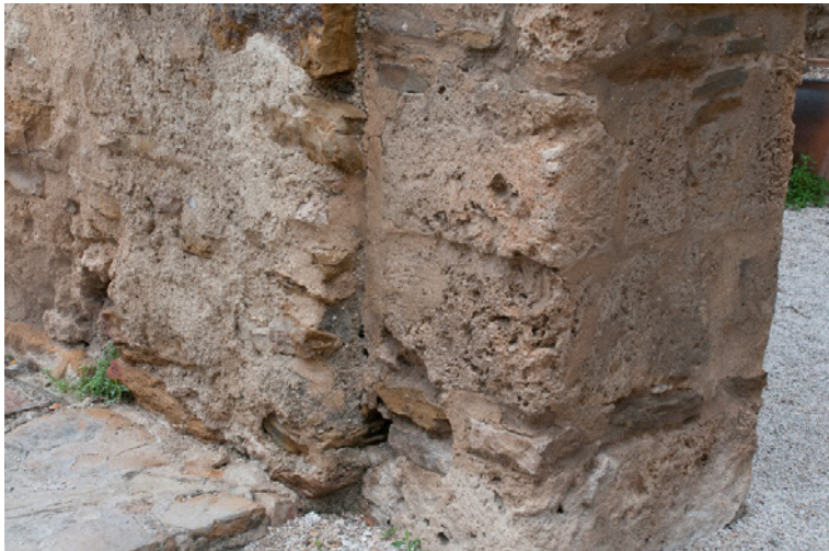
Figure 6.B.131: Room HS 203 E—Southwest corner, which features erosion and loss of mortar joints in the lower part.
