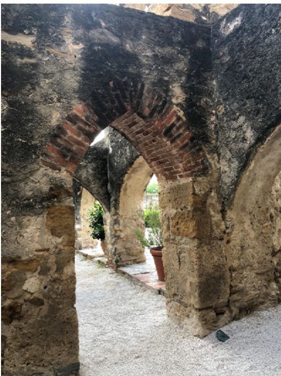
Figure 6.B.24: Room HS 203 F—East wall. Lancet arch in the southern end of the wall, which features a thick layer of vegetation growth in the area above the arch.
