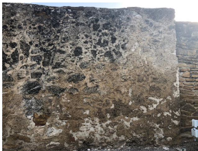
Figure 6.B.218: Exterior walls—South wall. East corner. Features several cracks, vegetation growth in the upper part, erosion in the bottom and multiple visually contrasting patching, which exhibit detachment of edges.
