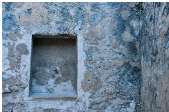
Figure 6.B.168: Room HS 203 K—East wall. Detail of the right corner. Exhibits erosion and several holes in its lower part, and visually contrasting brown mortar patchings.
