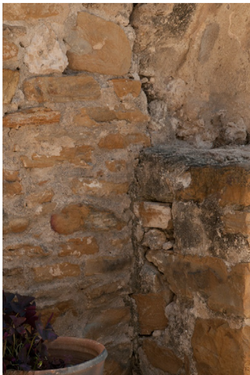
Figure 6.B.125: Room HS 203 E—Southeast corner, features a fracture in the connection of the south arcade and the east wall.
