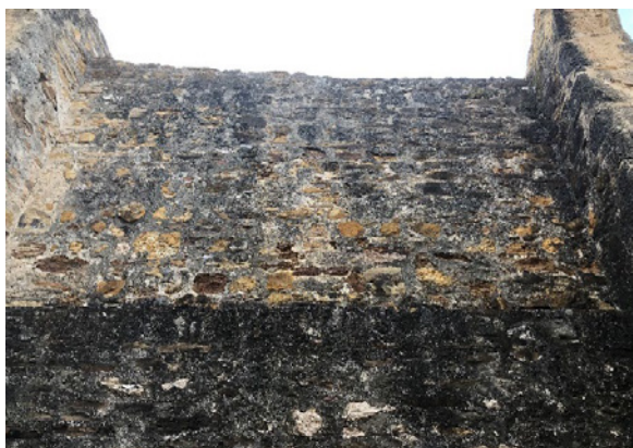
Figure 6.B.96: Room HS 203 B—East wall. Upper part of the east wall, which exhibits a thick black layer of vegetation growth in its bottom part and delamination of the stones in its upper part.
