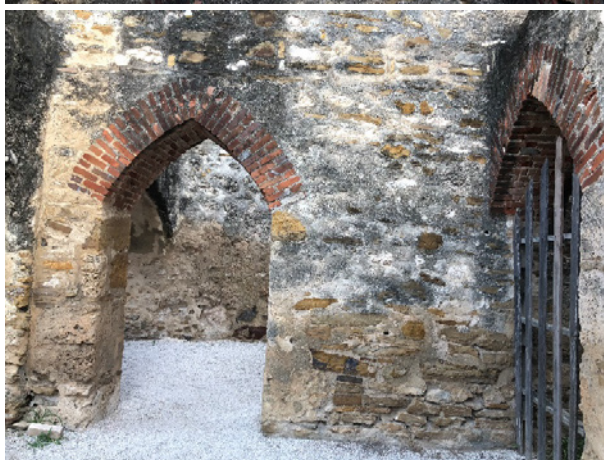
Figures 6.B.132 and 6.B.133: Room HS 203 E—West wall. Biological growth, concentrated under the door D24, associated with efflorescence under the arch. Erosion and loss of mortar joints in the lower part of the wall.
