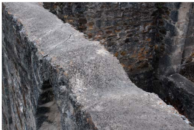
Figure 6.B.255: 203 B—North wall, Window 11. Fracture. View of the coping.
