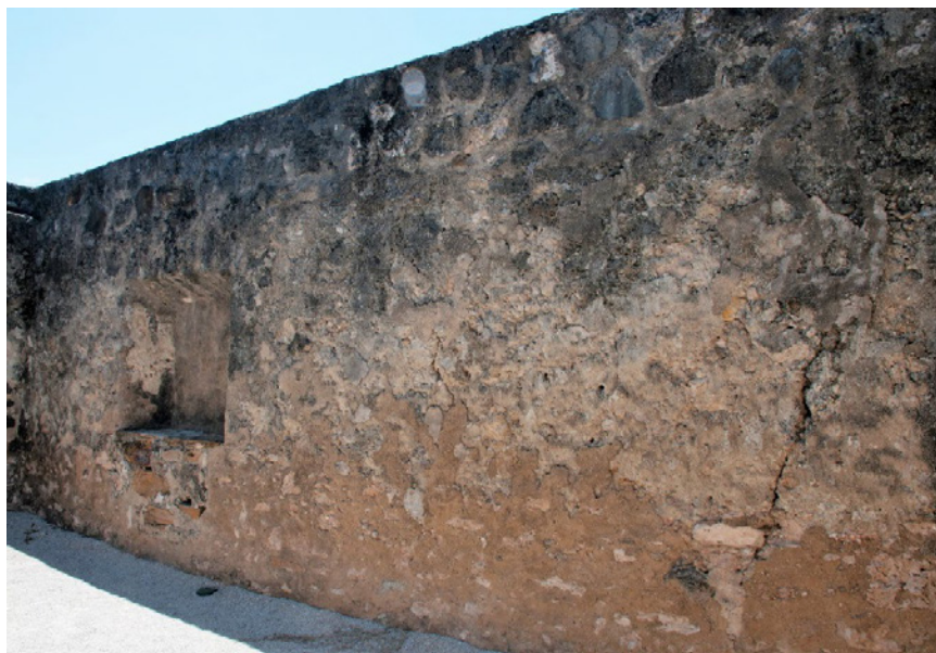
Figure 6.B.183: Room HS 203 R—South wall. General view. Feature biological growth in its upper part and visually contrasting patching in the lower area.
