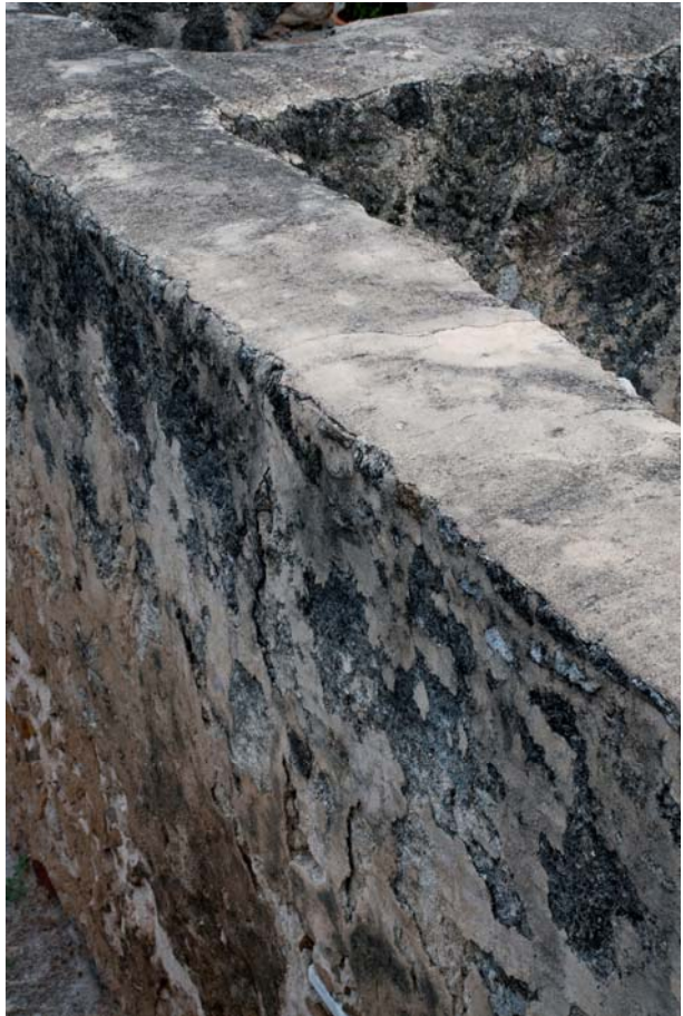
Figure 6.B.261: 203 R—South wall. Coping and wall fracture, located in the area where the interior niche is located.
