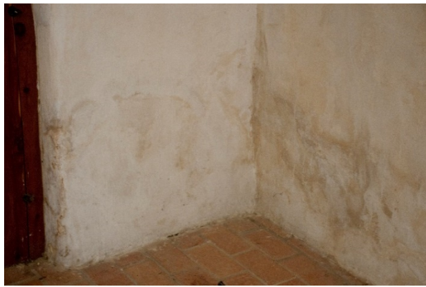
Figure 6.B.115: 104 F Refectory—South wall. Rising damp produces erosion of the plaster finishes, associated with stains. Stains produced by the presence of iron and manganese in the water composition.
