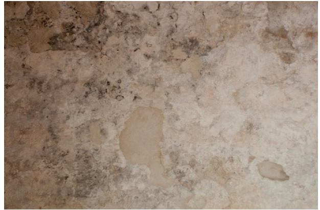
Figure 6.B.62: 104 D Portería—North part of the east wall (C4, C5). Visually intrusive patches are visible, surrounded by eroded historic plaster.
