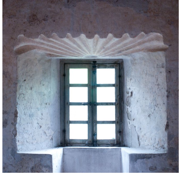
Figure 6.B.133: East wall, view of the decorative clamshell window openings. Its surface exhibits historic graffiti, a crack in its architrave, and detachment of the patching of the right jamb.
