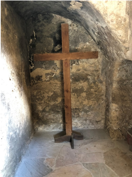
Figure 6.B.173: East wall under the staircase features mortar patching from different time periods.
