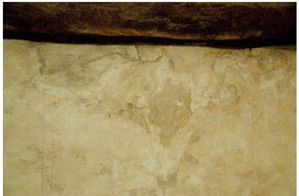
Figure 6.B.38: 104 B—North wall details (bottom photo, B2). Photos showing missing parts and detachment of edges of the historic plaster. In the upper photo we can see the addition of a plaster patching. The lower photo features detachment of edges of the plaster, patching, and efflorescence.
