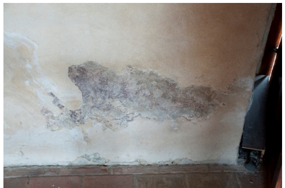
Figure 6.B.82: 104 E Library—East wall (A5). Features plaster patching surrounding the remnants of historic painted plaster. The painted finish show traces of efflorescence and erosion.
