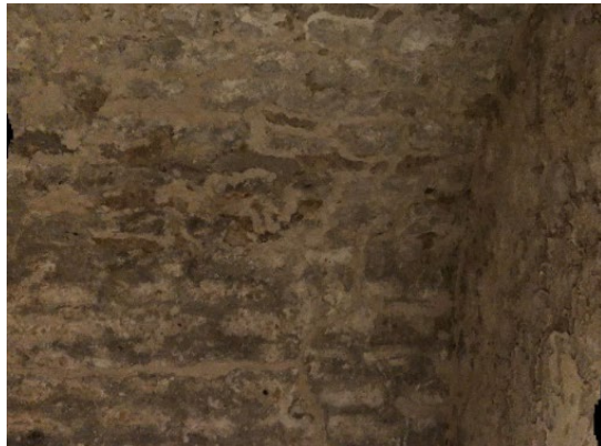
Figure 6.B.41: 104 B—Southeast area of the ceiling (C1, D1). Features efflorescence, repointed mortar joints roughly executed.
