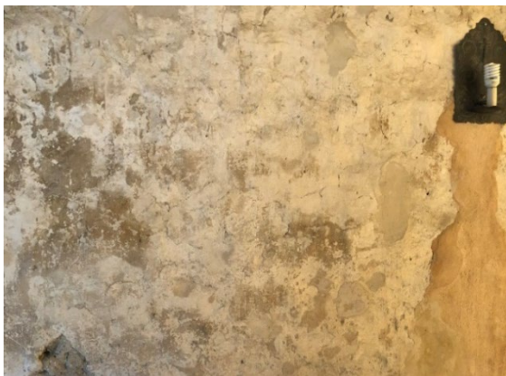
Figure 6.B.54: 104 C—West wall (B2, B3). In general the west wall is in better condition than the east, extensive craquelé, detachment of plaster from substrate, and numerous patchings of various dimensions.
