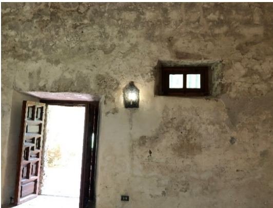
Figure 6.B.47: 104 B—West wall. Featuring plaster patching below the light and at the bottom of the wall, discoloration and graffiti below the window, and small remnants of painted plaster around the small window.
