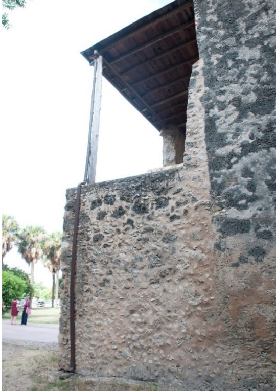
Figure 6.B.220: Exterior east wall, corresponding to the staircase, features a change in the masonry type, with wall made of small rubble and recently repointed brownish mortar.
