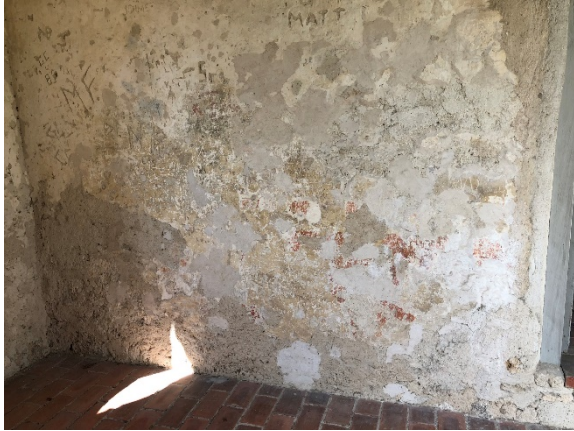
Figure 6.B.147: North wall. West part of the wall, left of the door. The surface features remnant of historic painted plaster (red/orange color), different types of patching, and historic graffiti.
