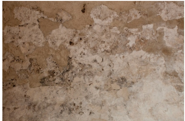
Figure 6.B.63: 104 D Portería—North part of the east wall (D4, D5) features discoloration and differential erosion of the plaster and intrusive brownish patchings.
