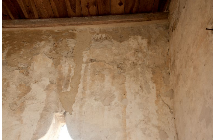
Figure 6.B.159: West wall. Upper part of the wall. Exhibits a crack starting from the upper point of the window that has been filled, concrete patching on the top of the wall, and detachment of edges of the plaster.
