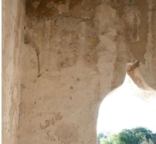
Figure 6.B.158: West wall. Upper left area. Features a crack starting from the corner of the wall, concrete patching in the connection with the roof, and detachment of edges of the plaster.
