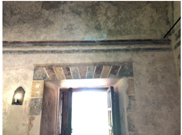
Figure 6.B.96: 104 E Library—West wall, door leading to the corridor, showing patching, craquelé, and erosion of the painted finish.
