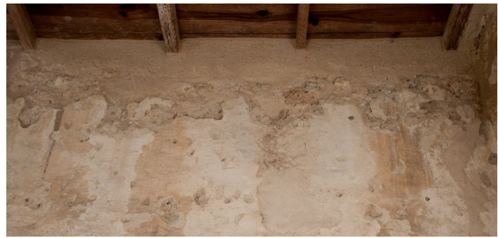
Figure 6.B.163: South wall. Upper right part. Shows mortar patching in the connection with the roof and detachment of edges of the plaster.
