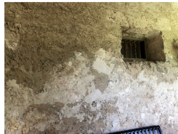
Figure 6.B.11: 104 A—Northern area of the east wall, showing erosion in the historic plaster.
