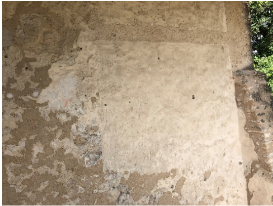
Figure 6.B.152: North wall. East end. Exhibits brown mortar patching in the left side, missing parts, and historic graffiti.
