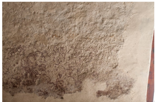
Figure 6.B.92: 104 E Library—South wall (A2). Bottom left corner of the door, showing patching around the jamb of the door and a strong differential erosion of the historic plaster.
