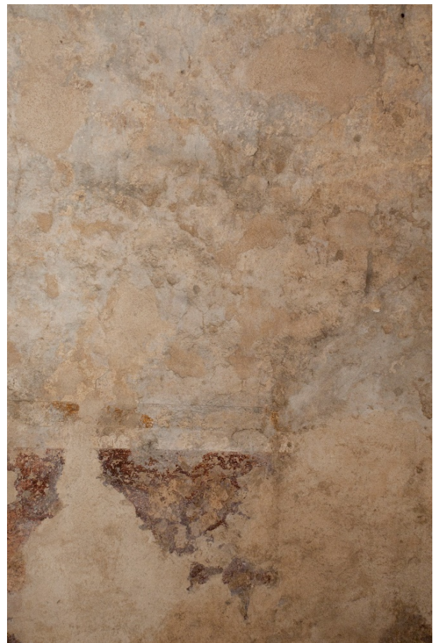
Figure 6.B.87: 104 E Library—Ceiling detail (A1, B1). Decorative geometric lines of painted plaster in yellow and red in the bottom part. Above the wainscot, erosion of the painted finish and well-executed patching, having material and visual continuity with the substrate.
