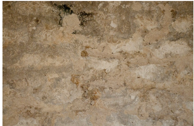
Figure 6.B.42: 104 B—Southwest part of the ceiling (H5). Features differential erosion on the remnants of historic plaster and different types of mortar patching.
