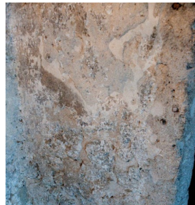
Figure 6.B.27: 104 A—South wall (A1), left part of the door. At the top of the picture two layers of plaster are observed featuring detachment and differential erosion. At the bottom part of the picture there is limewash directly applied to the tufa rubble stone.
