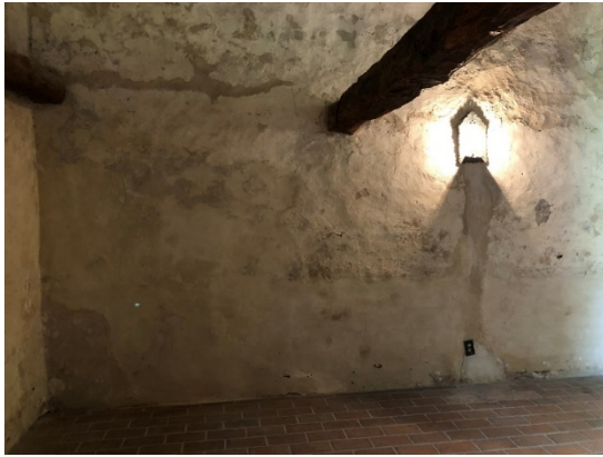
Figure 6.B.39: 104 B—East wall. The bottom part of the wall has been repaired with plaster patching, and it features efflorescence in the left corner.
