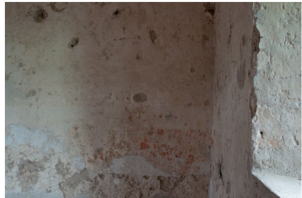
Figure 6.B.129: North wall (A1, B1). Shows the remnant of painted plaster in a red/orange color. The surface features erosion of the painted finish and historic graffiti.
