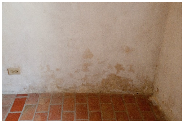
Figure 6.B.118: 104 F Kitchen. Rising damp in the wall, which produces stains and erosion of the surface.
