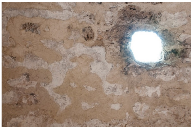
Figure 6.B.64: 104 D Portería—Ceiling (G2, G3) features remnants of historic plaster with efflorescence and roughly executed brown mortar repointing that partially covers the stone.
