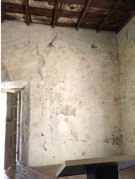
Figure 6.B.122: South wall, west corner. Diagonal cracks starting from the door architrave are visible.
