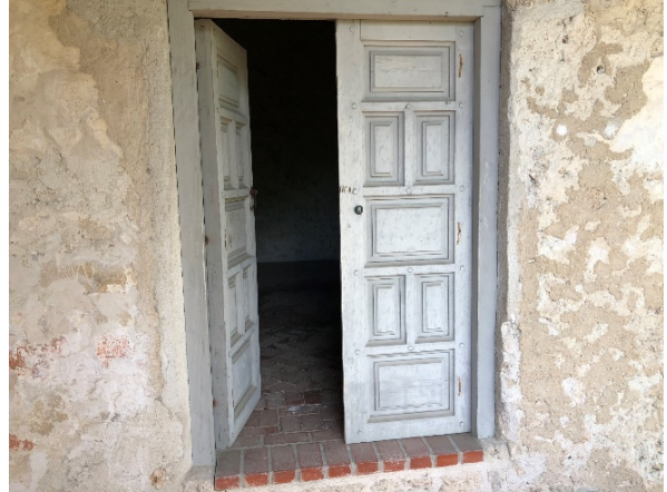
Figure 6.B.148: North wall. Door leading to Father President's office. Features brown mortar patching.
