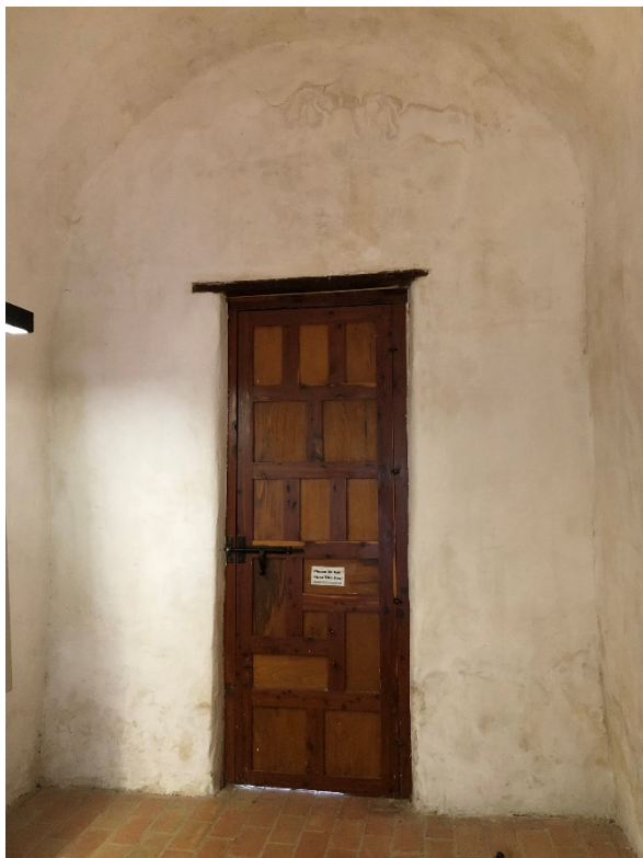
Figure 6.B.106: 104 F Refectory—South wall. Erosion of the painted surface and stains are located both on the lower portion of the wall and on the top, near the vault.
