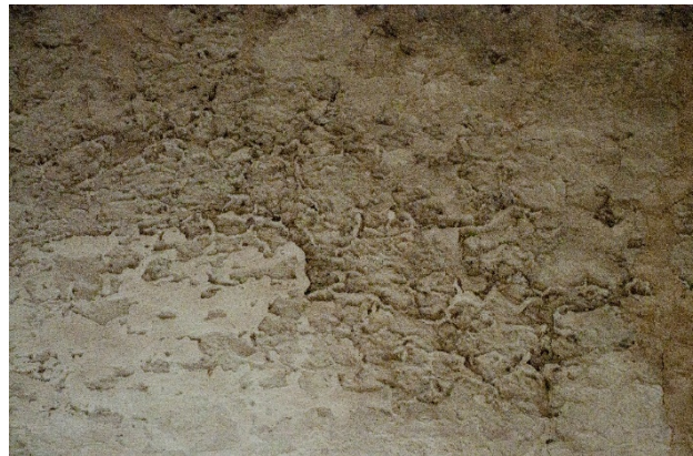
Figure 6.B.44: 104 B—South wall detail (D2, D3). The south wall of the storeroom has an extensive differential erosion of the plaster.
