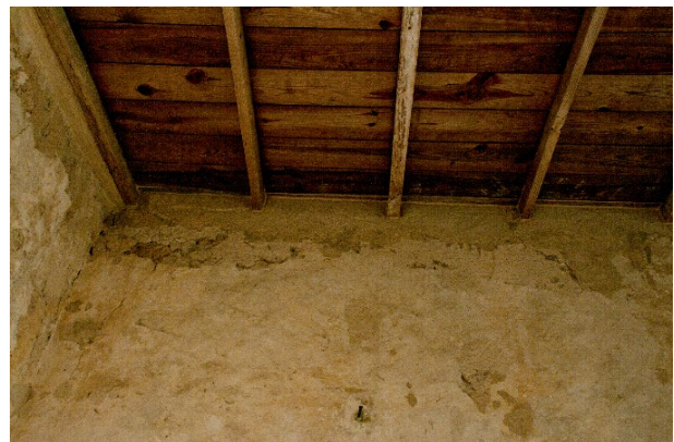
Figure 6.B.157: North wall. Upper left corner. Features a crack going down from the roof rafter, concrete patching on the upper part connecting to the roof, and disintegration of the plaster.
