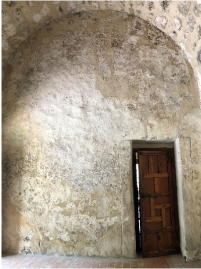
Figure 6.B.66: 104 D Portería—South wall. Historic plaster features large areas with differential erosion, the door architrave has a crack in the center.
