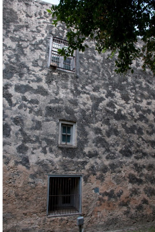
Figure 6.B.221: Exterior east wall, which features darkening of biological origin only on the tufa blocks. By contrast, the mortar repointing appears less receptive to biological colonization. Note the recent brown mortar patching on the lower portion of the wall.
