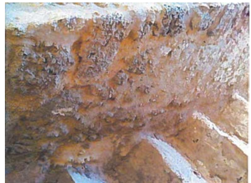
Figure 6.A.88: The stair wall required repointing featuring stone and mortar losses. Reprinted from Documentation of South & East Exterior Walls... , by Restoration Associates Limited, 2009, p. 8.
