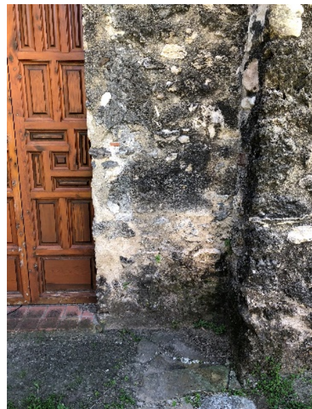
Figure 6.B.197: Right jamb of the door, where rising damp and high levels of moisture help the flourishing of biological growth.
