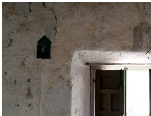
Figure 6.B.134: South wall (B5, C5, C4). Features several cracks, graffiti, and different types of patching.
