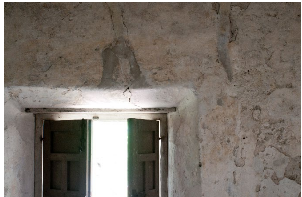
Figure 6.B.135: South wall (C4, C3, B3). Features several cracks, erosion of the painted finish, and missing parts of the plaster.
