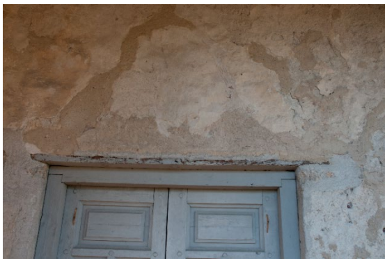
Figure 6.B.154: North wall. Area above the door. Features different types of mortar patching and an old crack that has been filled.
