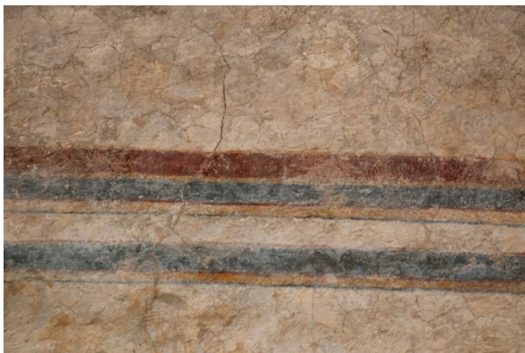
Figure 6.B.91: 104 E Library—South wall (C2, C3). It features decorative colored lines in the springer line of the vault and hair cracks in the historic plaster.
