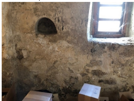
Figure 6.B.53: 104 C—East wall (A3, A4, B3, B4). High level of surface decay with efflorescence. Below the window sill are visible two major fractures around which mortar joints were repointed.
