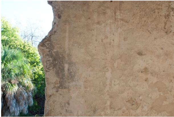
Figure 6.B.164: South wall. Middle area. Features well-executed patching that allows for the continuity of the plaster, remnants of painted plaster and graffiti.
