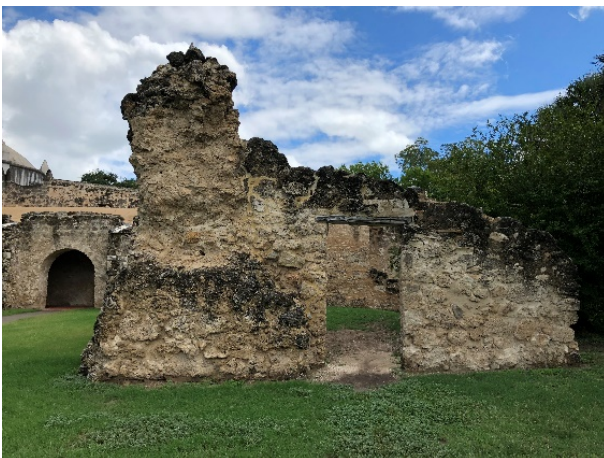
Figure 6.B.205: The west ruined wall has an irregular shape, due to the collapsed vaults. Masonry of the uppermost is in fragile condition.
