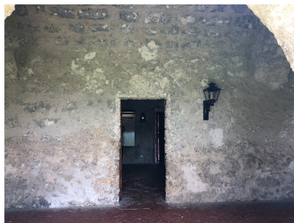
Figure 6.B.9: 104 A—East wall with door toward porteria. Around the door opening, large areas where limewash was applied directly on the tufa rubble masonry are visible.
