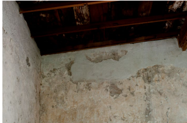
Figure 6.B.139: West wall (D4, D5). Shows the latex paint added in 1980s and erosion of the historic plaster.
