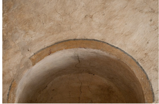
Figure 6.B.89: 104 E Library—South wall (B4, C4). Upper part of the 'bookshelf' niche. It features several hair cracks, including one in the middle of the arch. Discoloration of the historic plaster.
