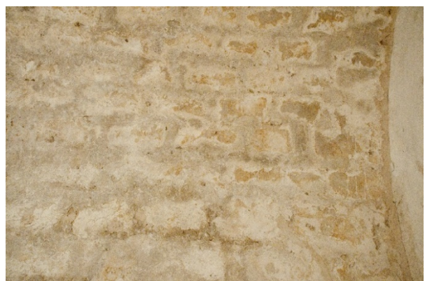
Figure 6.B.50: 104 B—Northwest part of the ceiling (C1, D1). Restoration mortar joints show discoloration due to efflorescence.
