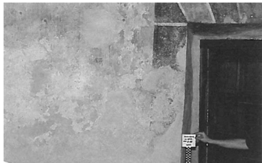
Figure 6.A.56: Sector EB5. Voids (detachment from the substrate) were identified in the area, showing also nails and iron pins. Stabilization was a chronic problem in this area.
