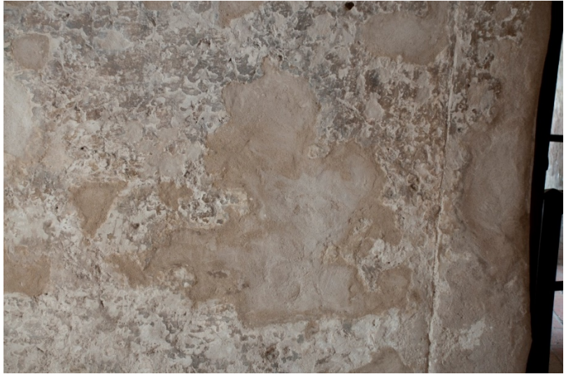
Figure 6.B.67: 104 D Portería—South wall left jamb of the door (A1, A2, B2). The remnants of historic plaster feature discoloration and differential erosion. Visually intrusive patchings were added to give continuity to the plaster.
