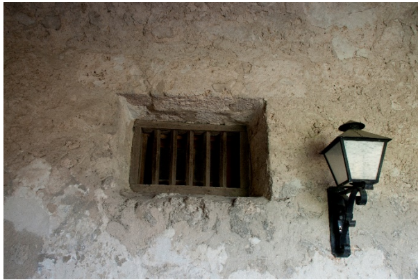
Figure 6.B.12: 104 A—East wall (B4, B5, C4, C5). Small window that connects with the storeroom. At the bottom part of the window there is some erosion of the historic plaster.
