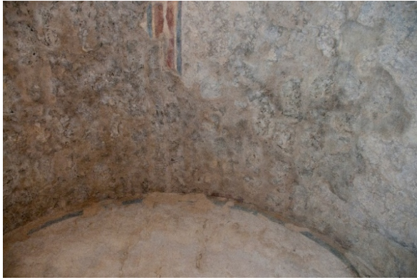
Figure 6.B.93: 104 E Library—South wall, connection of the south wall and the vault. The vault is crossed by a hair crack that goes through the middle, and when it approximates the walls divides in two in a Y shape.
