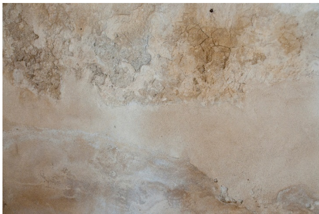
Figure 6.B.81: 104 E Library—East wall (A7, B7). Patching in the bottom part that features high level of efflorescence, and the upper part shows craquelé and delamination of the plaster layers.
