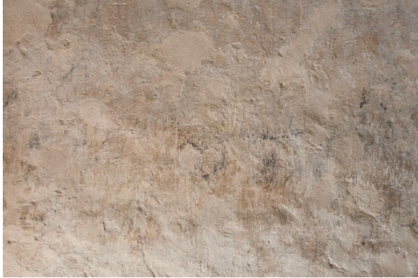
Figure 6.B.99: 104 E Library—West wall (B6). Its surface features well-executed and visually compatible patching, discoloration and historic incisions of the painted finish.
