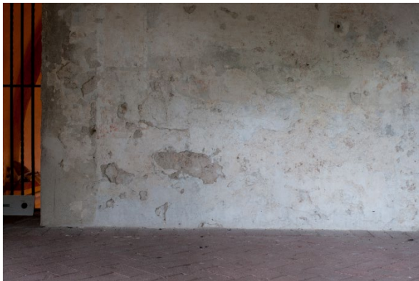
Figure 6.B.128: North wall (A4, A5, A6). Exhibits missing parts, differential erosion of the plaster and patching on the jamb of the door.
