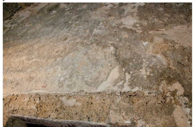
Figure 6.B.25: 104 A—Corridor. South wall (B2, B3), at least two layers of plaster are visible in the architrave of the door leading to the refectory. The area with no plaster on the architrave indicates that it was covered by a door frame, probably removed during some restoration work.
