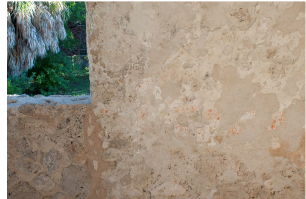
Figure 6.B.167: South wall. Detail of the connection of the wall with the parapet. Features different types of patching, remnants of painted plaster (red/orange color), and historic graffiti.
