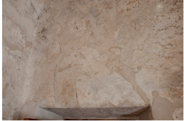
Figure 6.B.57: 104 D Portería—North wall (B4, C4). Architrave of the door leading to the storeroom. Features hair cracks in the patching plaster (probably added to repair a structural crack) and erosion of the painted plaster.
