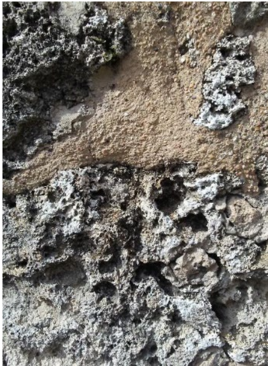
Figure 6.B.217: Brown mortar joints between heavily eroded stones.
