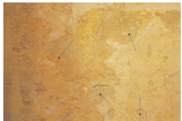
Figure 6.A.79: South wall. Arrows indicate cement plaster and historic plaster loss. Reprinted from Exposing Historic Wall Plasters... , by Restoration Associates Limited, 2008, p. 14.
