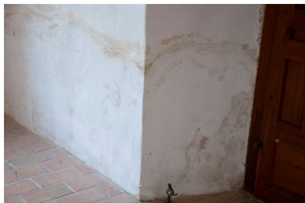
Figure 6.B.117: 104 F Kitchen. Rising damp in the wall, which produces stains and erosion of the surface.
