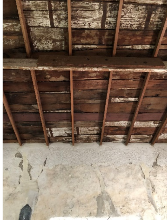
Figure 6.B.123: Ceiling and part of south wall. Cracks reach the ceiling.
