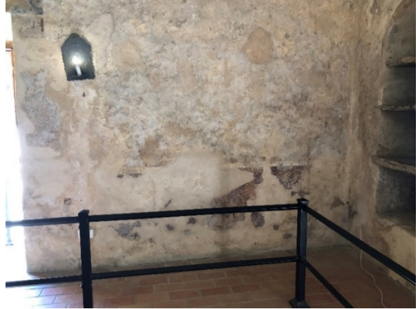
Figure 6.B.84: 104 E Library—East wall. Has multiple patchings. Painted plaster has erosion.
