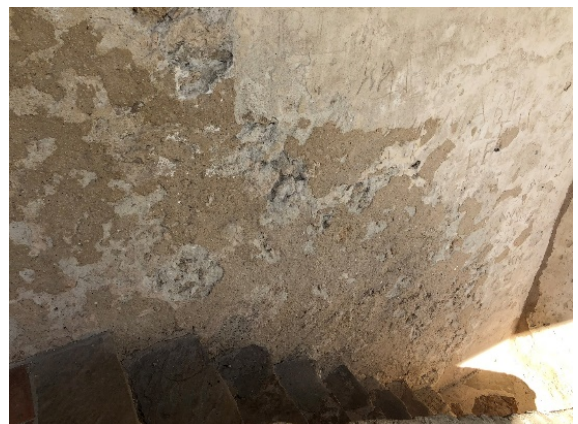
Figure 6.B.172: North wall of the staircase features brown patches that are visually not compatible, graffiti, and parts of missing mortar.
