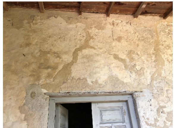
Figure 6.B.150: North wall. Area above the door. The door architrave features a filled crack starting from the left corner.
