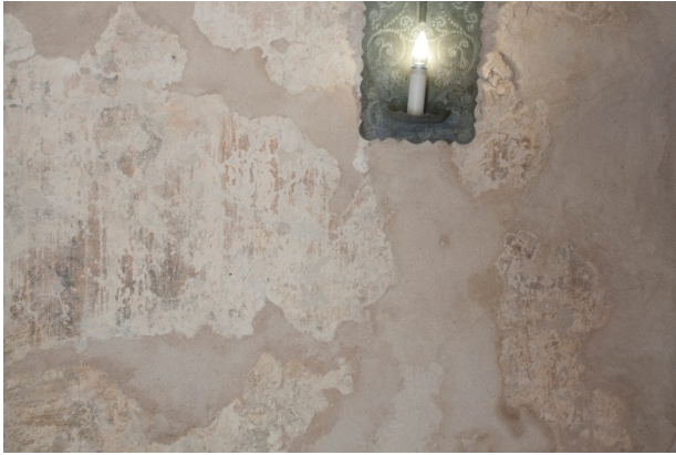
Figure 6.B.74: 104 D Portería—West wall (B4, B5), intrusive patching with discoloration in the edges and colored historic plaster with historic incisions and discoloration.
