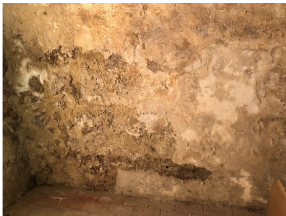
Figure 6.B.51: 104 C—Northern corner of the east wall (A6, A7, B6, B7). Surfaces feature a high level of deterioration with loss of plaster and abundant fluffy efflorescence.
