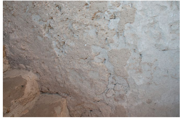
Figure 6.B.153: North wall. East end, view toward the steps. A crack separates the steps from the wall. Patches of different generations cover the wall surface.
