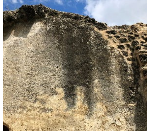
Figure 6.B.202: Segment B close up. The 18 th century plaster is covered by a thick patina of biological origin with typical rain flow marks.
