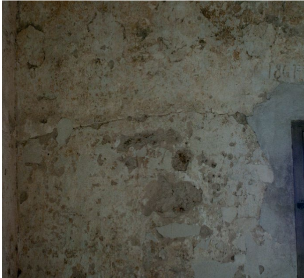
Figure 6.B.138: West wall (B4). Features numerous missing parts, a horizontal hair crack starting at the corner of the window, and visually intrusive patching at the jamb of the window.
