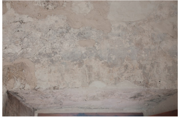
Figure 6.B.75: 104 D Portería—West wall, architrave of the door leading to the corridor (C3, C4). It features craquelé and historic incisions in the historic plaster and different types of patching, one brownish in the upper part of the wall and another more grayish in the architrave of the door.
