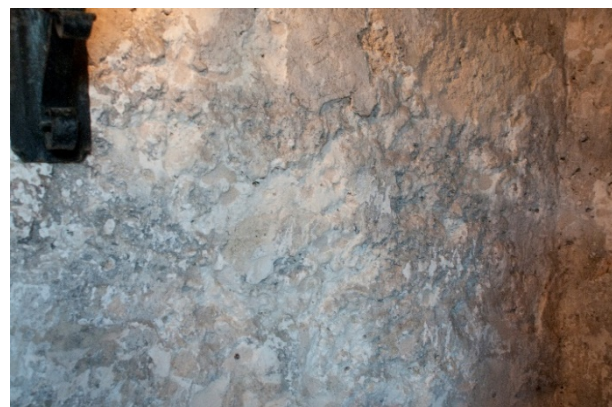
Figure 6.B.26: 104 A—Southern corner of the east wall (B18). The wall has different layers of plaster, and it features differential erosion of the painted plaster, detachment of edges, and graffiti.
