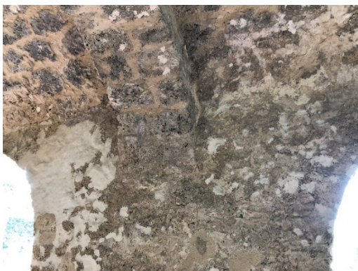
Figure 6.B.28: 104 A—West wall (C10, C11, C12), showing natural hydraulic lime-based mortar patchings that are compatible with the masonry but visually intrusive.
