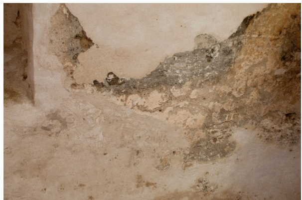
Figure 6.B.60: 104 D Portería—North wall, area right of the niche (A1, A2). Remnants of colored historic plaster that is highly eroded and numerous visually intrusive patches.
