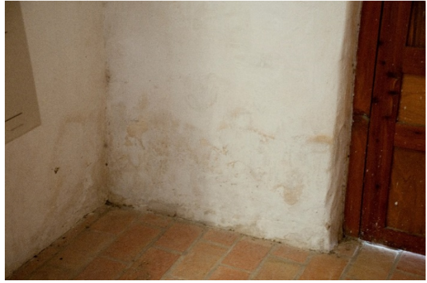
Figure 6.B.114: 104 F Refectory—South wall. Rising damp in the wall, which produces stains.
