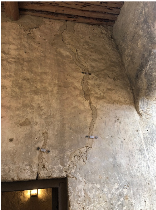
Figure 6.B.176: North wall has deep fractures filled with mortar. The wall may need stabilization.
