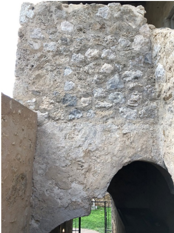
Figure 6.B.171: West wall of the staircase features patches of mortar possibly done in different times.
