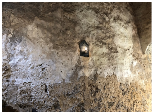
Figure 6.B.177: South wall features mortar patching of different periods and its partial erosion.
