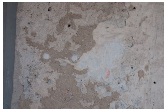
Figure 6.B.155: North wall. Area right of the door. It exhibits different types of mortar patching (one brownish and one grayish), traces of historic painted plaster (red/orange color), historic graffiti, and missing parts.
