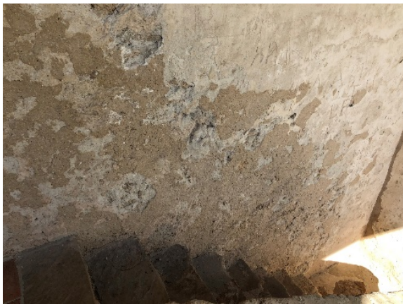
Figure 6.B.149: North wall. East section of the wall, above the stairs. Exhibits several missing parts and brown mortar patching.
