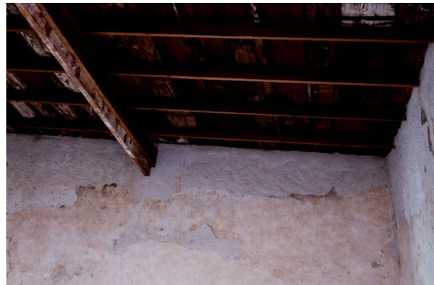
Figure 6.B.131: East wall (D1, D2, D3). Exhibits several visually intrusive patchings.
