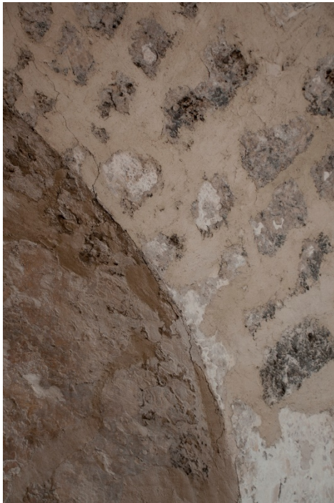
Figure 6.B.70: 104 D Portería—Southwest corner (C1, D1). Features a hair crack that starts at the corner and then extends to the vault, erosion of the painted finish of the historic plaster, and roughly executed brown mortar repointing in the masonry of the vault. Some stones have remnants of whitewash.
