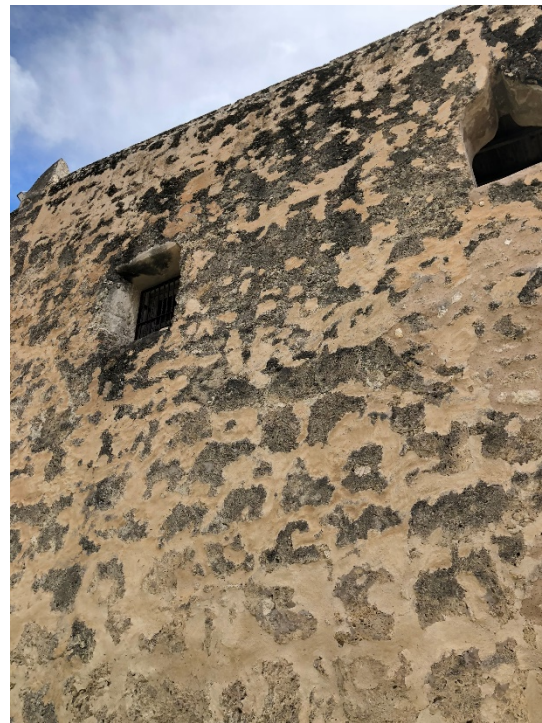
Figure 6.B.227: Exterior west wall. Upper part of the wall features brown mortar repointing, roughly executed, covering part of the stone. The tufa stone has a dark color, due to biological growth imbued into the stone cavities.
