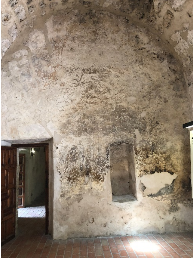
Figure 6.B.56: 104 D Portería—North wall. High level of surface decay with efflorescence. Fractures on the windowsill.
