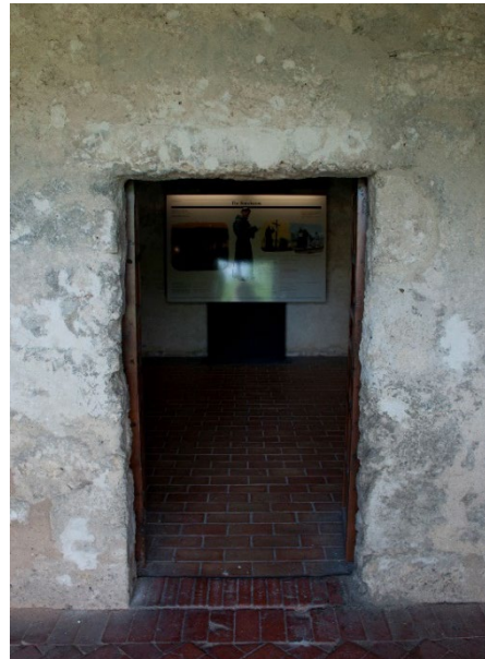
Figure 6.B.13: 104 A—East wall (A6, A7, B6, B7), door leading to the storeroom. On the left side of the door, a fragment of red painted plaster is still visible. The surrounding areas feature erosion of the historic plaster. The door architrave features extremely well-executed patching, perfectly blended with the surrounding areas. Their execution can be considered a reference point for future interventions
