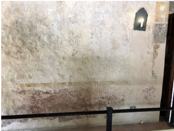
Figure 6.B.95: 104 E Library—West wall, the painted plaster features erosion.
