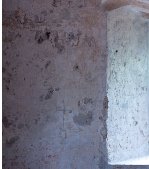
Figure 6.B.132: East wall (B4, B5). Features several intrusive patches, historic graffiti, and painted plaster (red/orange color) on the bottom part.
