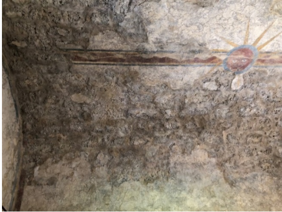
Figure 6.B.83: 104 E Library—On the ceiling, a crack is visible in the middle of the vault from north to south. The vaulted ceiling surface features several craquelé, detachment of edges, and loss of joints on mortar.
