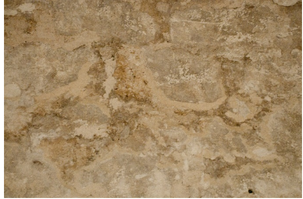
Figure 6.B.46: 104 B—Southwest part of the ceiling (D6, D7). Features differential erosion of plaster stabilized in a previous conservation campaign.
