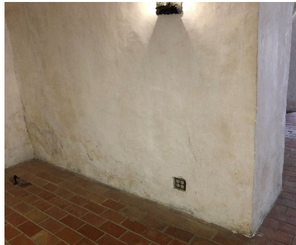
Figure 6.B.107: 104 F Refectory—West wall. Stains due to rising damp are visible on the south west corner.
