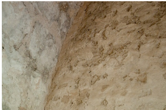
Figure 6.B.43: 104 B—Southeast corner (C4, D4). Features hair cracks in the corner plaster patching (which was probably added to repair a structural crack), and differential erosion of the historic plaster in the south wall.
