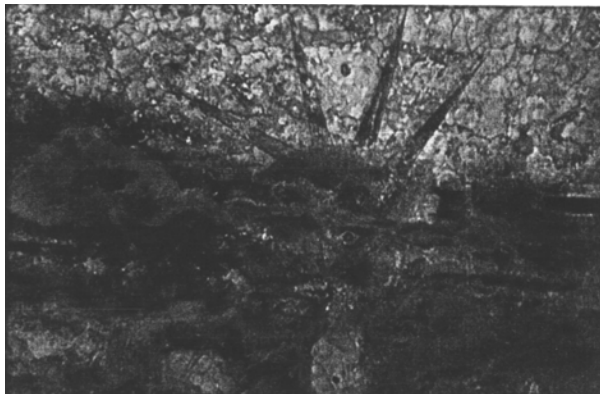
Figure 6.A.6: Vaulted ceiling in the library at mission Concepción with a detail of the “Eye of God,” showing patches and 20 th -century repairs. Reprinted from Summary Project Report for the Paint and Plaster Conservation... , by Anthony Crosby, 1988, p. 12.
