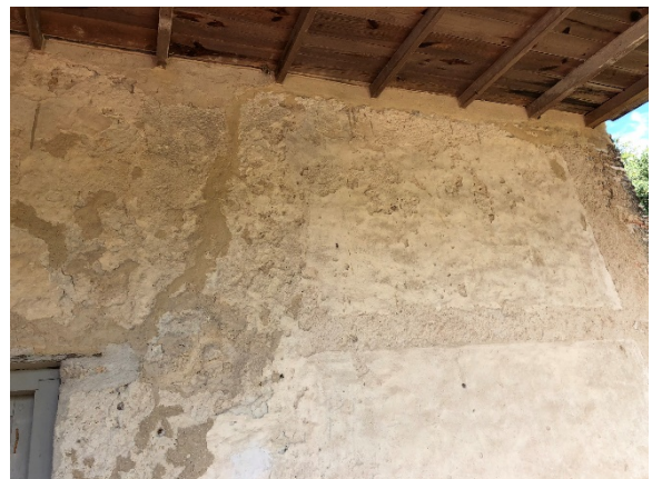
Figure 6.B.151: North wall. Upper east corner. Shows historic graffiti and mortar patching in the shape of a horizontal line.
