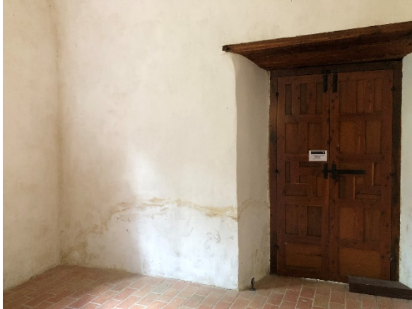
Figure 6.B.108: Room 104 F Kitchen—North wall toward the west corner. Rising damp up to approximately 2½ ft. produced erosion and detachment of the modern paint layer.
