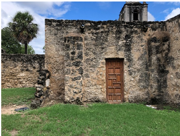
Figure 6.B.203: South wall (segment D), corresponding to the kitchen. Features darkening of biological origin with flow marks from the parapet.
