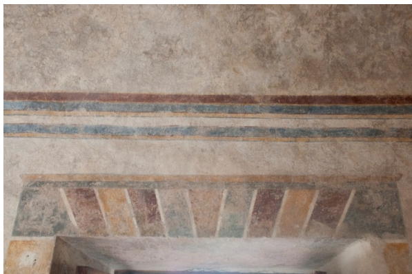
Figure 6.B.102: 104 E Library—West wall (C2, C3). Detail of the painted faux voussoirs above the door and painted architectural bands at the vault's springer line. They feature erosion of the painted finish and discoloration.
