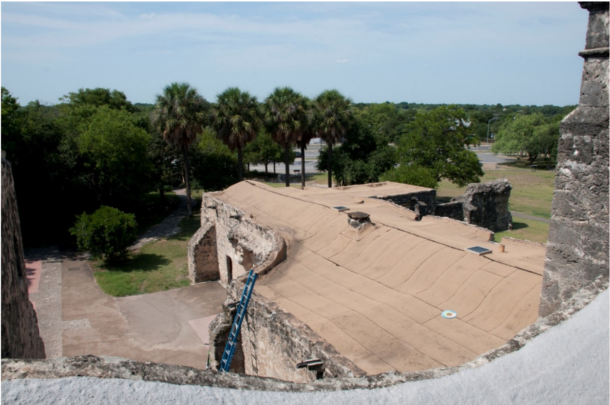
Figure 6.B.230: Convento roof. View from roof of the church. The asphalt-base roof is still performing correctly, but it has reached the end of its useful life. It requires a redesign to improve rainwater drainage in some areas. The most urgent areas are the north and east.
