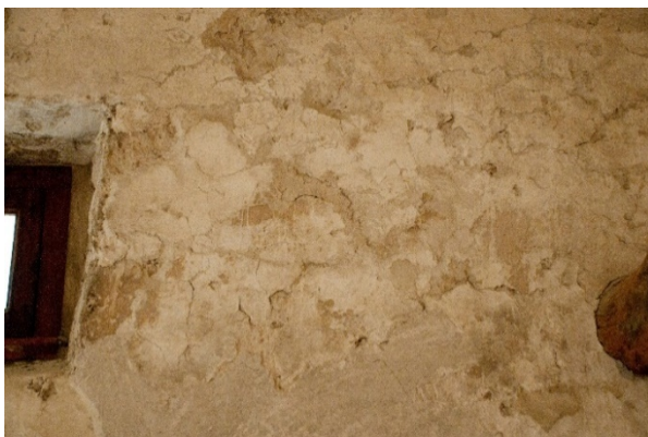
Figure 6.B.49: 104 B—West wall (B3, C3). Part between the small window and the southern timber beam features craquelé and differential erosion of the historic plaster.
