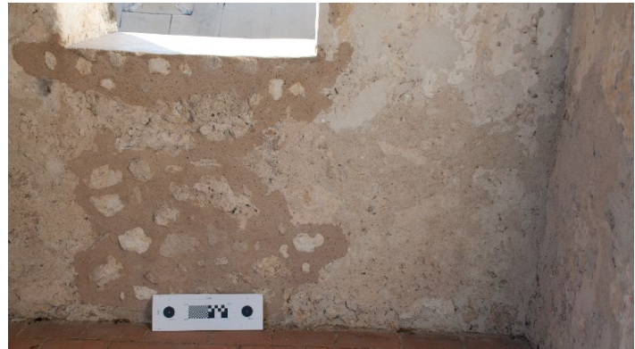
Figure 6.B.161: West wall. Bottom part of the wall under the Moorish style window. It features different types of mortar patches, the large brown patching is unfinished and visually contrasting.
