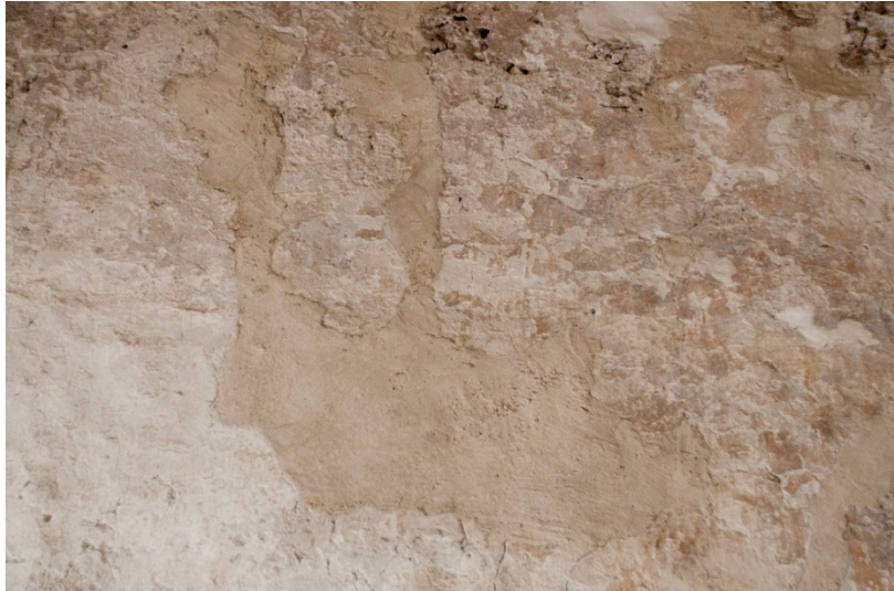
Figure 6.B.69: 104 D Portería—Upper part of the south wall (C2, D2). Showing plaster patching and discoloration and erosion of the historic plaster.
