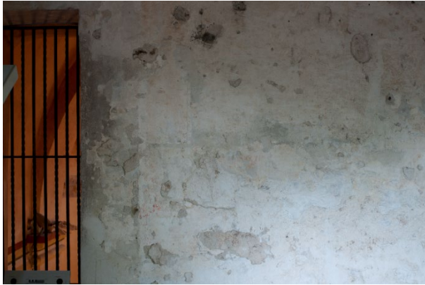
Figure 6.B.126: North wall (B5, B6). The area features numerous missing parts of the plaster.
