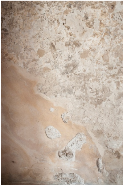
Figure 6.B.68: 104 D Portería—Left corner of the south wall (A3, A4). At the bottom left part of the image, blistering, efflorescence and detachment of the patching are visible. And at the upper right we see historic plaster featuring discoloration, differential erosion, and graffiti.
