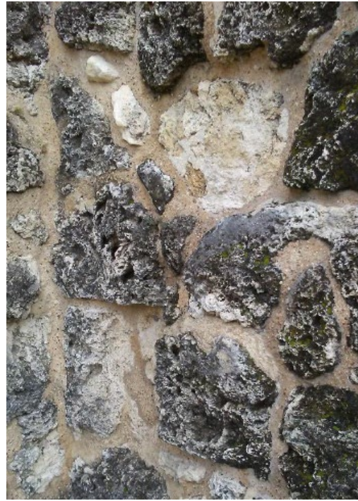
Figure 6.B.191: Detail of buttress with evident biological colonization.
