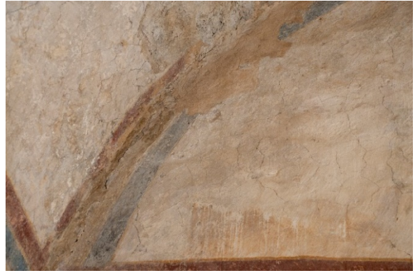
Figure 6.B.94: 104 E Library—South wall (D4), shows hair cracks, discoloration with flow marks, and historic incisions of the plaster. Intrusive brownish patching.
