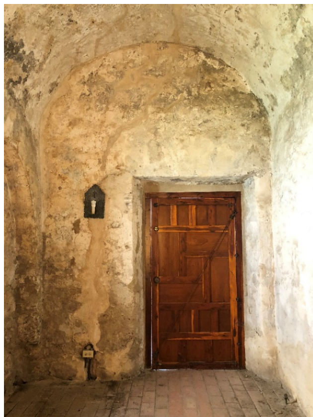
Figure 6.B.55: 104 C—South wall. Patching and filled fractures are observed on a historic plaster featuring a high level of erosion.
