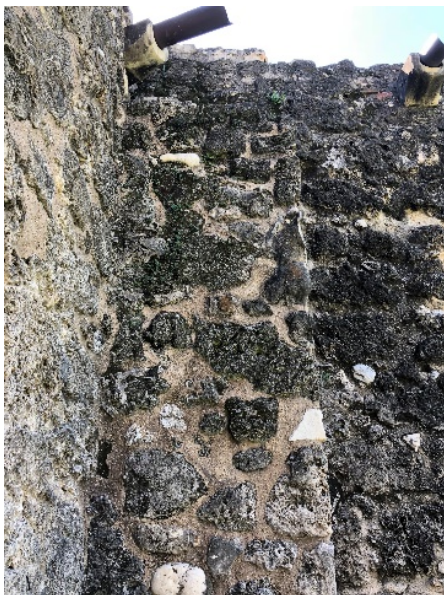
Figure 6.B.196: Buttress located at the corner between north and west facade is characterized by a rich biological growth, also exacerbated by the presence
