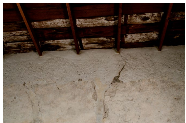
Figure 6.B.137: South wall (D2, D3, D4). Exhibits a crack starting from the wooden rafter and extending downward.
