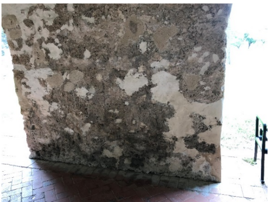
Figure 6.B.29: 104 A—West wall (A10, A11, A12, B10, B11, B12). Different types of mortar patching are visible: brown mortar and natural hydraulic lime-based mortar. Both are visually contrasting.
