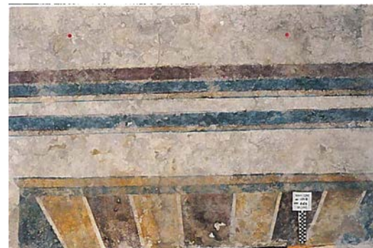
Figure 6.A.55: Sector EC4. Minute blisters, pattern cracks and one large crack were identified in this area.
