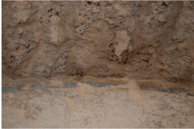
Figure 6.B.80: 104 E Library—North wall (E3). Upper part of the north wall, connection with the vault. Features hair cracks, patching, and erosion of the painted finish.
