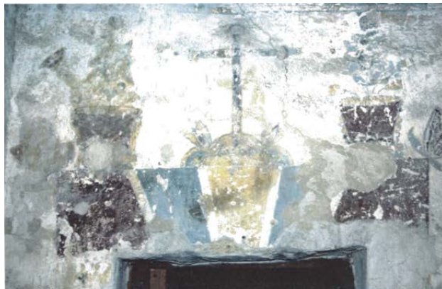
Figure 6.A.50: Pre-treatment condition of north door of the library, July 1986. Reprinted from 1988 Conservation Project Completion Report... , by Anthony Crosby, 1997, p. 61.
