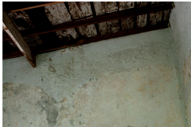
Figure 6.B.140: West wall (D1, D2, D3). Shows the latex paint added in 1980s and erosion of the historic plaster.
