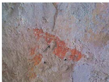
Figure 6.A.91: Areas showing edge stabilization, Portland cement patches overlapping Spanish Colonial plaster and graffiti. Reprinted from Documentation of South & East Exterior Walls... , by Restoration Associates Limited, 2009, p. 10-11.
