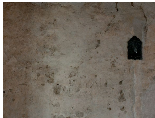
Figure 6.B.136: South wall (B5, B5, C5, C6). Exhibits numerous missing parts, graffiti, and erosion.
