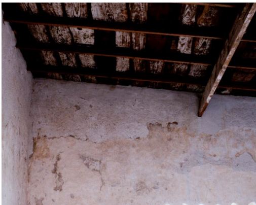
Figure 6.B.130: East wall (D4, D5, E4, E5). A crack is visible in the corner of the wall. Under the ceiling is a large area with latex paint.
