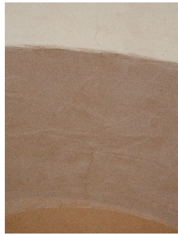
Figure 6.B.116: 104 F Kitchen. Hair crack in the middle of the arch in between the refectory and the kitchen.
