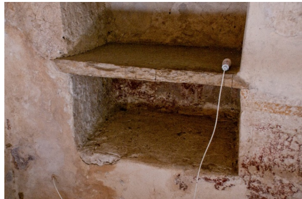
Figure 6.B.90: 104 E Library—South wall (A3, A4). Detachment and discoloration of the brownish patching on the bottom left of the 'bookshelf.' Around and inside the bookshelf there is erosion of the painted finish. All the southeast corner of the library should be an area of concern.
