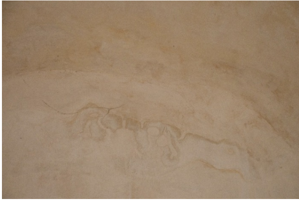
Figure 6.B.113: 104 F Refectory—South wall. Stain due to water infiltration from the roof and wall.
