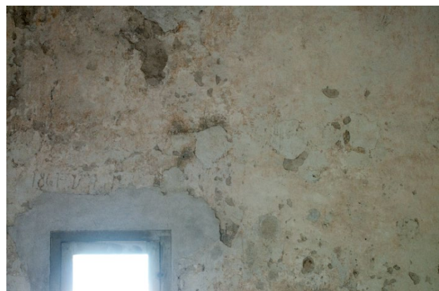
Figure 6.B.142: West wall (B3, B2, C3, C2). Features visually intrusive patching surrounding the window, historic graffiti, and numerous missing part of the painted finish and the plaster.
