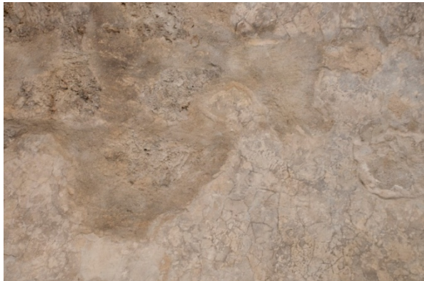
Figure 6.B.101: 104 E Library—West wall (D6). Craquelé of the historic plaster and roughly executed mortar repointing on the masonry of the vault, partially covering the stones.
