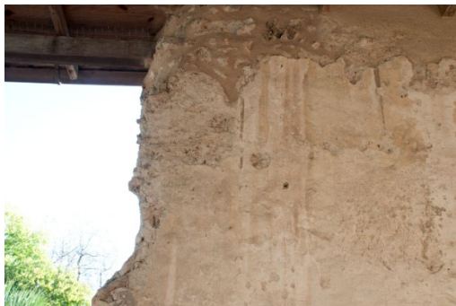
Figure 6.B.162: South wall. Upper left part. Features brown mortar patching near the connection with the roof and discoloration of the plaster.
