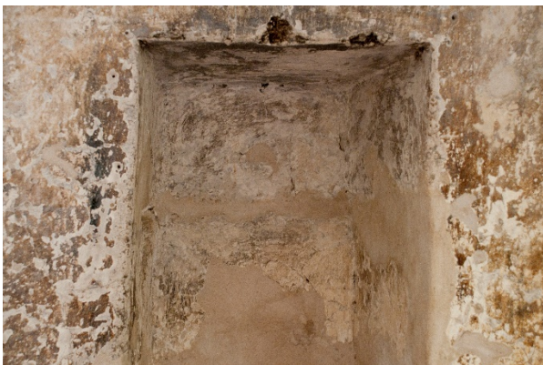
Figure 6.B.59: 104 D Portería—Niche of the north wall (B2). Features hair cracks and plaster patching inside the niche, and erosion of the painted plaster outside the niche.
