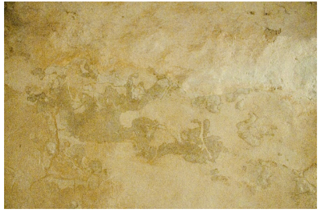
Figure 6.B.40: 104 B—East wall (B6, B7). Area in between the two timber beams. Plaster patching repair was added until this point, which also features a high level of humidity.
