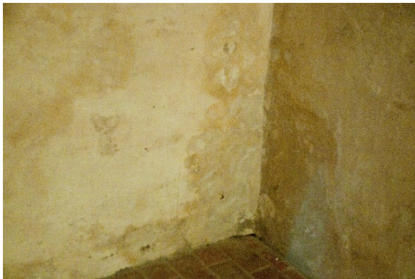
Figure 6.B.37: 104 B—Northeast corner (A1). This corner connects to the guest room to the right and to the exterior (where the air-conditioning is currently in place) to the northeast, and it features a high level of humidity and efflorescence.
