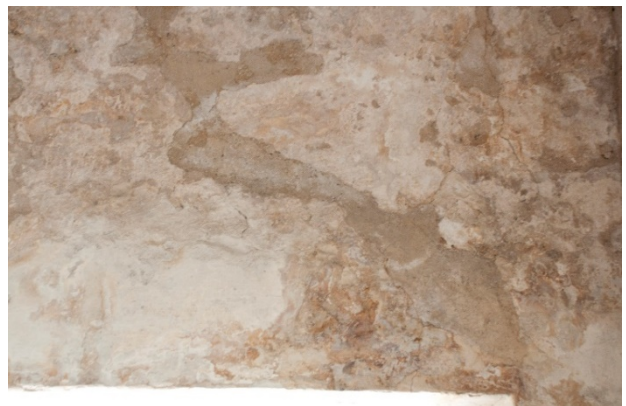
Figure 6.B.65: 104 D—East wall (C1), architrave of the door features eroded remnants of colored plaster and a visually intrusive plaster patching.
