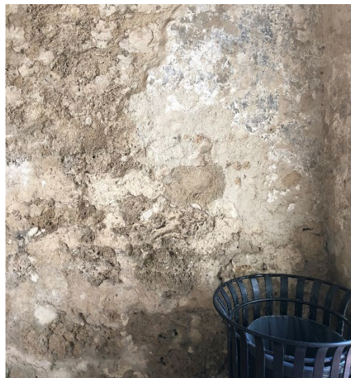
Figure 6.B.31: 104 A—Northern corner of the west wall (A18, B18). Powdering and differential erosion of the historic plaster.
