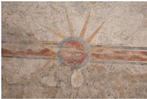
Figure 6.B.85: 104 E Library—Ceiling detail (F4, G4). Detail of the central painted decoration, which is characterized by a filled crack featuring a pinking mortar. A newer hair crack passes across the decoration. Craquelé in the plaster is also visible. Roughly executed mortar repointing covers a little corner of the drawing.
