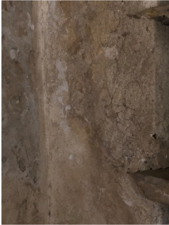
Figure 6.B.88: 104 E Library—South wall, featuring efflorescence and several hair cracks.
