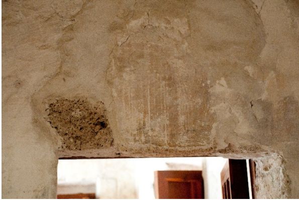
Figure 6.B.45: 104 B—South wall (B1, C1). Architrave of the door connecting with the porteria. Historic plaster featuring erosion, hair cracks, plaster patching, and historic incised patterns.
