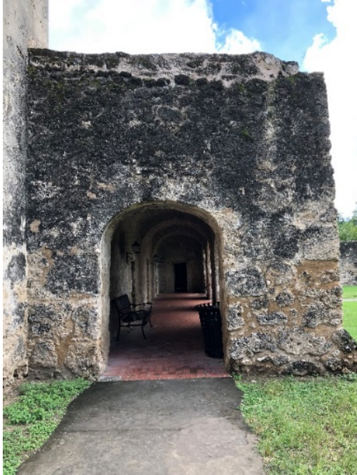
Figure 6.B.178: Exterior north elevation of the corridor. Dark film of biological growth featured on the top part.
