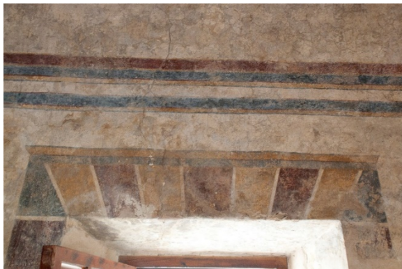
Figure 6.B.86: 104 E Library—Ceiling detail (C3, C4, C5). Decorative painted plaster around the door, representing faux voussoirs, and at the springer line of the vault. A crack in the architrave of the door is visible. Craquelé in the plaster and erosion of the painted finish.
