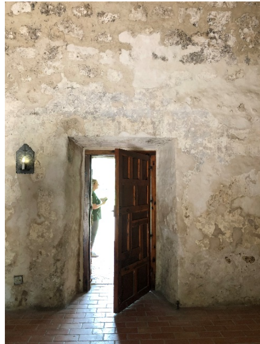
Figure 6.B.71: 104 D Portería—West wall, large patching interrupts the continuity of the historic plaster finish.
