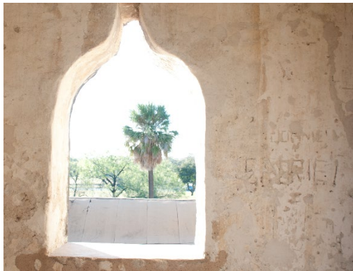
Figure 6.B.160: West wall. Moorish style window. Features different types of patching and historic graffiti.
