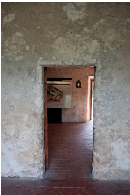
Figure 6.B.14: 104 A—East wall (A11, A12, B11, B12), door leading to the portería. Around the door several types of mortar patching can be found.
