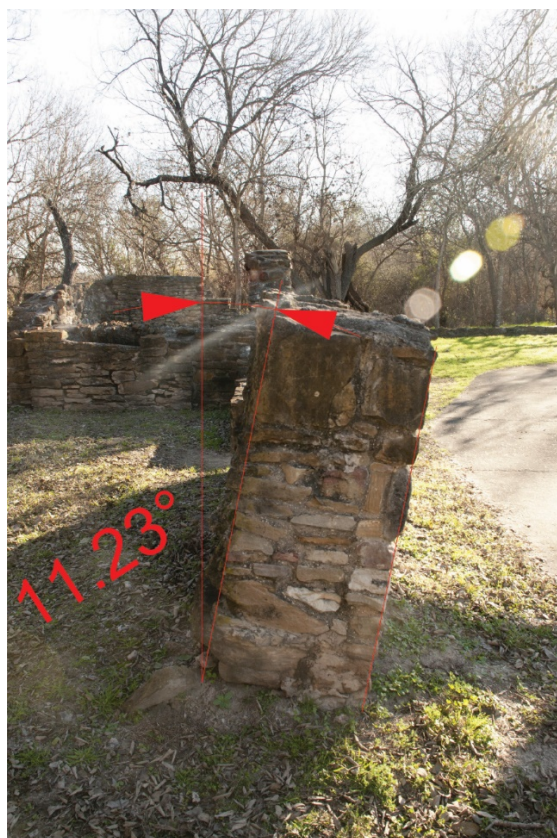
Figures 3.1 (left) and 3.2: Side views looking east of the north gate illustrating the severity of its lean. The west section of the wall does not lean as dramatically as the east section.
