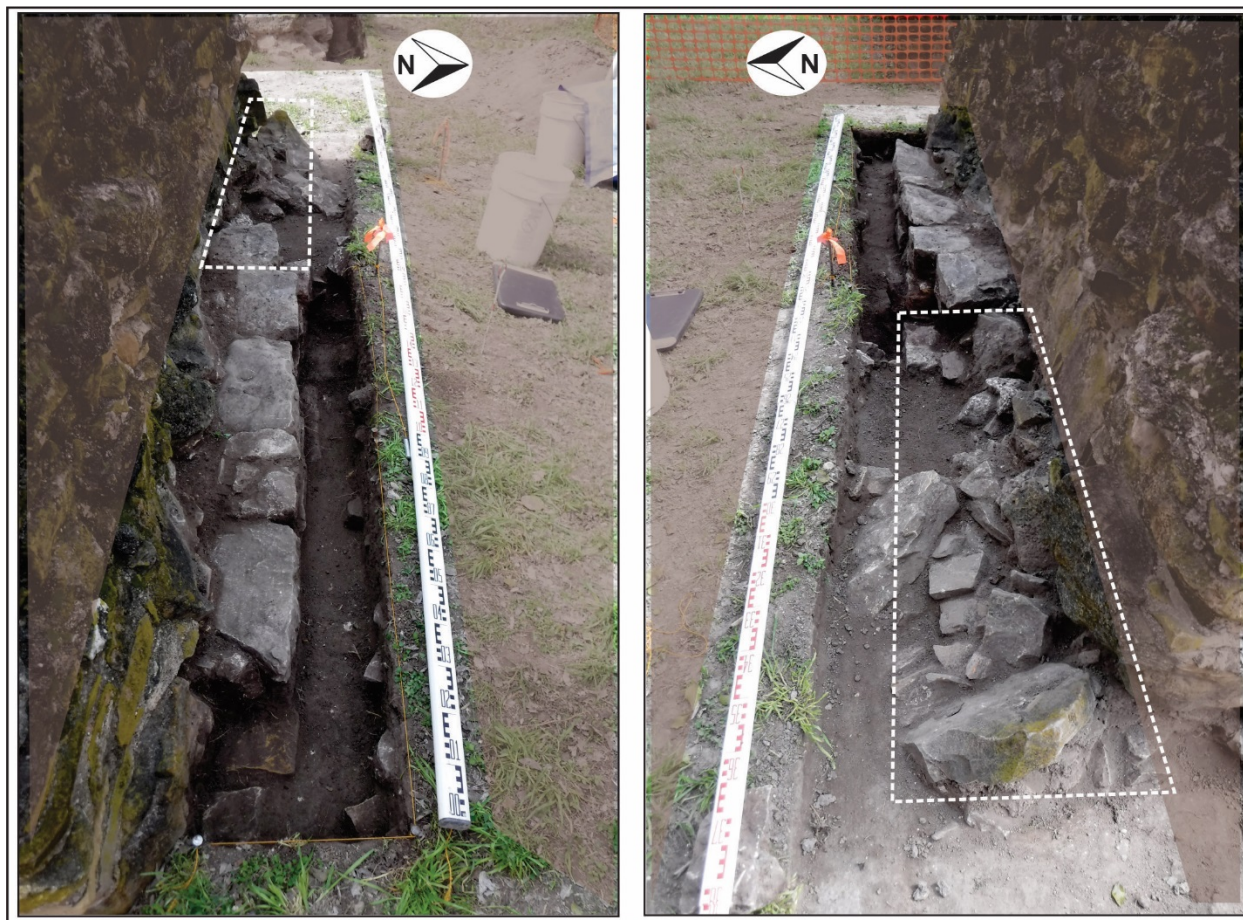
Figures 4.11 and 4.12: East wall segment—view west (left) and view east (right); note poorly reconstructed section (outlined).
