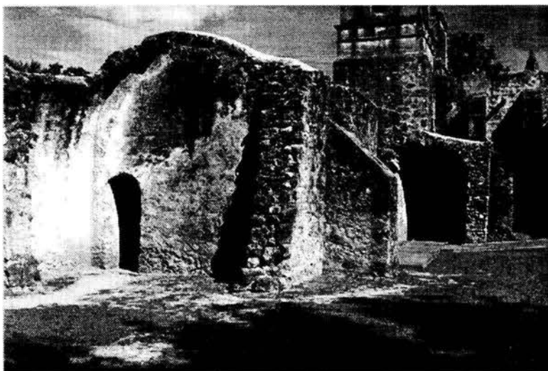
Figure 49. Ruins of exterior wall and collapsed barrel vault roof at south side of convento.
