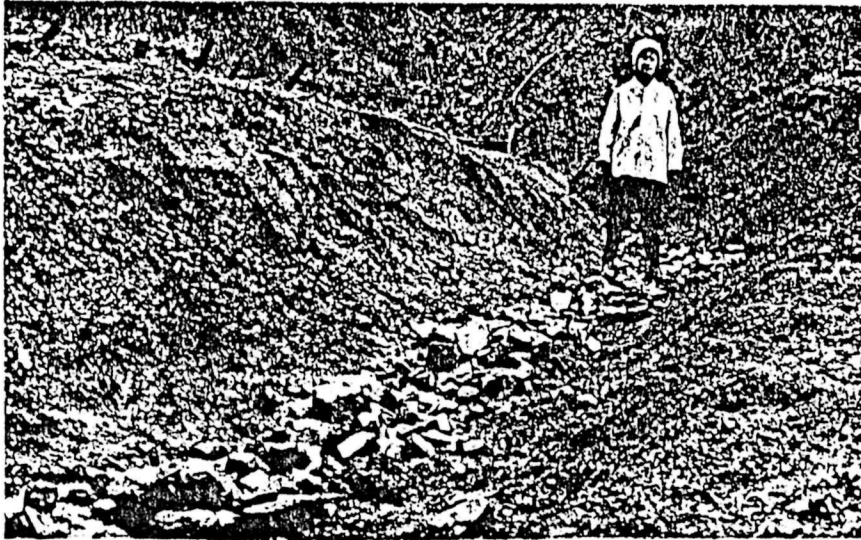
Photo 11: Cross road drain lined with coarse rock to prevent downcutting. C-90 Road, Harry Weir (Emerald) Creek.
