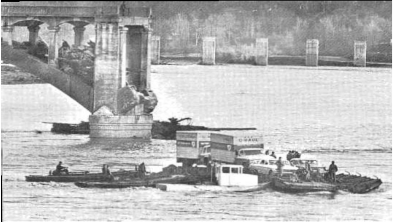
Figure 29. The Fourth Infantry engineers ferried vehicles across the Klamath River for two months after floods took out a span of the Douglas Memorial Bridge pictured behind (east) of the ferry. Piers for the replacement (and current) bridge are in the background. The 1965 bypass and new bridge began construction before the flood. A temporary span across the destroyed bridge section was erected about two and a half months after the flood and the current bridge was completed later that year (Eureka Newspapers, Inc. from California Highways and Public Works 1965).
