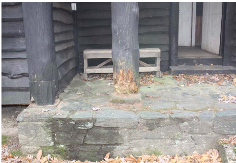
Building 1-50, Administration Building, deterioration of the wood column
