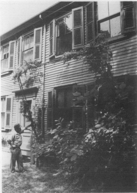
Figure 4. The pipe and strapping system, constructed with swivel sockets, allows the rigid support system to fold down away from the house. The strapping can also be removed from the pipe support for limited maintenance. Photo by Karen Day.
