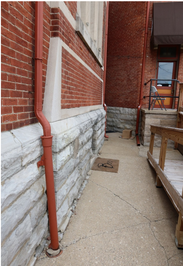
Figure 2.46: Downspouts drain to the ground near the building or to subsurface drain tiles. This appears to be a likely contributor to water infiltration in the basement.
