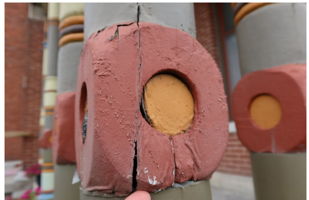
Figure 2.20: Deterioration at lower part of porch post.
