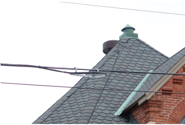
Figure 2.43: Roof of cellblock. Note loose and missing shingles at upper part of hip.
