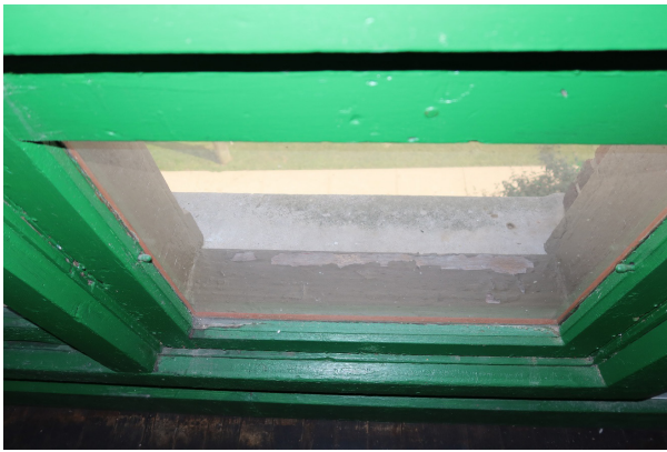
Figure 2.31: Typical historic wood window at jail attic showing overall condition. Note peeling paint on exterior sill.
