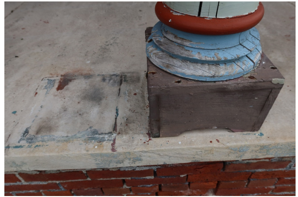
Figure 2.19: Typical deterioration to new-growth wood at replacement base of porch post.
