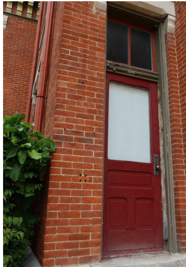
Figure 2.37: Dining room door. this door needs to be restored and should be fitted with a new storm door.
