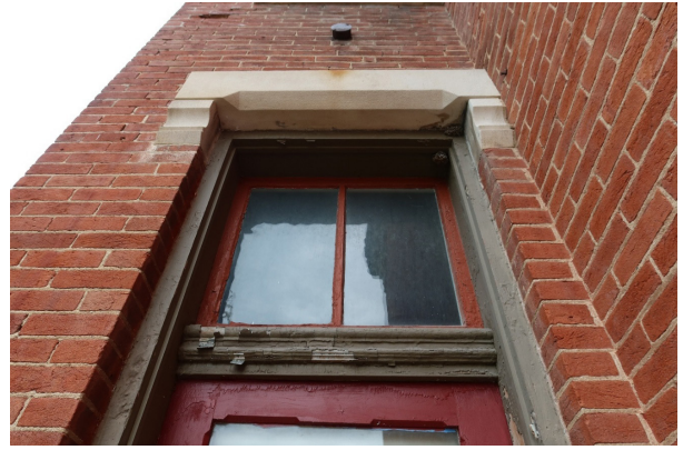
Figure 2.40: Paint failure at transom bar of dining room door.
