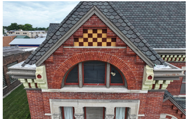
Figure 2.28: The cornice appears to be slightly displaced on either side of the east gable. (Drone photo by Arsee).
