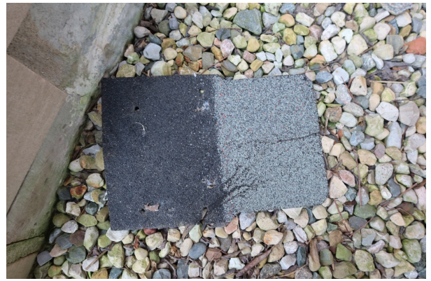
Figure 2.44: Loose shingle on the ground next to cellblock.
