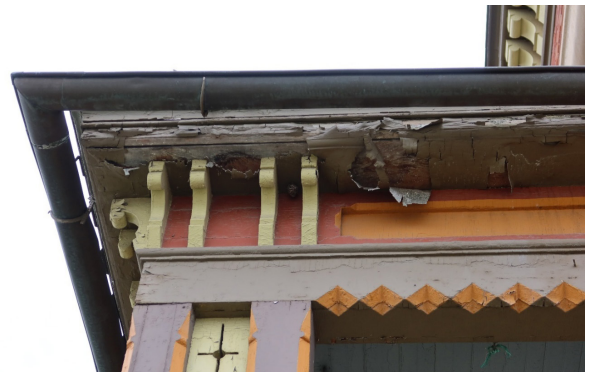
Figure 2.21: A leaking gutter is causing deterioration to the north end of the porch.
