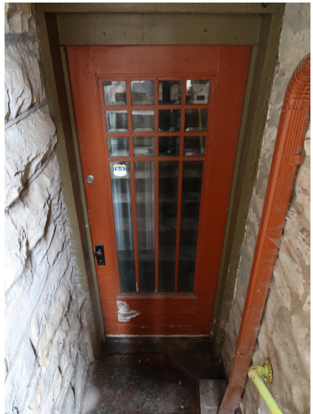
Figure 2.42: Basement door showing paint failure and damp conditions at areaway.
