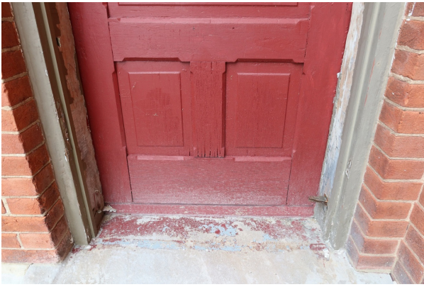
Figure 2.38: Dining room door showing paint failure and weathering since removal of storm door around 2006.
