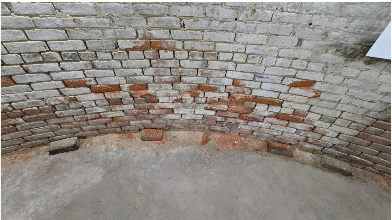
Figure 2.9: Damage is believed to be caused by rising damp.
