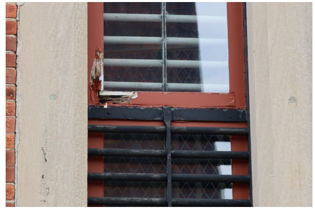
Figure 2.34: Typical deterioration of non-historic replacement windows at cell block.
