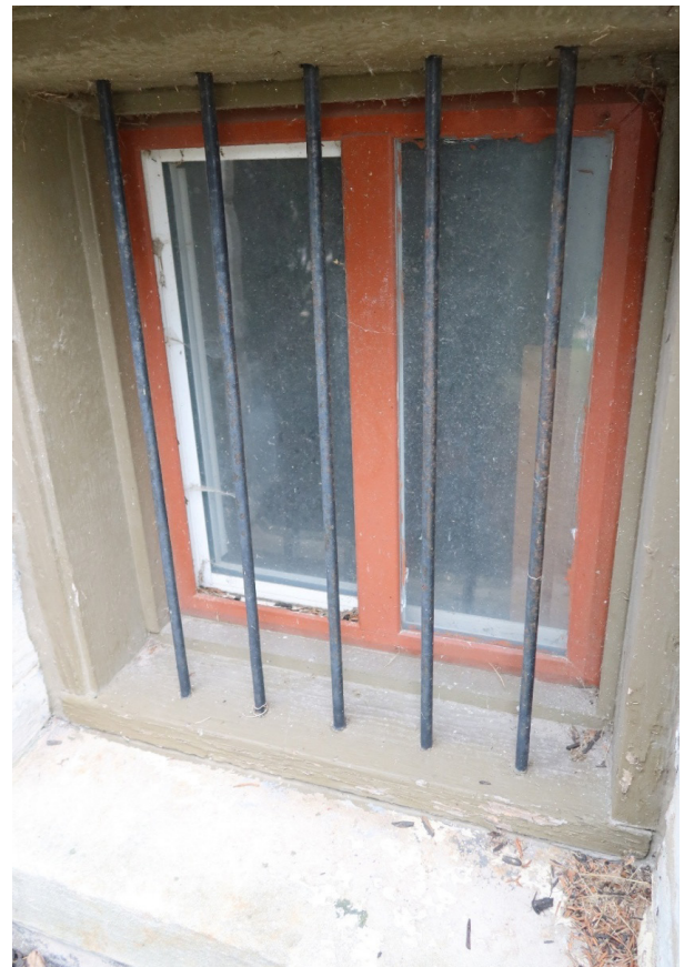
Figure 2.35: Non-historic basement window. This window is missing its screen (left).
