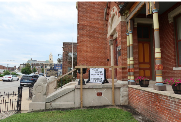
Figure 2.23: The museum's insurance provider required the addition of a handrail to the north side of the front porch. The handrail is bolted into the ends of the stone stoop slabs. This is likely to cause cracking and deterioration of the stone over time. Consider future replacement with a less intrusive metal railing.
