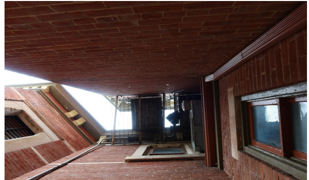
Figure 2.27: Missing brackets at notch between house and jail (left). These appear to have been salvaged to replace missing brackets in more visible locations.
