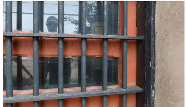
Figure 2.41: Typical deterioration of paint finishes at guard room door.
