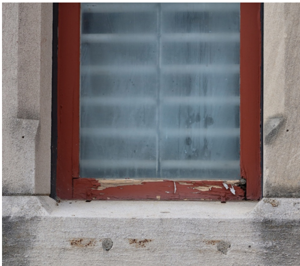
Figure 2.33: Typical deterioration of non-historic replacement windows at cell block.
