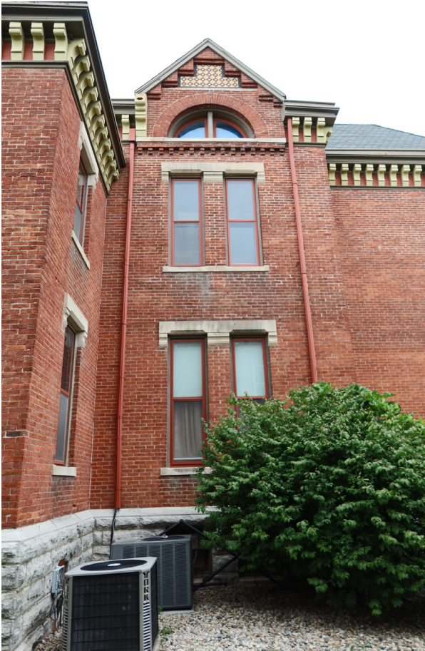
Figure 2.26: The east bracket (right) on the south gable of the residence has been missing for many years.
