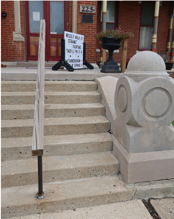
Figure 2.22: Critical: the present wood handrail is not a code-compliant handrail. It is too thick to meet the requirements for safe use. The wood is also cracking.
