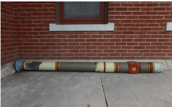
Figure 2.18: This porch post recently fell during a storm.
