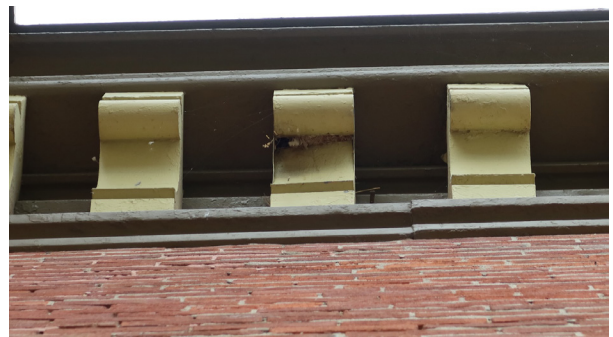
Figure 2.29: Minor damage to one cornice bracket with evidence of birds nesting inside bracket.
