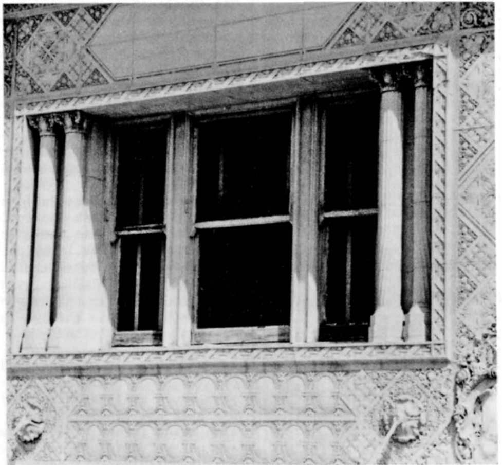
Figure 2. Original second-floor wooden windows of the Colcord Building. Note the high degree of ornamentation with the composition of the triple windows, the deep setbacks, the paired Corinthian columns, and the Sullivanesque terra-cotta panels surrounding the windows. The windows on the upper floors are of a simpler composition being paired one-over-one double-hung windows. (Photo: Jack Graves, AIA)
