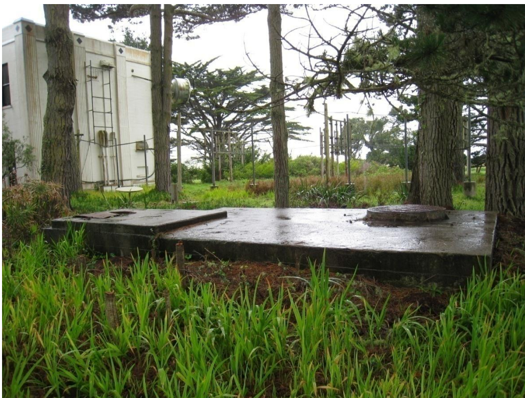
RCA Transformer Vault, looking northwest. (PWRO 2010)
